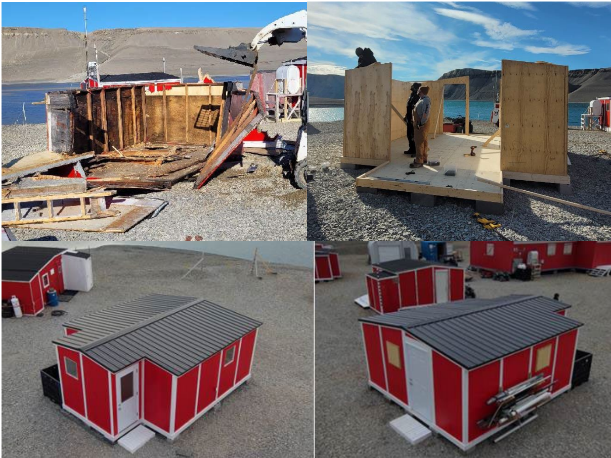
Photo 6 – Top left: Teardown of workshop. Top right: Rebuild of workshop. Bottom: New workshop with steel roofing.
