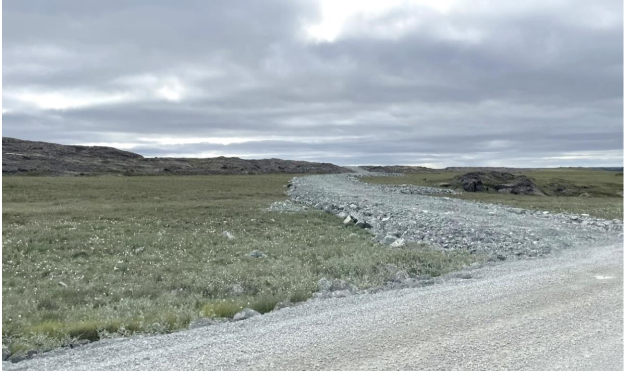
Photo 42: Under-Construction road for Wind Turbine 2- no equipment or materials at the site yet
