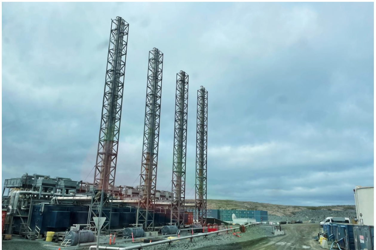
Photo 24: Power Plant – Doris Camp
