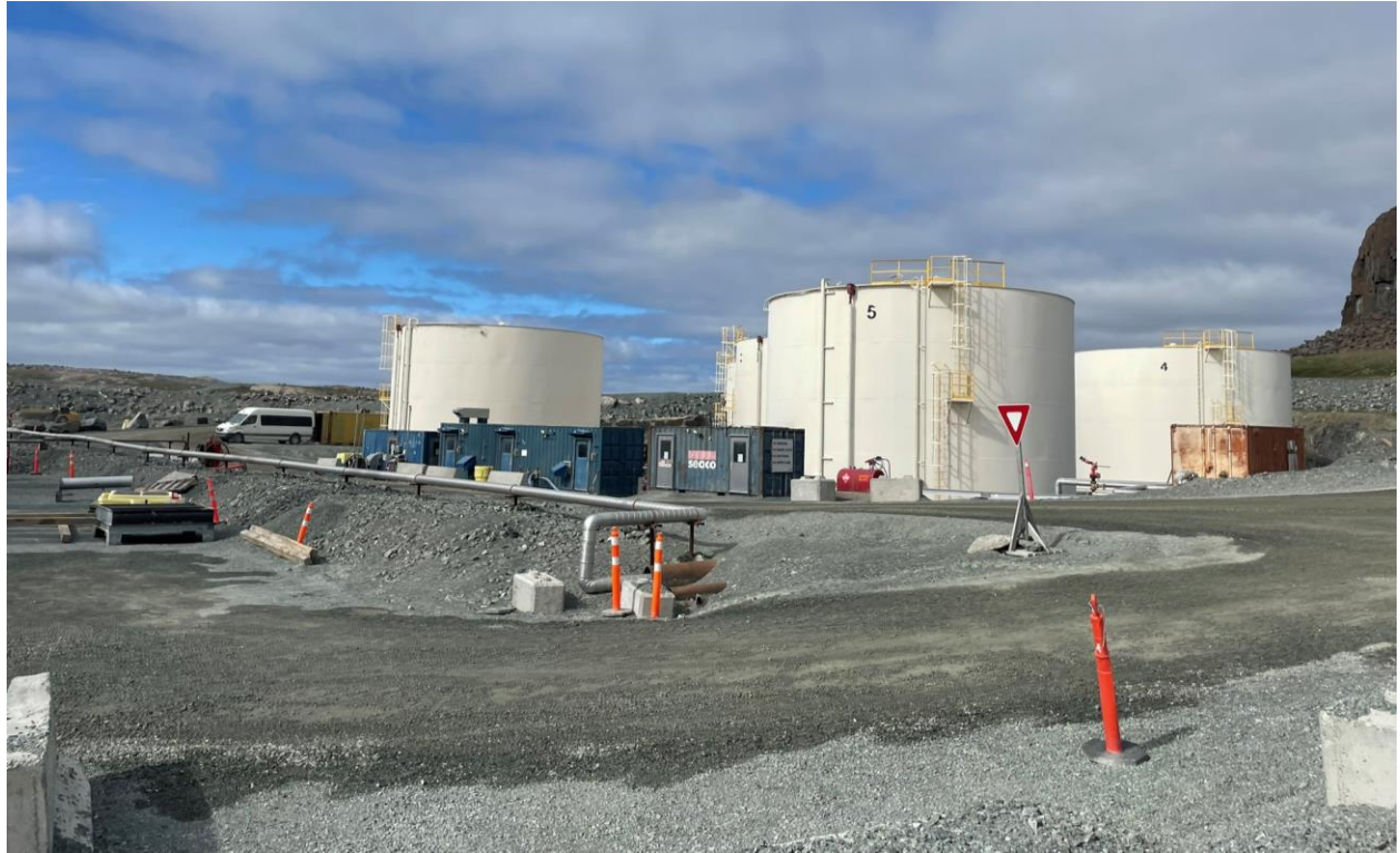
Photo 23: Tankfarm and Fuel Modules - Doris Camp
