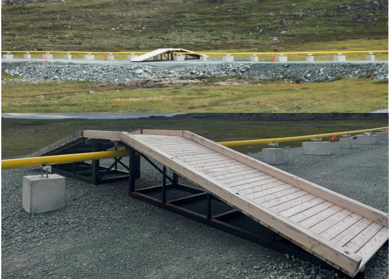
Photo 7: Snowmobile Crossing Ramp with unsafe drop - requires design modification 1
