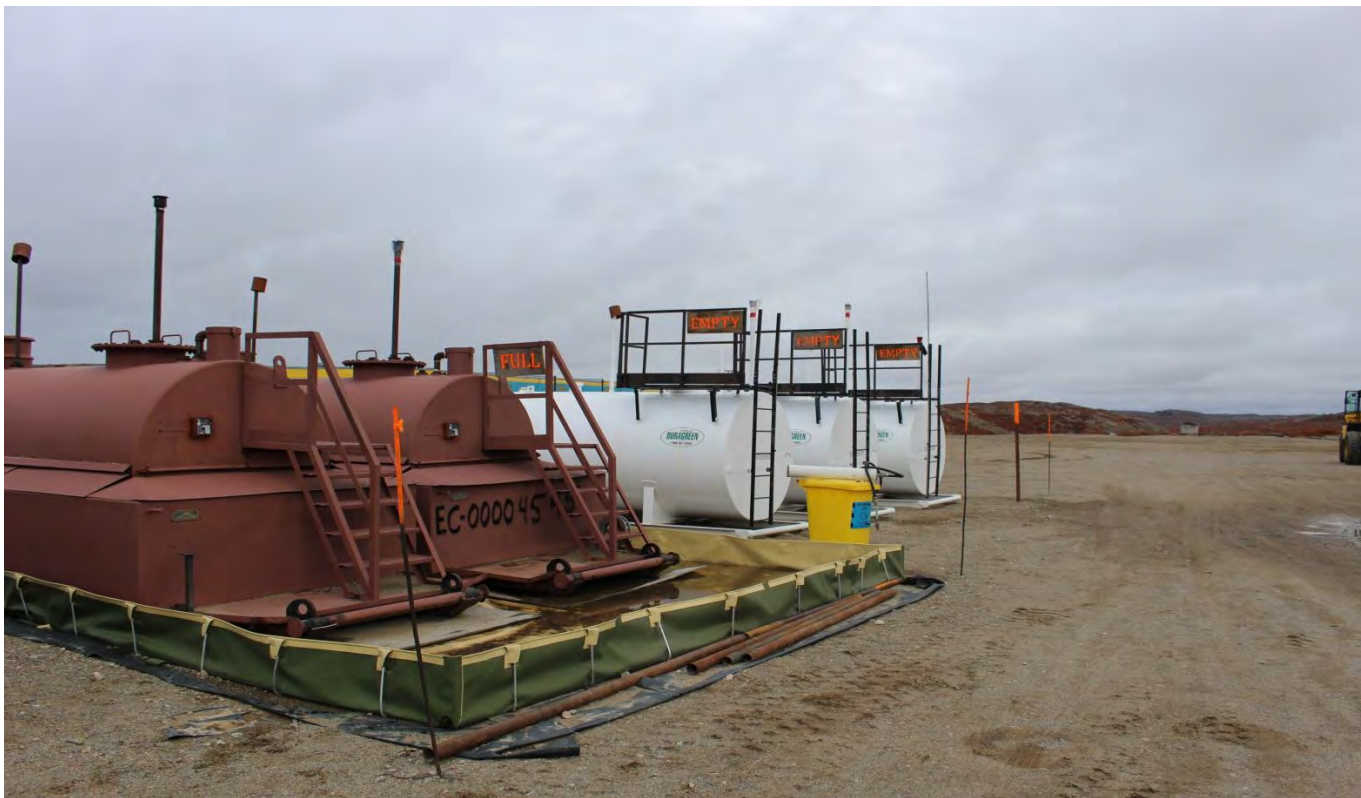
Bulk fuel tanks
