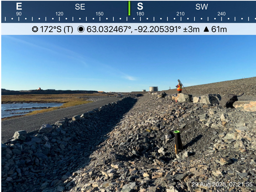
D-CP1 - Photo 13: Dike D-CP1: Downstream rockfill cover and collection ditch. Facing south.
