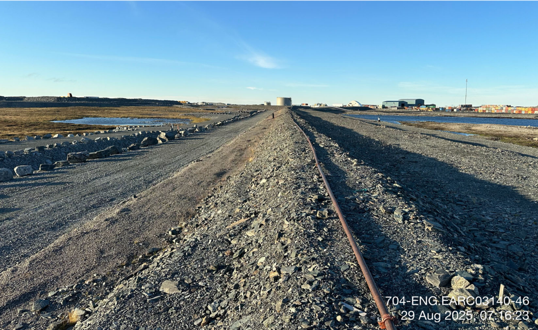
D-CP1 - Photo 4: Dike D-CP1: Dike crest view - downstream on left, upstream on right. Facing south.
