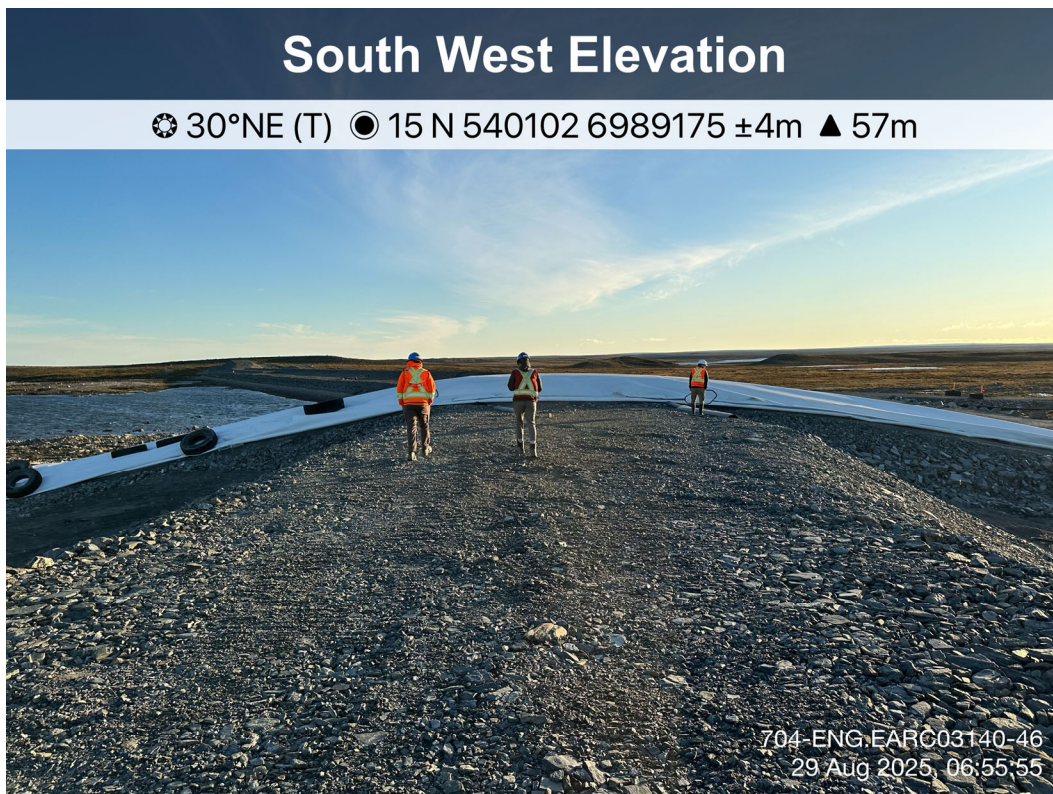
D-CP1 - Photo 14: Dike D-CP1: Pipelines crossing at Station 1+250 of Dike D-CP1. Facing northeast.
