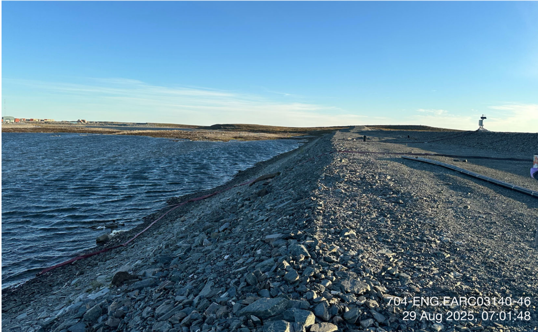
D-CP1 - Photo 3: CP1: Upstream view of CP1- water level well managed. Facing north.
