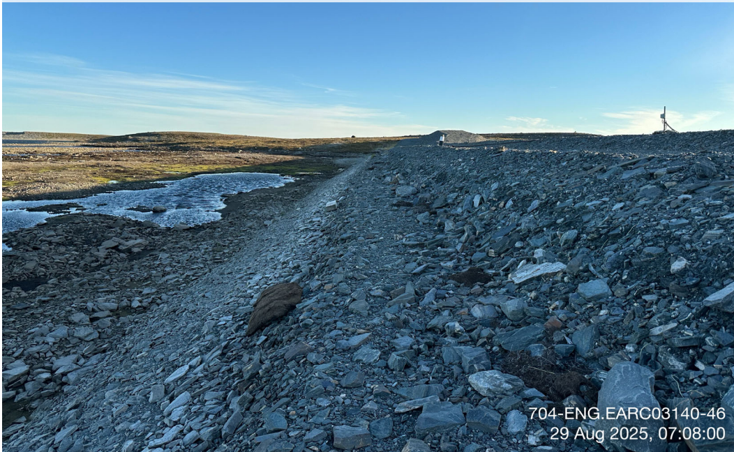
D-CP1 - Photo 2: Dike D-CP1: Upstream face – some wave erosion evident from 2019/2020 high water level event, no change from previous years. Facing north.
