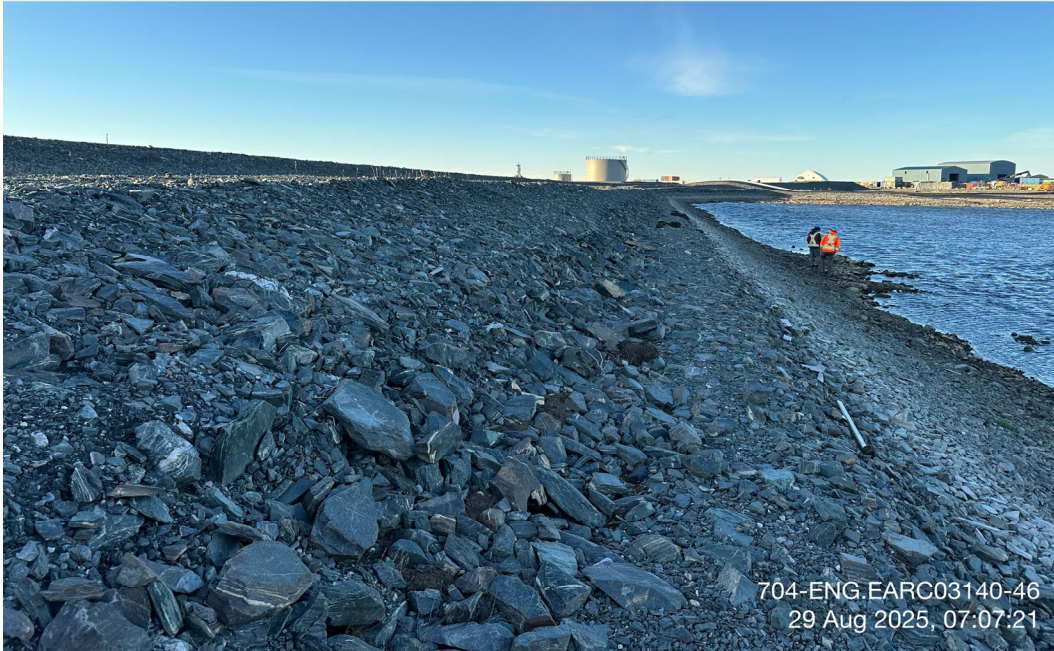
D-CP1 - Photo 1: Dike D-CP1: Upstream face – some wave erosion evident from 2019/2020 high water level event, no change from previous years. Facing south.
