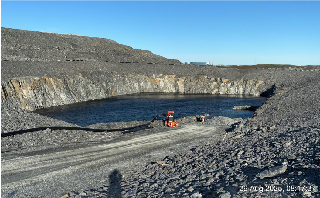
CP2 - Photo 1: CP2: Pumping system, bedrock slopes with fractured rock, no stability concern. Facing west.
