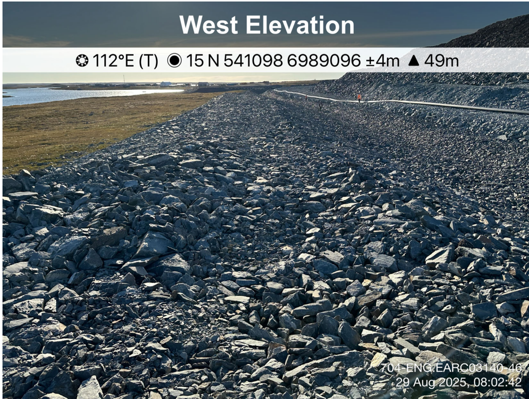
Channel9 Berm - Photo 9: Channel9 Berm: West end of Channel9 Berm, minor settlement and cracking. Facing east.
