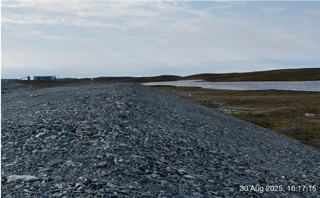
CP2 Thermal Berm - Photo 5: CP2 Thermal Berm: Overview of downstream side slope, minor deformation observed at east end, no stability concern. Facing northwest.
