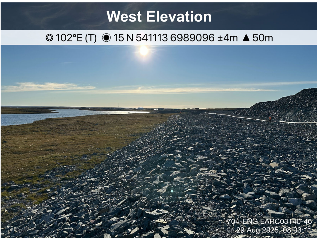
Channel9 Berm - Photo 10: Channel9 Berm: Overview of crest and downstream slope, performing well, no stability concern. Facing east.
