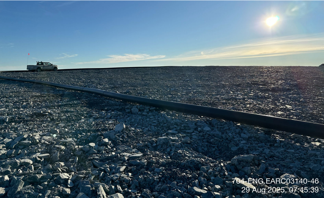
CP6 - Photo 6: CP6: Overview of cover placement at the east side perimeter. Facing east.
