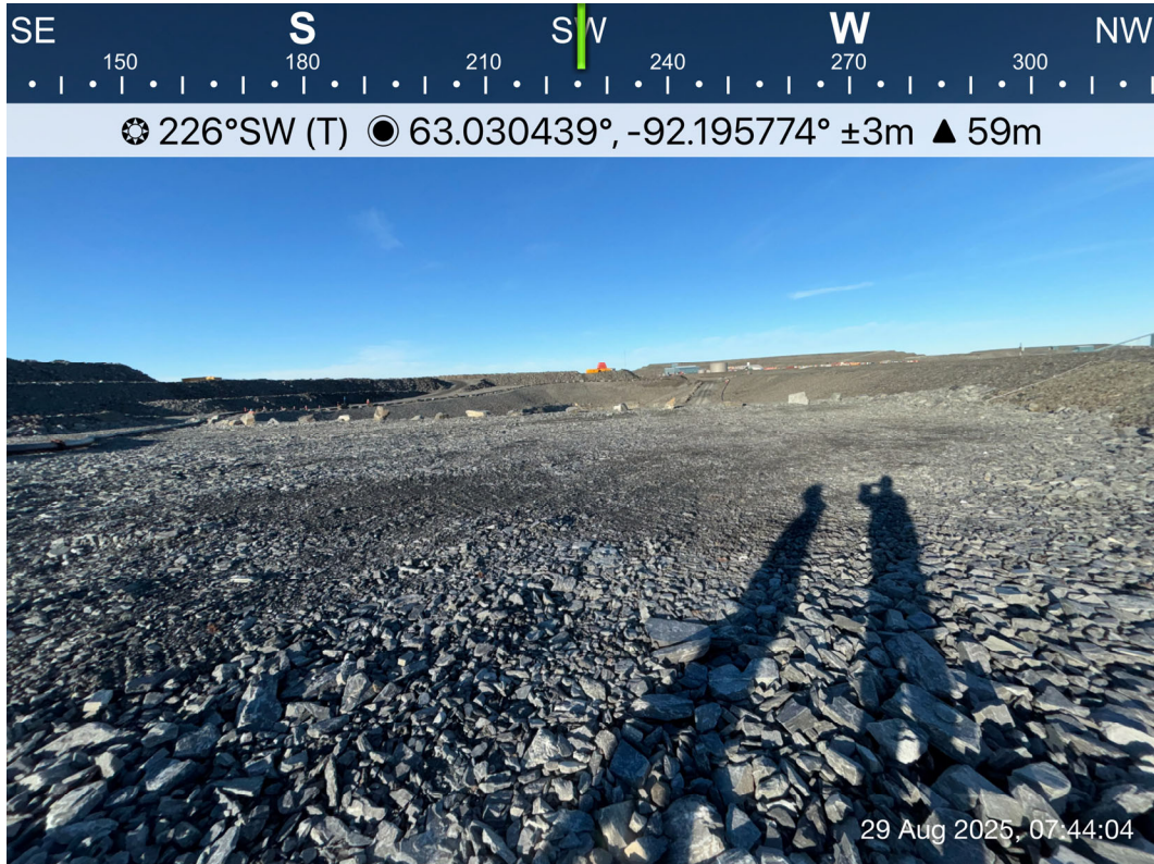
CP6 - Photo 7: CP6: Overview of cover placed at the east perimeter of CP6 and against the CP6 Thermal Berm upstream slope. Facing southwest.
