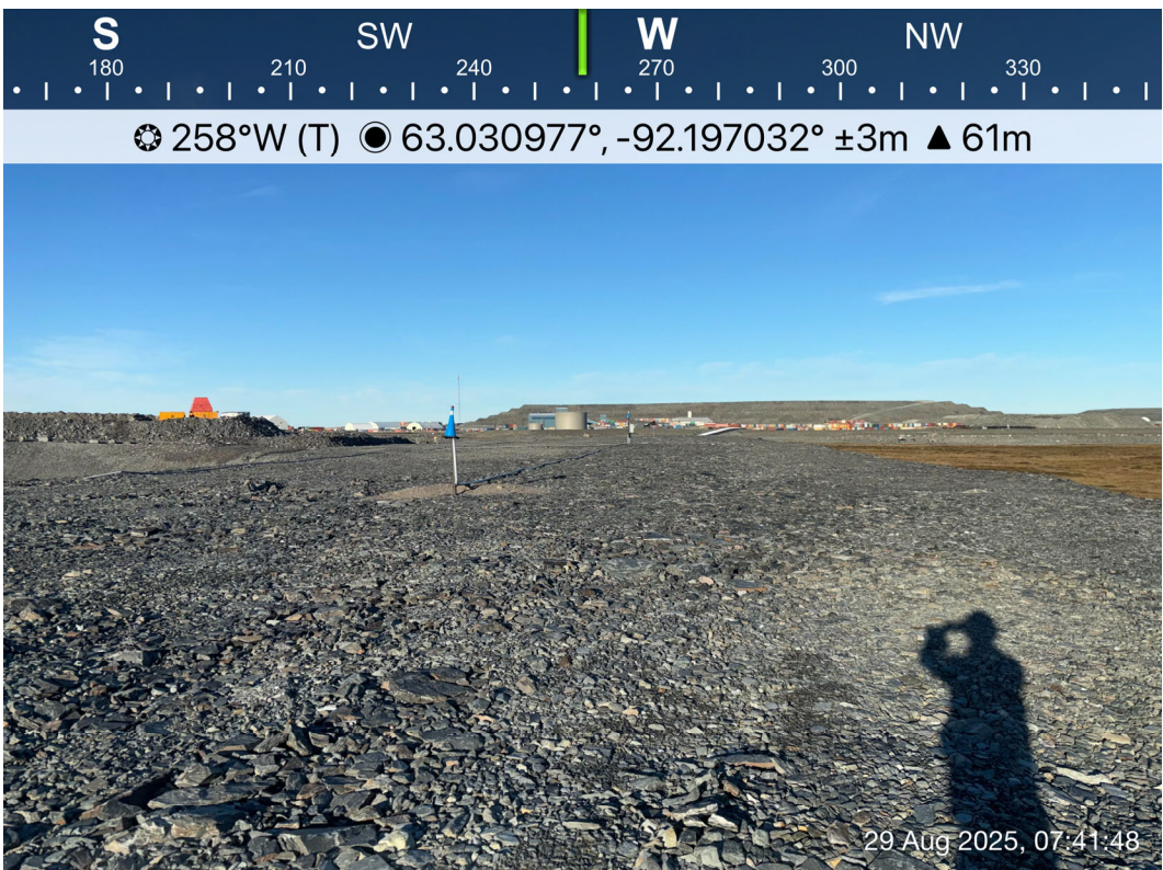
CP6 Thermal Berm - Photo 8: CP6 Thermal Berm: Overview of thermal berm Crest, thaw settlement observed at various areas. Facing west.
