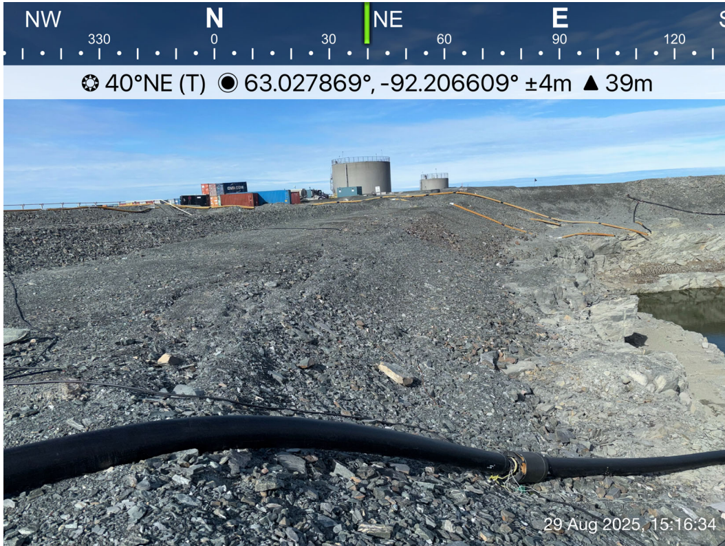
SP1 - Photo 5: SP1 Saline Pond: Overview of southwestern side of SP1, deformation and cracking observed on top of the overburden protected slope. Facing north-east.
