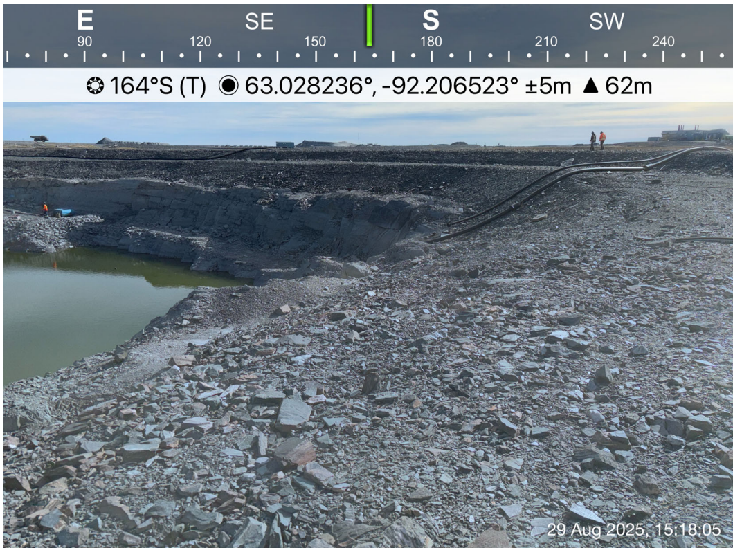
SP1 - Photo 4: SP1 Saline Pond: Overview of southwestern side of SP1, deformation and cracking observed on top of the overburden protected slope. Facing south.
