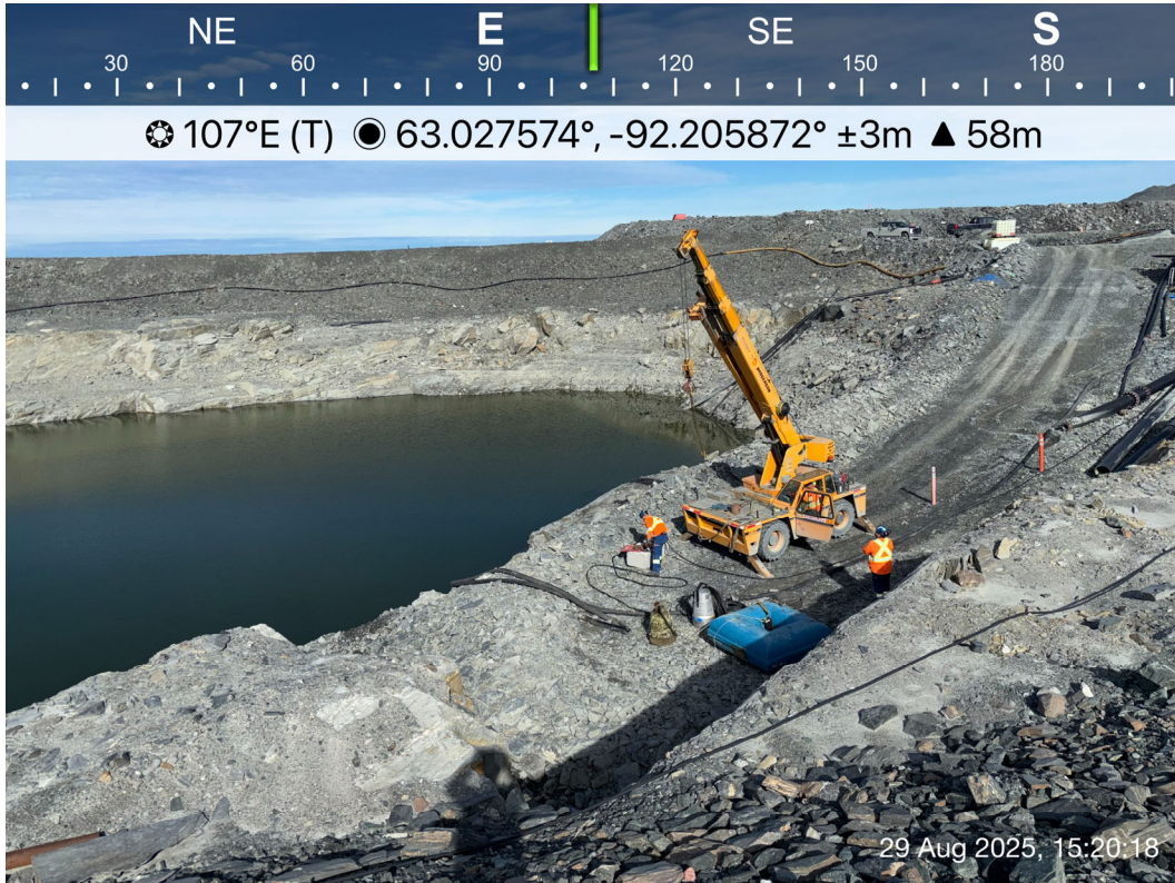
SP1 - Photo 3: SP1 Saline Pond: Overview of access ramp, pipelines, and safety berms. Facing east.
