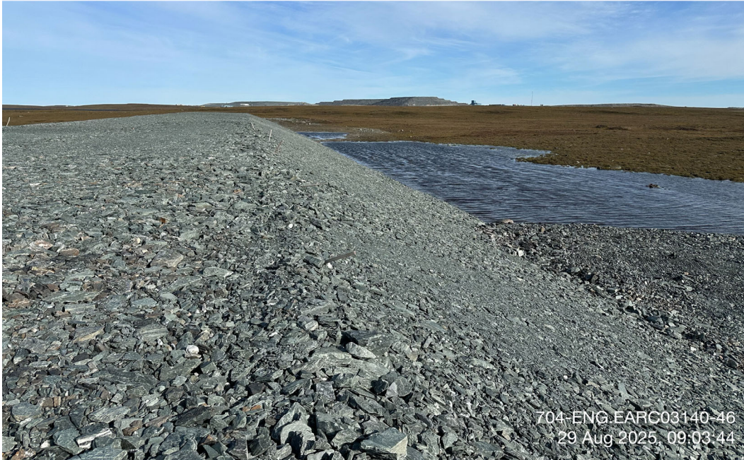
CP9 Thermal Berm - Photo 5: CP9 Thermal Berm: Upstream side slope of CP9 Thermal Berm, ponding water observed at the toe of the berm. Facing north.
