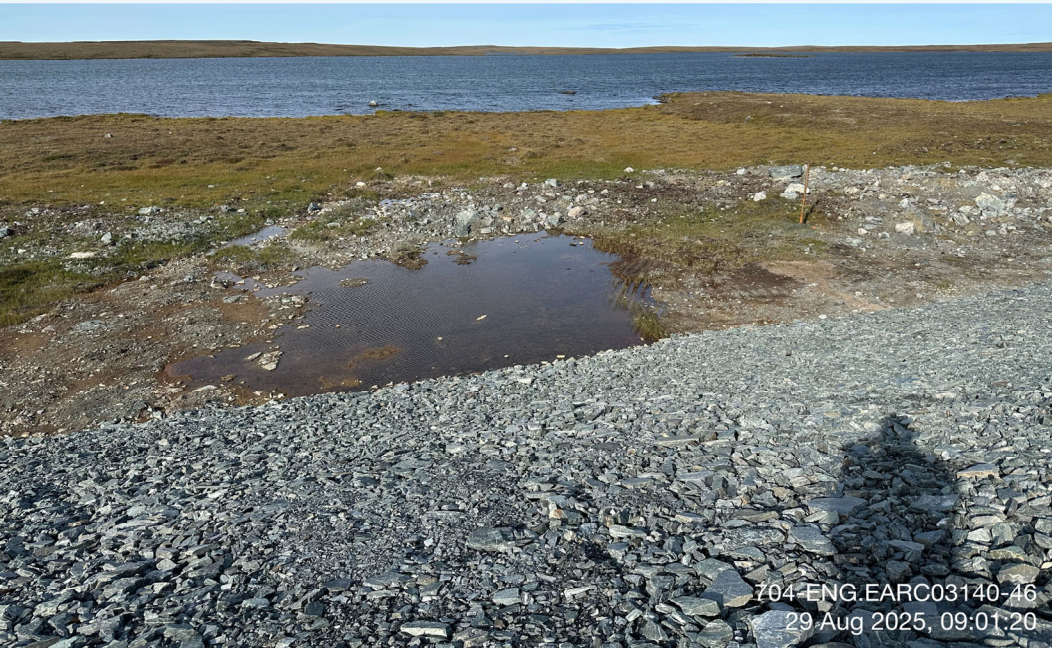
CP9 Thermal Berm - Photo 6: CP9 Thermal Berm: Area of ponding water at the downstream toe of CP9 Thermal Berm. Facing west.
