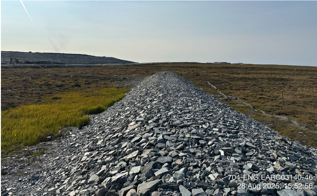
Channel2 Berm - Photo 19: Channel2 Berm: Overview of the Channel2 Berm. Facing northwest.
