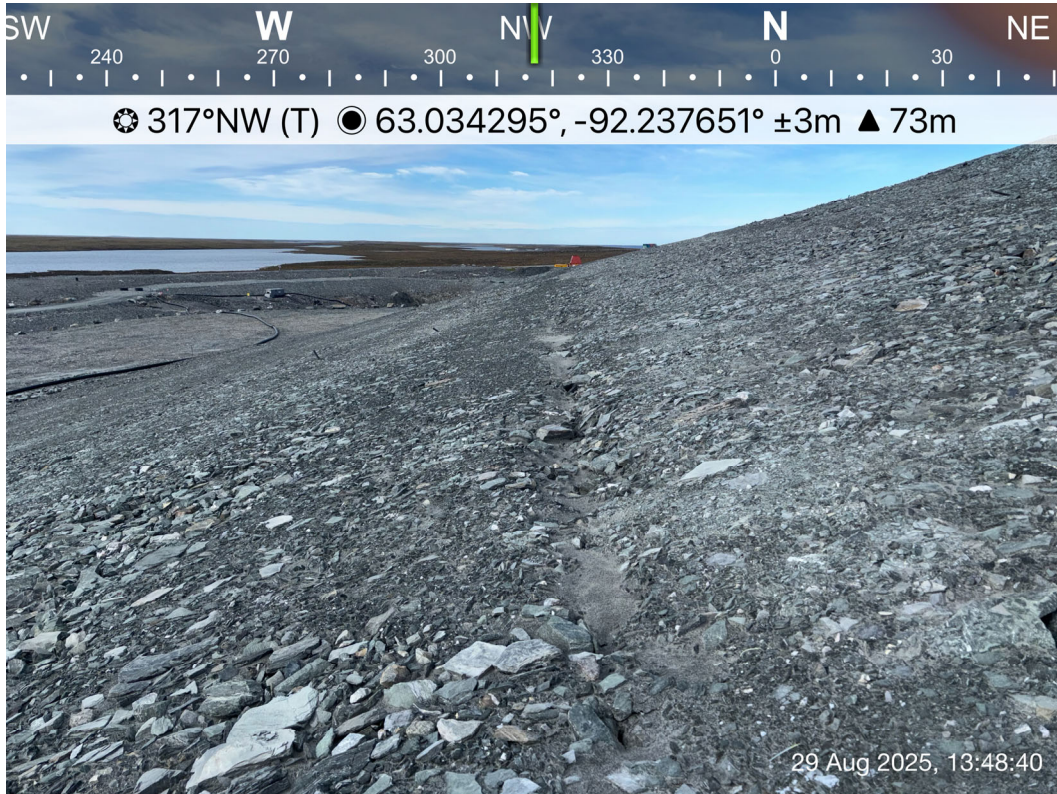
TSF - Photo 3: TSF: Overview of south slope of TSF Cell 1. Facing northwest.
