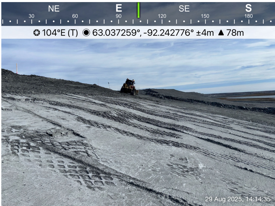
TSF - Photo 6: TSF: Rockfill cover and west slope of TSF Cell 2, active placement of tailings. Facing east.
