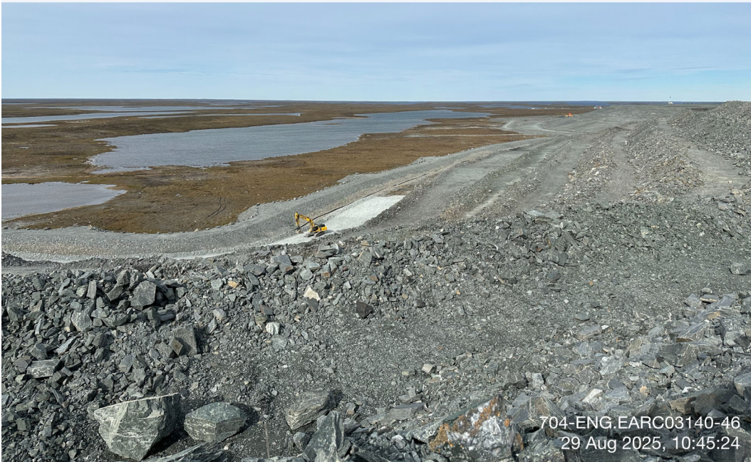
WRSF1 - Photo 2: WRSF1: Overview of west side benches and slopes, Channels 3 and 4 in the background. Facing northwest.
