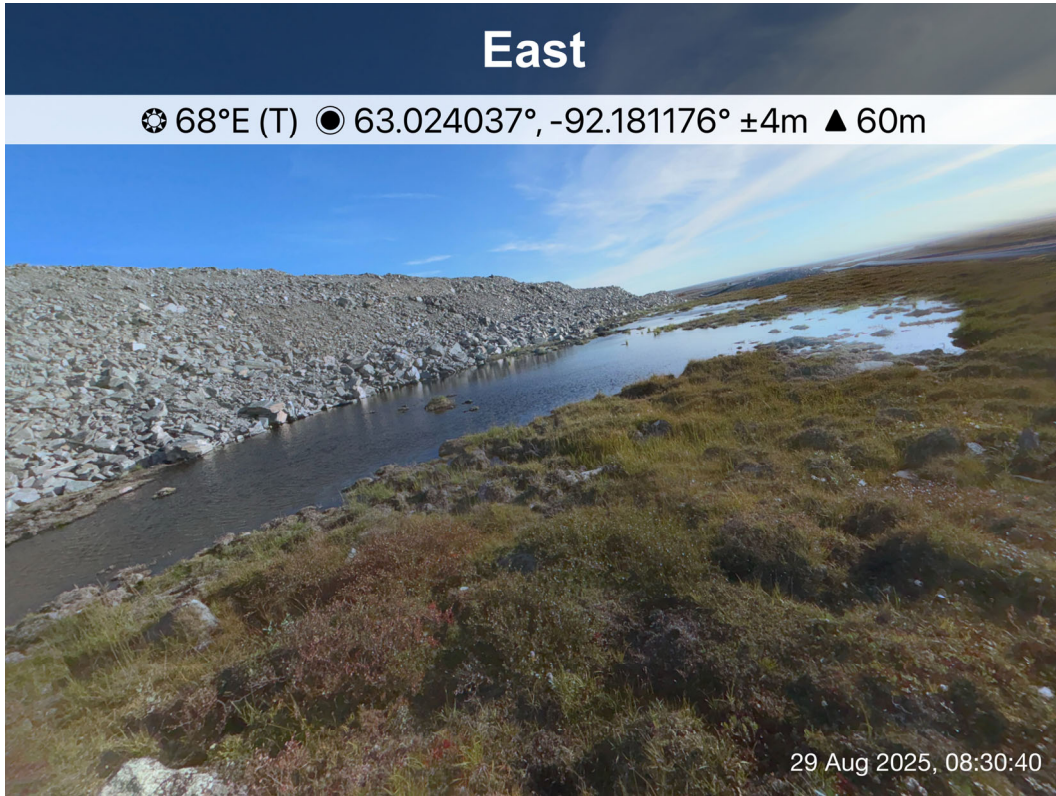
WRSF3 - Photo 5: WRSF3: Overview of ponded water observed at southwest corner of WRSF3. Facing east.
