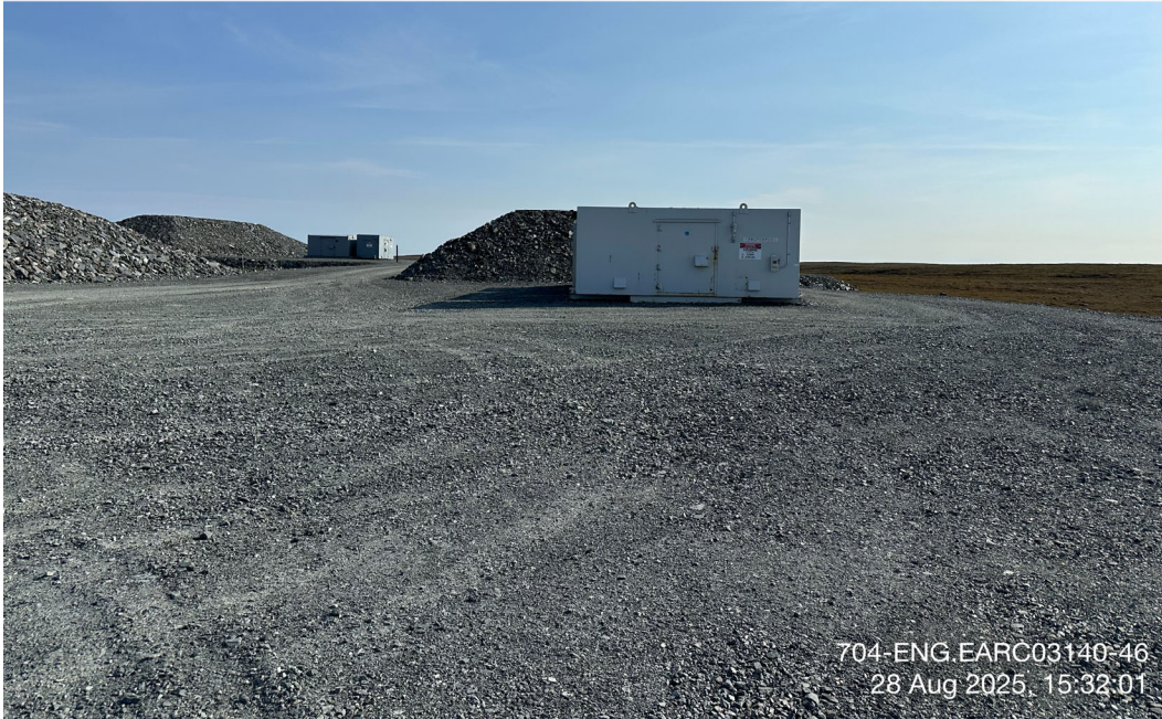
Emulsion Plant Pad - Photo 11: Emulsion Storage Pad: Overview of pad and storage. Facing southeast.
