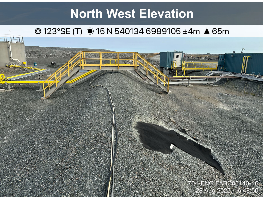
Mine Site Fuel Tank Farm - Photo 34:
