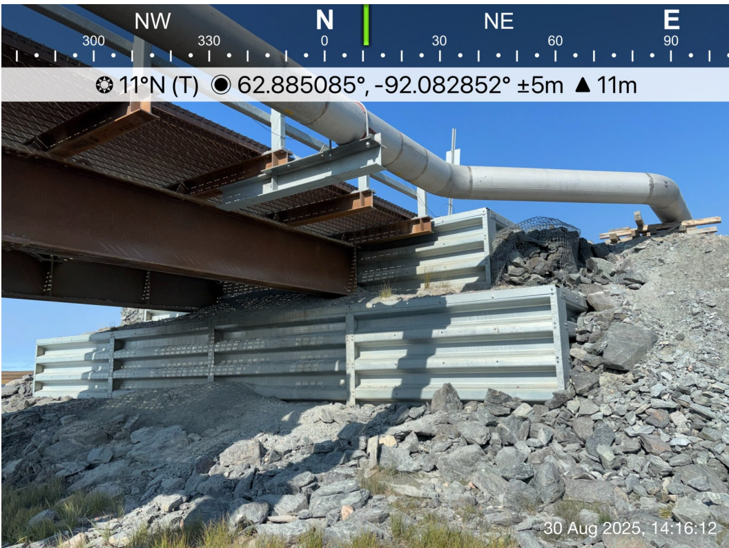
AWAR Road/ Culvert - Photo 34: M-5 Bridge KM 10.5: North abutment, damaged gabion basket.
