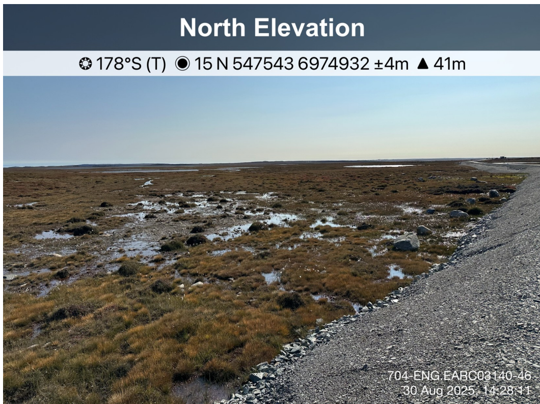
AWAR Road/ Culvert - Photo 38: KM 12.6: No culvert installed, poor drainage condition, no sign of water flow.
