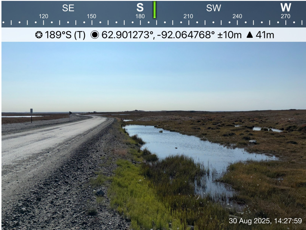
AWAR Road/ Culvert - Photo 37: KM 12.6 :No culvert installed, poor drainage condition, no sign of water flow.
