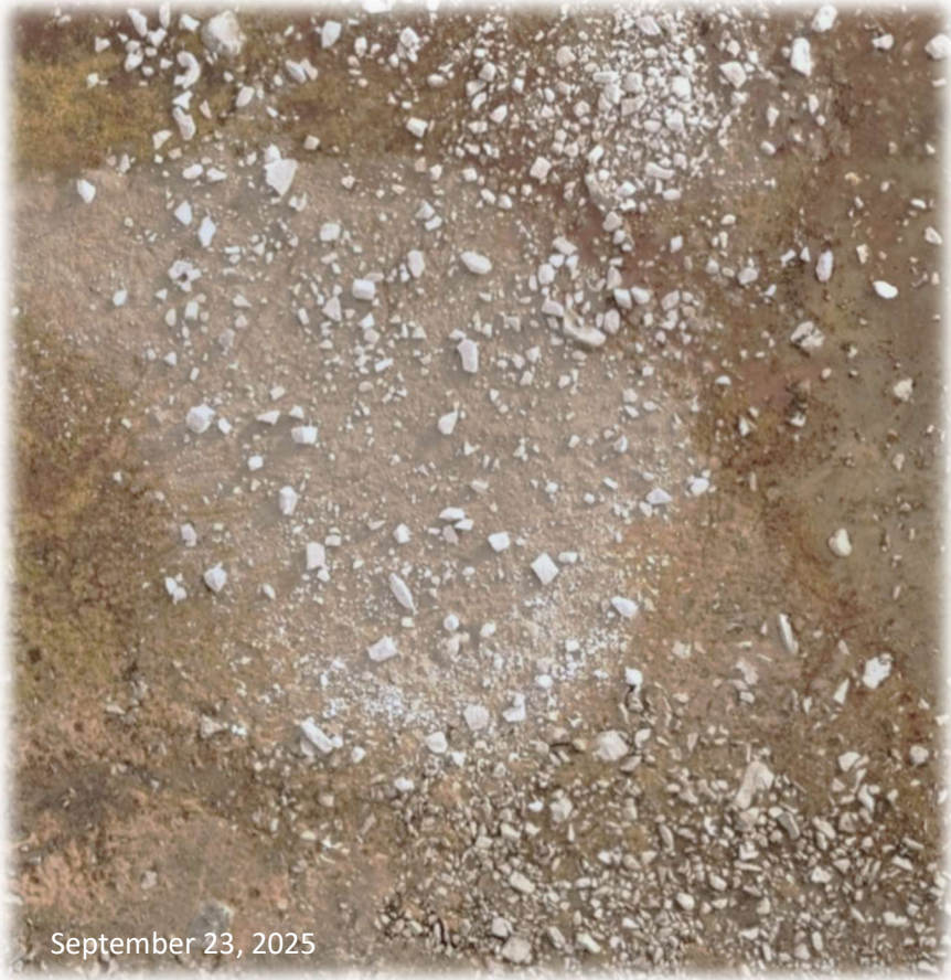
Silt Fences Installed Between the Wetland and the Quarry North End were removed
