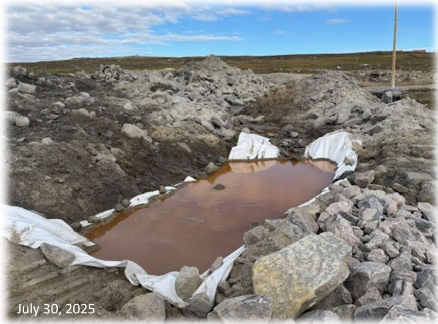
New sediment decantation pond installed at the Dredge Spoil Dewatering Area in 2025
