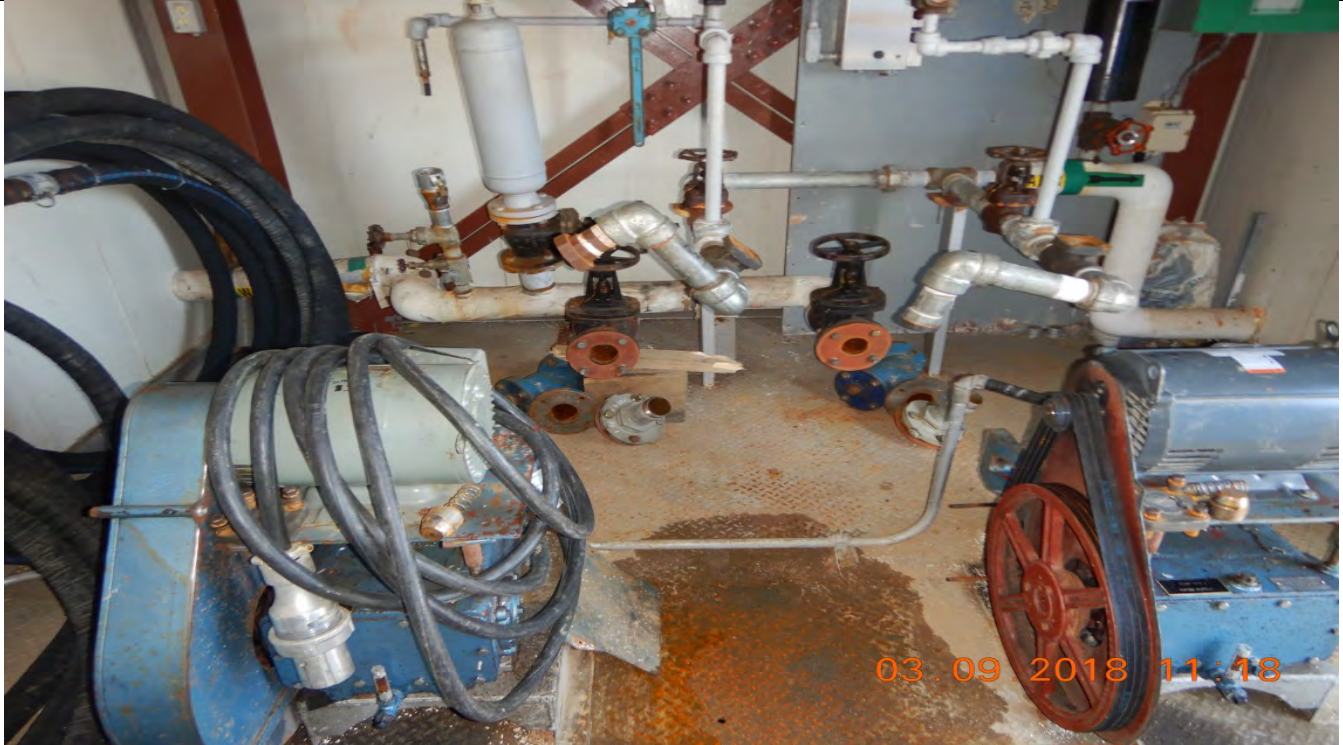
Description: Two water pumps in pump house at potable Fresh Water Lake
