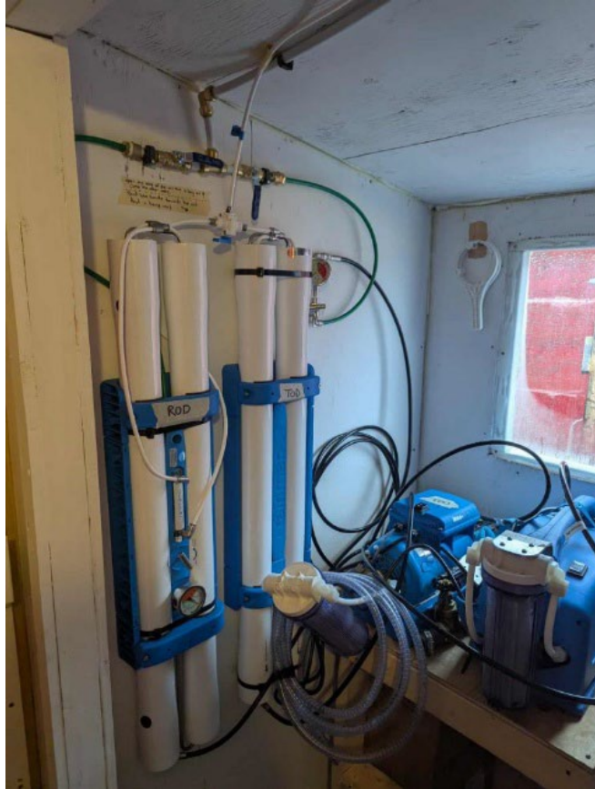
Photo 3 – Reverse-osmosis unit; saltwater pump and tank not pictured.
