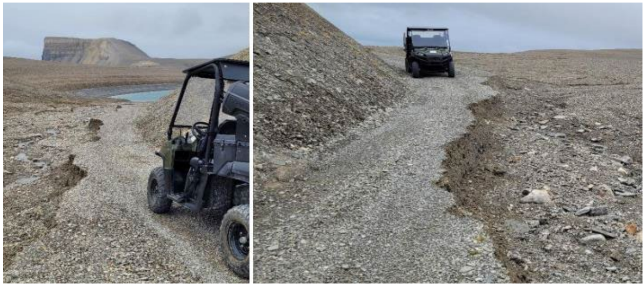
Photo 10 – Erosion of the perimeter road to the beach (2024 photo).
