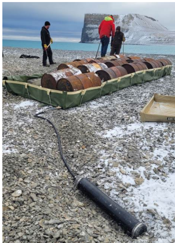
Photo 12 – Construction of temporary fuel cache containment area for non-DRDC-owned drums by DRDC.
