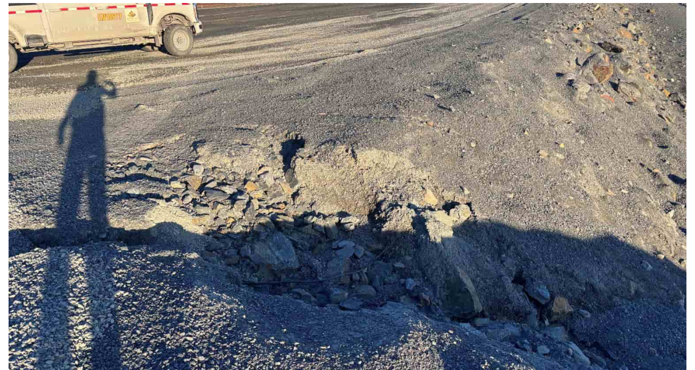
G-82: Erosion pathway at NW end of airstrip
