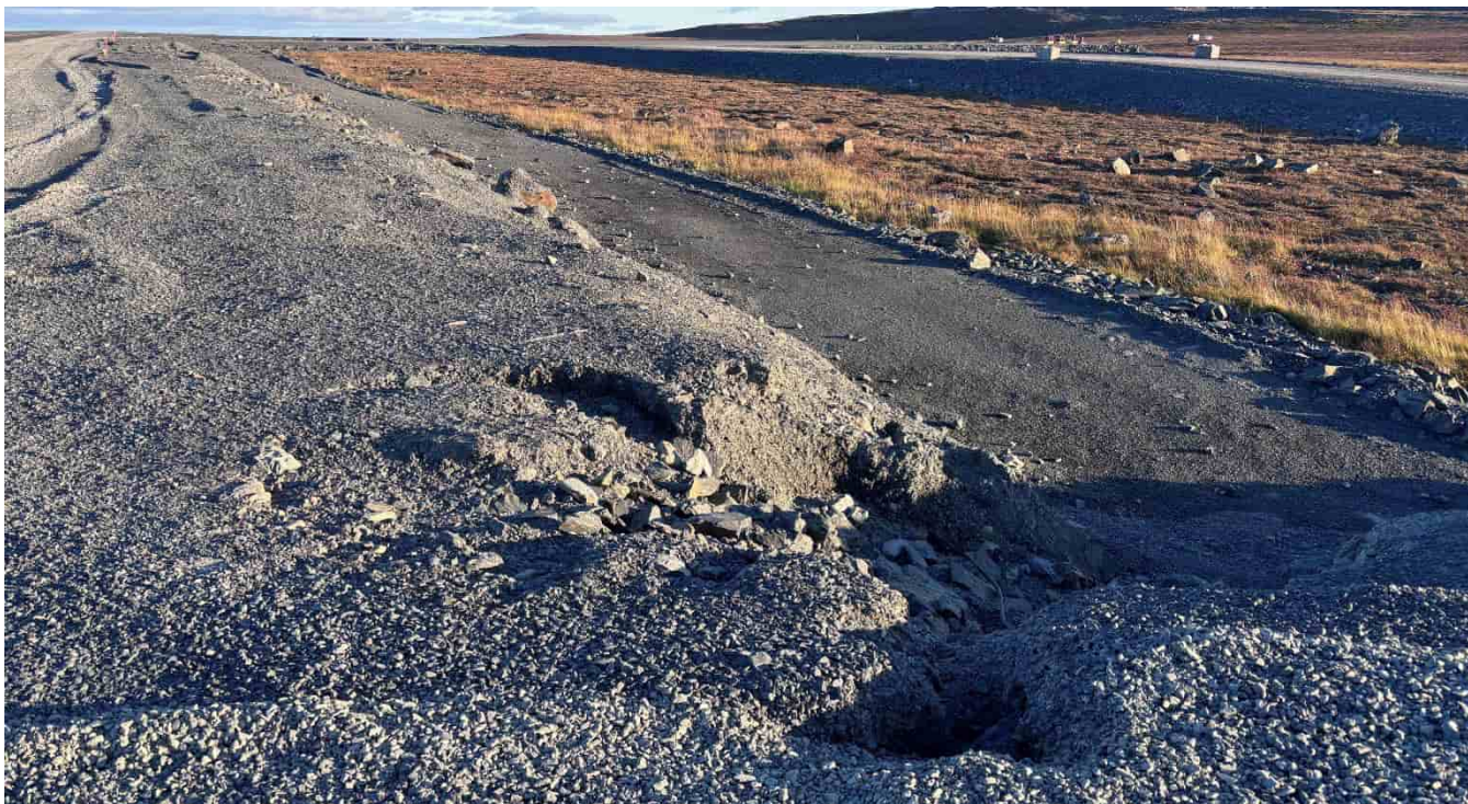
G-81: Erosion pathway at NW end of airstrip
