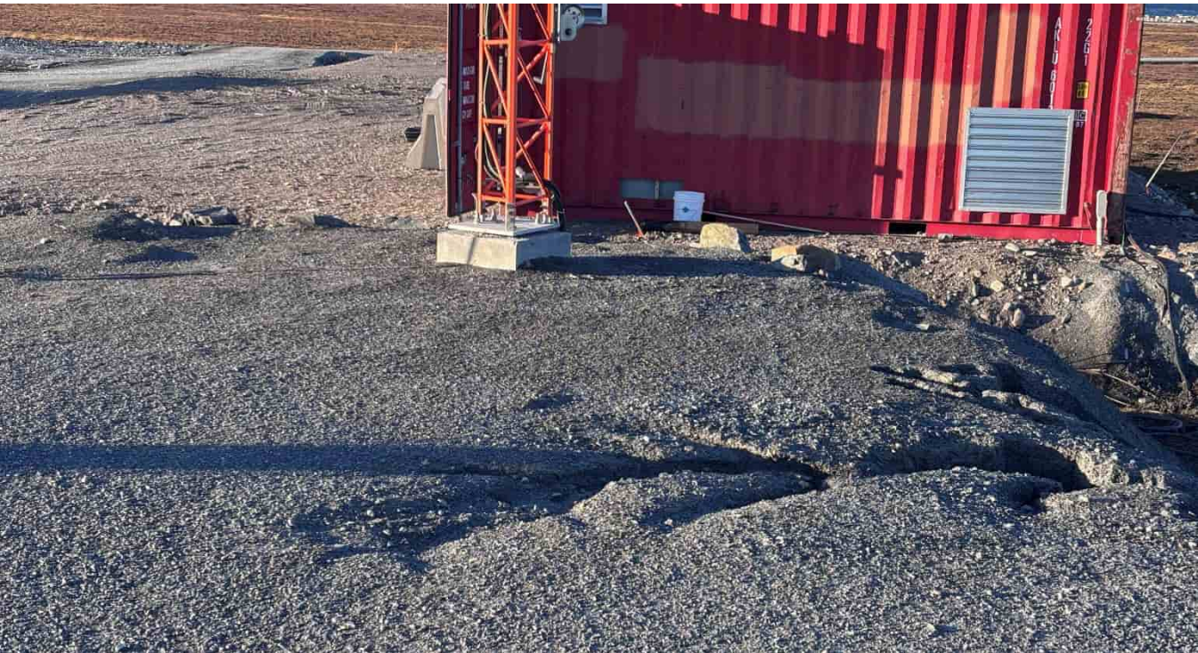
G-70: Erosion NE apron, facing N
