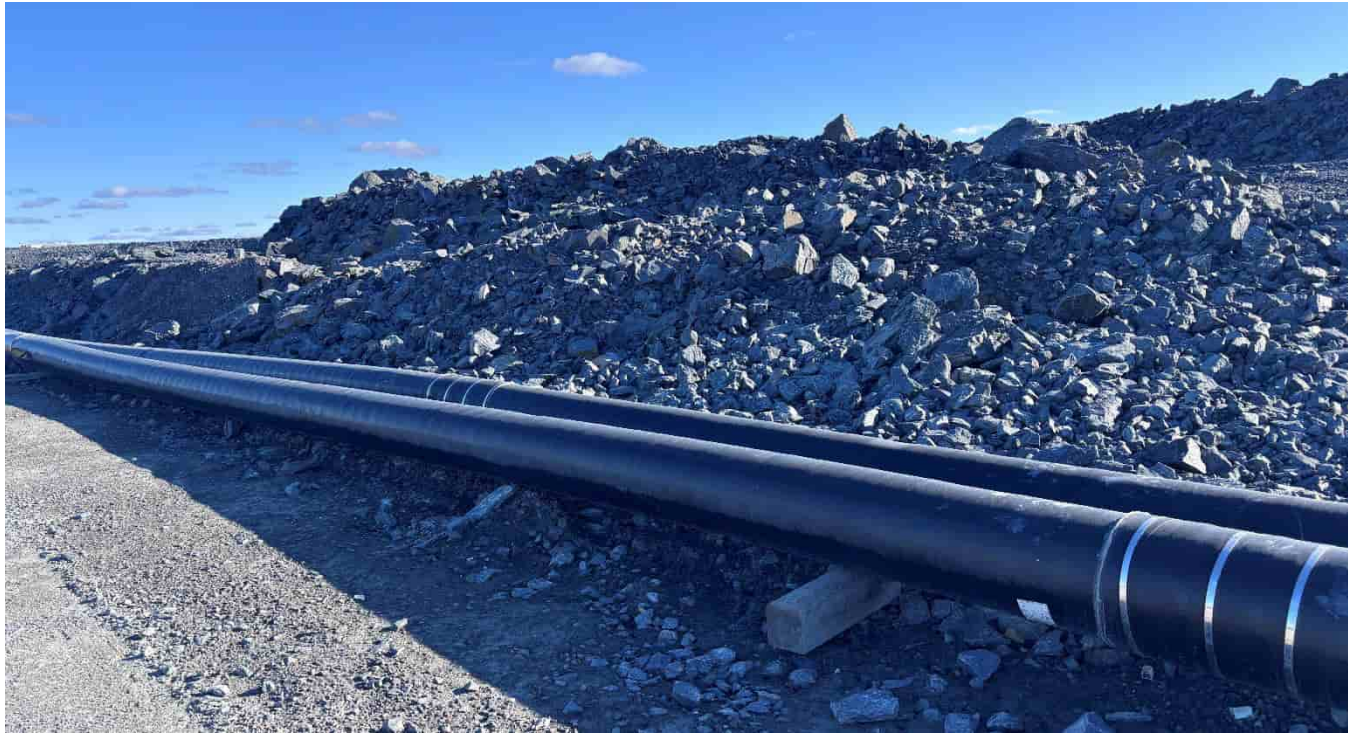
G-164: tailings pipeline along road beside water treatment plant
