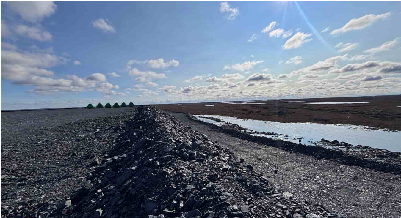
G-136: Top of berm, looking SE – Ponding water beside waste rock area
