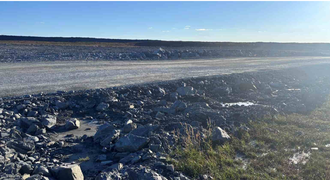
G-99: N side of All-Weather Road – lower road thickness in area
