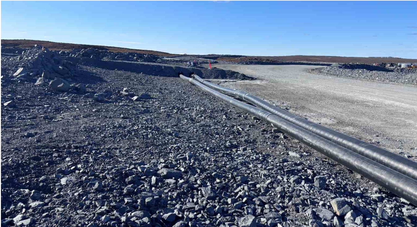
G-165: tailings pipeline along road beside water treatment plant, looking SE
