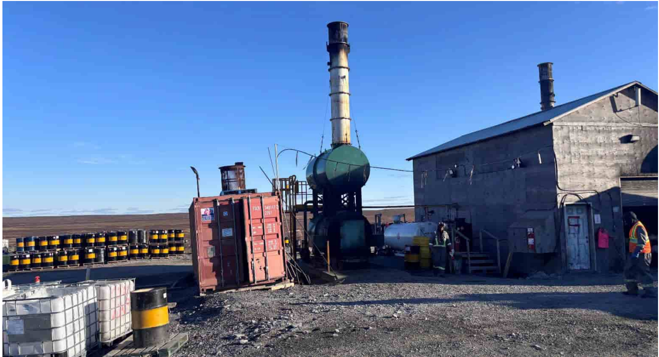
G-9: Temporary fuel storage facility and incinerator, looking S
