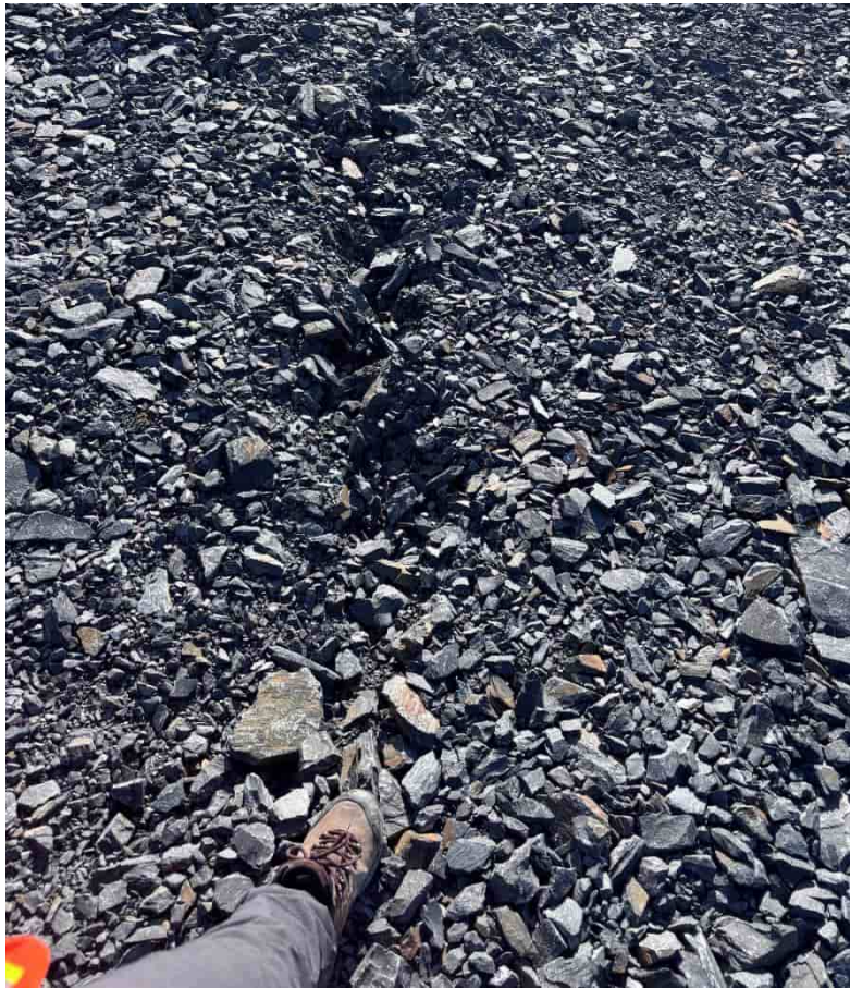
G-140: Tension / settlement crack in diversion
