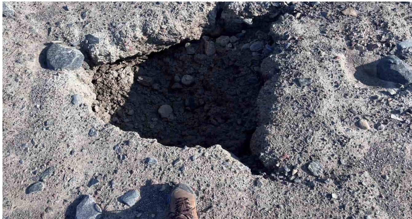
G-132: Example of sinkhole in the eastern side of the stockpile
