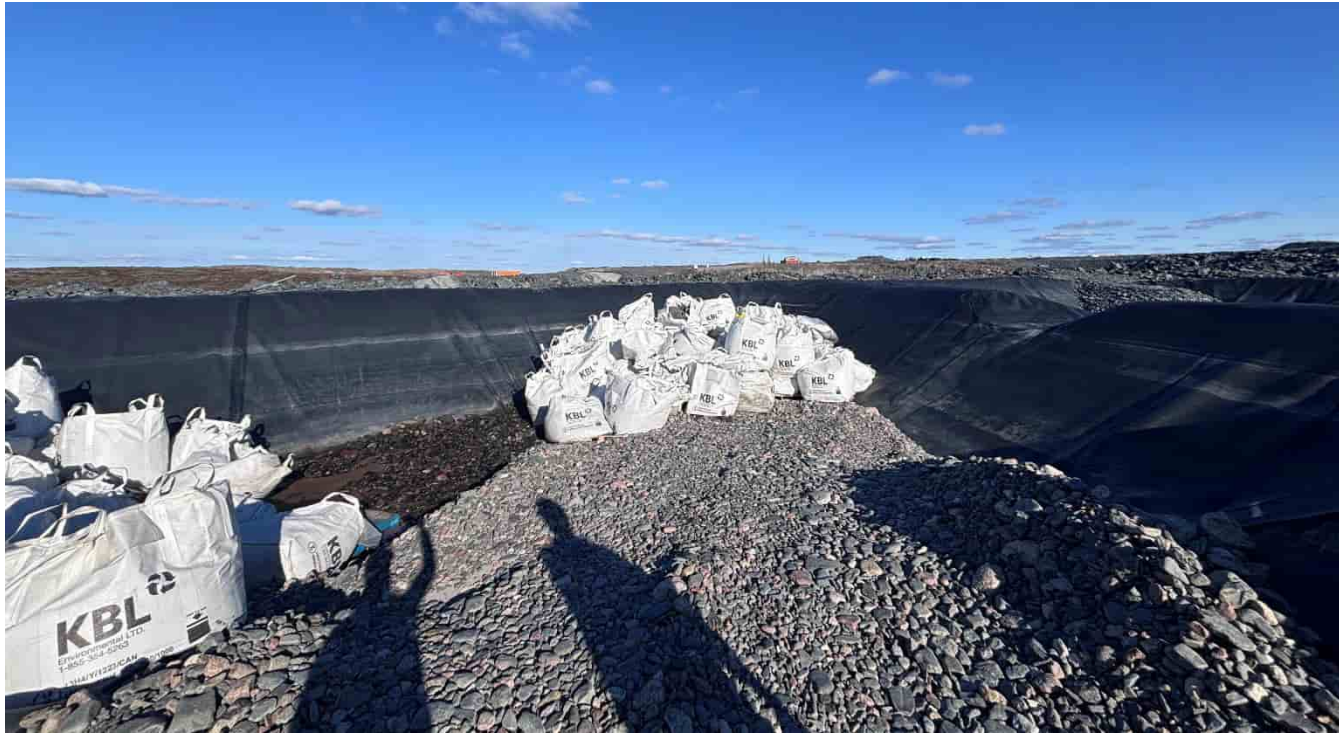
G-160: Northernmost treatment pond with rock over liner
