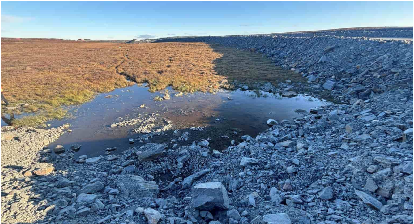
G-94: Ponding on SE corner of junction between the All-Weather Road and Echo Pit Haul Road
