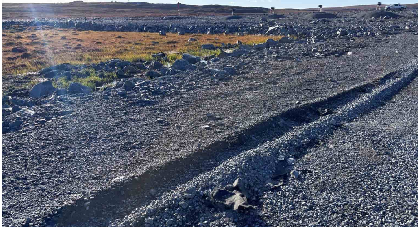
G-55: View towards airstrip lighting apron, looking W – Exposed geotextile visible
