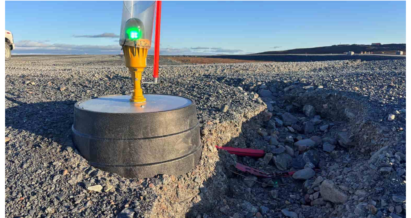
G-80: : Erosion at NW end of runway – exposed cables
