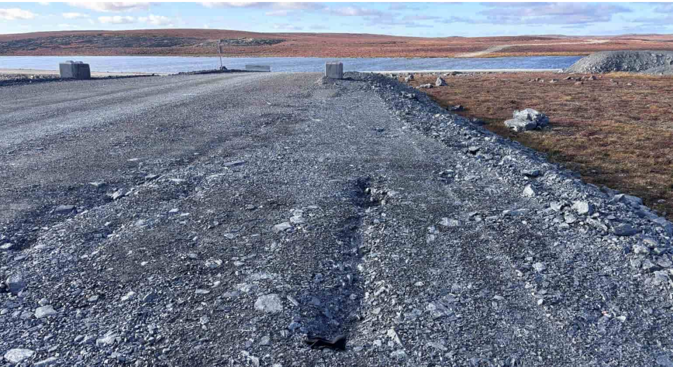
G-46: Airstrip runway access road settlement, looking NW
