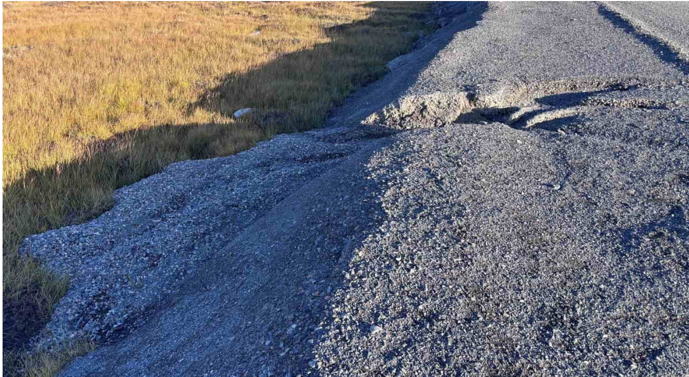
G-63: Erosion pathway on NE side of airstrip – Looking SE
