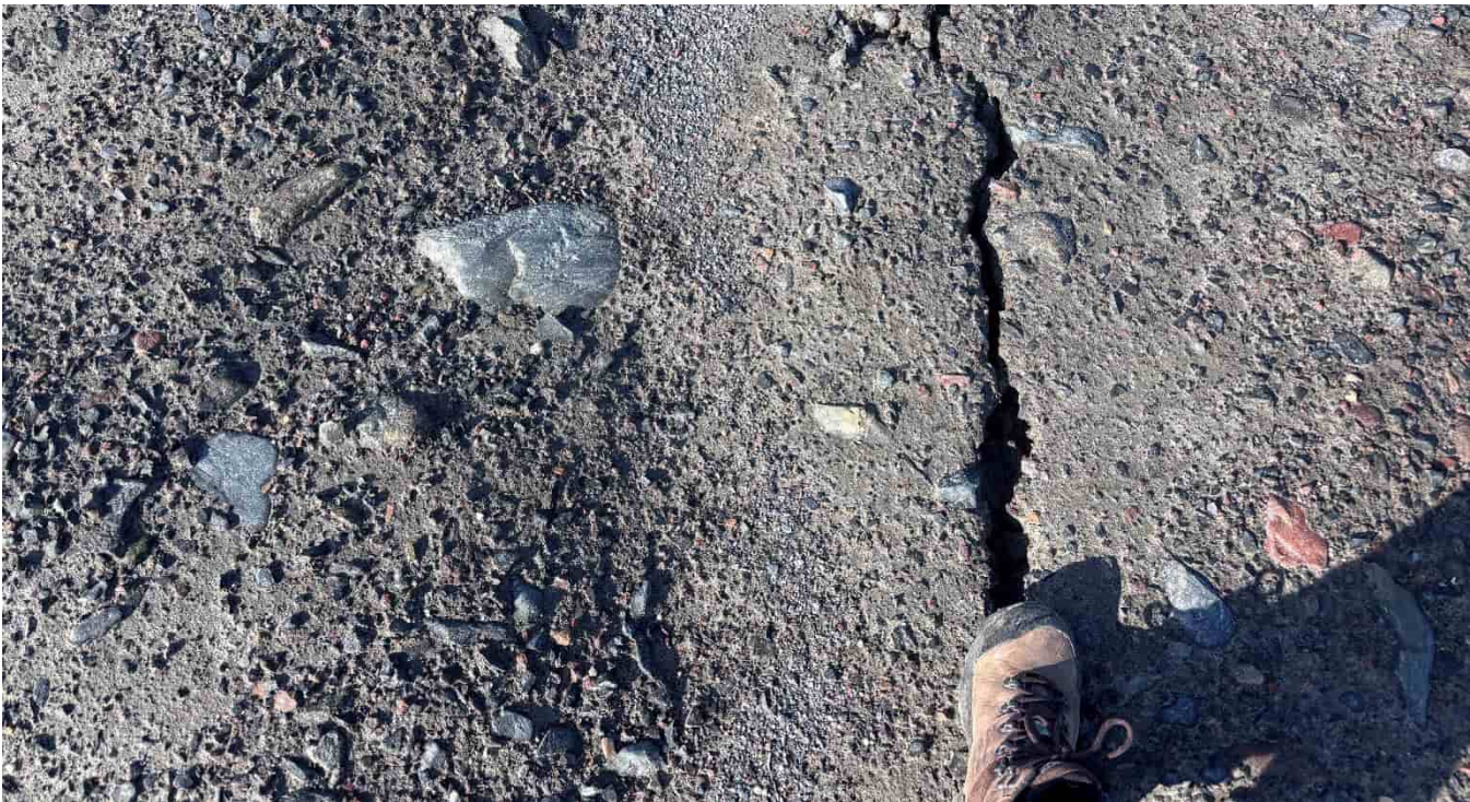
G-129: Tension cracks in overburden stockpile pad (from settlement and melt – no large scale stability concerns)
