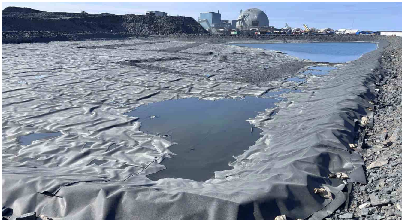
G-231: Looking E along northern edge of pond – minimal tie-in / anchoring
