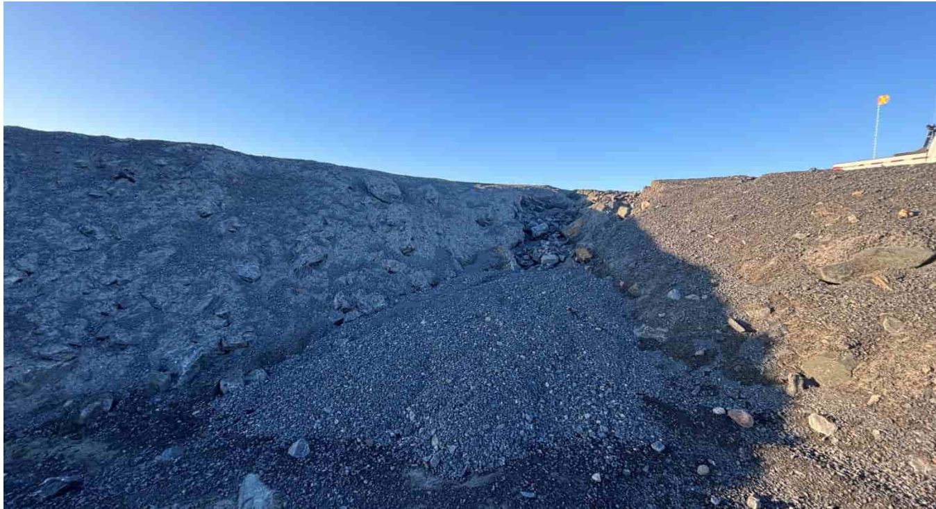
G-83: Erosion at NW end of airstrip
