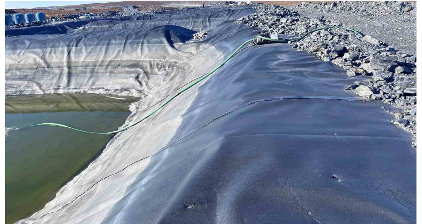
G-153: Treatment pond oversteepened slope and liner damage
