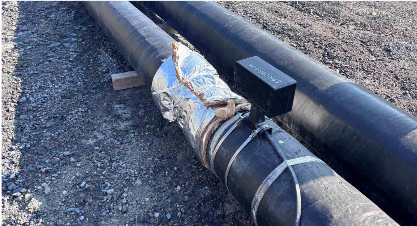
G-119: Typical tailings pipeline connection
