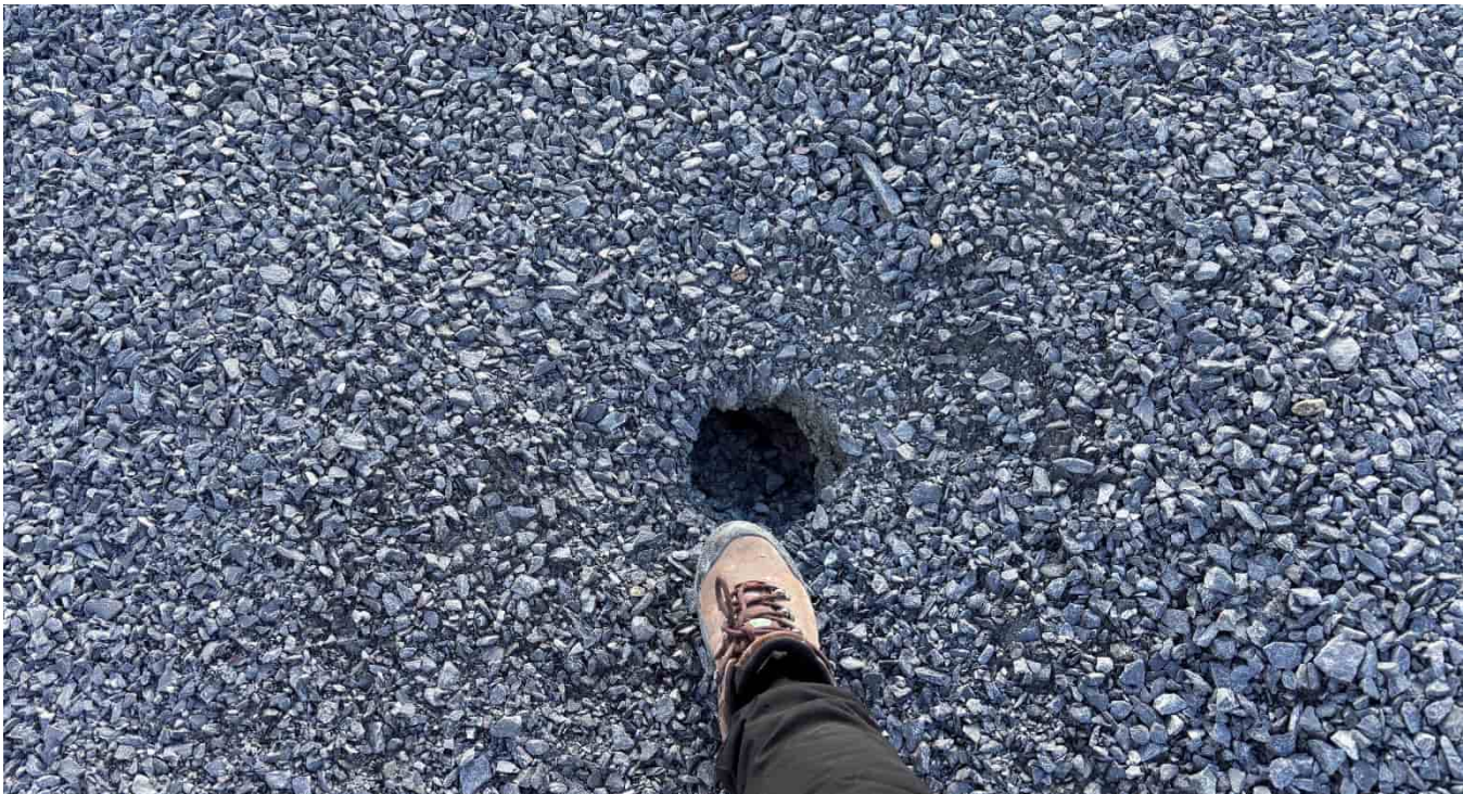
G-42: Smaller sinkhole in SW apron (expected from crush material migration in to voids of larger material)
