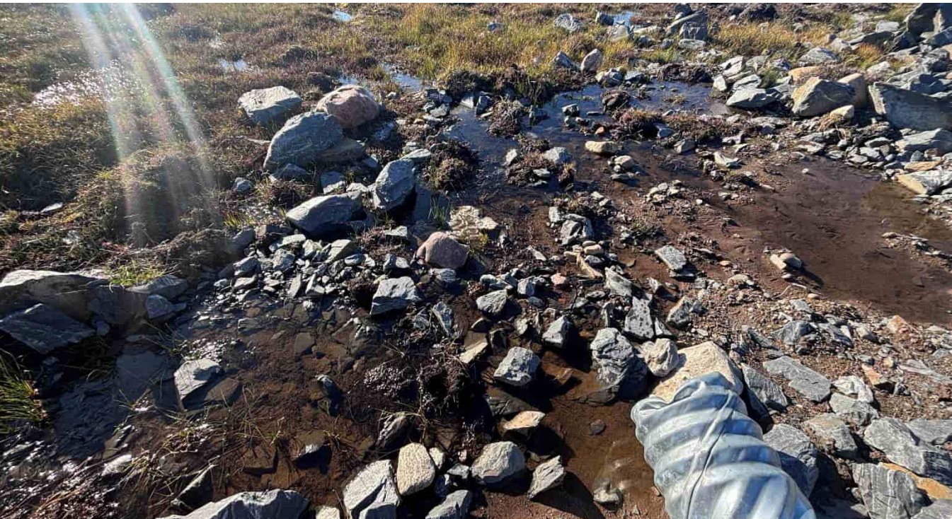
G-159: Downstream of culvert – Some damage to pipe
