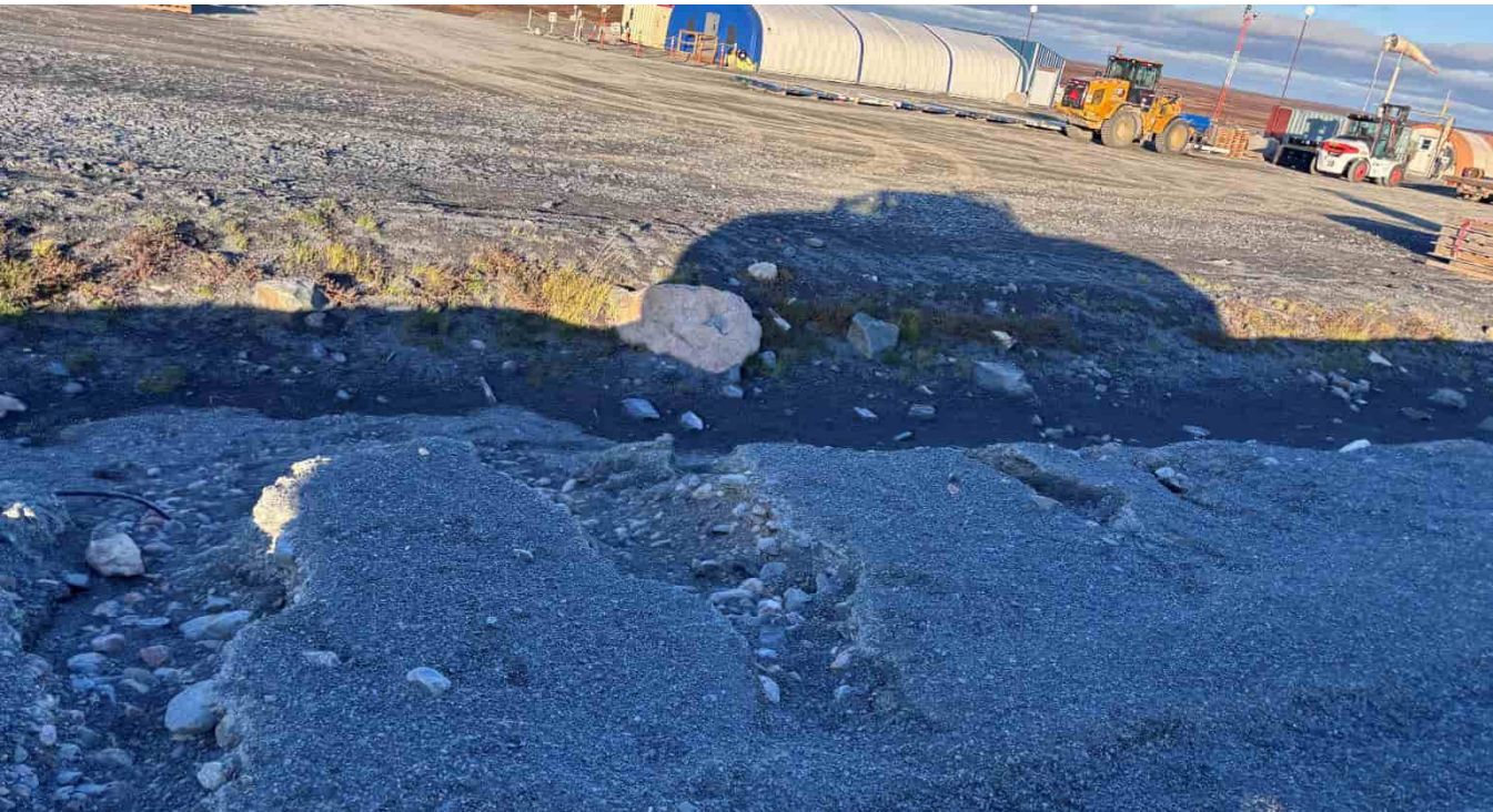
G-74: Erosion beside laydown area
