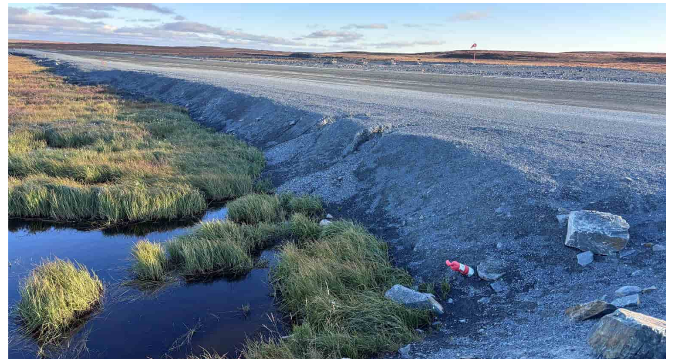
G-66: Erosion pathways and ponding on NE side of runway
