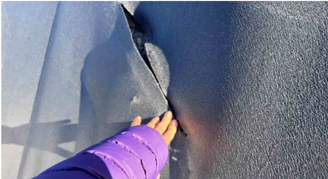
G-162: Liner damage on northernmost pond
