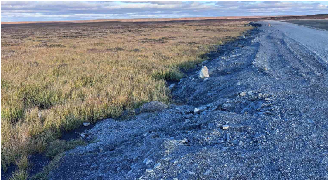
G-65: Erosion pathways on NE side of runway
