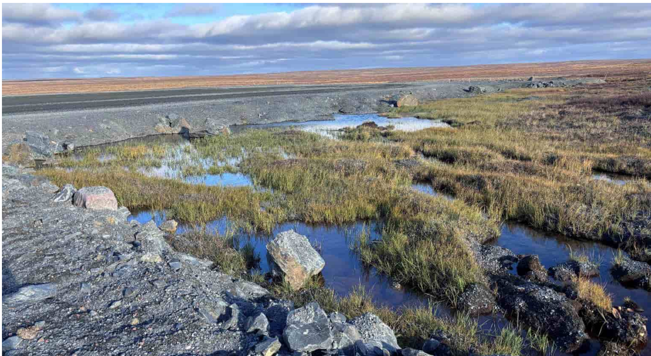
G-57: Ponding at SE end of runway, looking E
