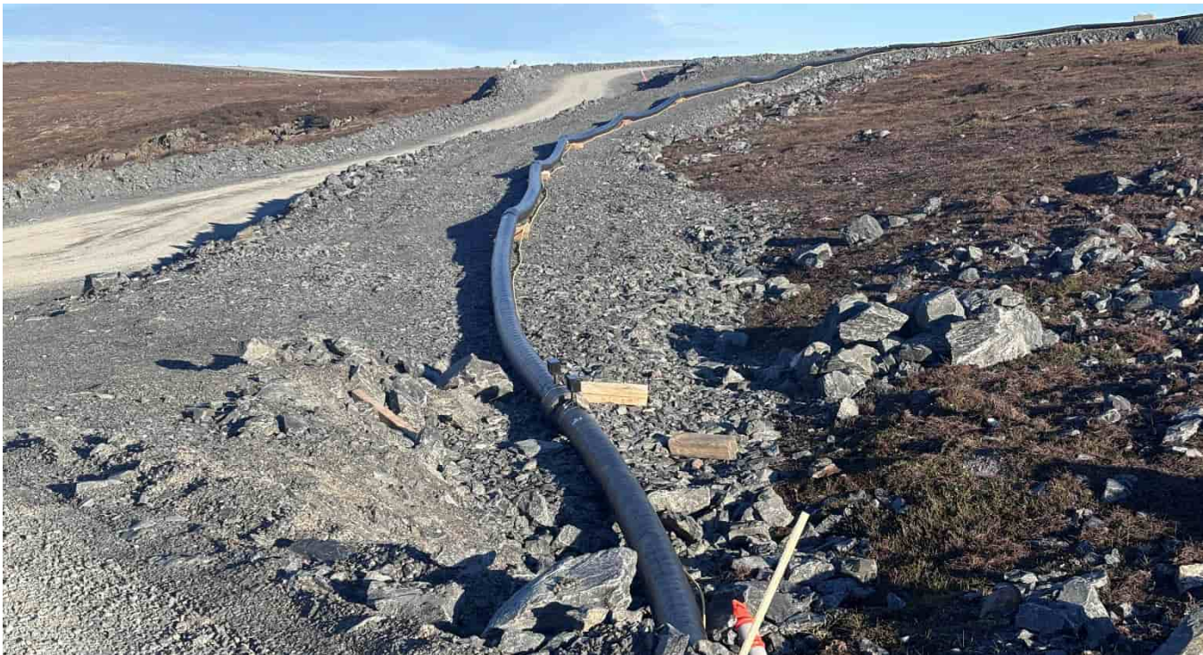
G-181: Barge area pipeline, looking SE
