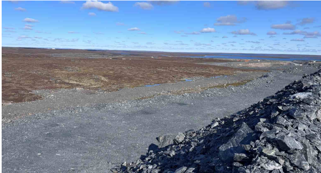
G-138: Looking N towards Echo Diversion from waste rock storage area – ponding water beside diversion and steep slope of waste rock dump
