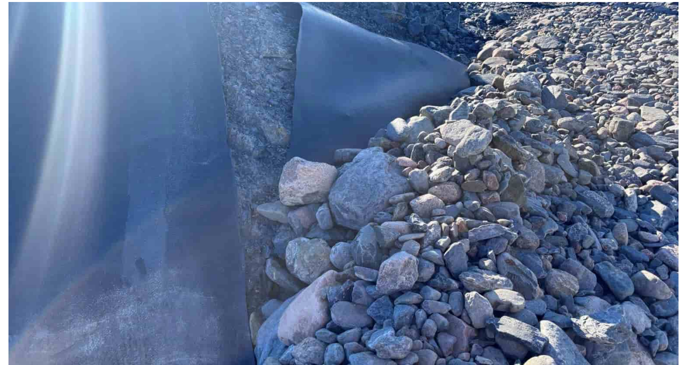
G-163: Inconsistent liner placement underneath rock fill
