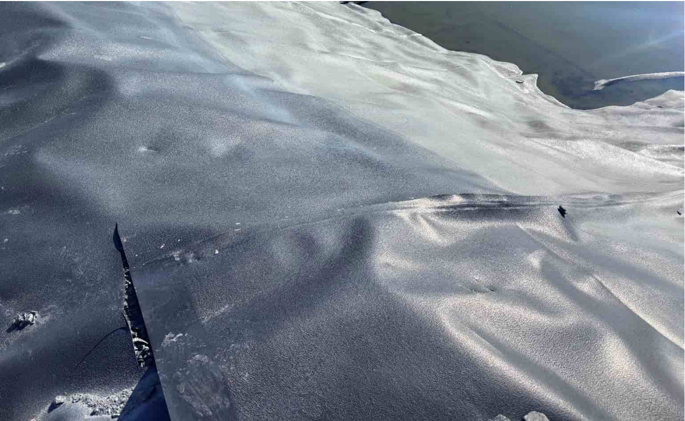
G-151: Treatment pond liner damage above / top of slope
