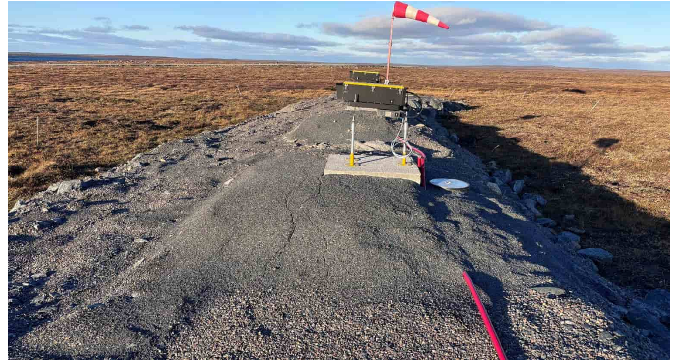
G-76: Unfinished construction of airstrip lights
