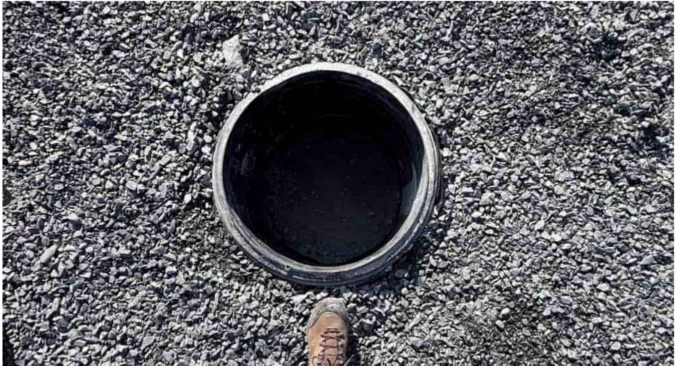
G-212: Tote Storage Facility: sump
