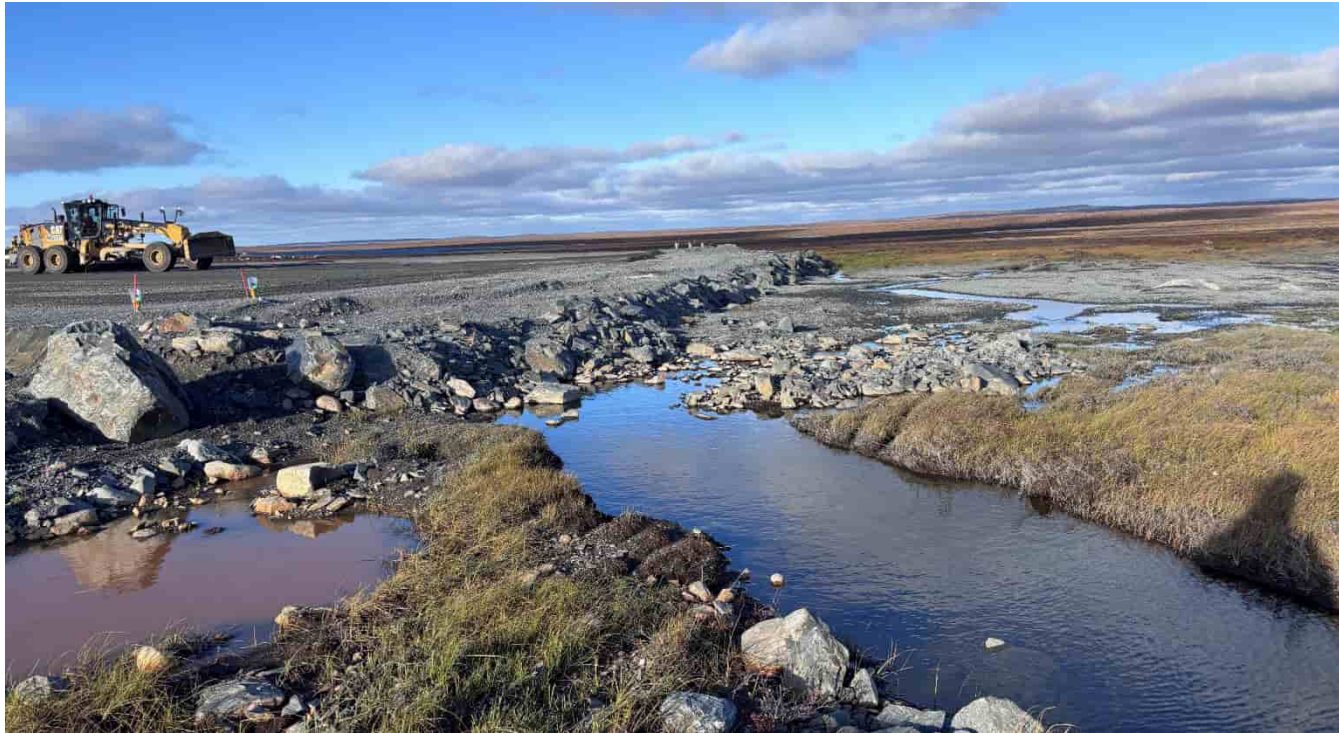
G-59: Stream beside SE end of runway, looking NE – lower pad thickness in area, ongoing settlement
