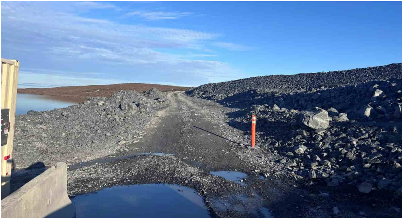
G-177: Barge access road, looking E – Note ponding water
