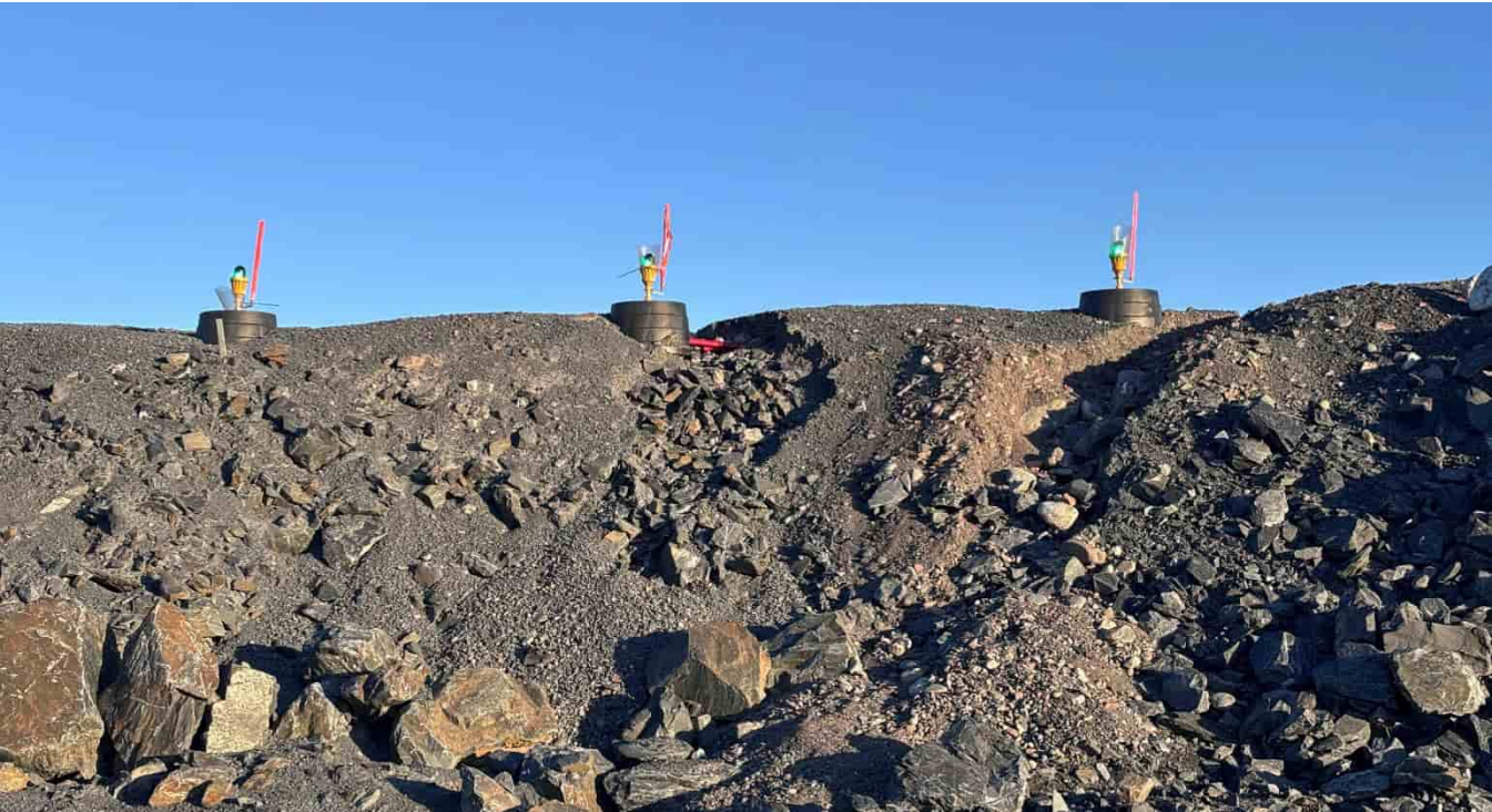
G-84: Erosion pathways at NW end of airstrip beside airstrip lights
