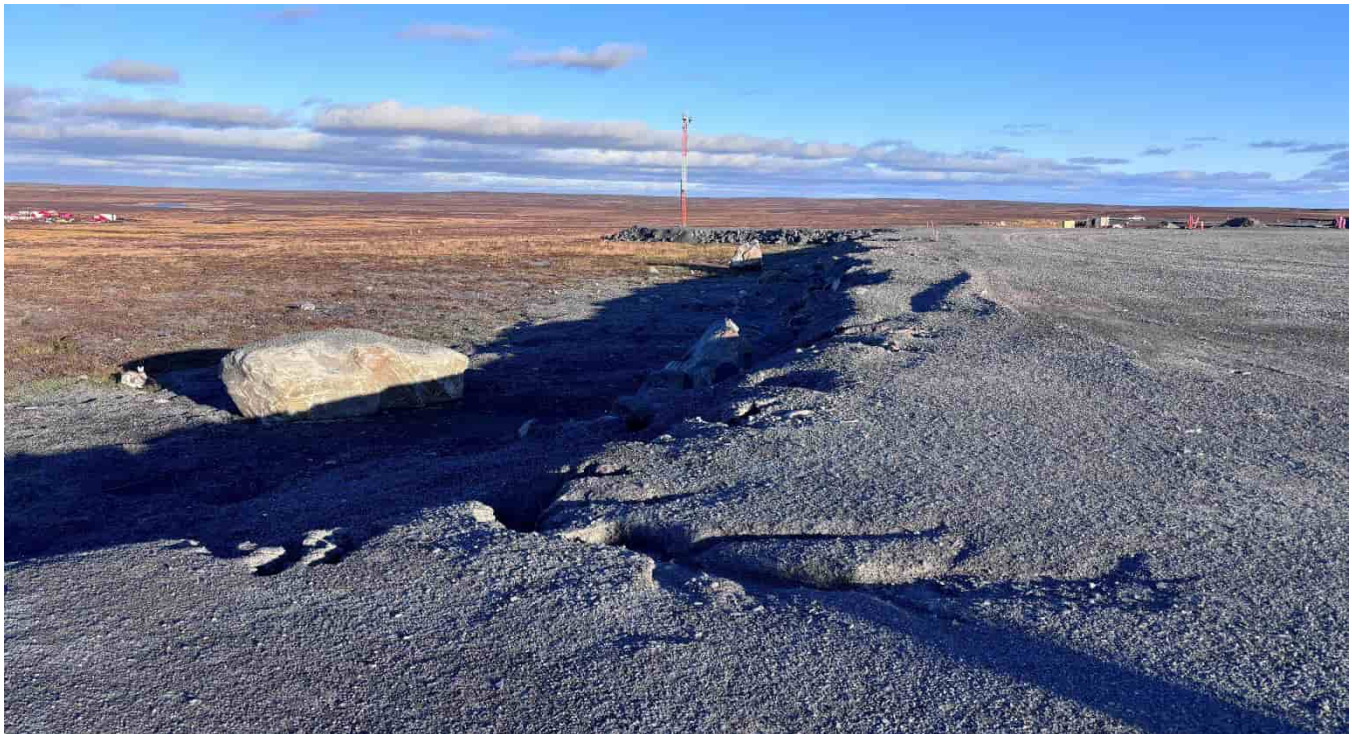
G-69: Erosion on NE apron, looking SE
