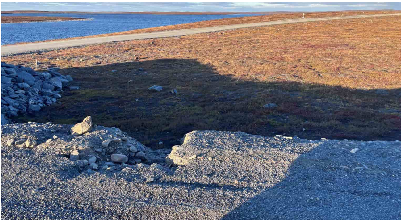
G-77: Erosion pathway at NW end of runway
