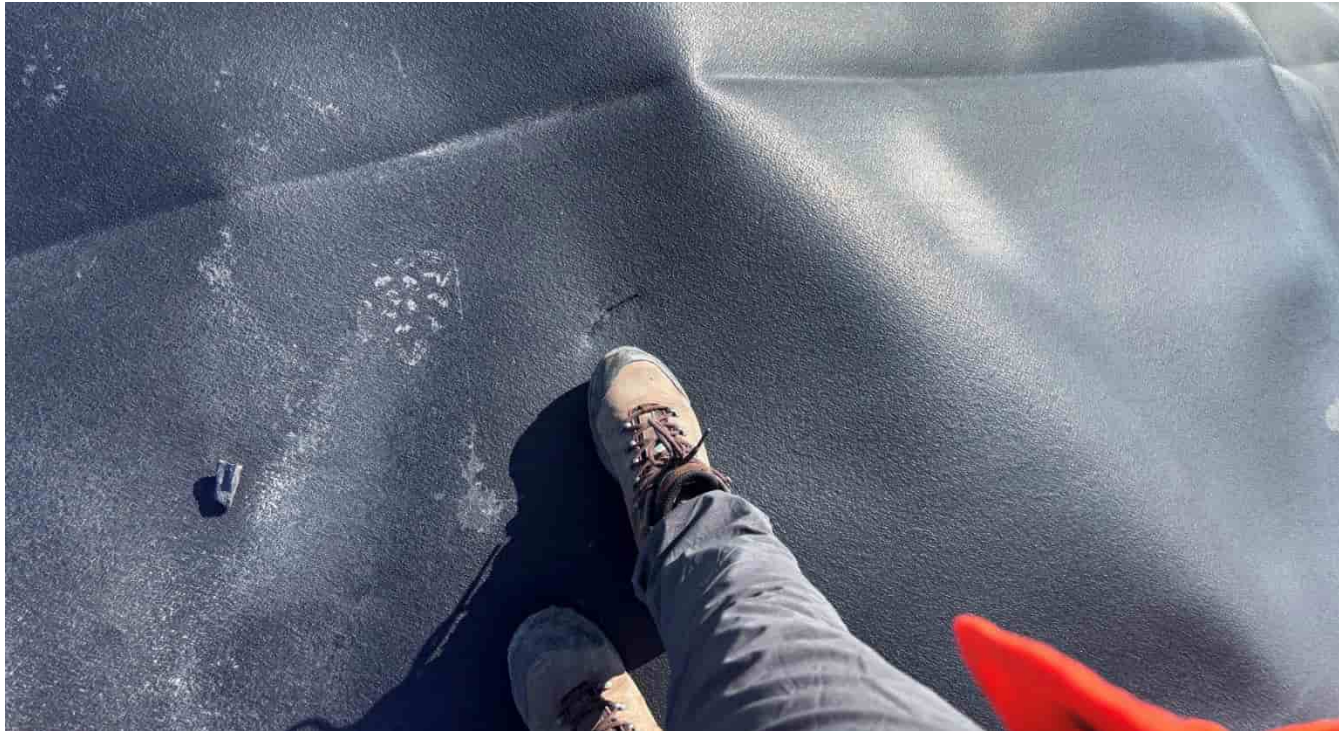
G-152: Exampke liner damage beside southernmost pond
