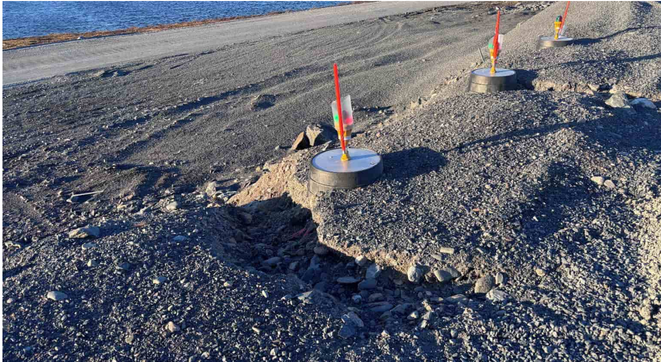
G-79: Erosion at NW end of runway, above All-Weather Road
