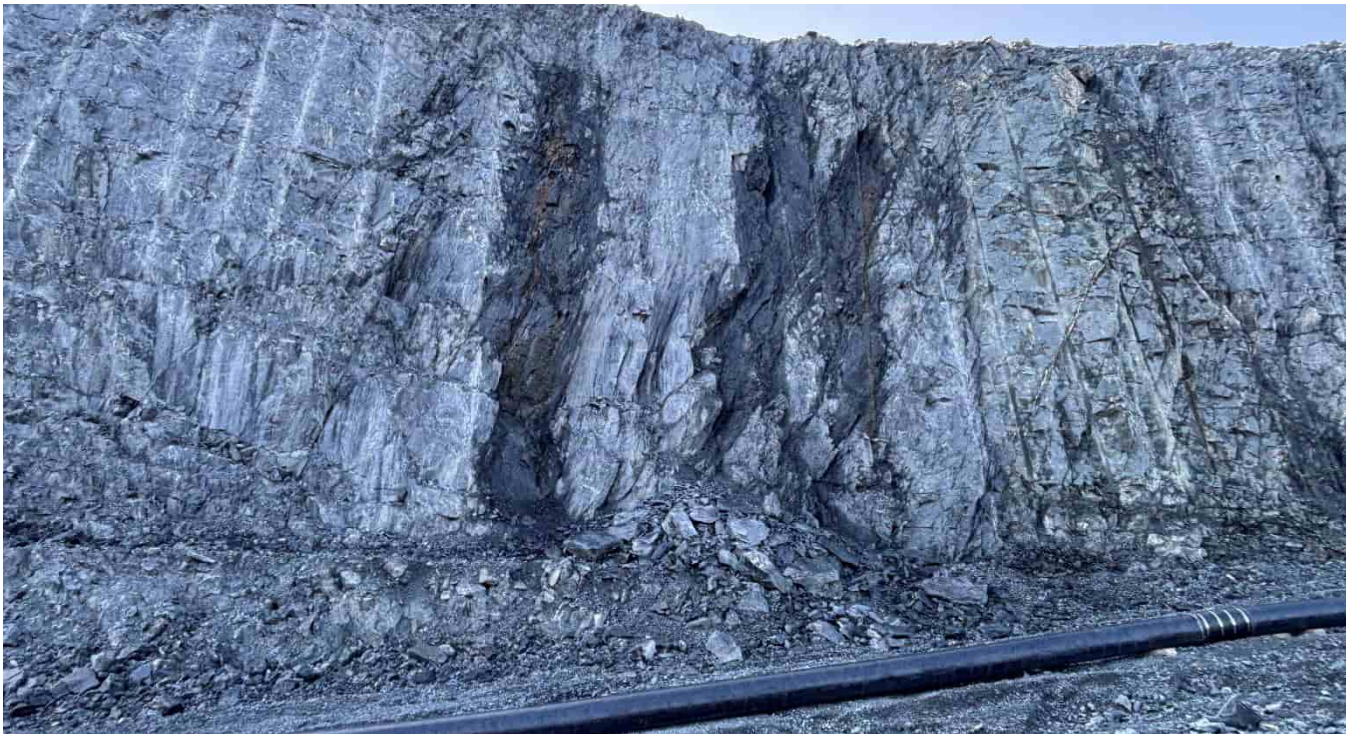
G-122: Tailings pipeline, eastern highwall
