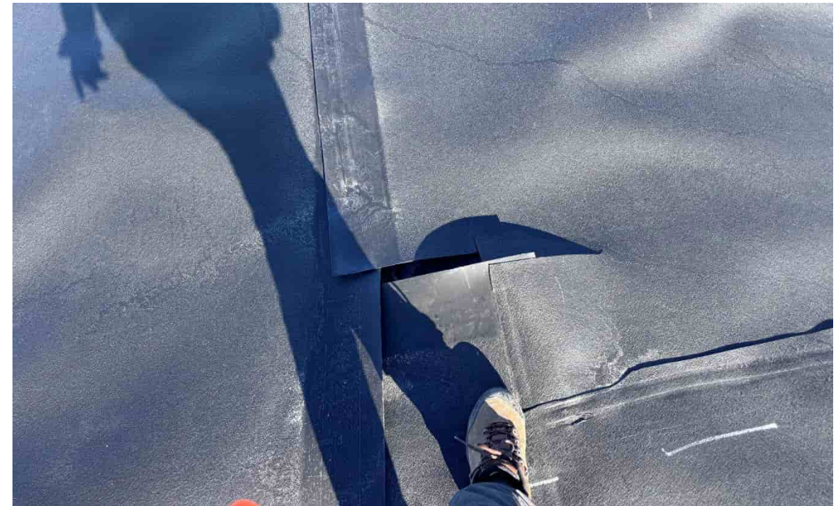
G-149: Gap in treatment pond liner – higher elevation
