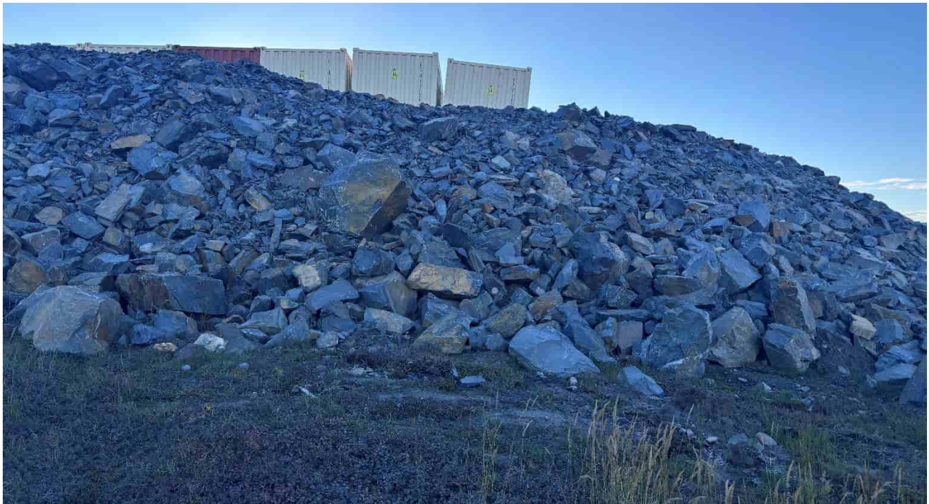
G-198: Slope beside laydown, facing W – Note differential settlement of northernmost seacan
