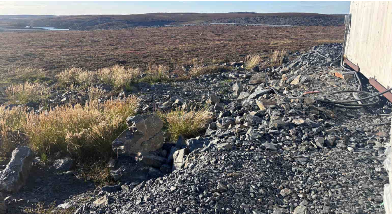
G-104: Pad toe, slope and erosion beside Seacan
