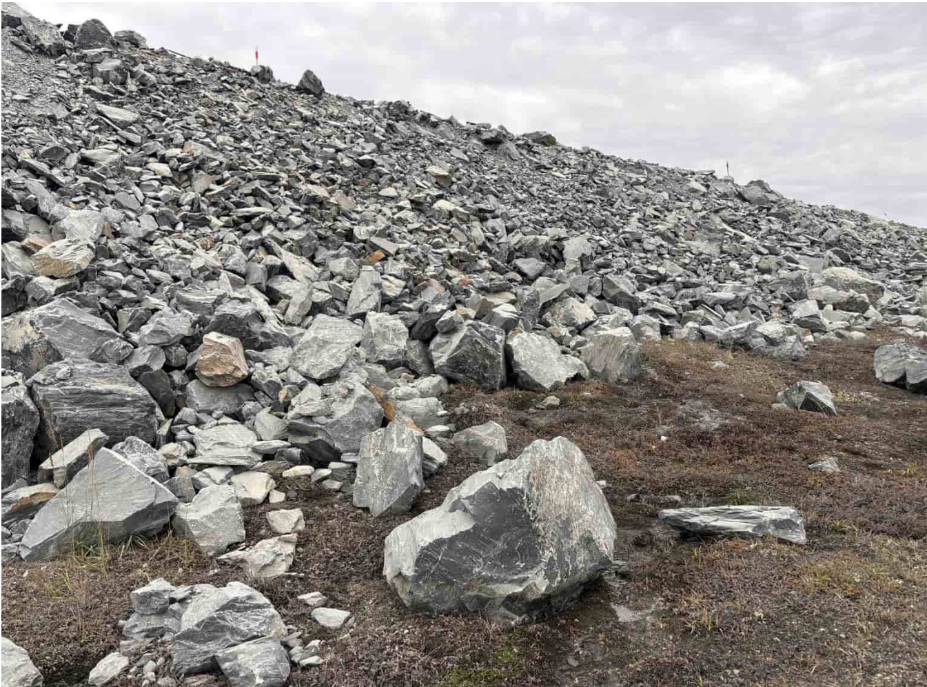
G-257: Water seepage from road rockfill
