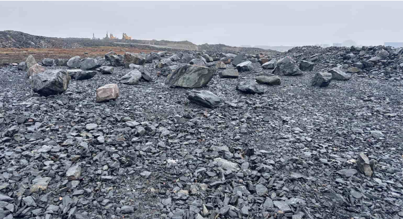
G-455: Large blast rocks at end of spillway, looking S
