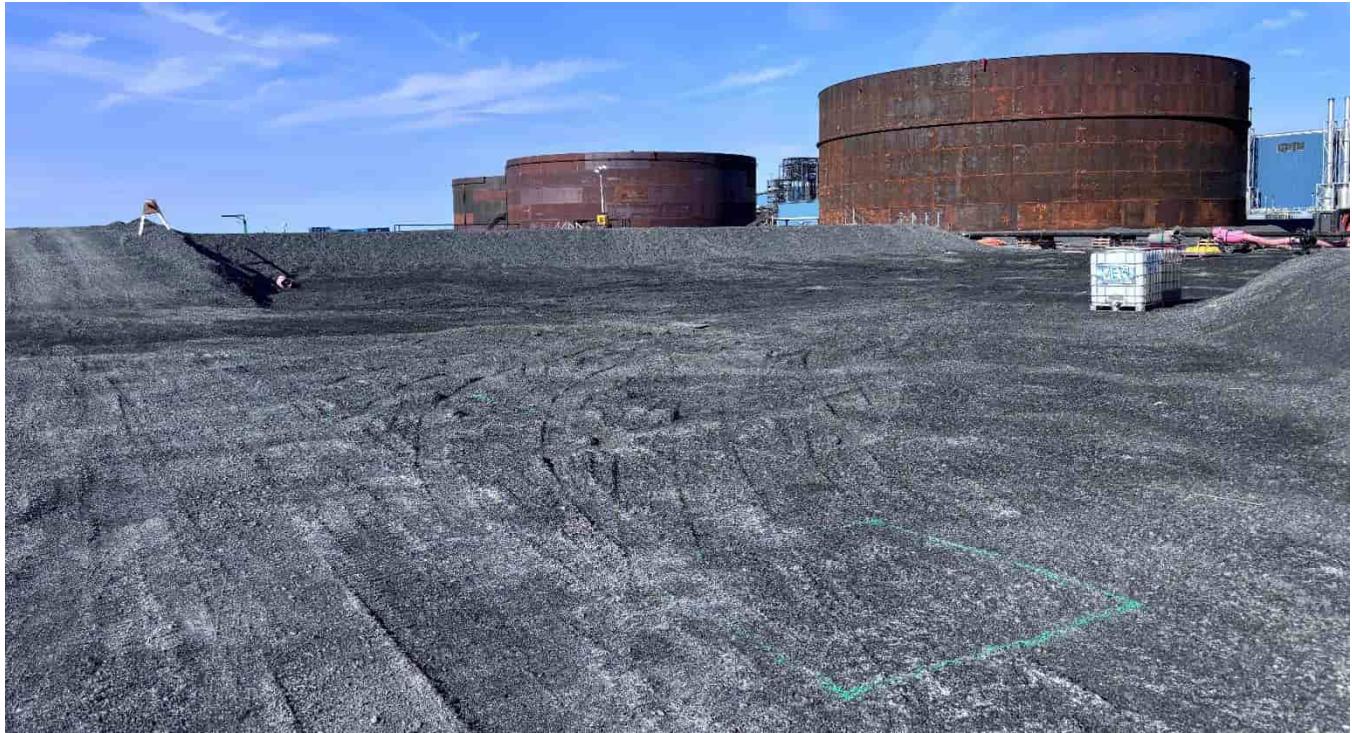
G-365: Tank farm surface conditions at southeastern end, looking NW
