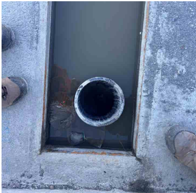
G-379: Fuel transfer / refueling sump
