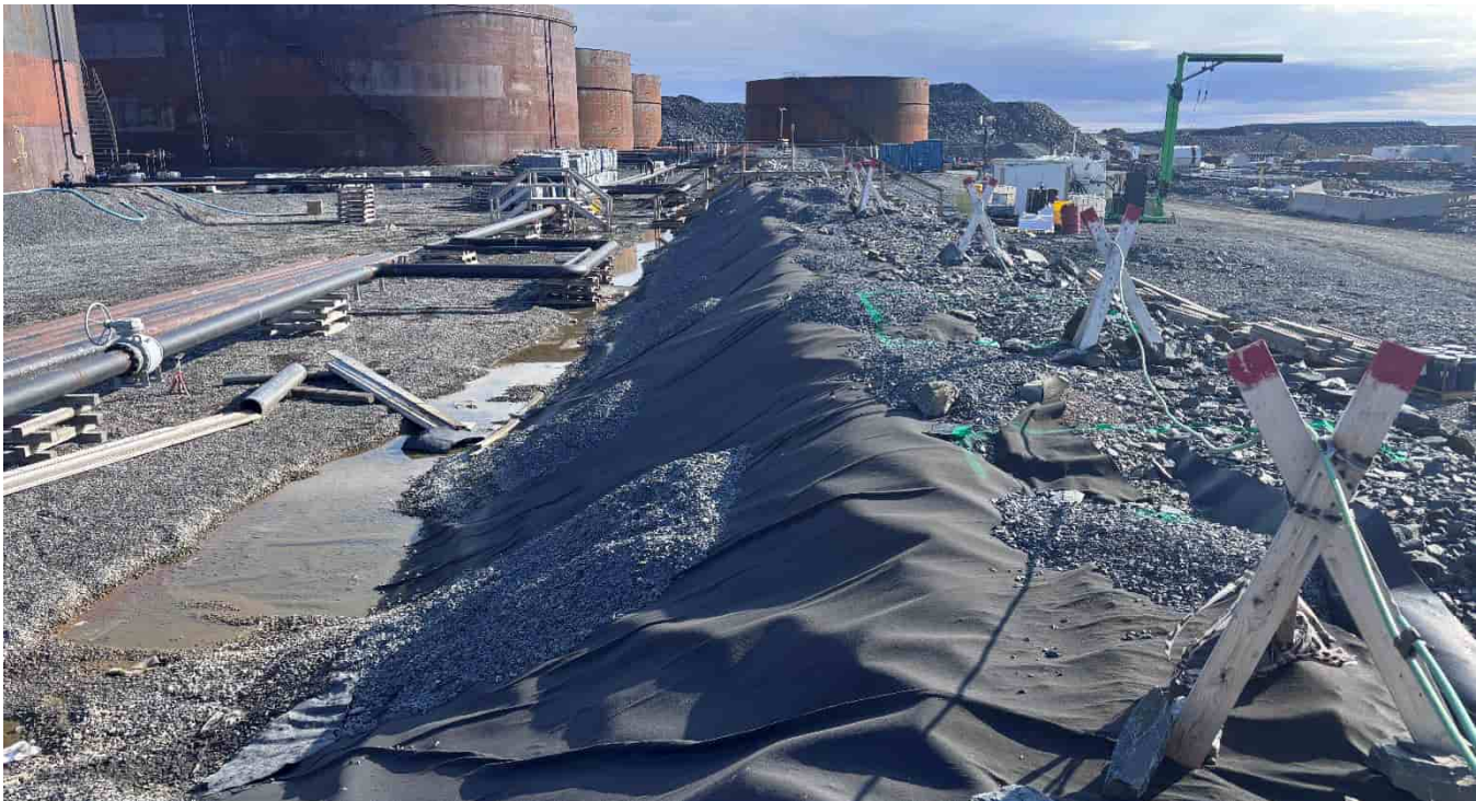
G-349: Exposed geotextile on southern berm – ponding at toe of slope, undulating liner anchoring
