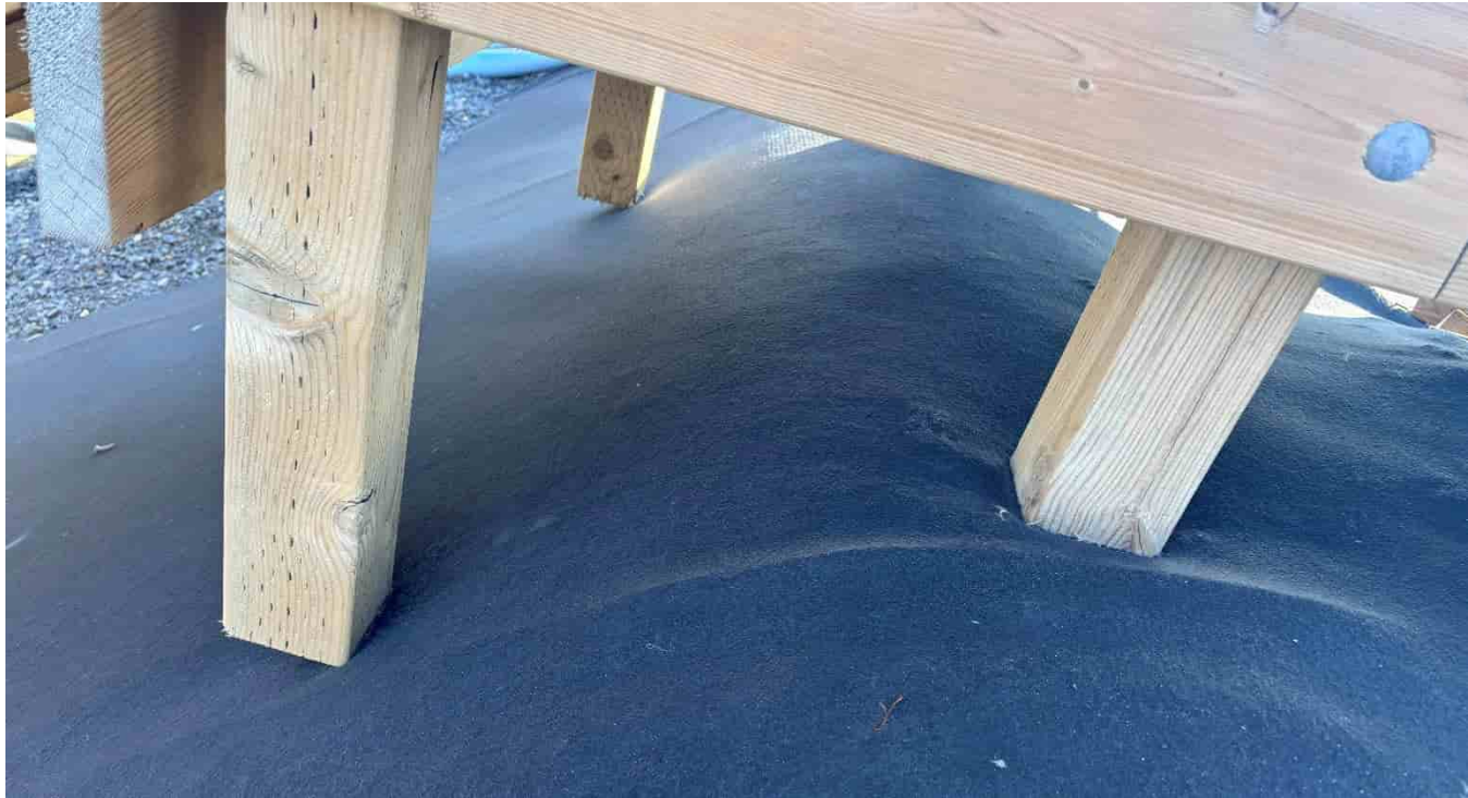
G-354: Wooden stairwell supports on exposed geotextile
