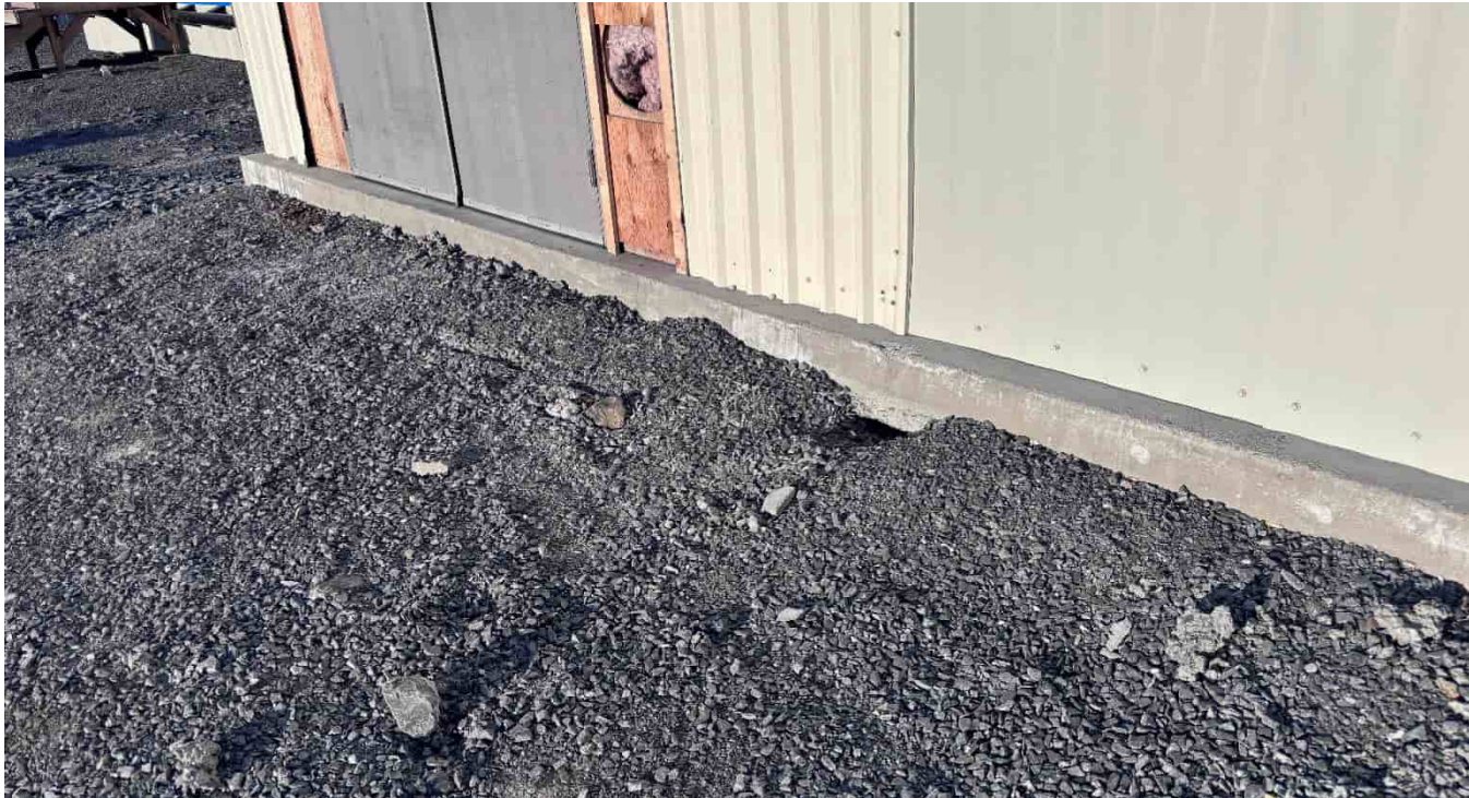
G-270: Surface water flow path / erosion under infrastructure foundation
