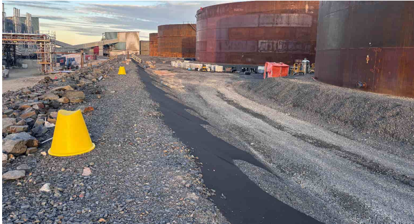
G-343: Exposed liner on tank farm northern berm slope, looking E
