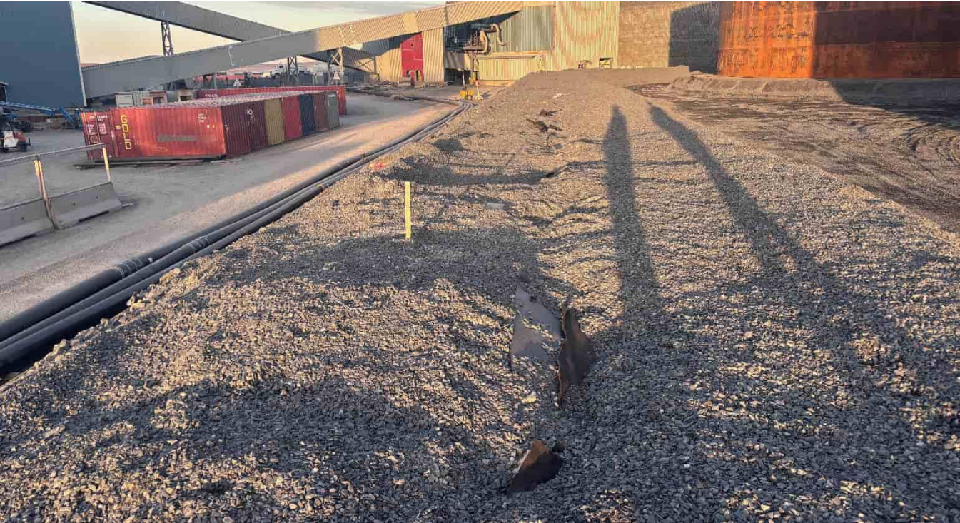
G-339: Exposed liner on northern berm, looking E
