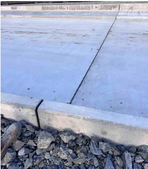
G-372: Fuel transfer / refueling concrete pad Seam
