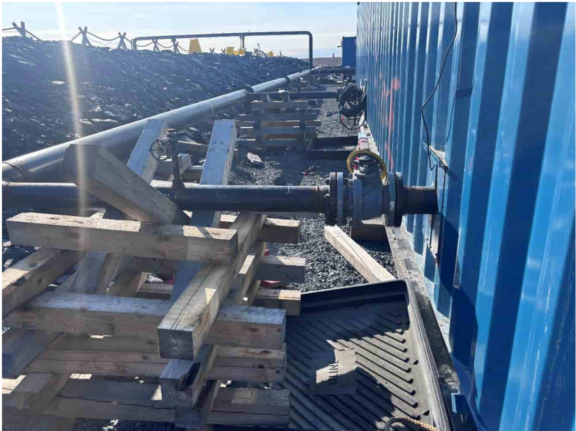
G-378: fuel transfer / refueling pipe connection to seacan
