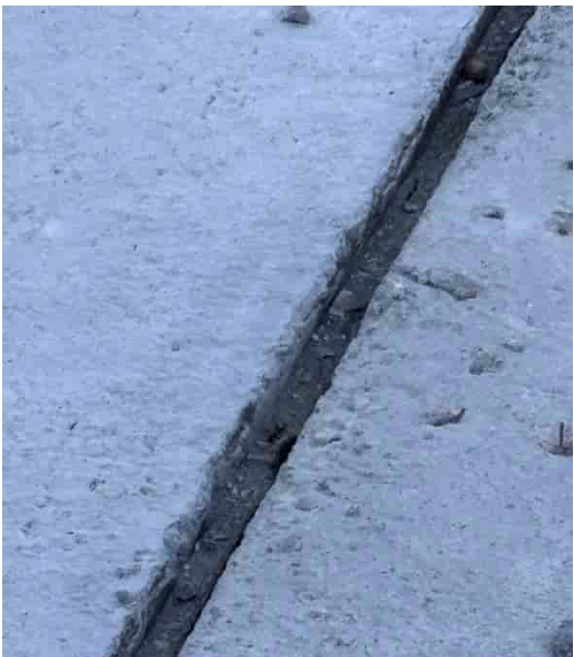
G-373: Close-up view of fuel transfer / refueling concrete pad seam
