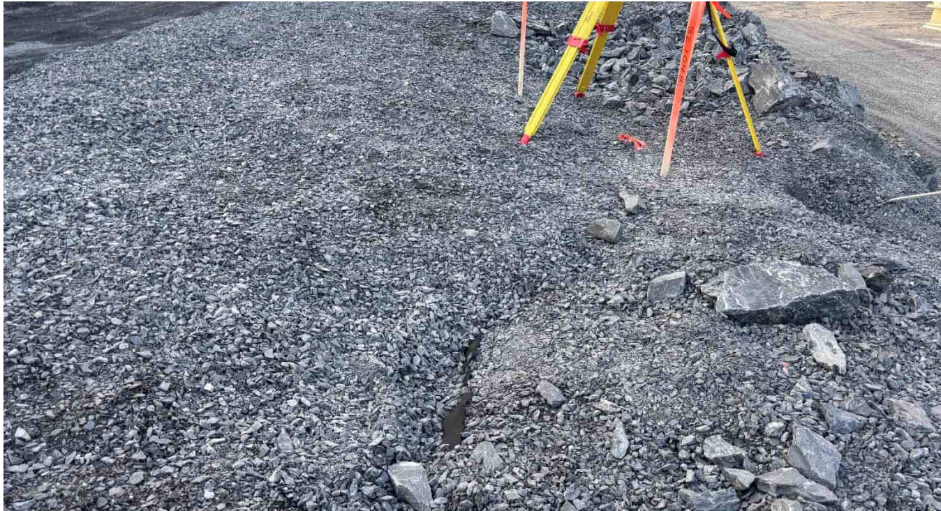
G-330: Exposed liner and degradation to overliner cover tank farm berm
