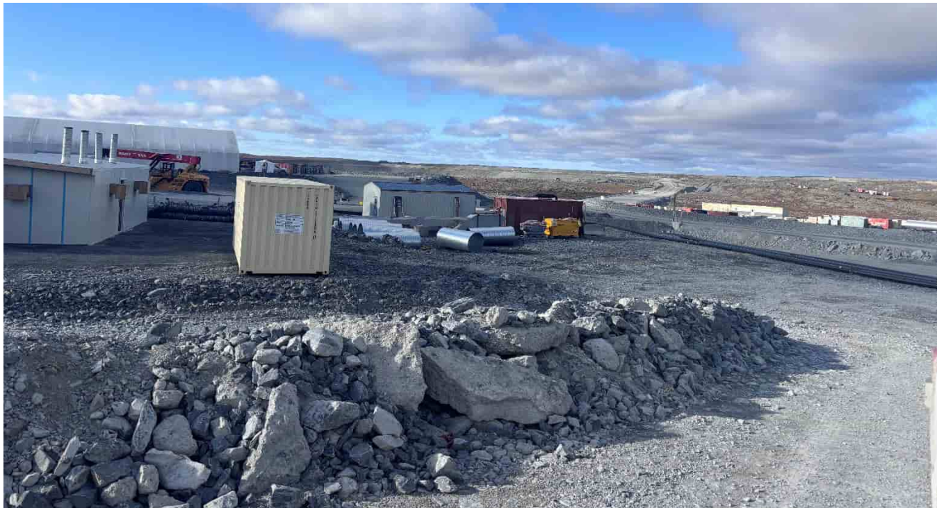
G-306: Looking W towards vent raise, laydown, All-Weather Road, and tailings pipeline
