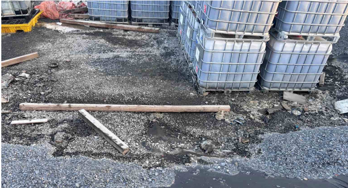
G-346: Tote storage area below northern berm
