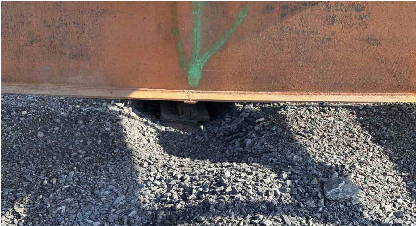
G-364: A gap between pedestal and base of Tank 5
