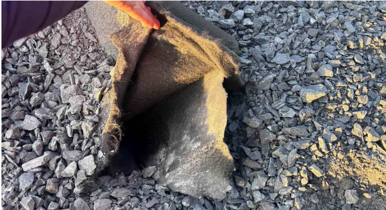
G-334: Exposed and damaged liner on tank farm northern berm slope
