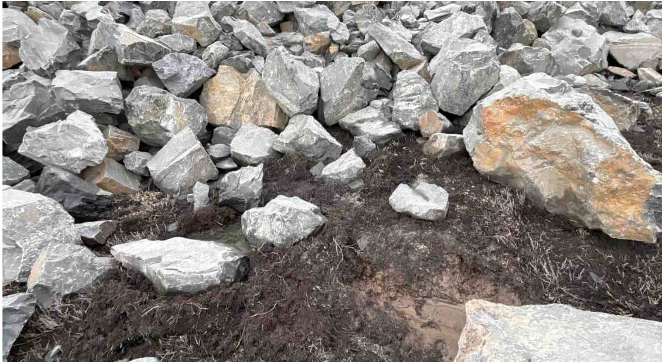
G-252: Damage to tundra due to rockfall from oversteepened slope of All-Weather Road N rockfill – water seepage noted through / below rockfill
