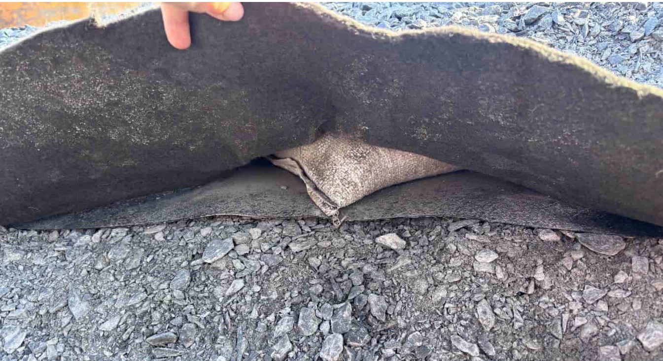
G-357: Sand bag noted below geotextile near crest of berm
