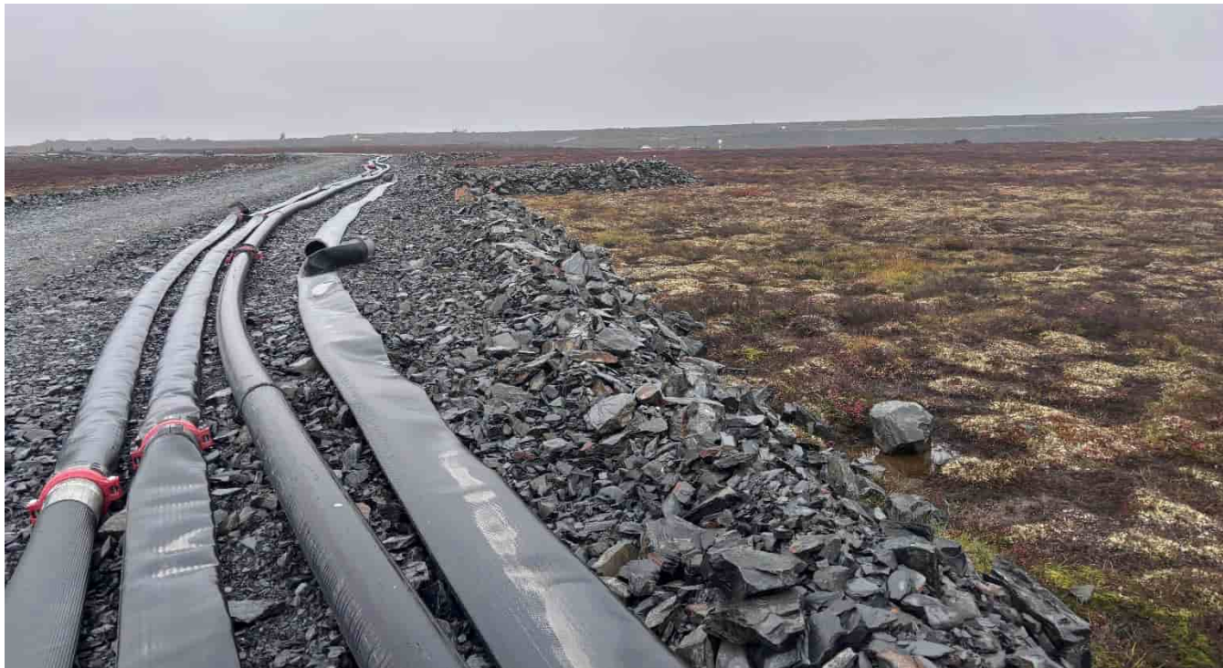
G-446: Unfinished piping along SWP Dam Access Road, looking N
