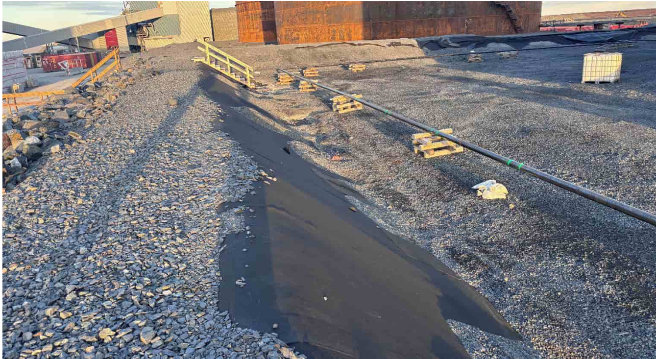
G-342: Exposed liner on tank farm northern berm slope, looking E
