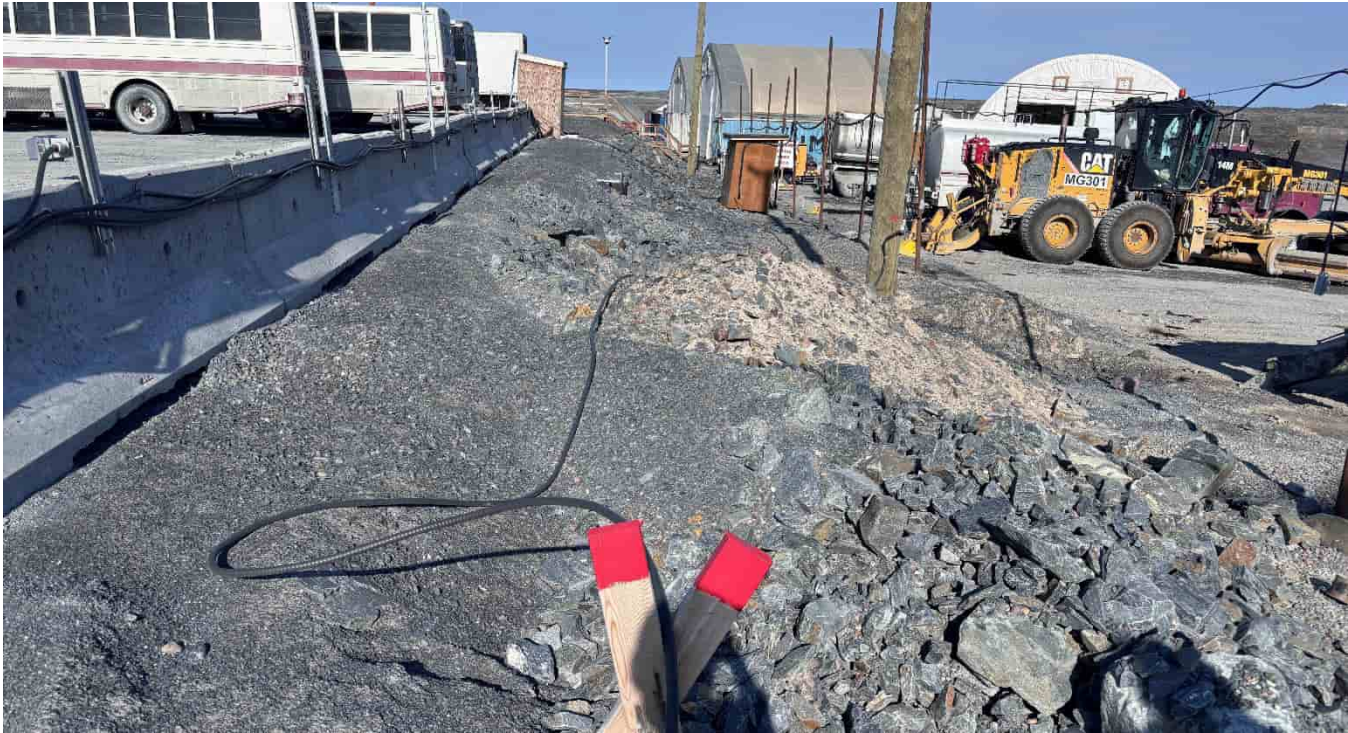
G-301: Laydown area E of main camp, looking S at erosion to slope
