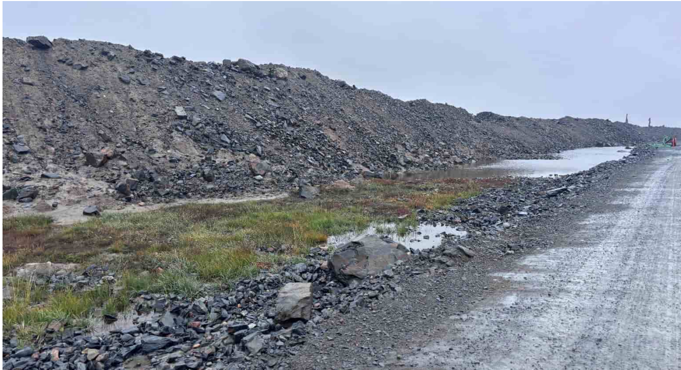
G-406: Ponding between road and N slope of stockpile pad, looking W – thinner rockfill road in area
