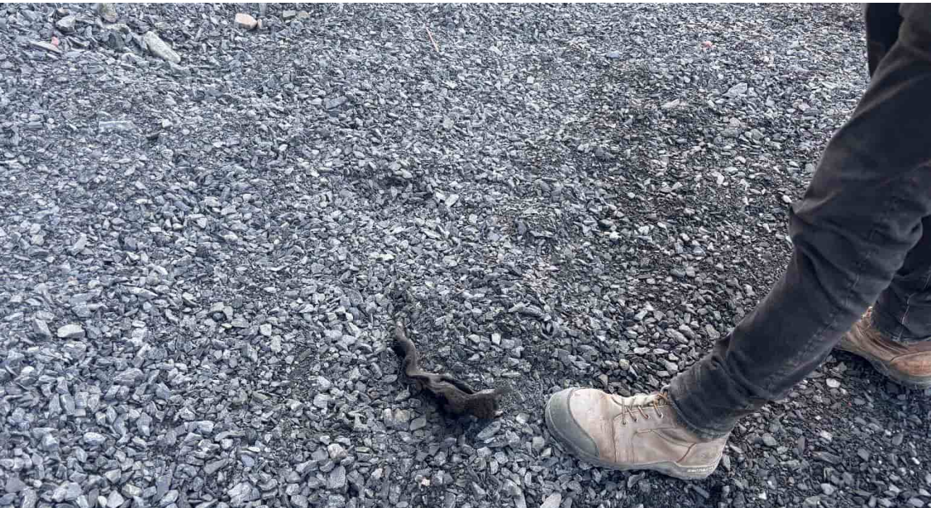
G-337: Exposed and damaged liner on tank farm northern berm slope
