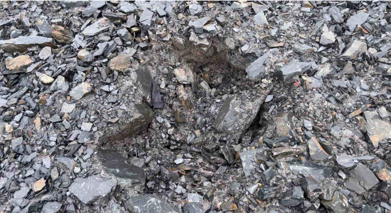
G-411: Sinkhole in storage area pad surface
