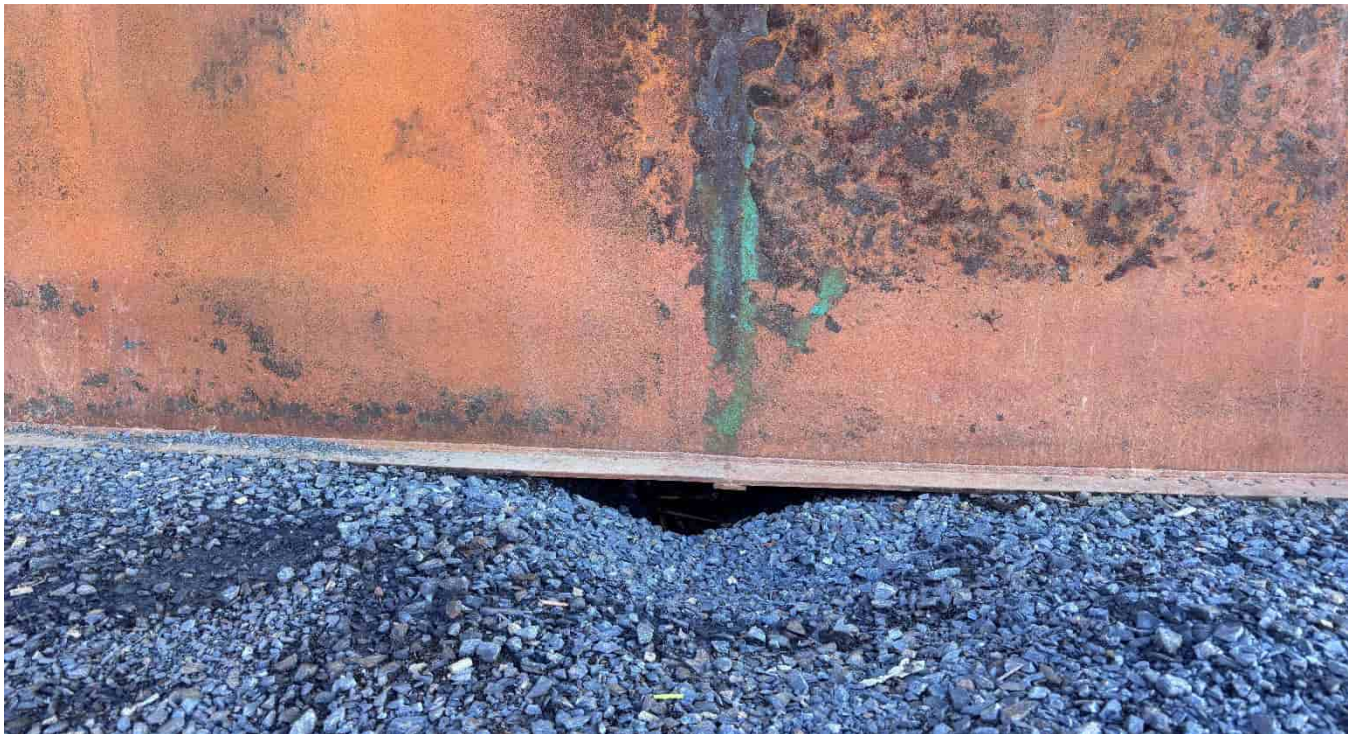
G-363: A gap between pedestal and base of Tank 5 – former installation jack location based on tank marks
