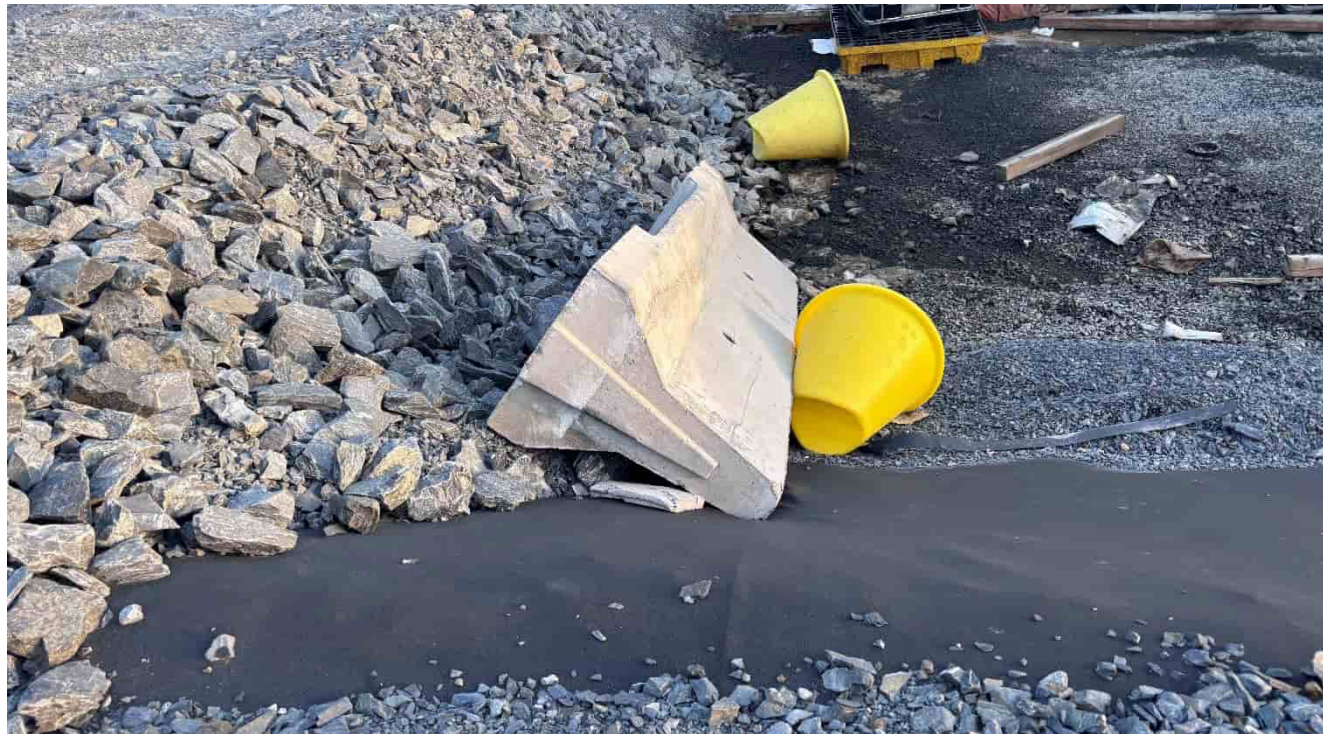
G-344: Fallen barrier on western berm liner, looking E
