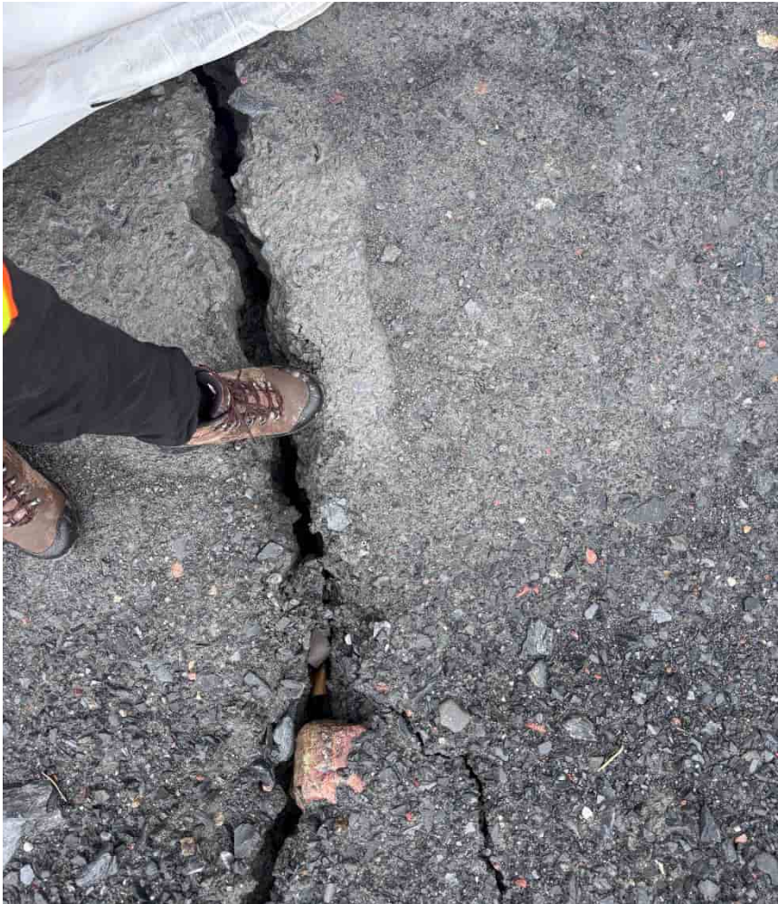
G-438: Large tension crack near building foundation
