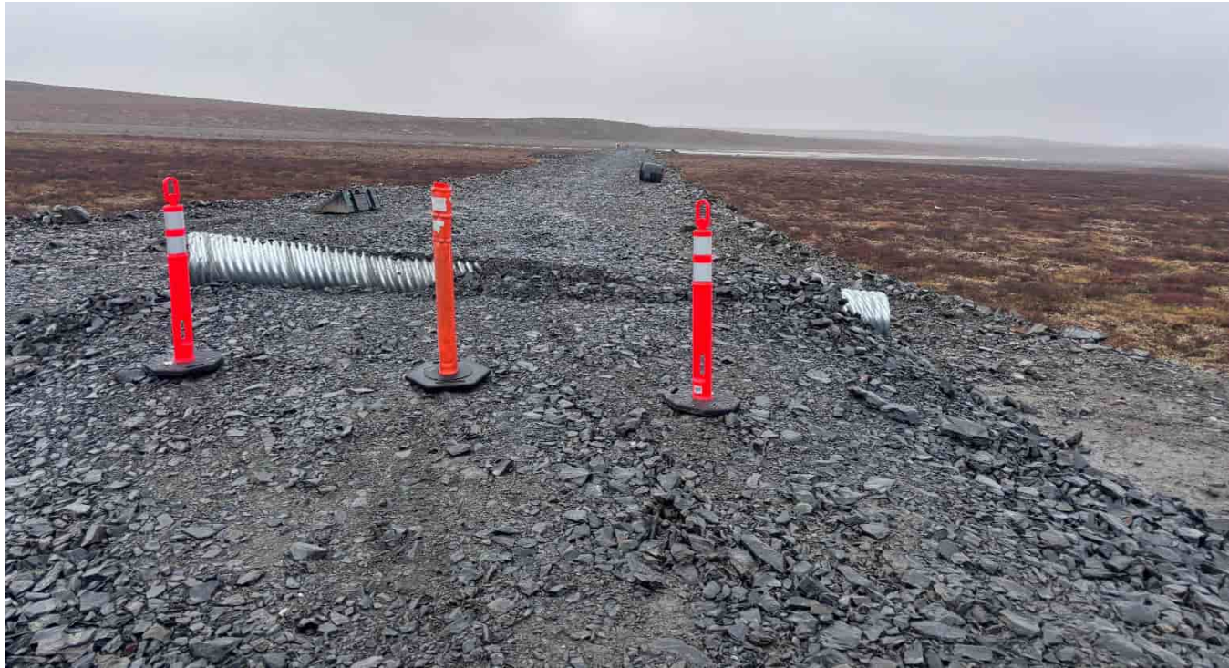
G-440: Exposed culvert on Saline Water Pond Access Road, looking W
