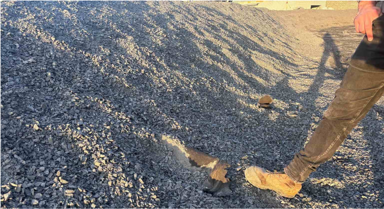
G-335: Exposed and damaged liner on tank farm northern berm slope
