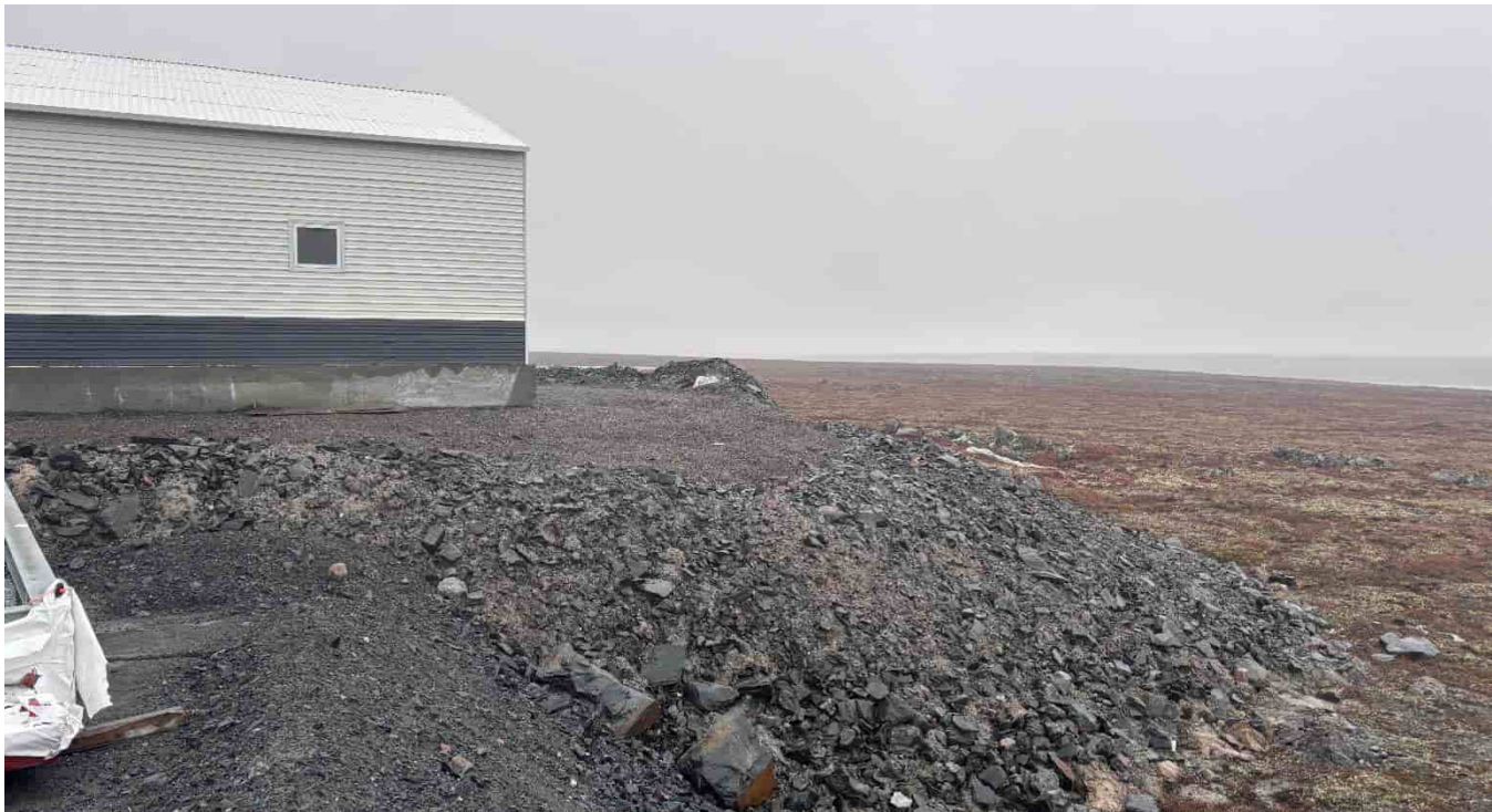
G-439: Settlement of pad near building, looking N
