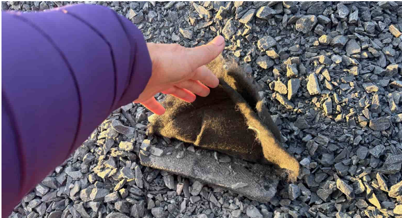
G-336: Exposed and damaged liner on tank farm northern berm slope
