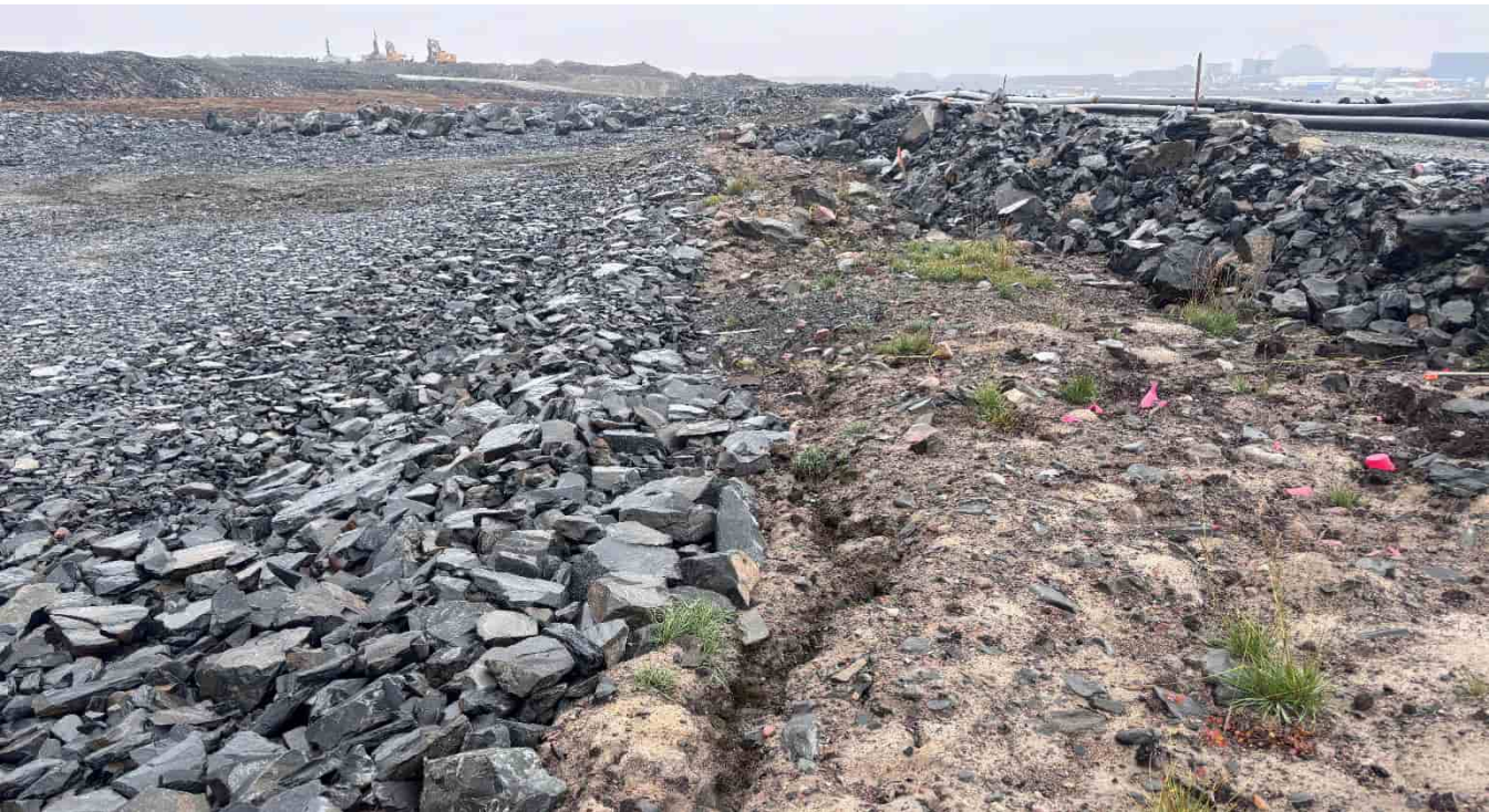
G-457: Spillway: western berm, looking S, thin rock cladding thickness in areas
