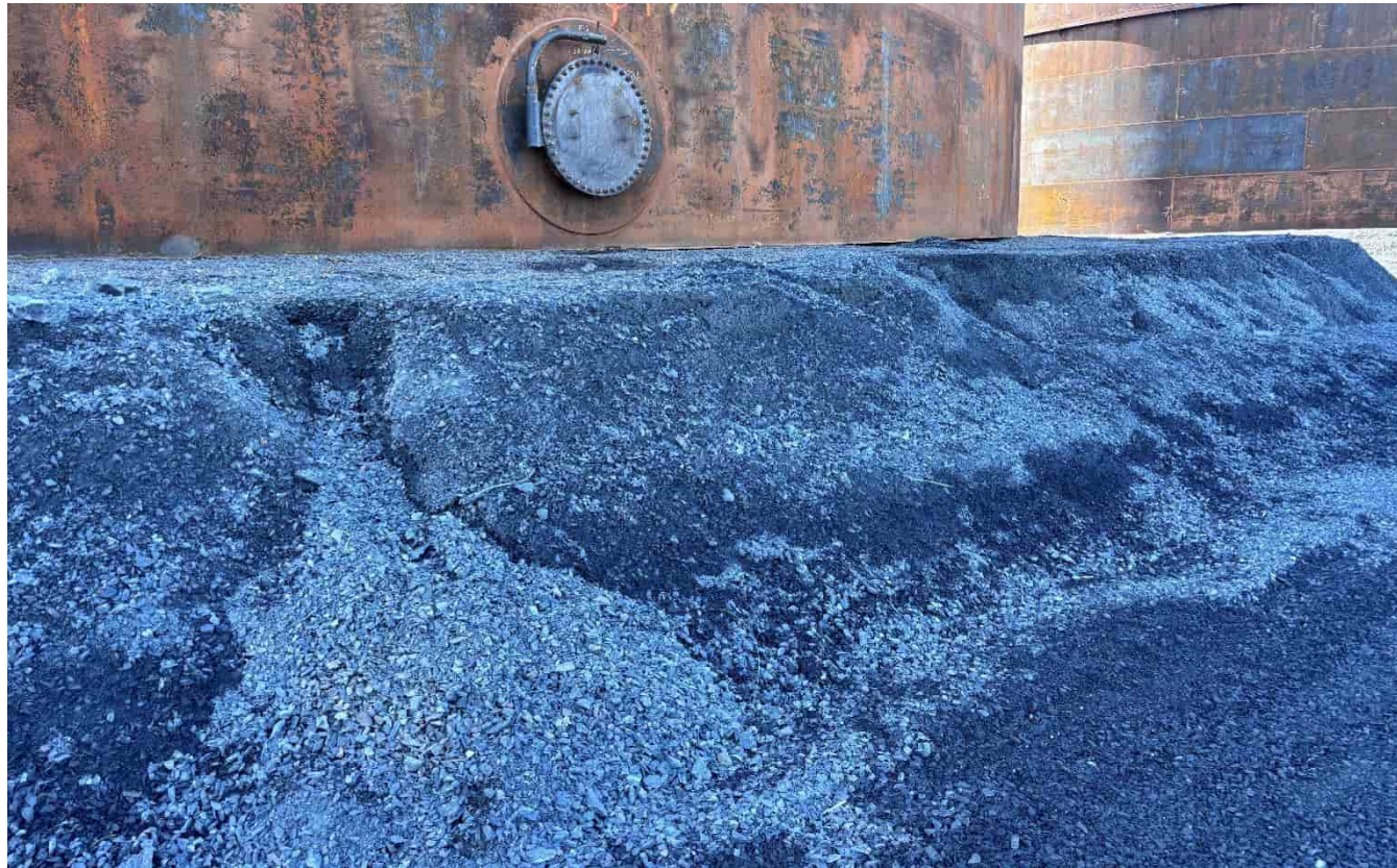
G-369: Pedestal for Tank 1 erosion tracking
