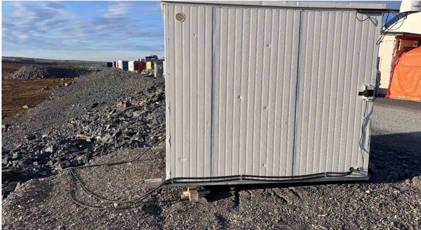
G-273: Storage container close to western pad edge, looking N – settlement and gap beneath container noted
