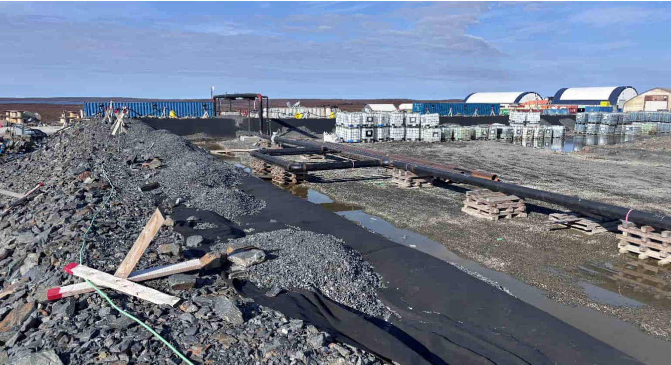
G-355: Southern berm, looking W – exposed liner
