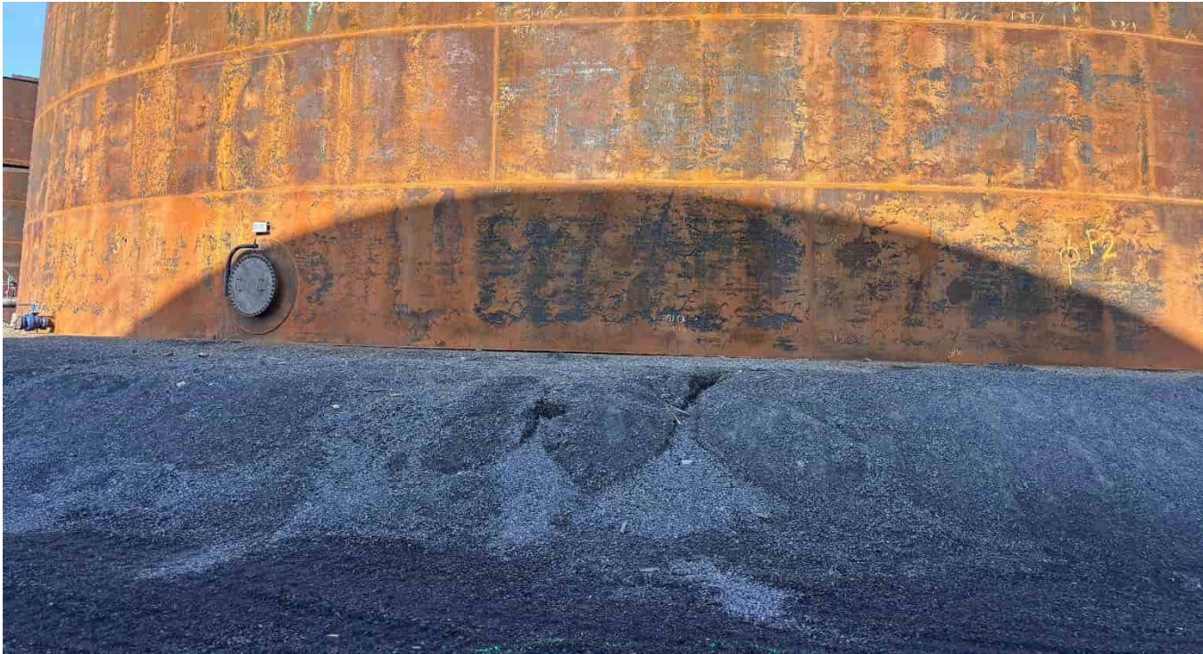
G-366: Erosion pathways starting on on slope beside northeastern tank
