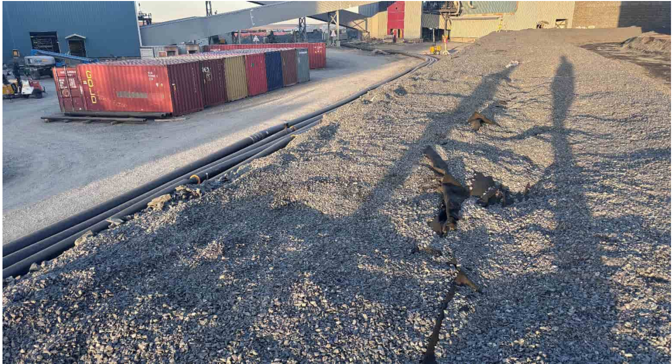
G-338: Exposed liner on northern berm, looking E
