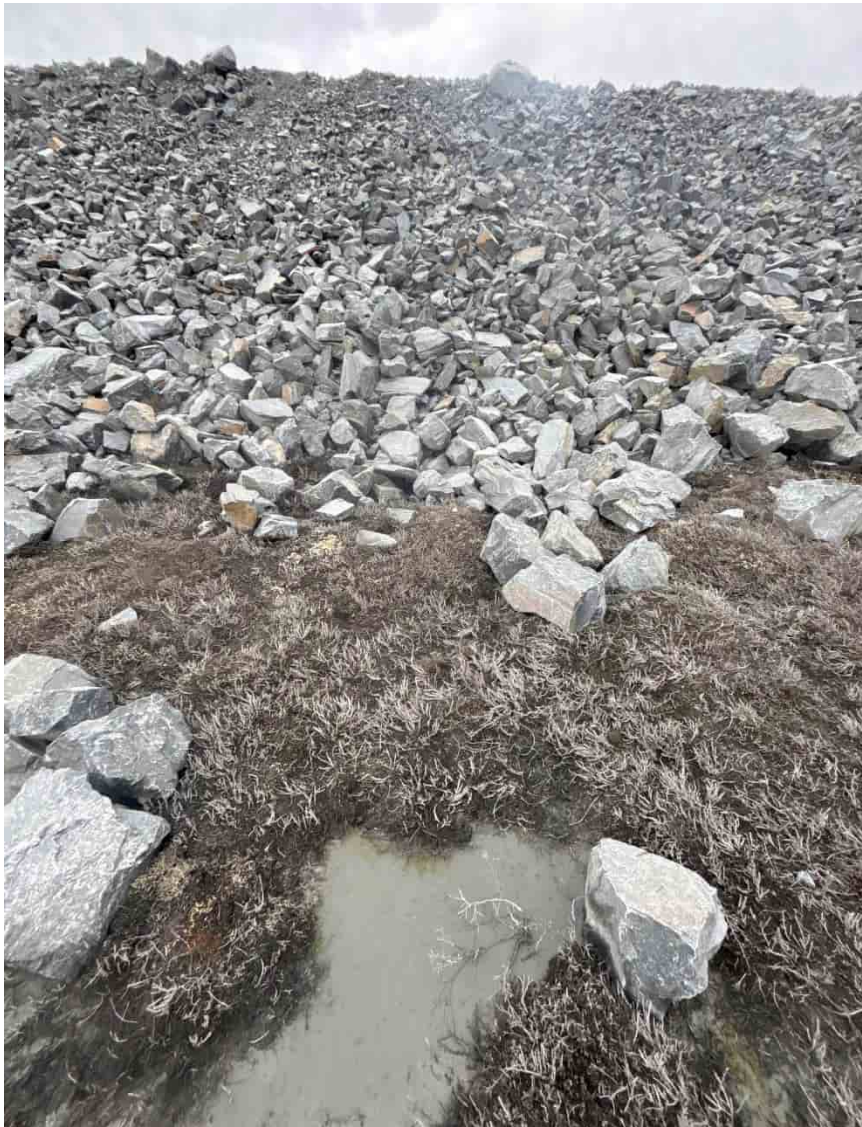
G-256: Water seepage from road rockfill
