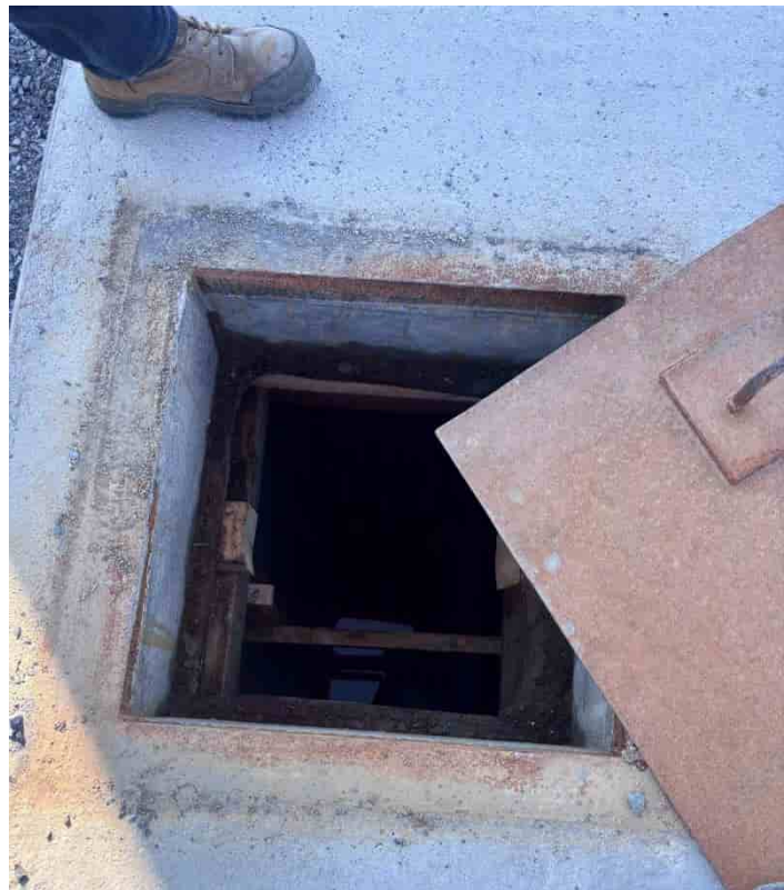
G-380: Fuel transfer / refueling sump access hatch
