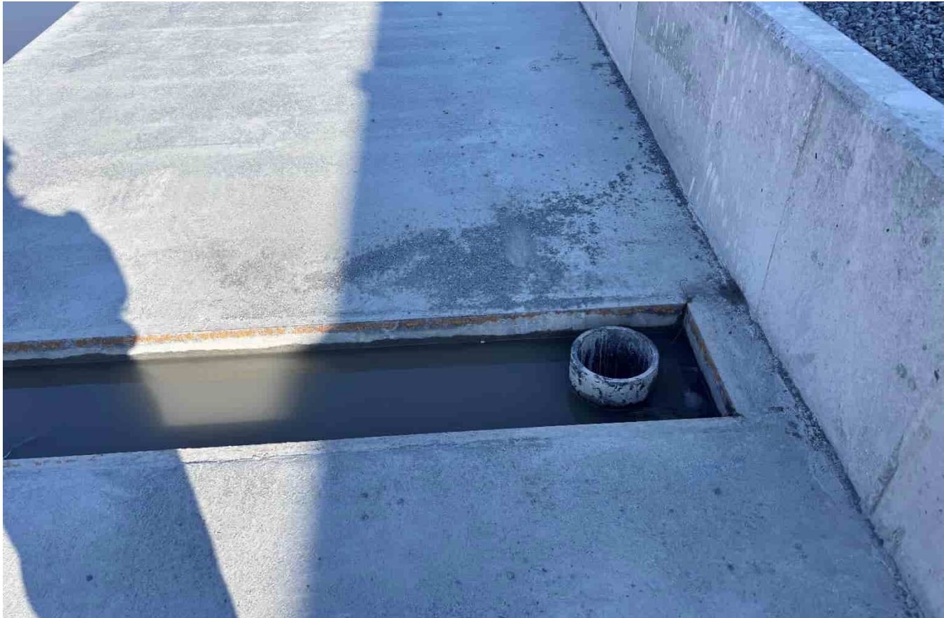
G-381: Fuel transfer / refueling sump, looking N
