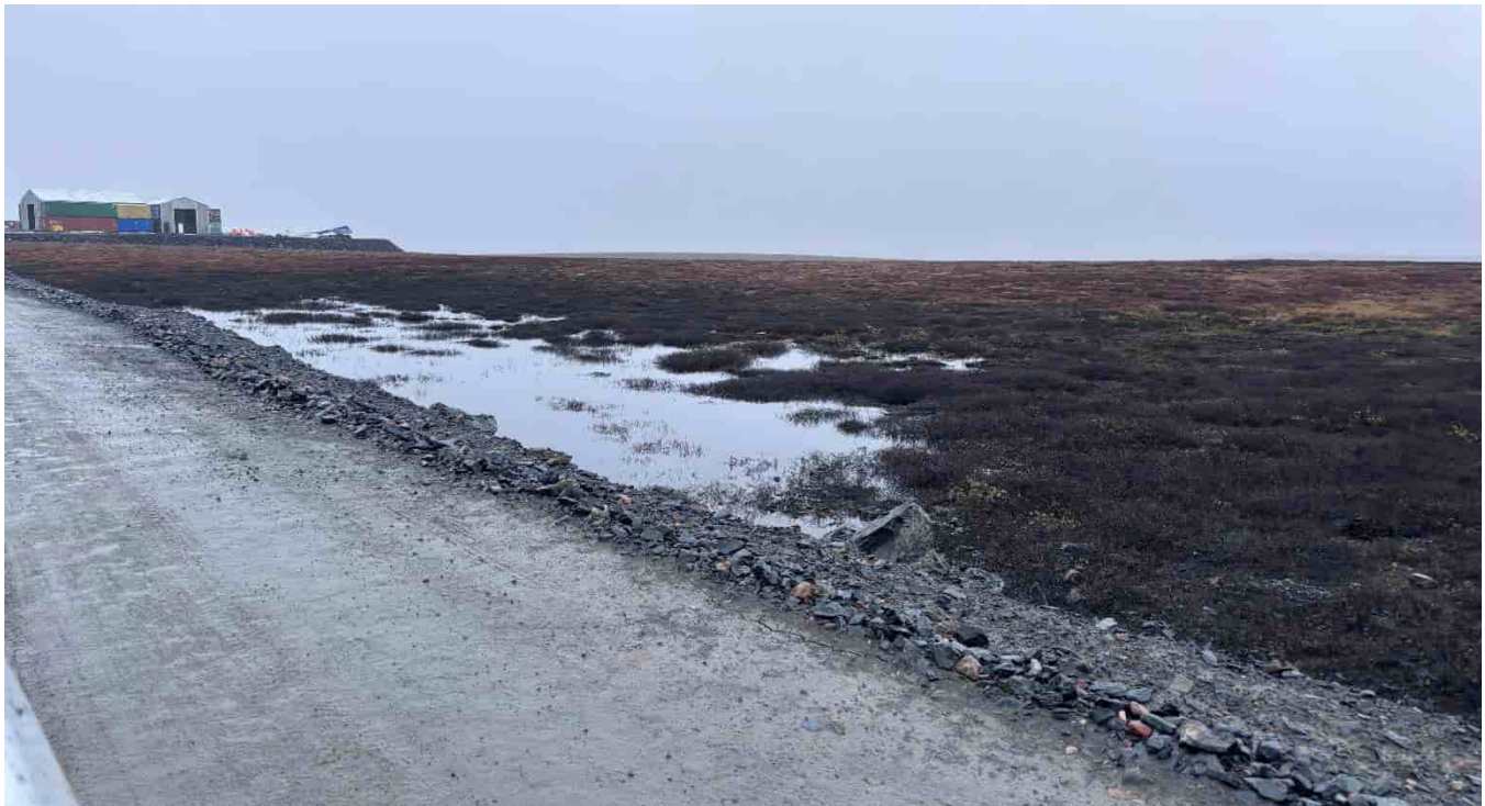
G-427: Ponding beside access road, looking E
