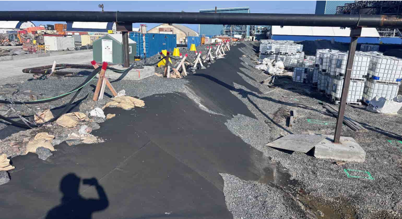
G-351: Western berm, looking N – exposed geotextile and ponding at toe
