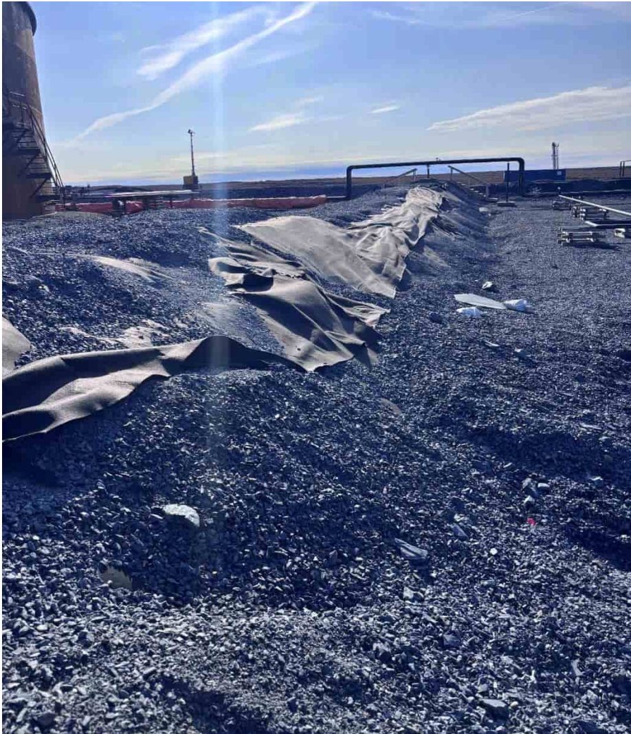
G-359: Exposed geotextile and HDPE liner on slope berm between Tank 2 and Tank 3, looking S
