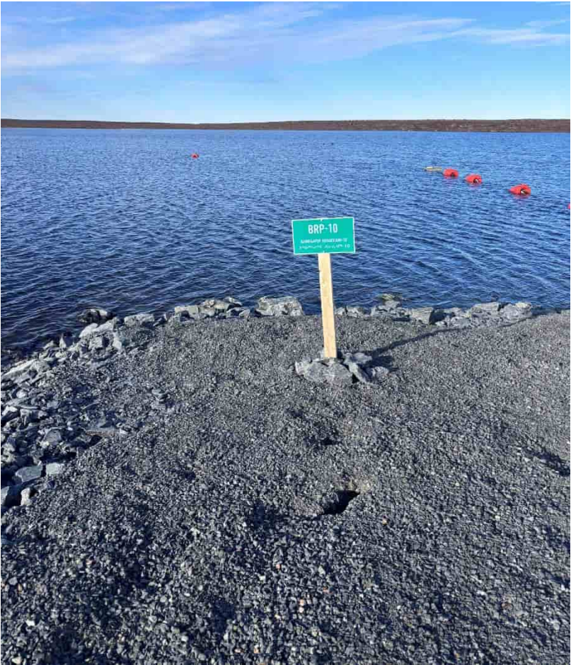
G-478: Sinkholes in the reclaim pipeline access road pad, looking northeast. A series of sinkholes developed due to the placement of surfacing material directly over the ROQ without placement of Transition layer in some areas (ie crush migration into voids in coarser rockfill). Note this area is upstream (not structurally connected) to the main Primary Pond dam structure (so less of a technical concern at this time).
