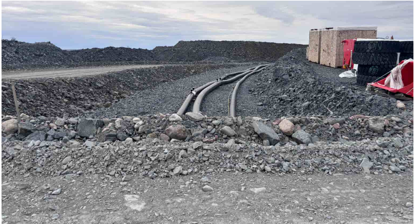
G-515: Tailings pipelines crossing under ROM stockpile eastern access road, looking W
