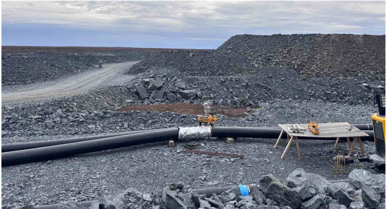
G-511: Tailings pipeline connection, looking SW towards ROM stockpile
