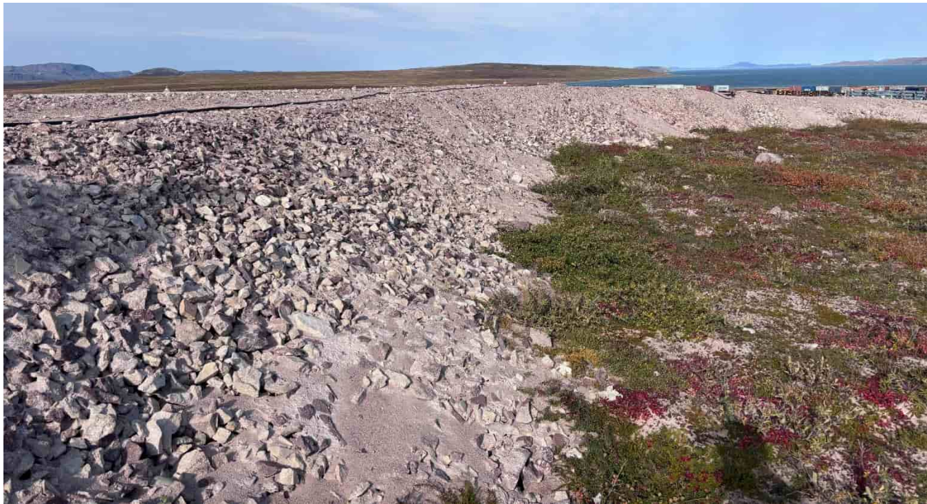
M-71: Airstrip embankment – Note erosion
