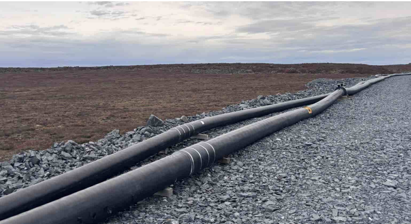
G-518: Tailings pipeline along southern rockfill, looking W
