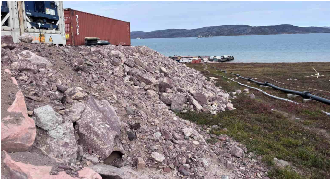
M-54: Eroding slope of camp pad extension, looking NE
