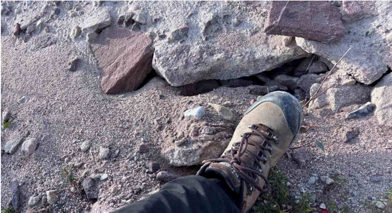
M-2: Voids in pad slope beside airstrip
