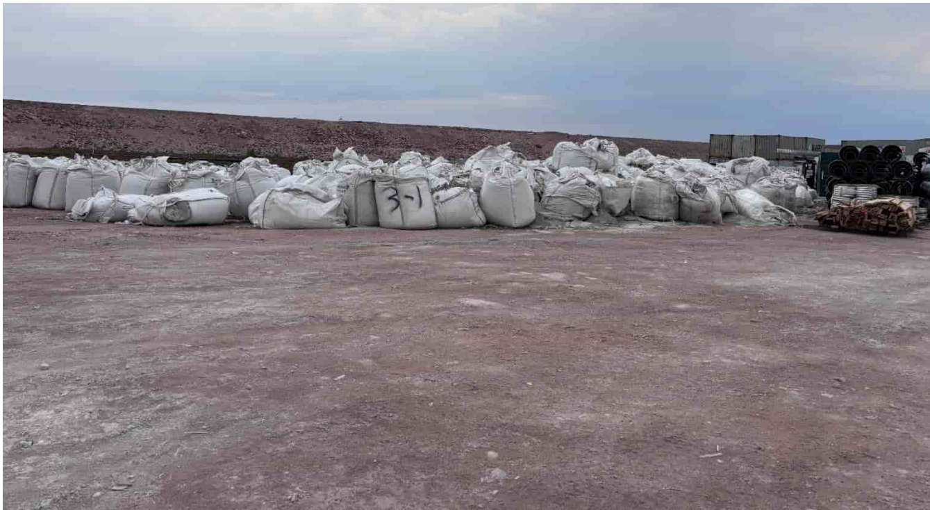
M-34: Broken bags on W side of pad
