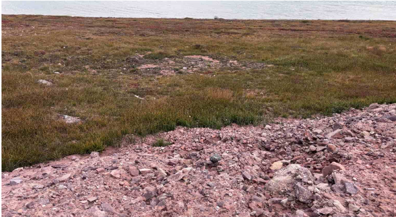
M-25: Erosion channel on NE pad slope
