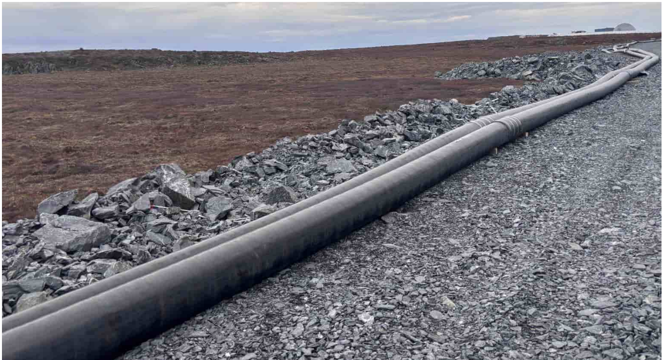
G-517: Tailings pipeline along southern rockfill, looking W
