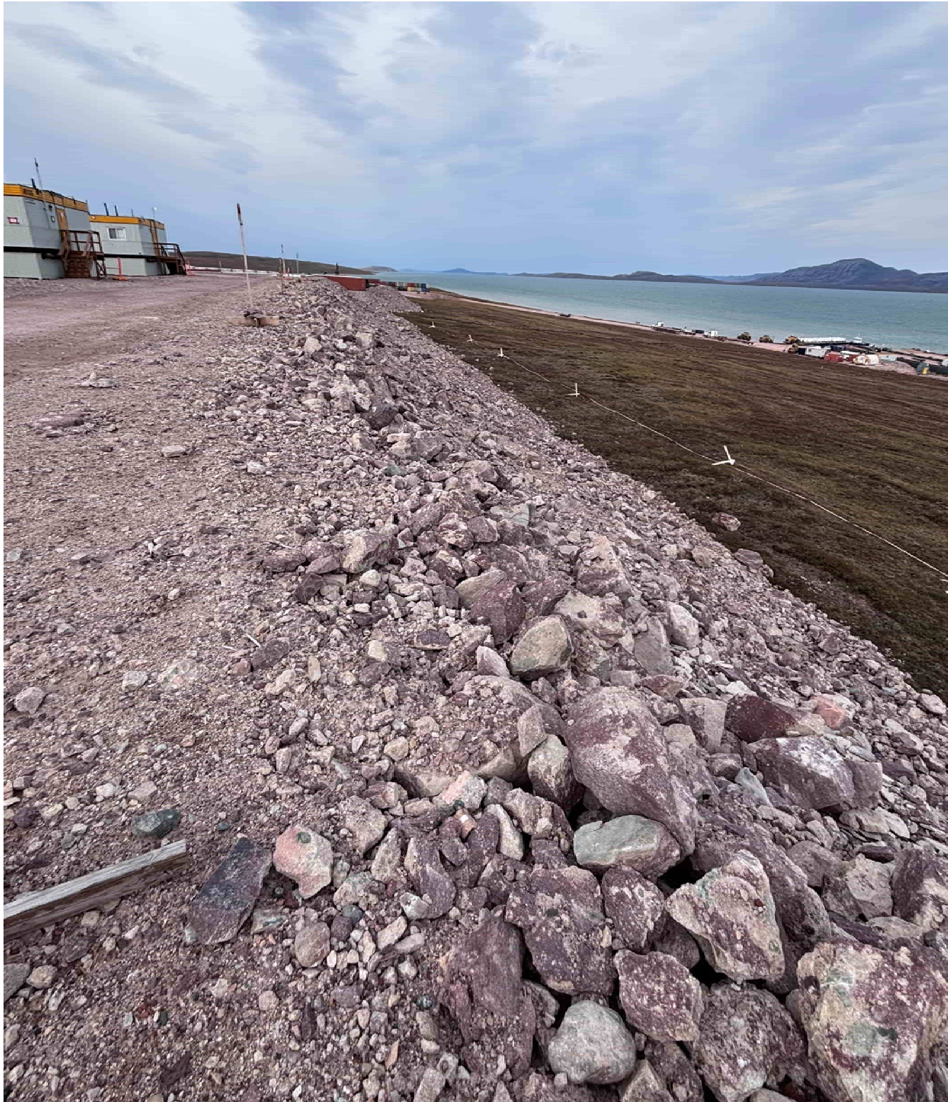
M-61: Eastern pad slope typical condition
