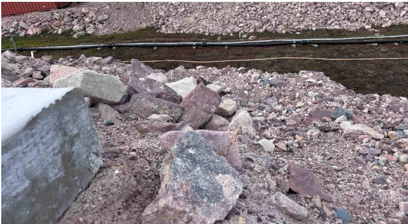
M-58: Camp pad, north corner. Note the NW corner of the concrete slab located too close to the crest of the pad
