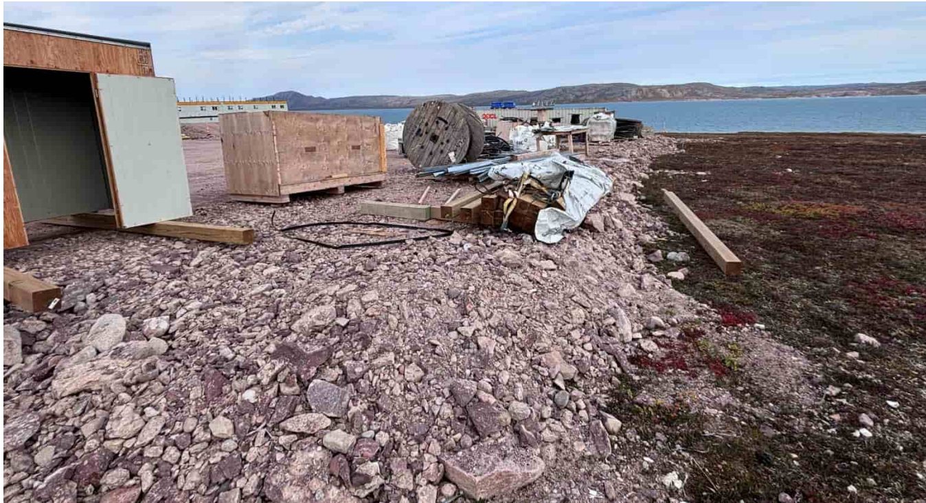
M-45: Southern pad slope – Note oversteepened slope and laydown beside edge of pad
