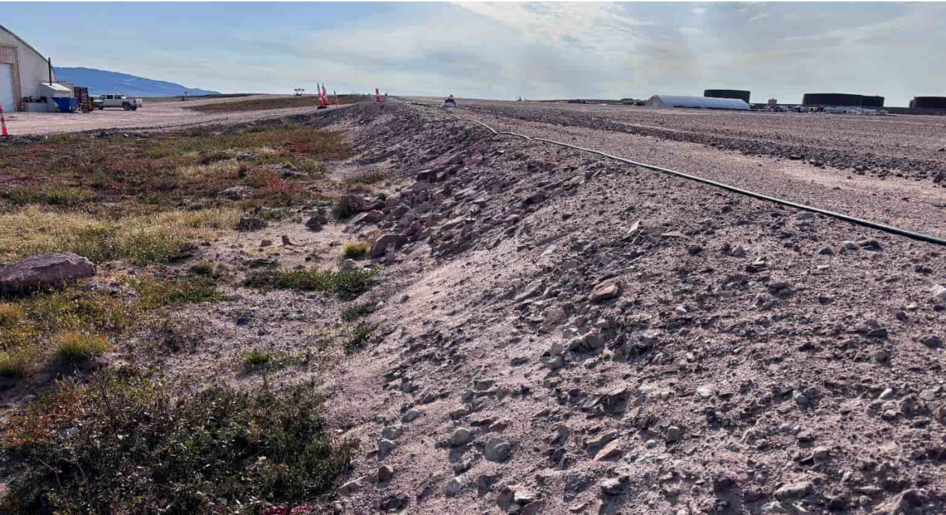
M-66: Airstrip embankment, looking SE – Note erosion
