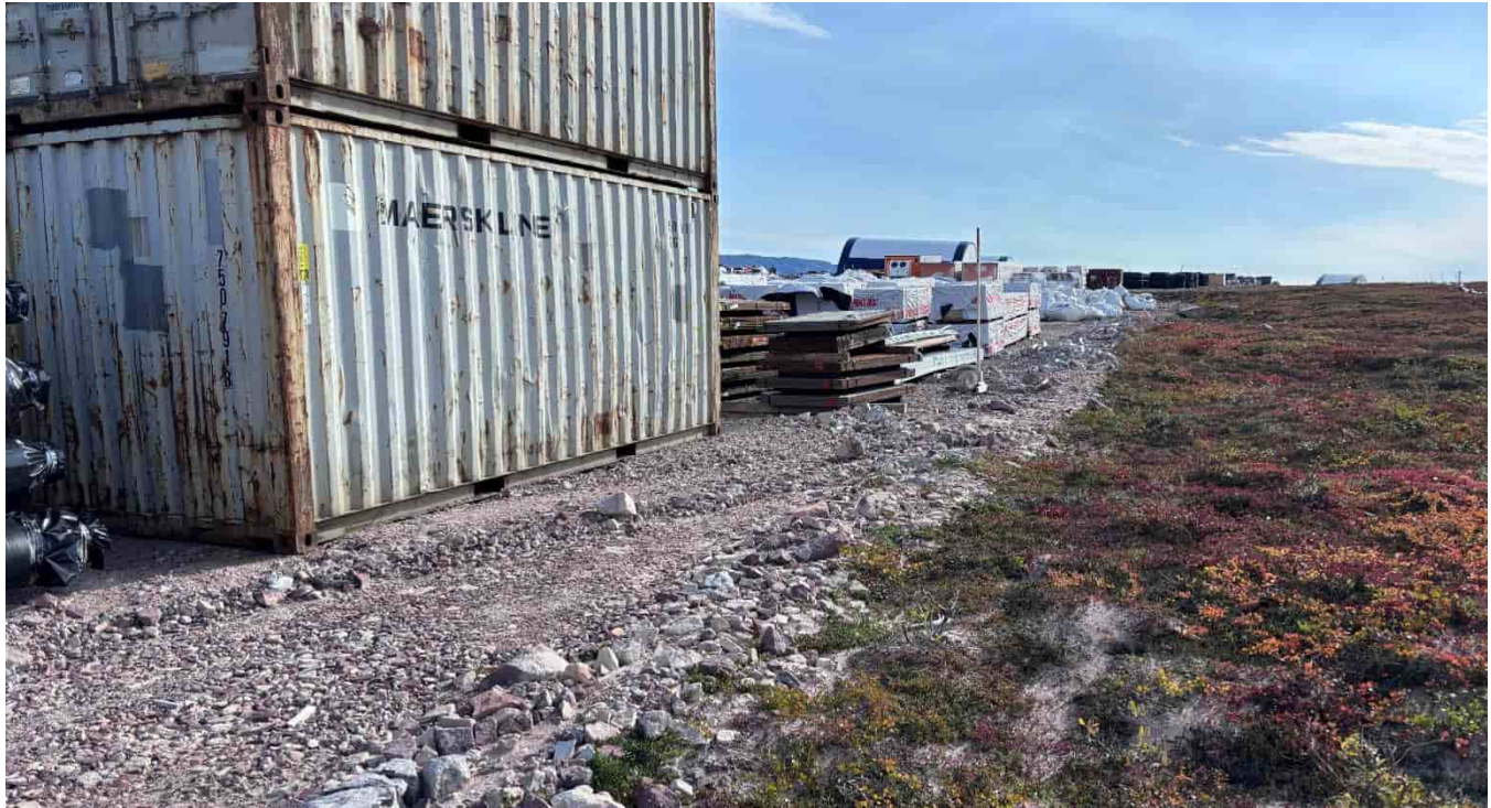
M-5: Laydown area beside airstrip – Note thickness of pad is too thin
