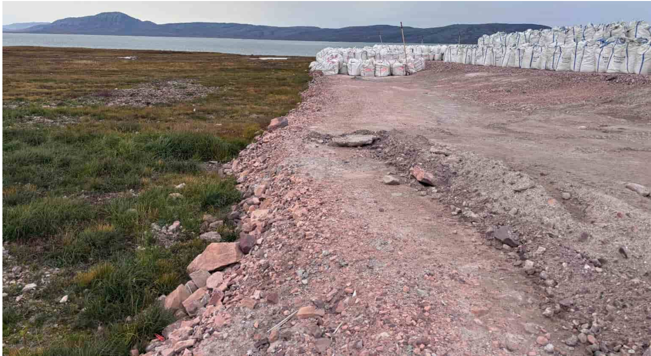
M-32: Damage to pad on northern side
