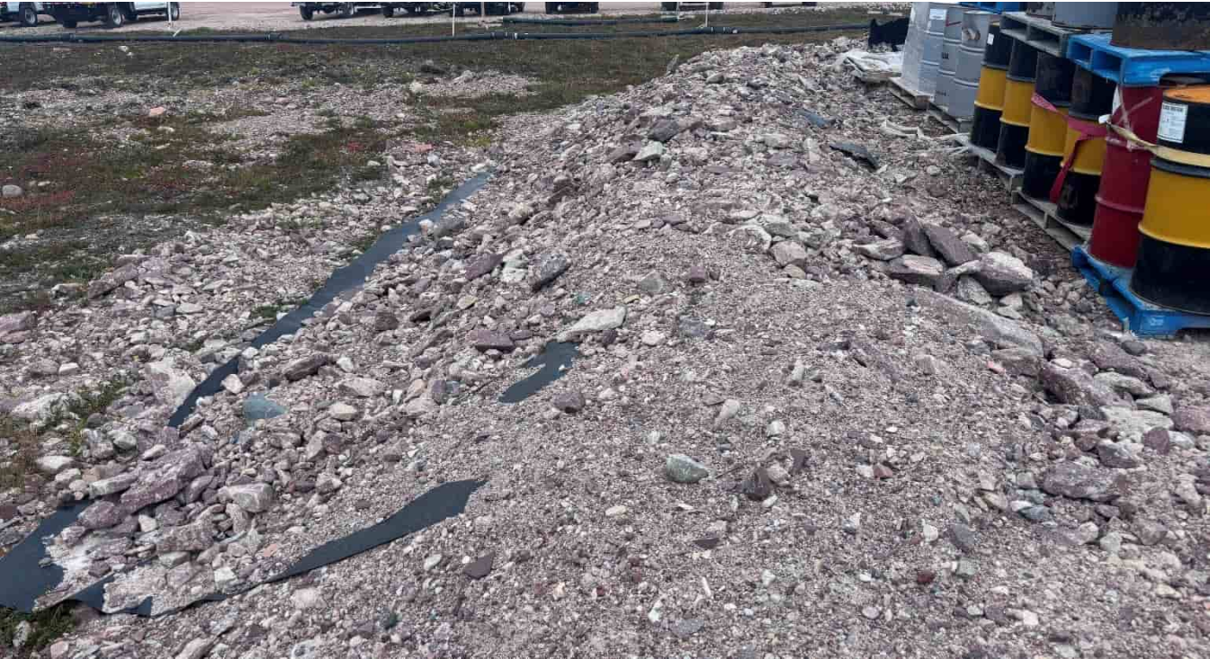
M-43: Exposed liner in pad slope beside fuel storage
