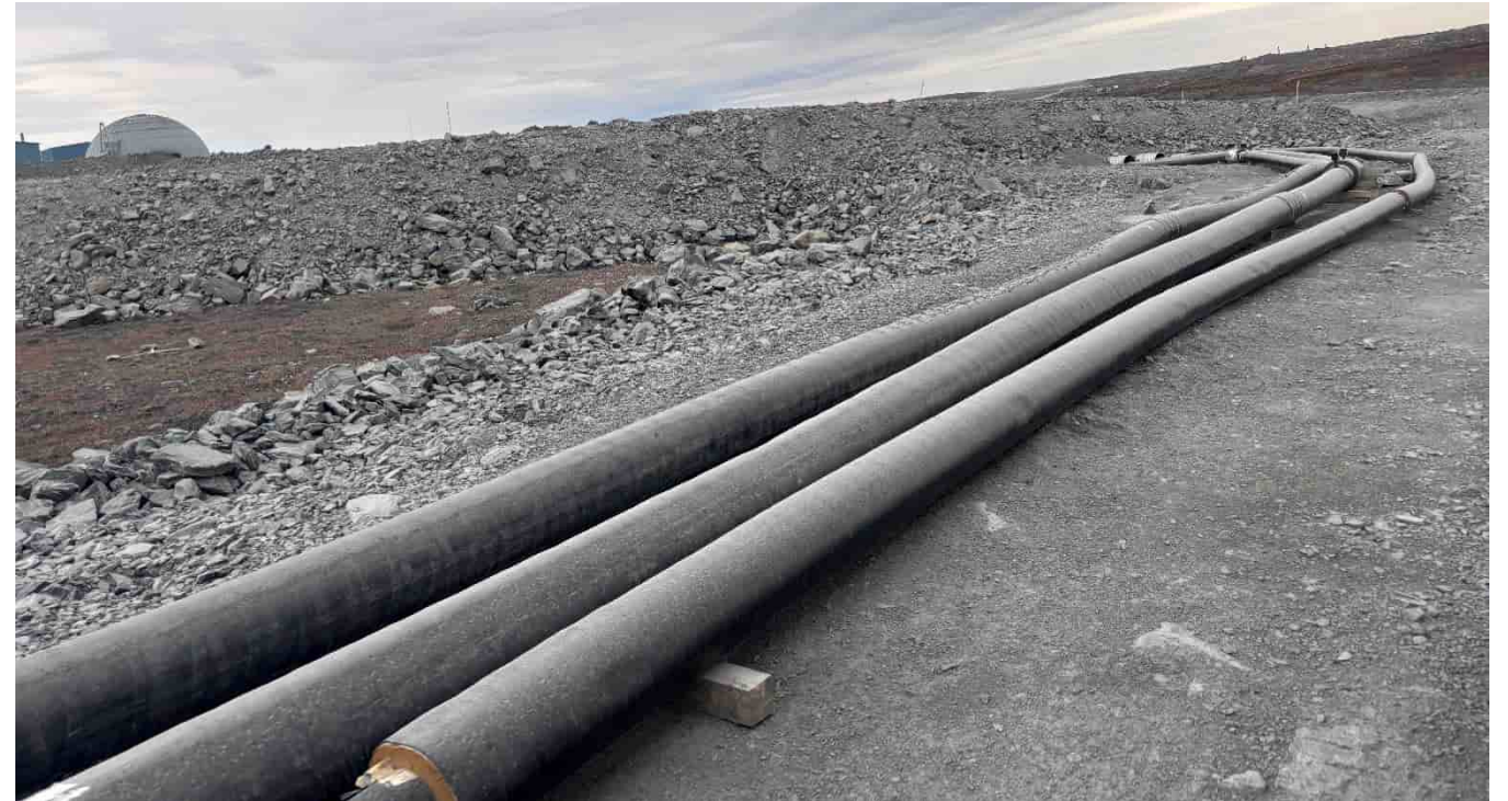
G-508: Tailings pipelines, looking NW
