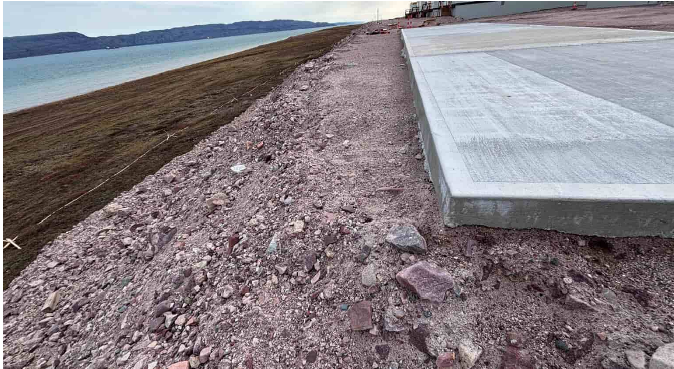
M-56: Erosion under concrete pad at N corner of camp pad, looking E
