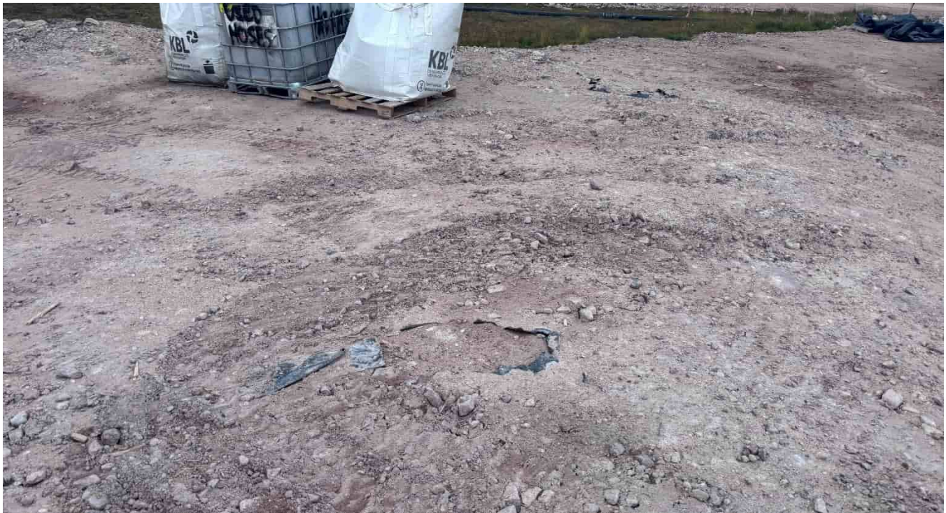
M-44: Temporary fuel storage - Damaged liner
