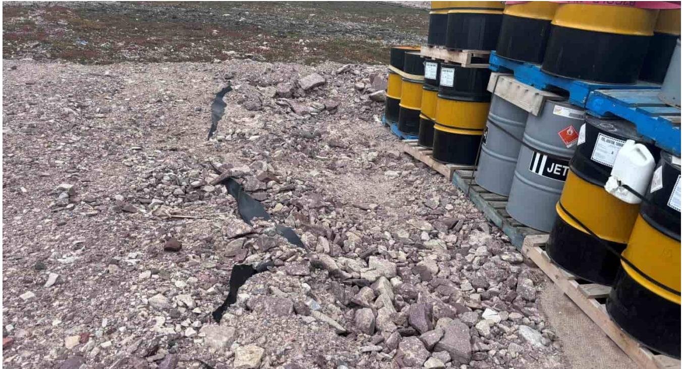
M-42: Temporary fuel storage – Note exposed liner
