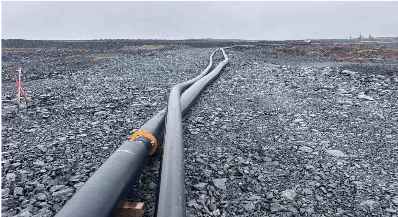
G-488: Typical water reclaim pipeline layout, looking SE
