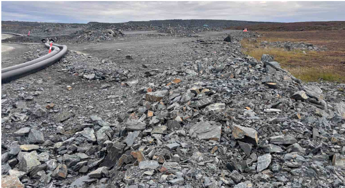
G-521: Tailings pipeline crossing under Water Treatment Plant access road, looking SE
