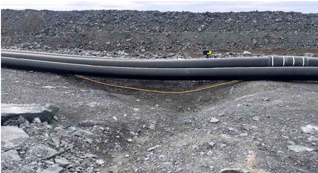
G-509: Depression in tailings pipeline road, piping suspended in smaller sections
