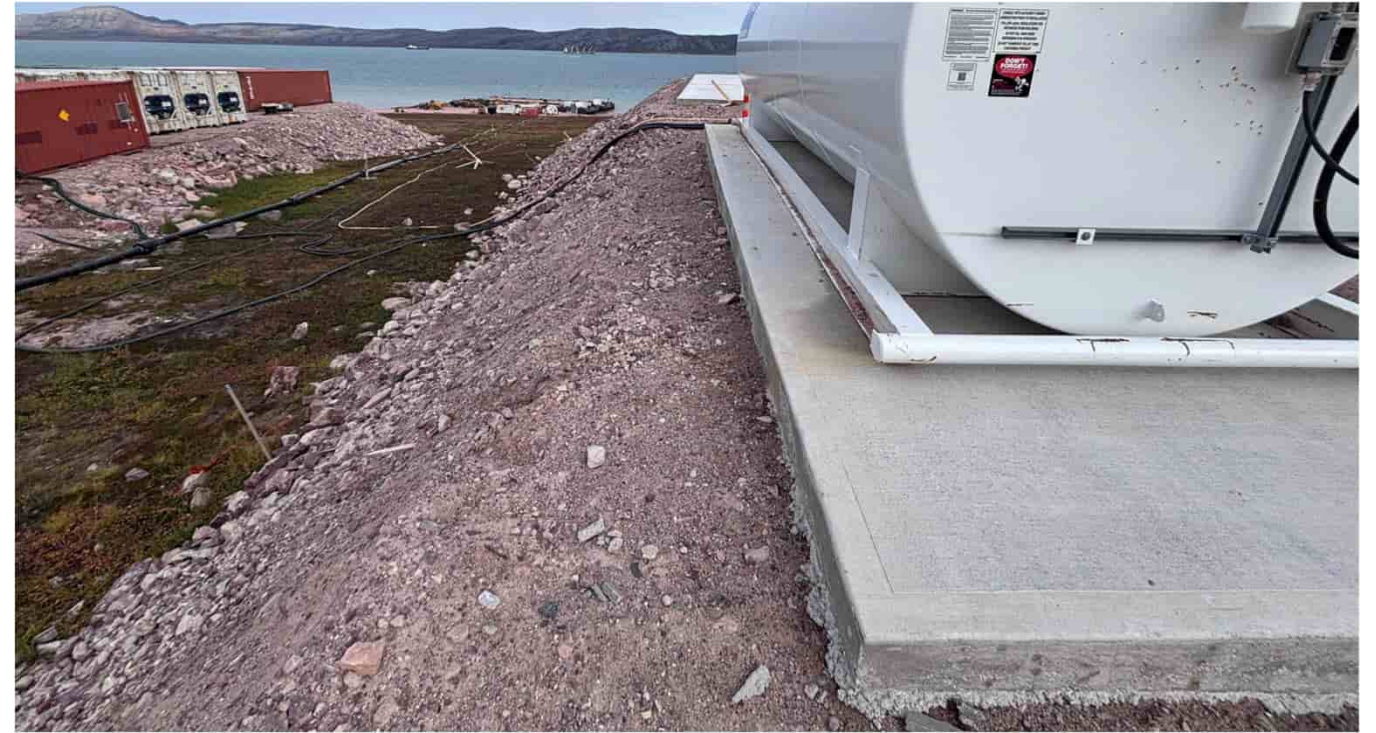
M-57: Concrete slab is located <1m from the crest of the pad, looking N
