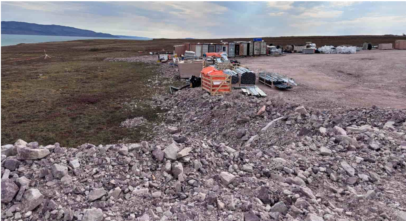
M-62: Undefined edge of slope beside laydown at SE corner of pad
