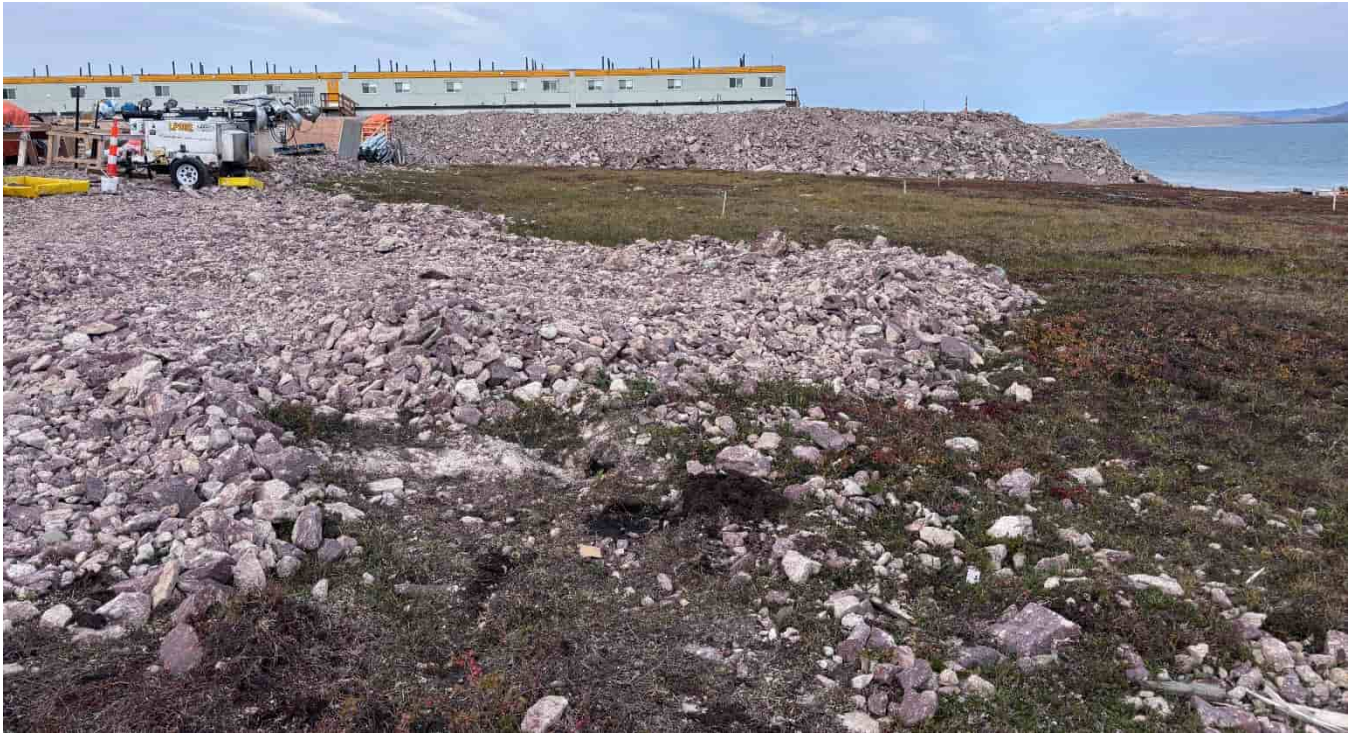
M-46: Undefined edge of pad at SE corner
