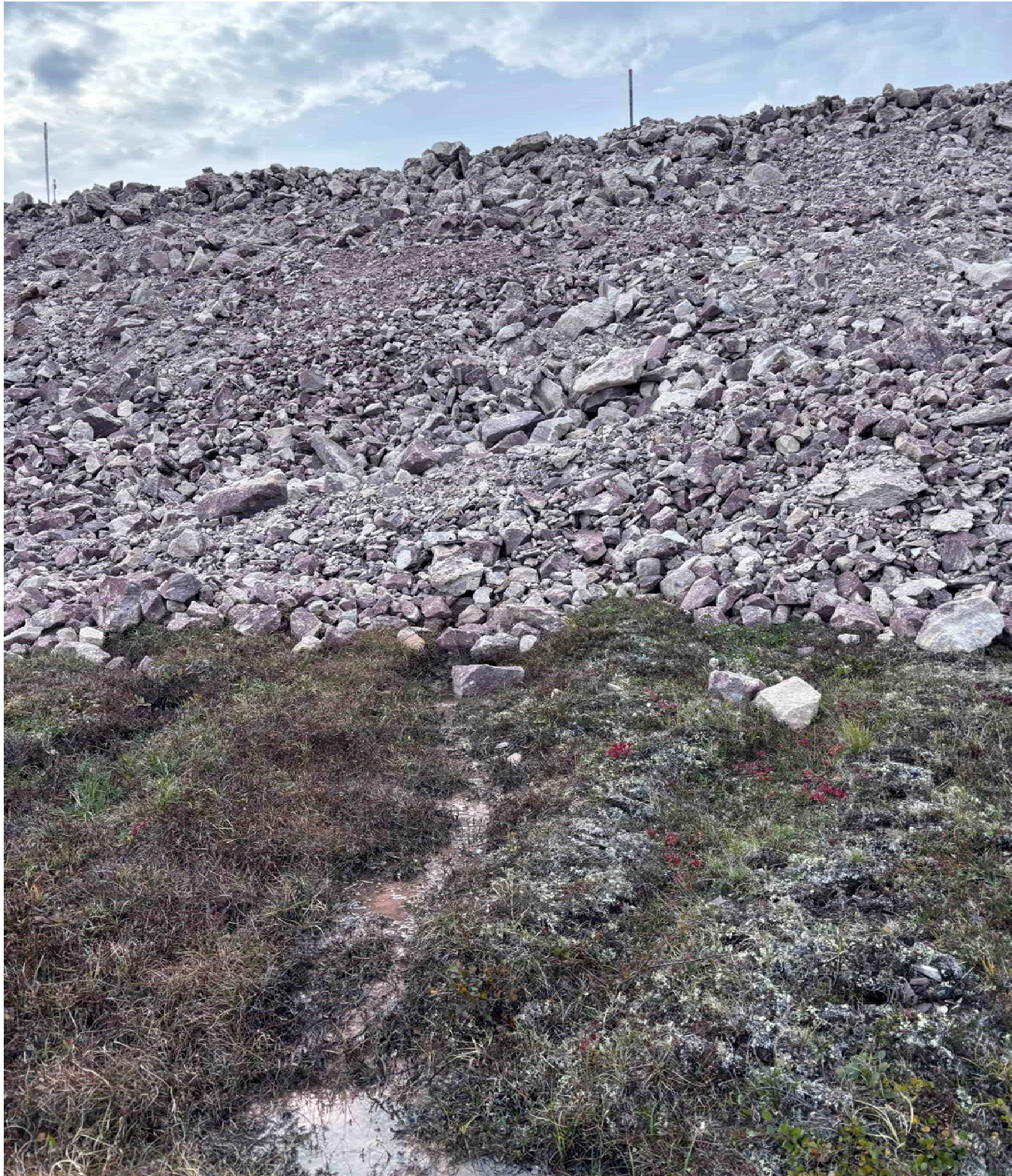
M-50: Water seepage from eastern pad slope
