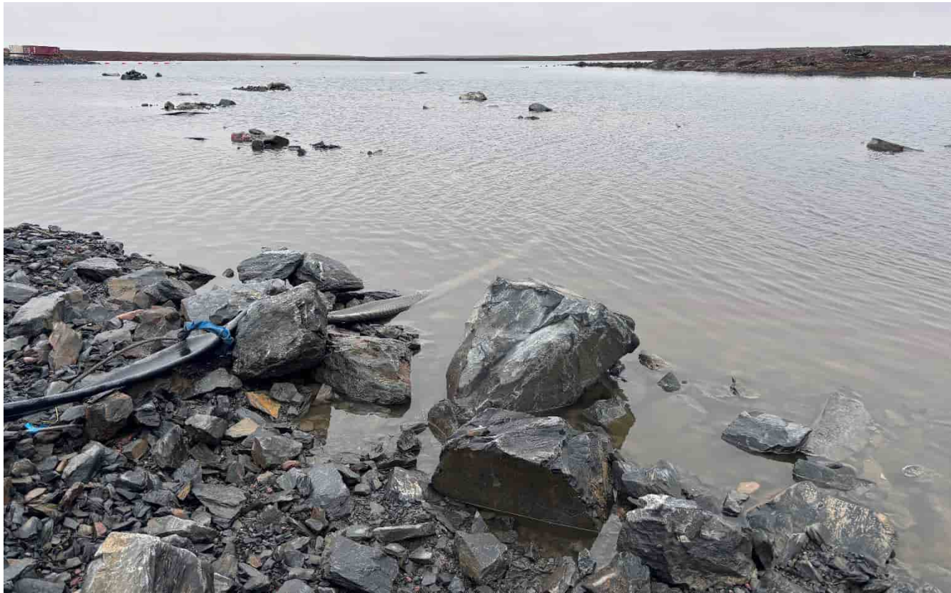
G-484: Pipeline entering water at southern end of pond
