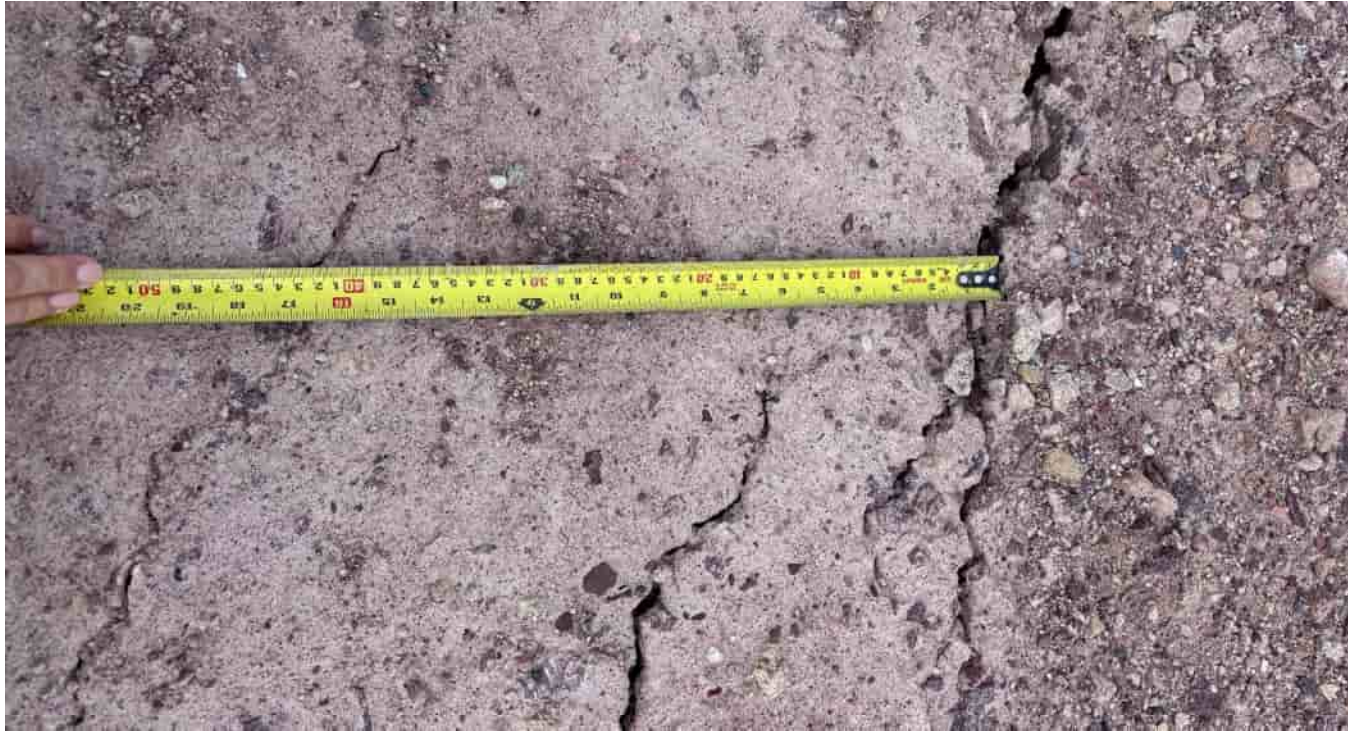
M-101: Tension cracks in airstrip surface
