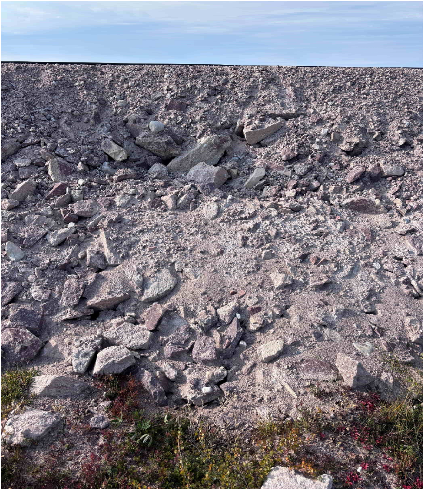
M-74: Eastern airstrip embankment erosion
