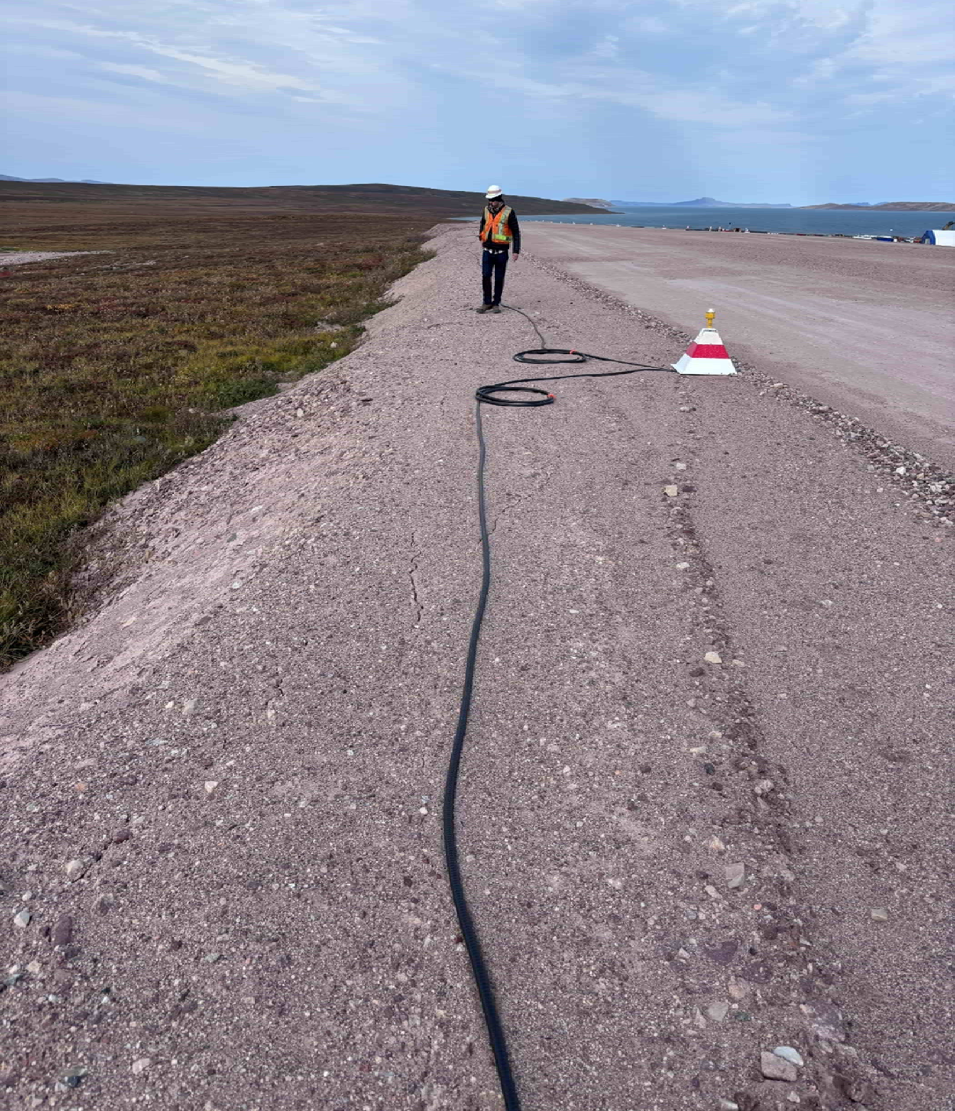
M-91: Tension cracks in western embankment
