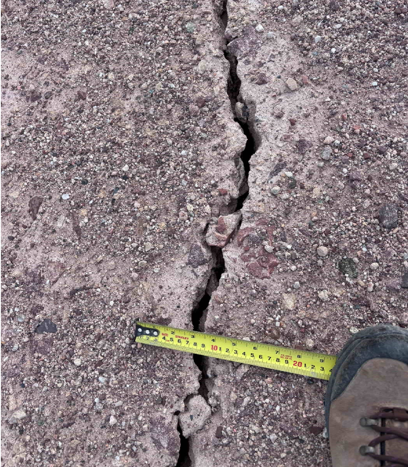
M-100: Typical tension crack width
