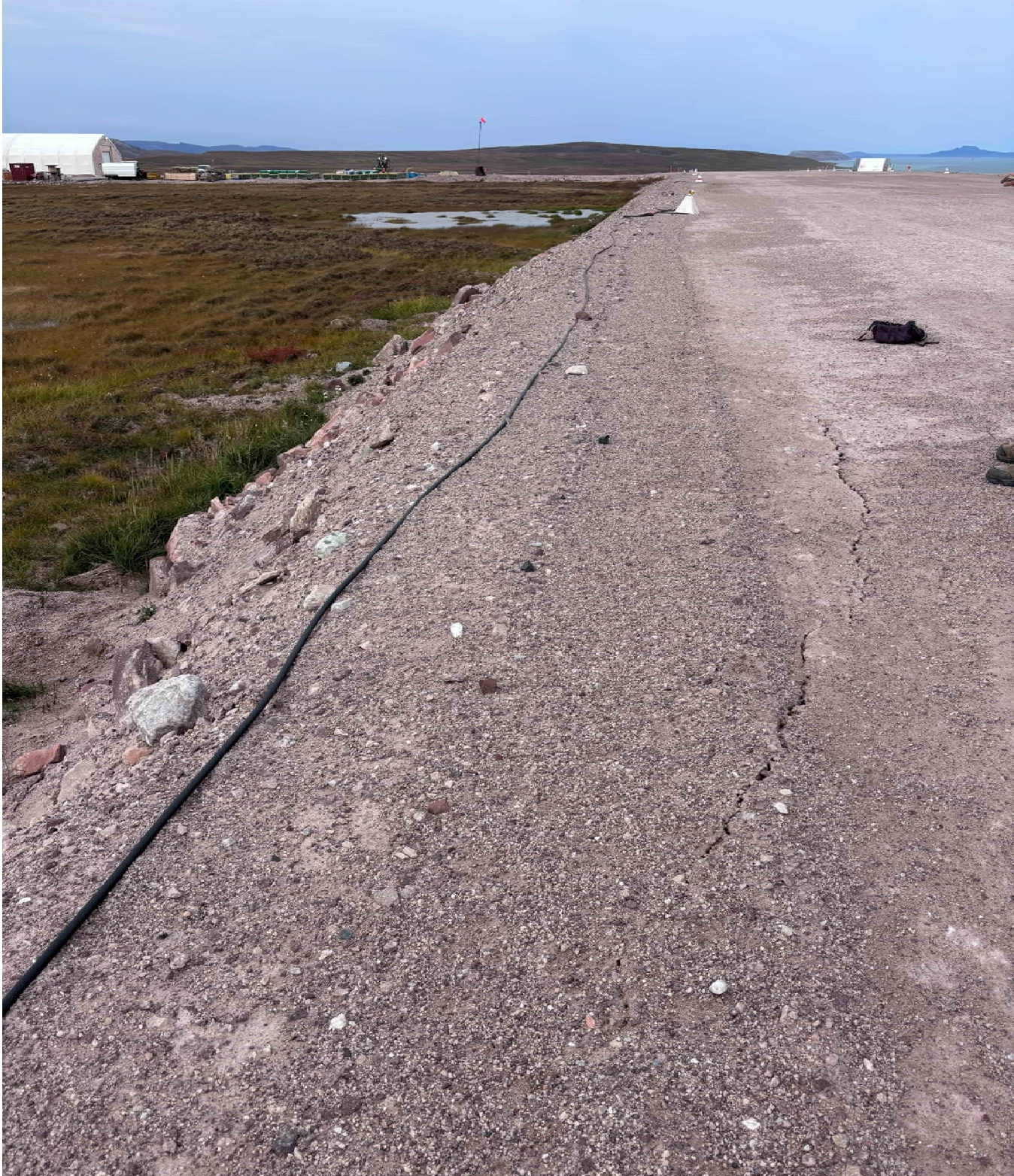
M-103: Tension cracks in airstrip surface, looking NW
