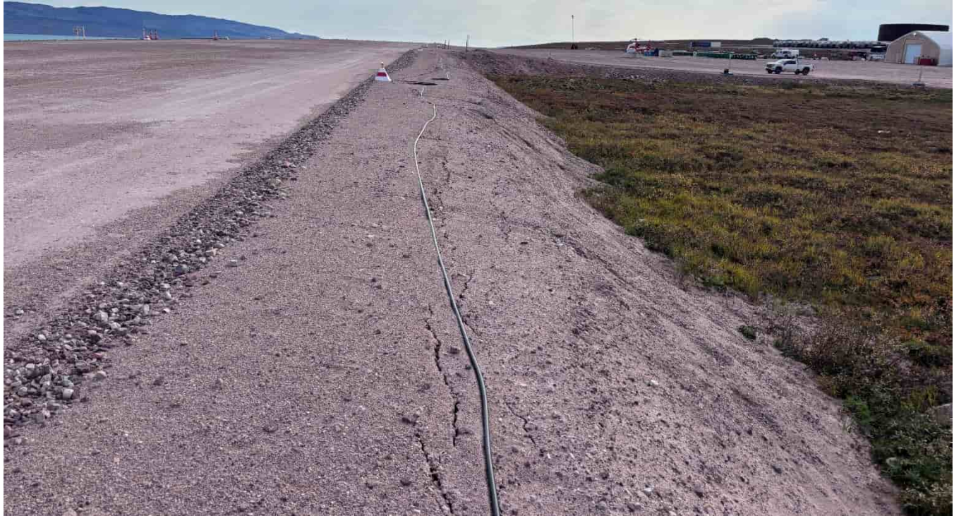
M-89: Tension cracks in western embankment
