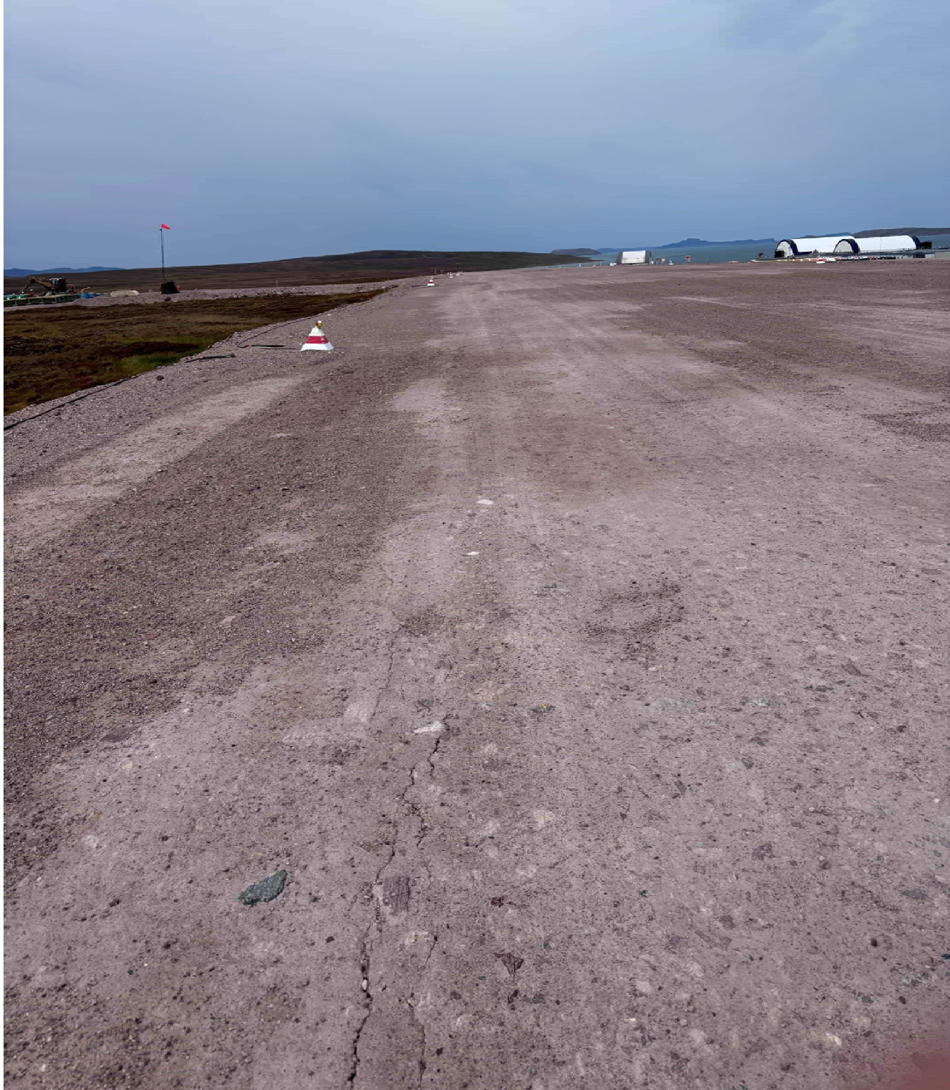
M-99: Tension cracks in airstrip surface, looking NW
