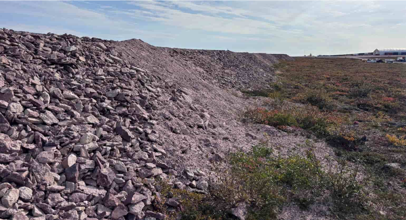
M-88: Western airstrip embankment, looking SE – Note erosion
