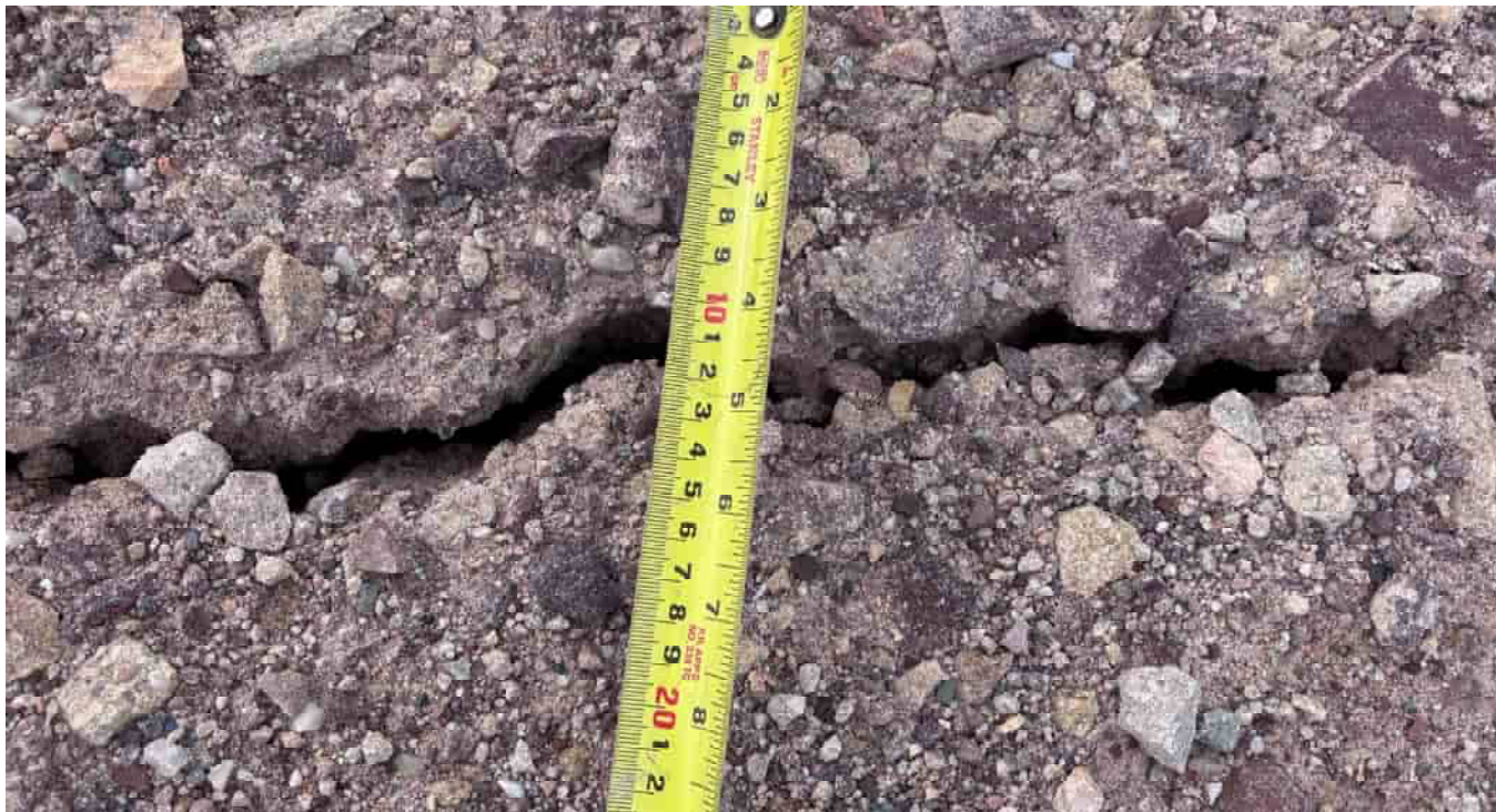
M-102: Tension crack in airstrip surface
