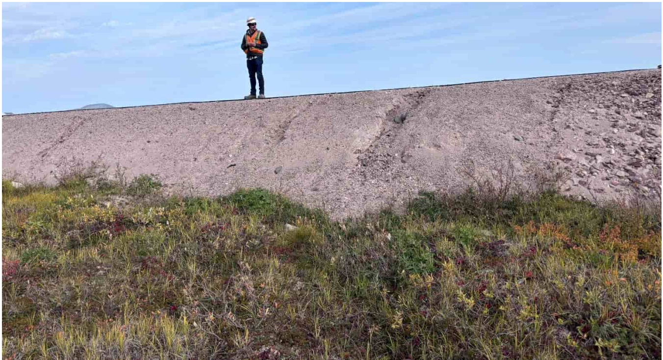
M-90: Erosion pathways in western embankment
