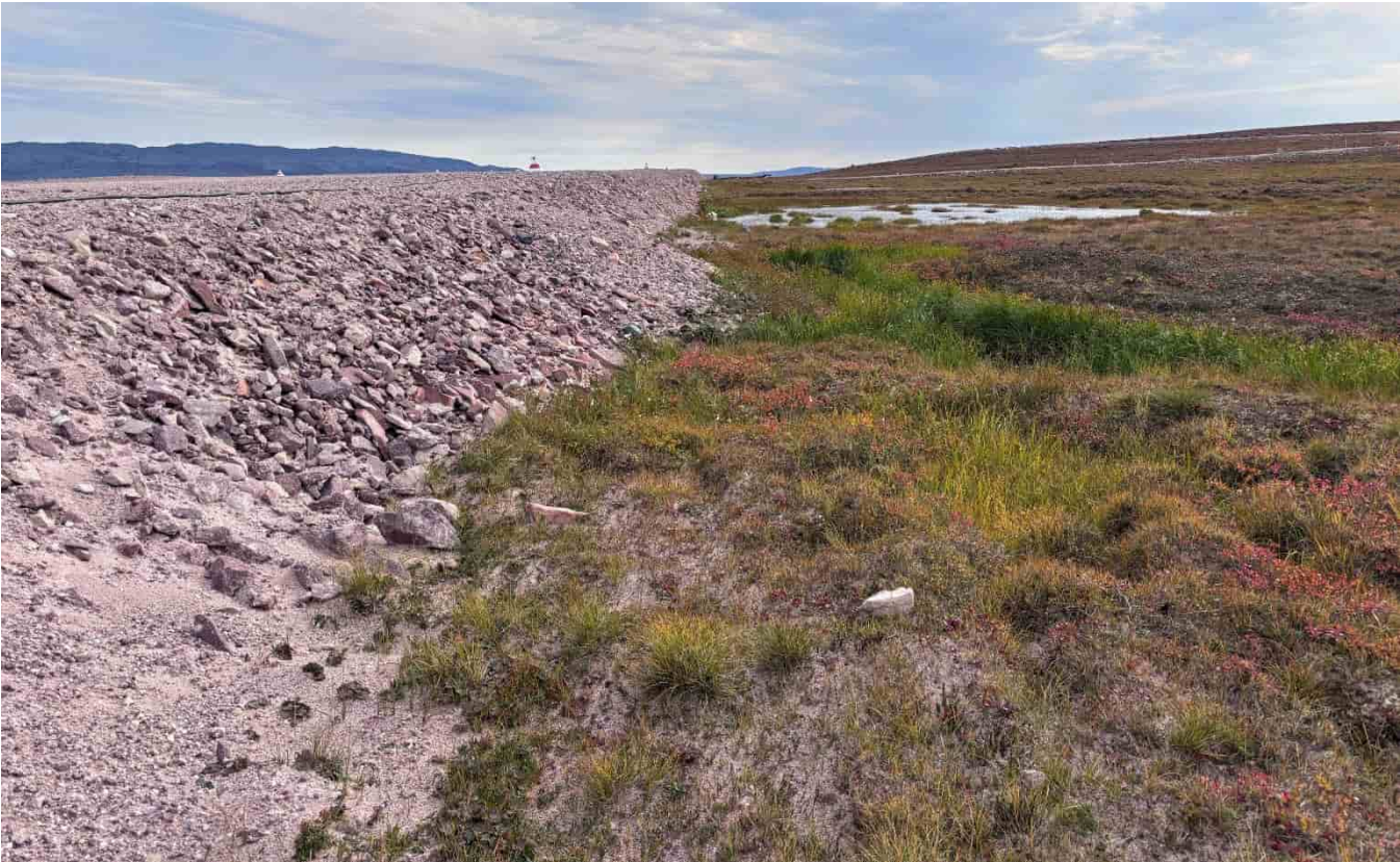
M-97: Western airstrip embankment, looking SE – Note ponding water
