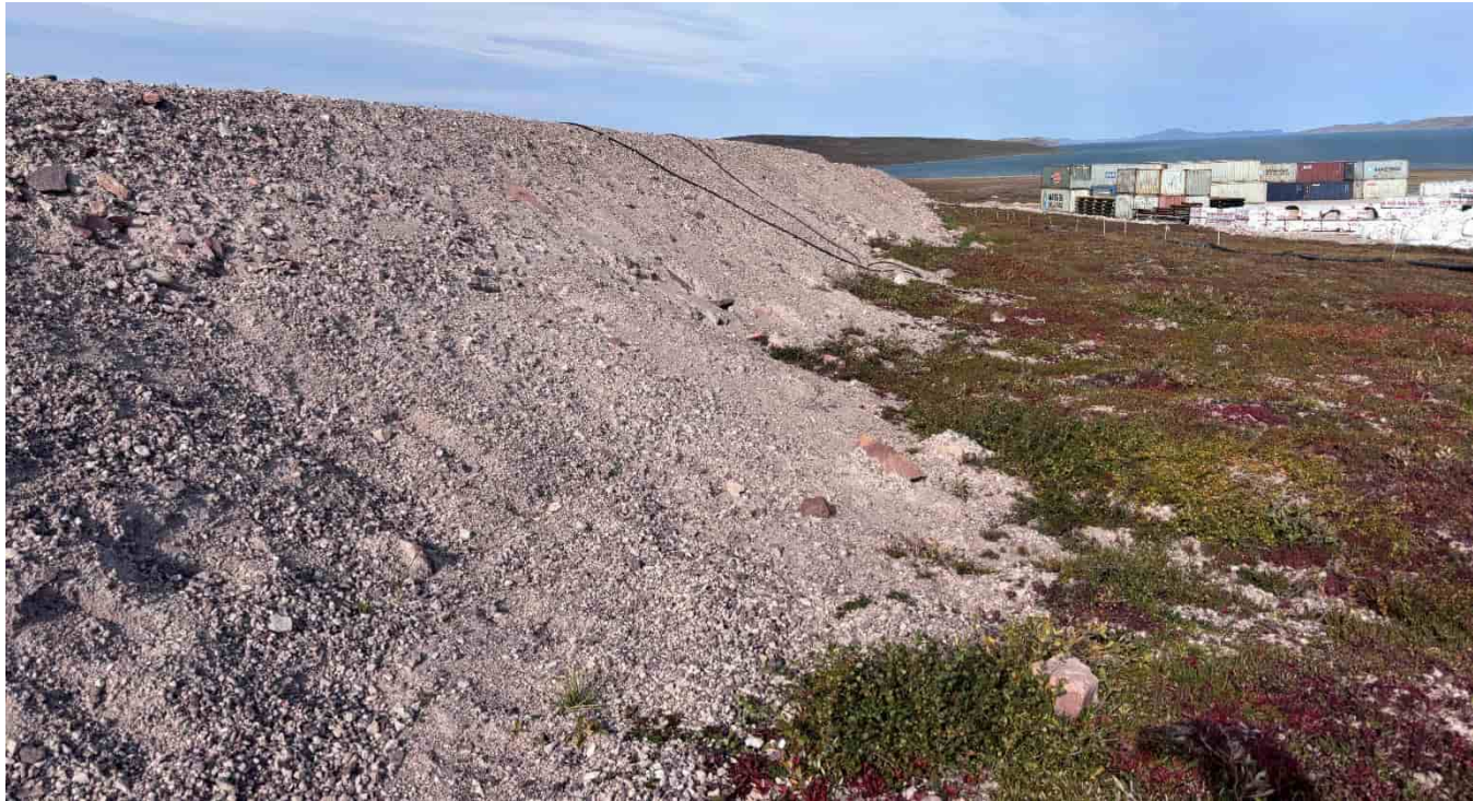
M-75: Eastern airstrip embankment erosion
