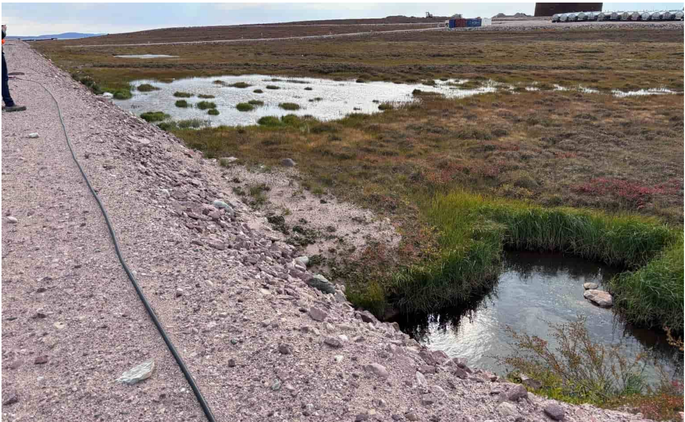
M-98: Ponding water below western airstrip embankment
