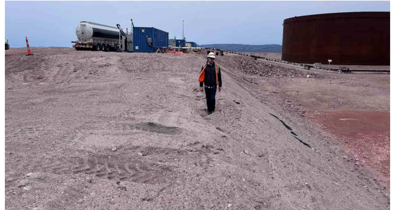
M-154: Sluffing of the fill material at SW corner of tank farm
