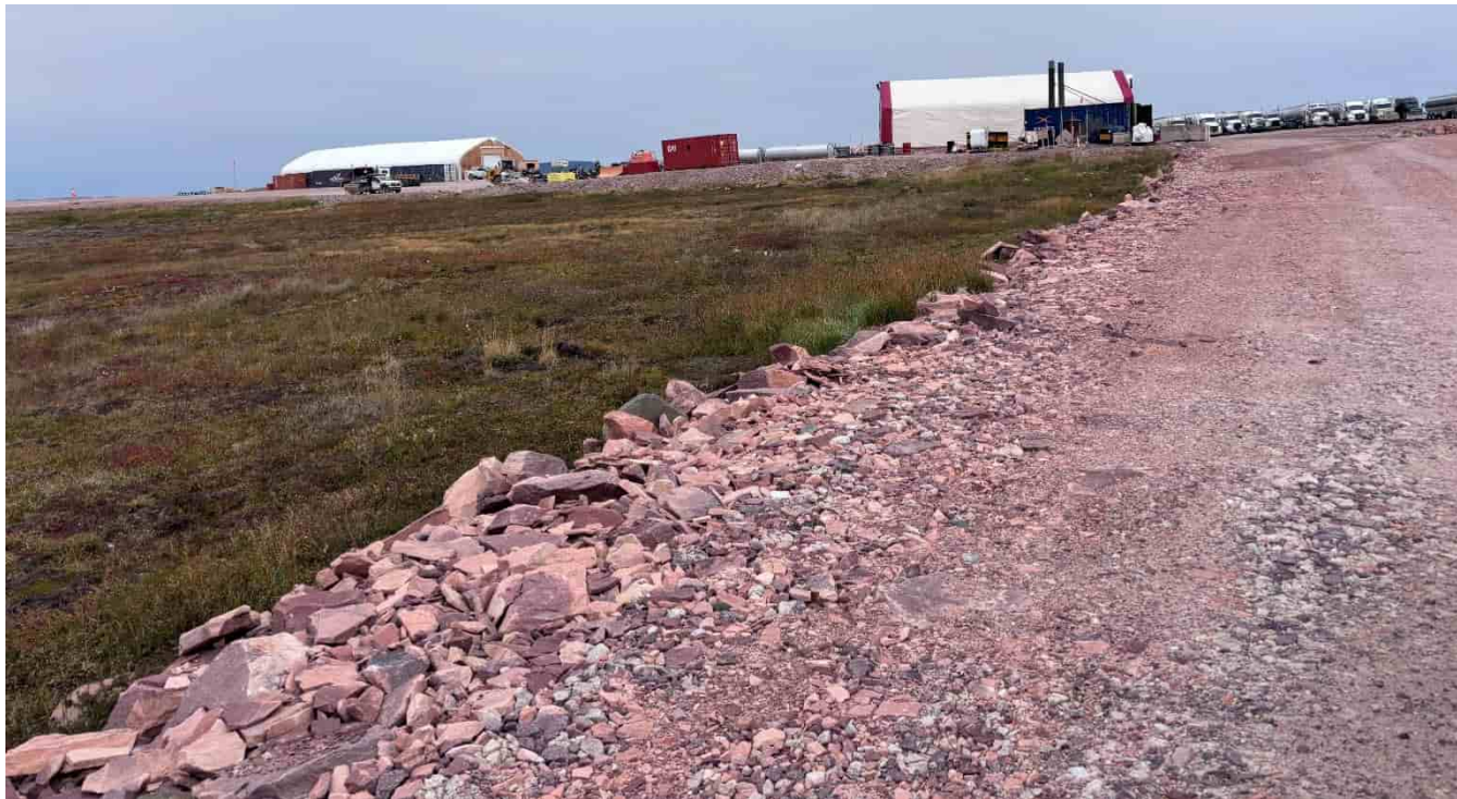
M-128: Former explosives storage access road, looking SE – Note fill is too thin
