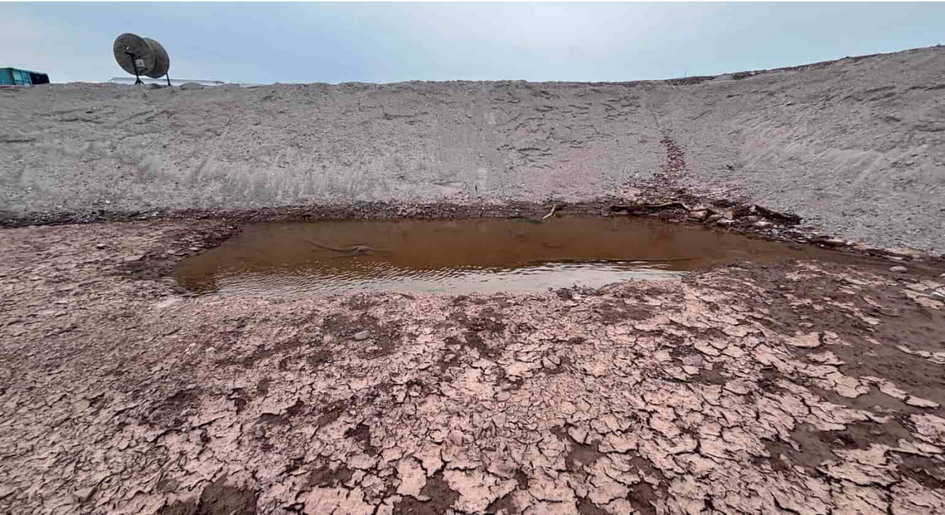
M-146: Ponding water at NW corner of tank farm
