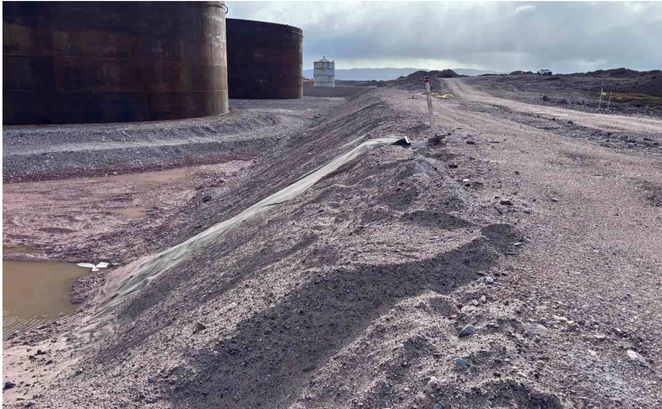
M-175: Ponding water below southern berm, looking E
