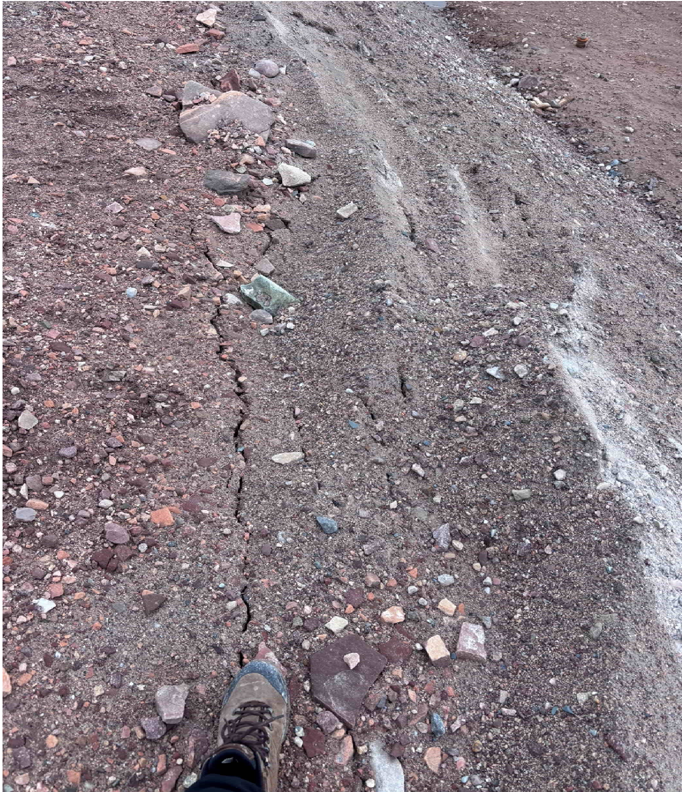
M-179: Tension cracks - crest of western berm
