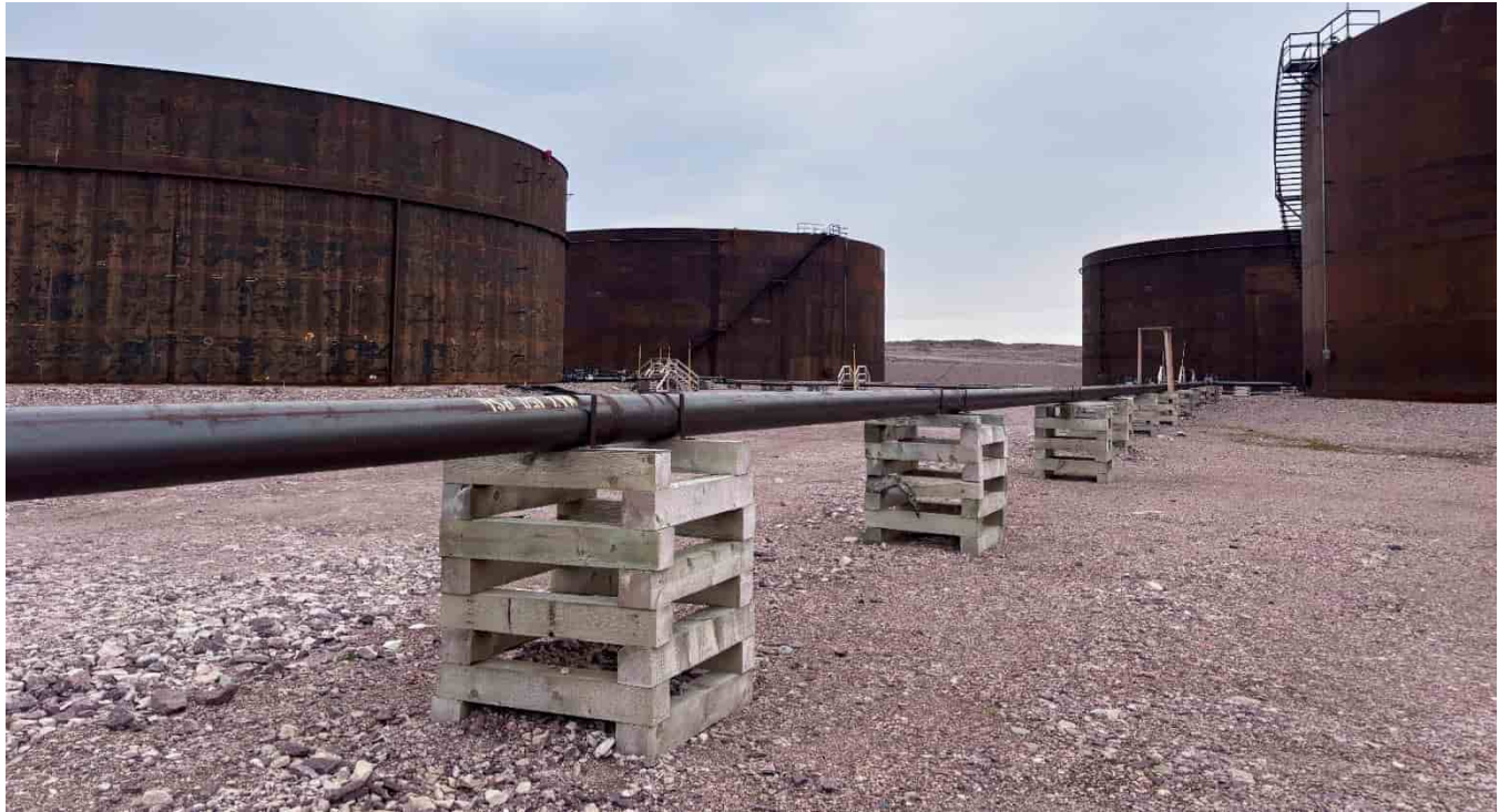
M-145: Typical pipe supports in tank farm
