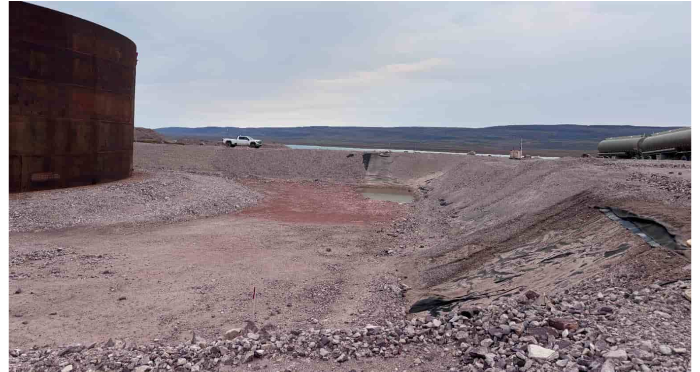
M-150: Western berm, looking S – Note exposed liner
