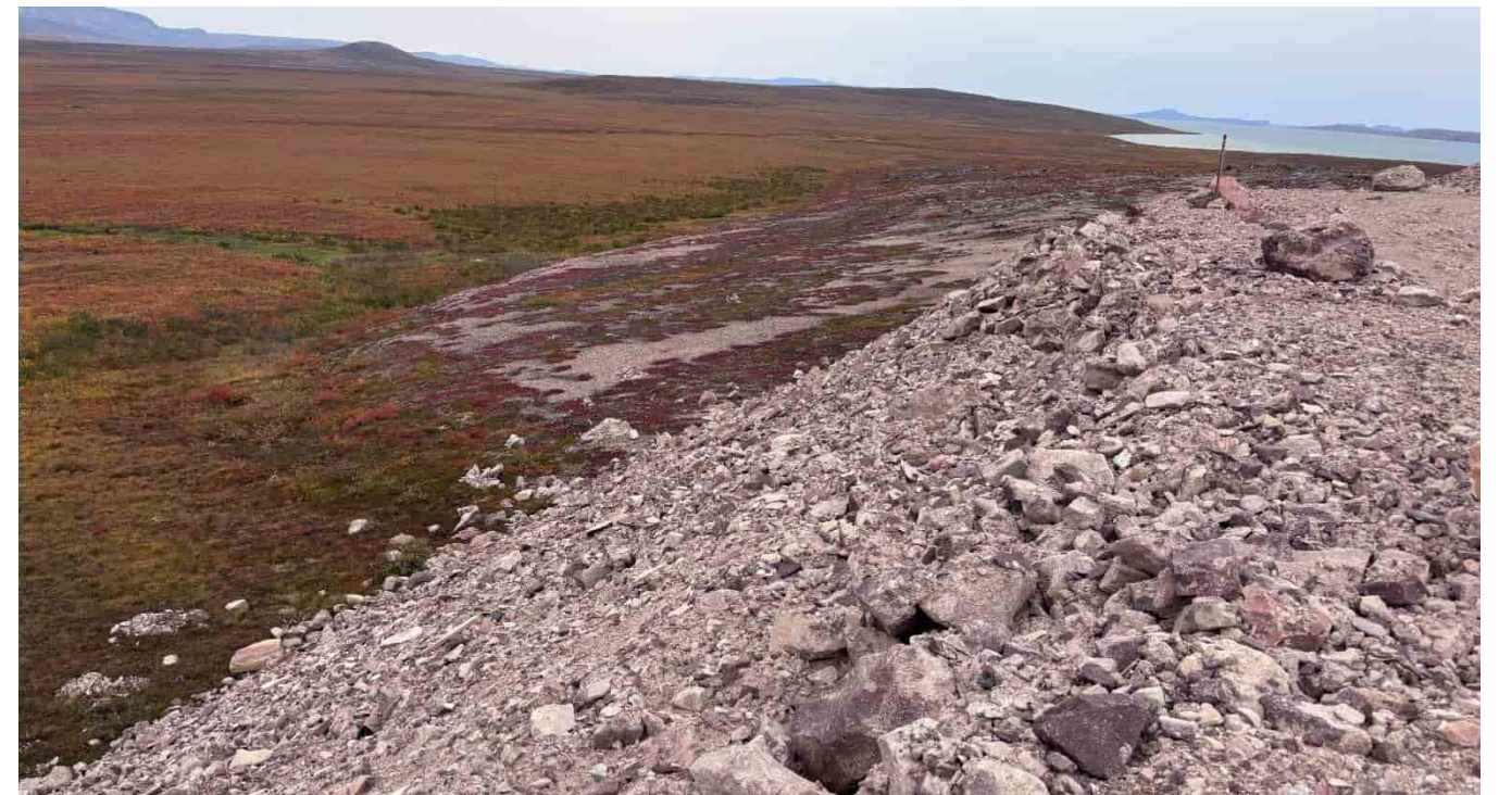
M-156: Tank farm pad slope at SW corner – Note oversteepened slope
