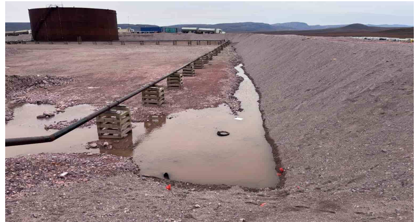
M-140: Ponding water along toe of berm at NE corner of tank farm
