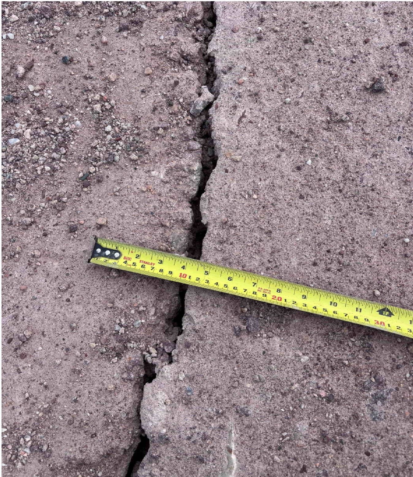
M-104: Tension crack in airstrip surface
