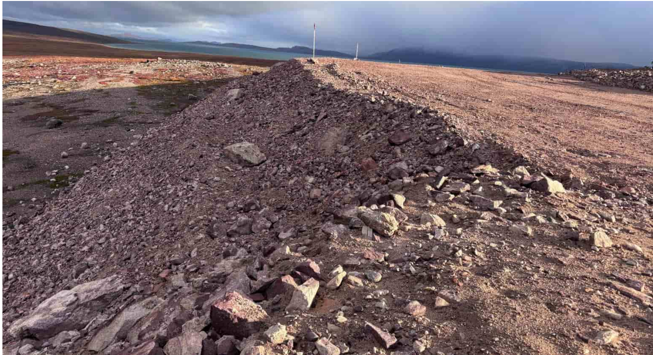
M-167: Oversteepened road embankment, looking N
