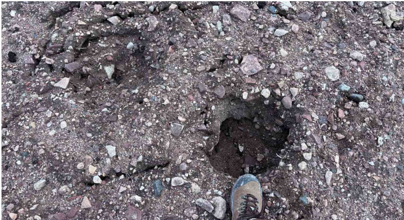
M-169: Sinkhole in southern berm
