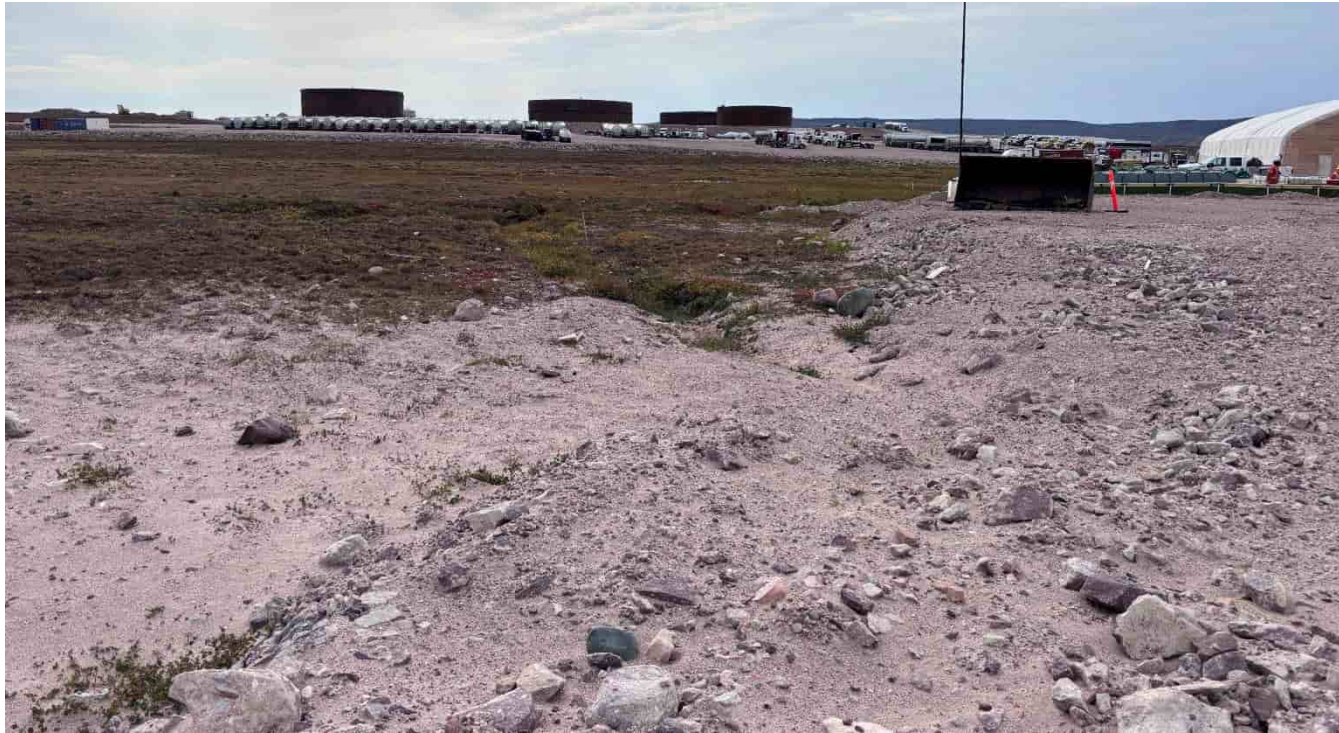
M-126: Undefined S edge of pad between airstrip and tank farm
