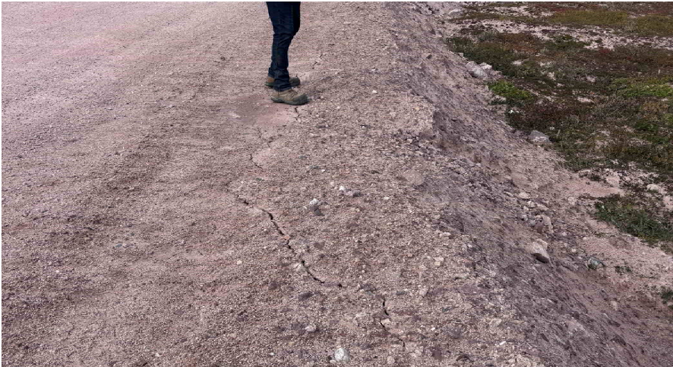
M-114: Tension crack in access road embankment, looking NW
