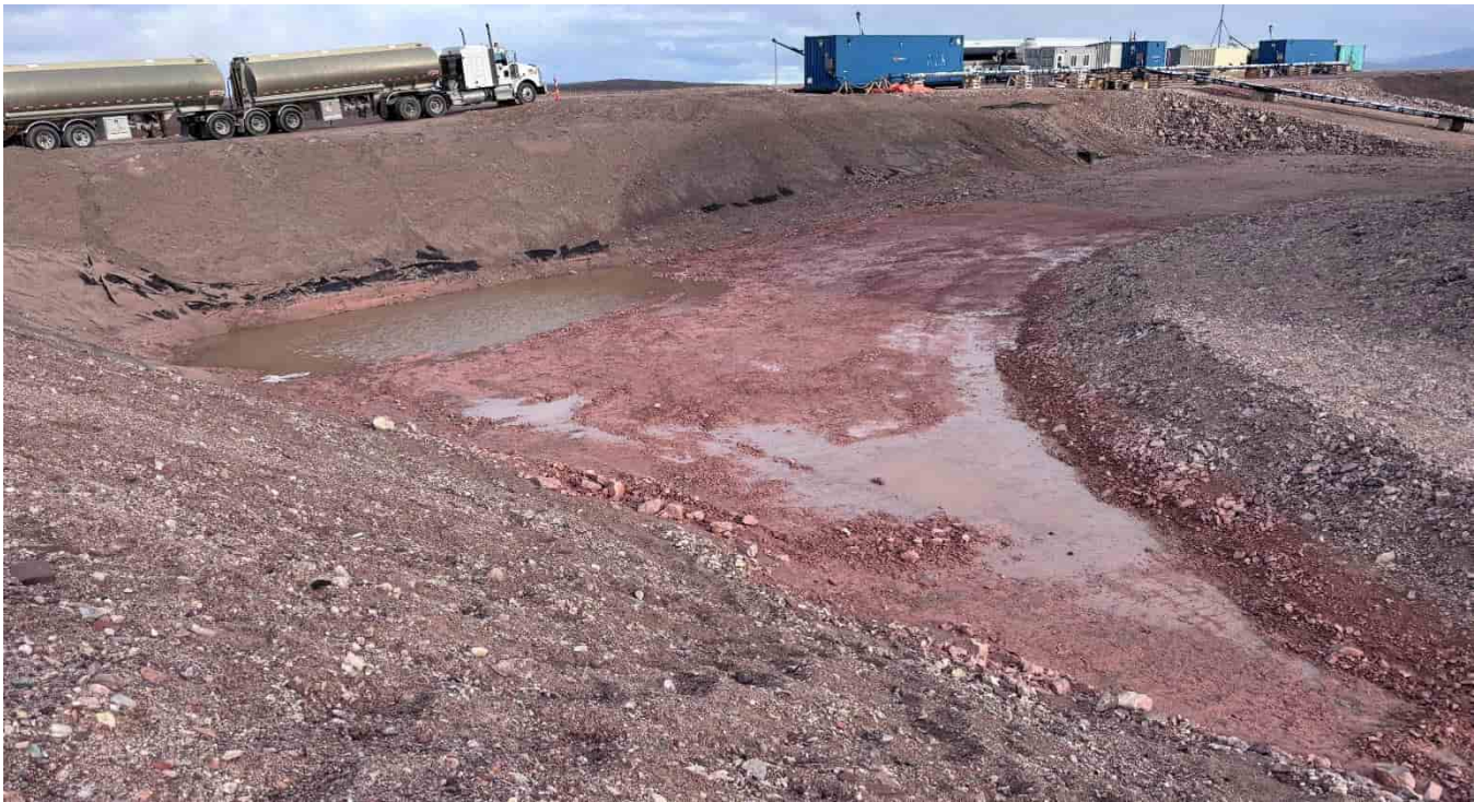
M-174: Ponding water and exposed liner below fireball
