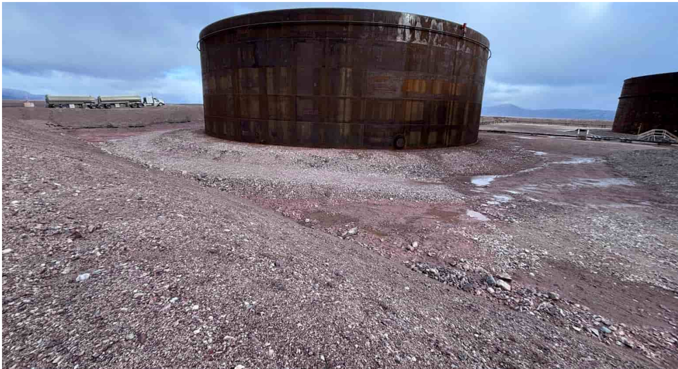
M-173: Ponding water between tanks, looking NW
