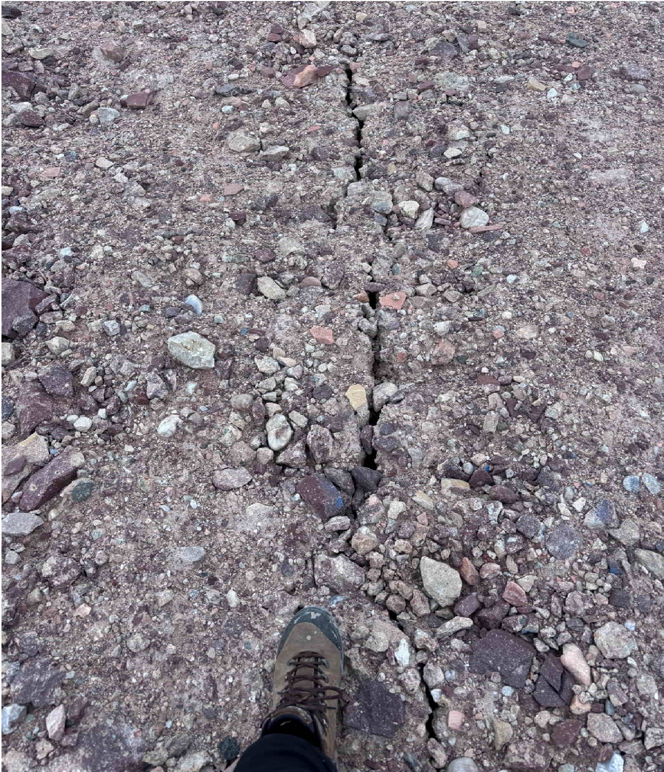
M-159: Fireball Pad - Typical tension crack above western pad slope
