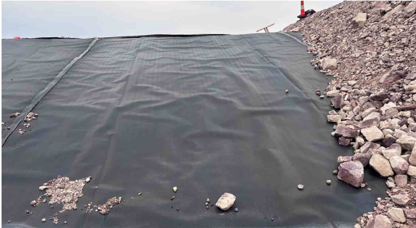
M-141: Exposed liner beside entrance to tank farm
