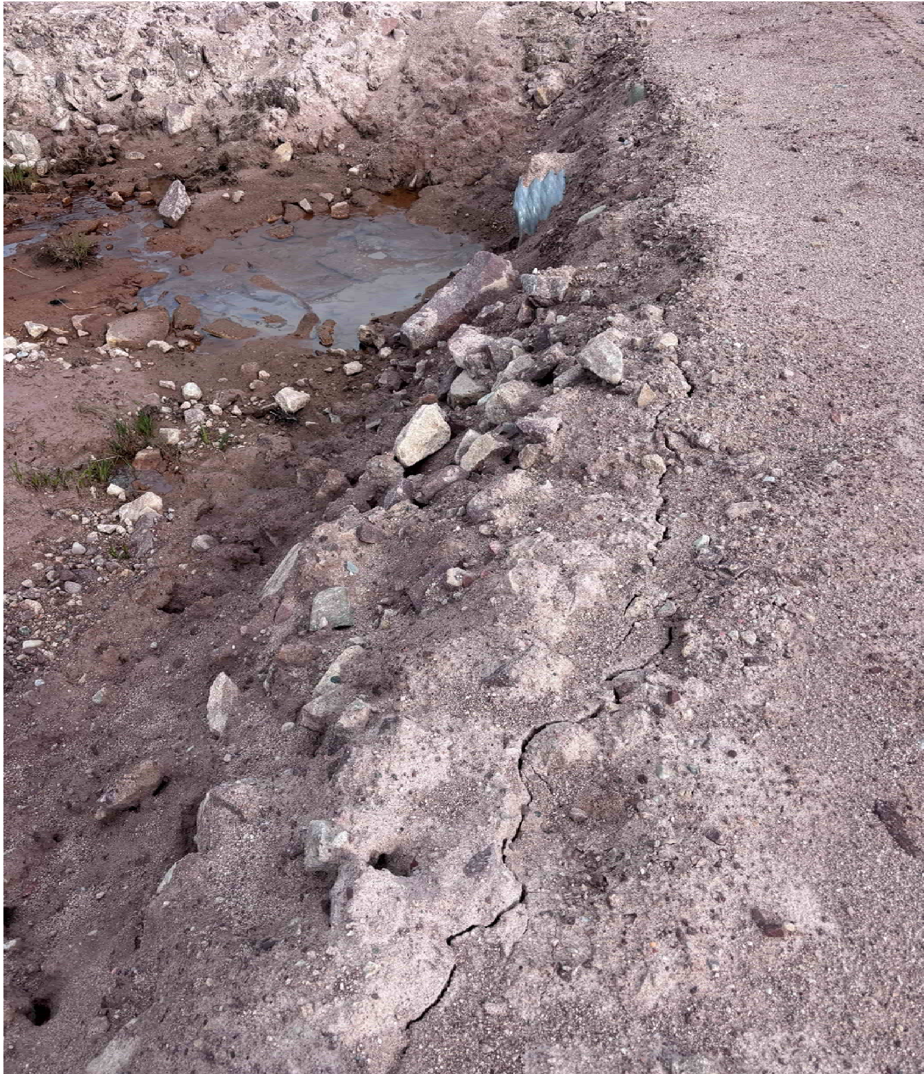
M-111: Tension crack in airstrip access road embankment, beside culvert inlet under road
