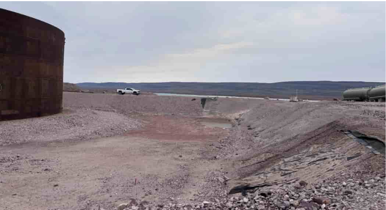
M-148: SW corner of the tank farm. Note areas with exposed liner
