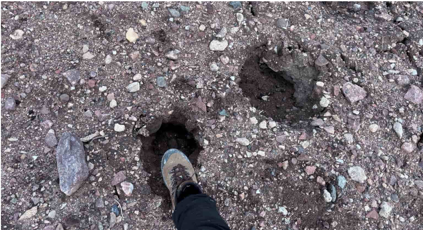
M-170: Sinkholes in southern berm
