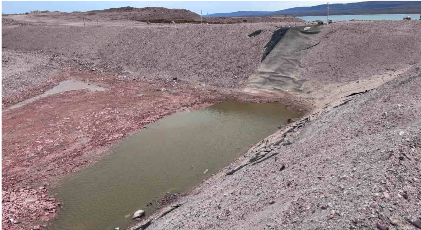
M-153: Ponding water and exposed liner at SW corner of tank farm
