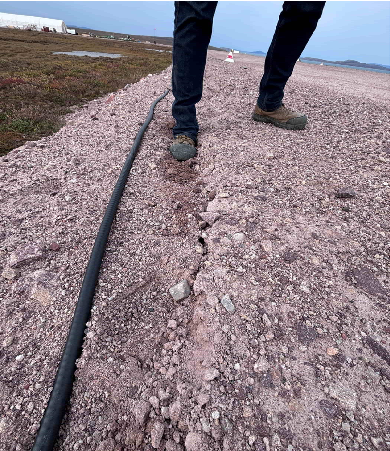
M-105: Settlement of western embankment at SE end of airstrip
