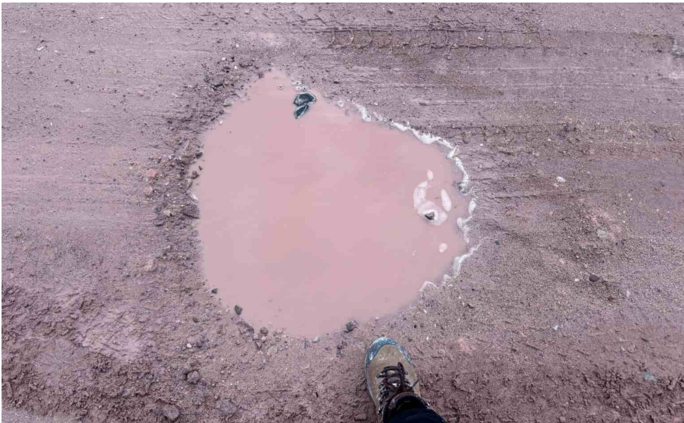
M-177: Typical size of ponding water on fireball pad
