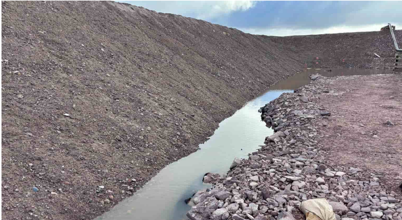
M-189: Ponding water along toe of northern berm
