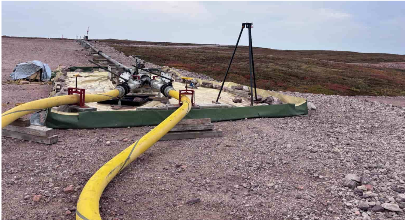
M-245: Fuel offload area piping
