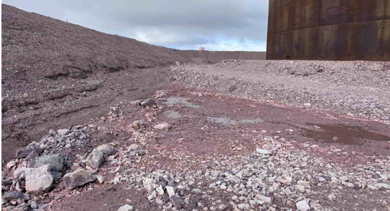
M-201: Ponding water beside SW tank and southern berm
