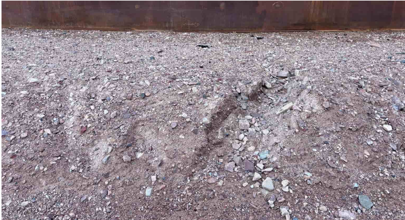
M-193: Erosion pathways beside eastern tank
