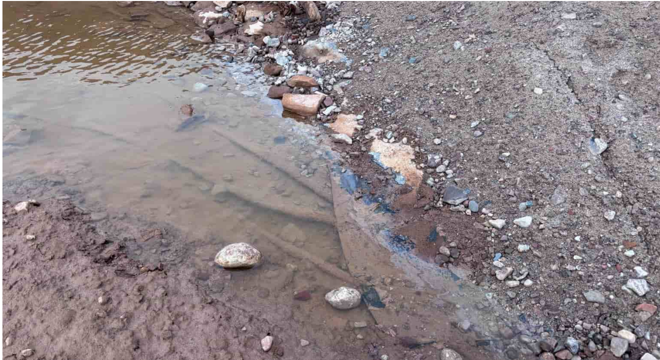
M-185: Ponding and exposed liner below western berm
