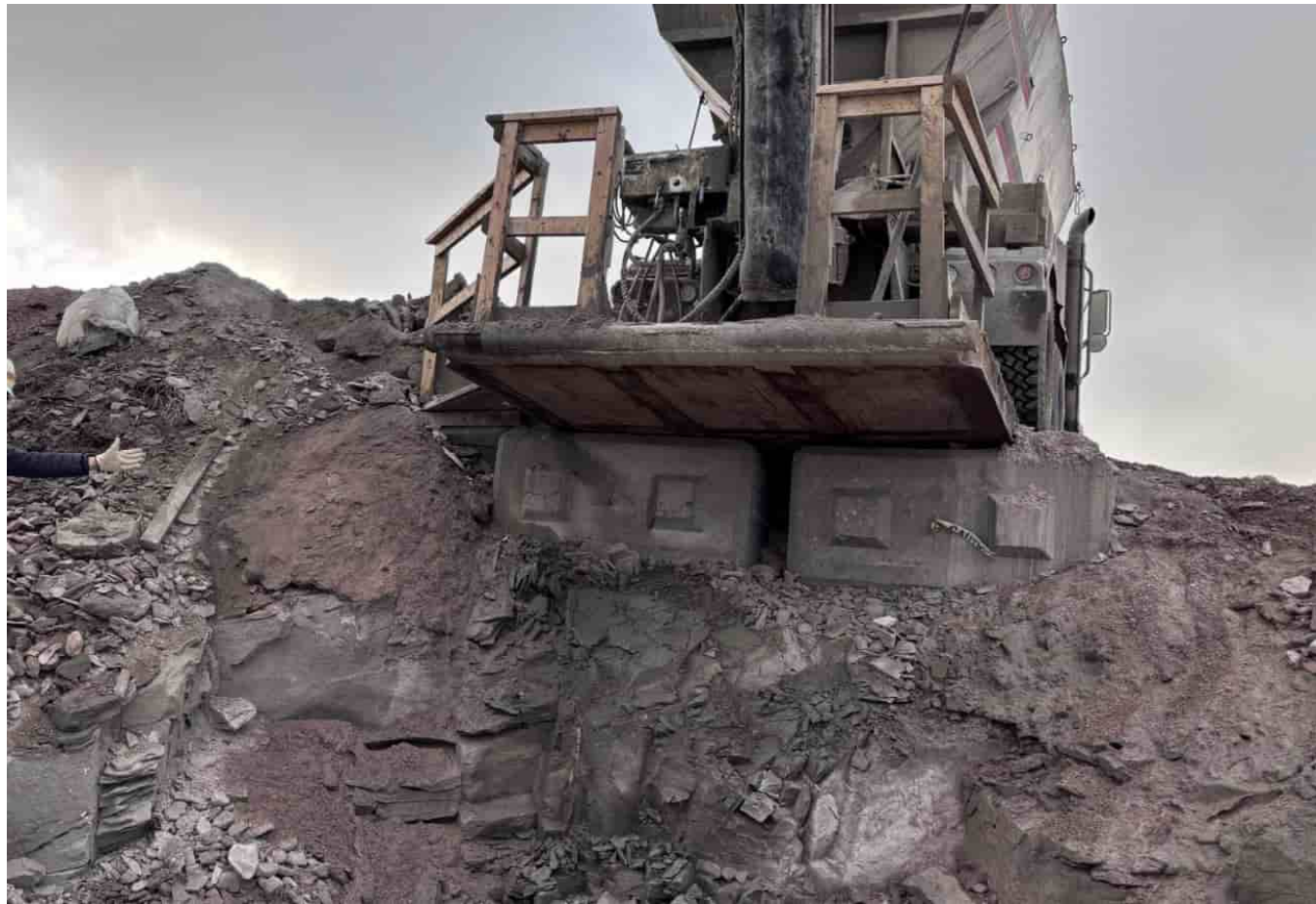
M-219: Batch plant east to the quarry. Note the sandstone joint, which may have contributed to the failure of one concrete block.
