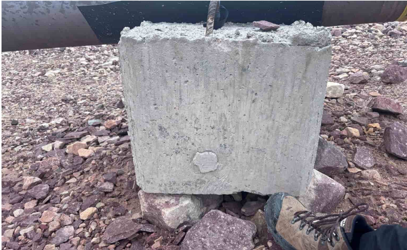
M-234: Pipe bracing supported by rocks
