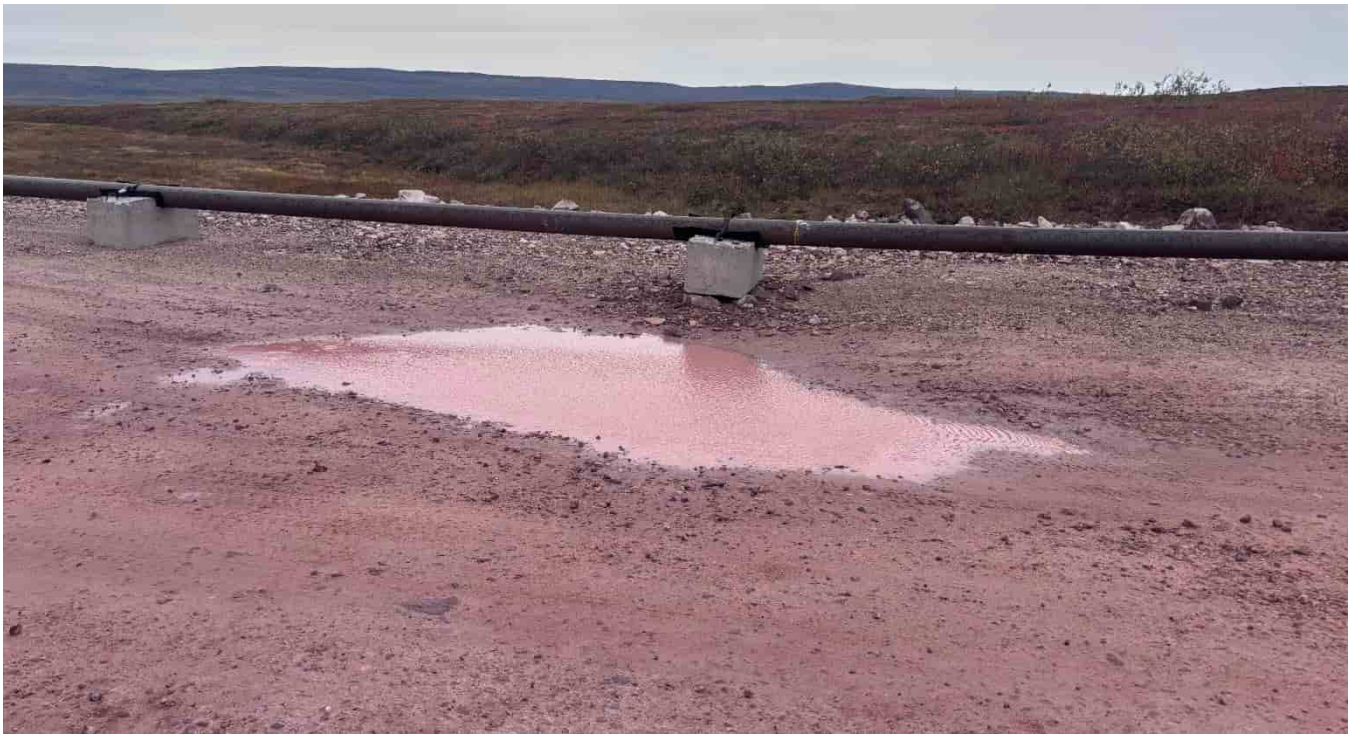
M-233: Ponding water beside piping
