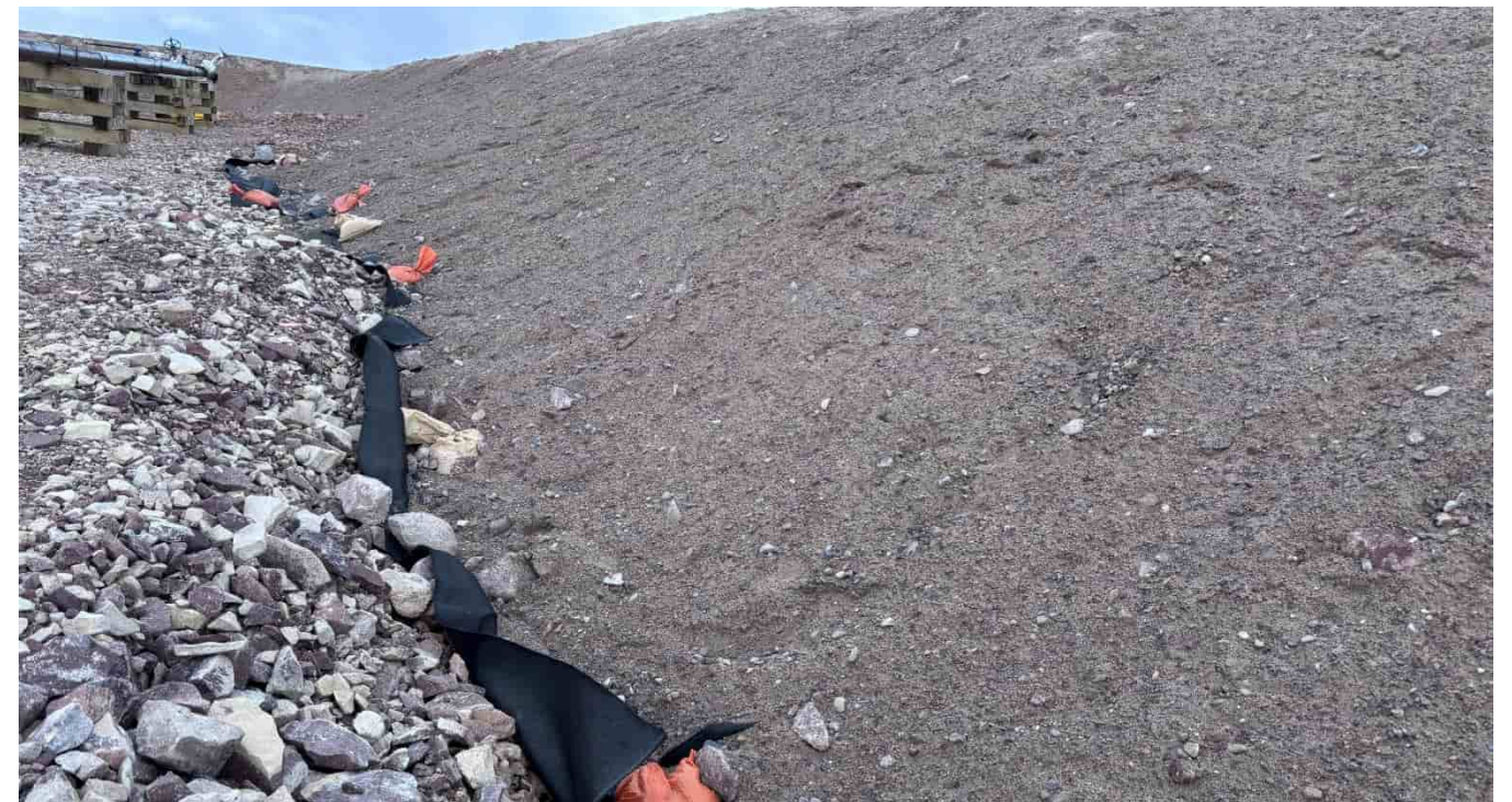
M-188: Exposed liner beneath fill at toe of northern berm, looking W
