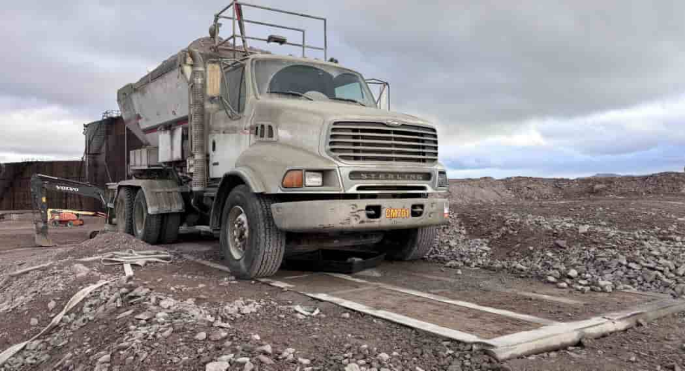
M-216: Batch plant east to the quarry. Note the deck is not anchored
