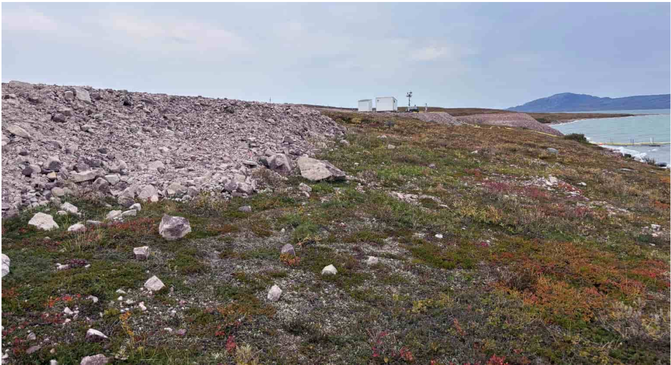
M-248: Erosion of pad slope, looking N
