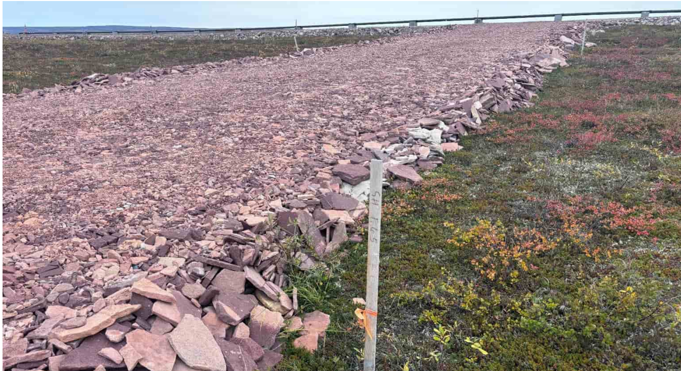
M-237: North anchor pad access road – Note pad thickness too thin
