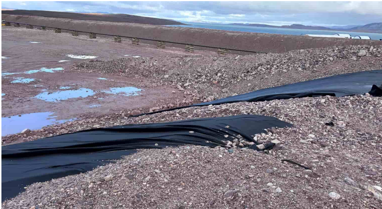
M-191: Exposed liner and ponding beside access road to tank farm
