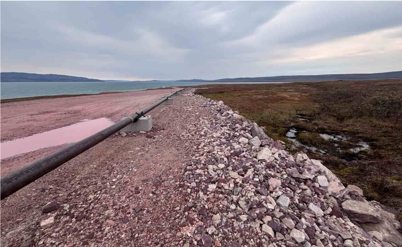
M-235: Piping, looking S towards anchor pad area
