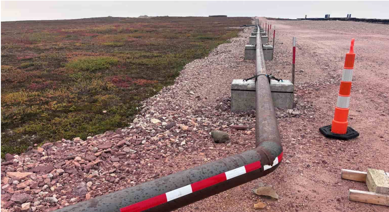
M-232: Piping, looking NW
