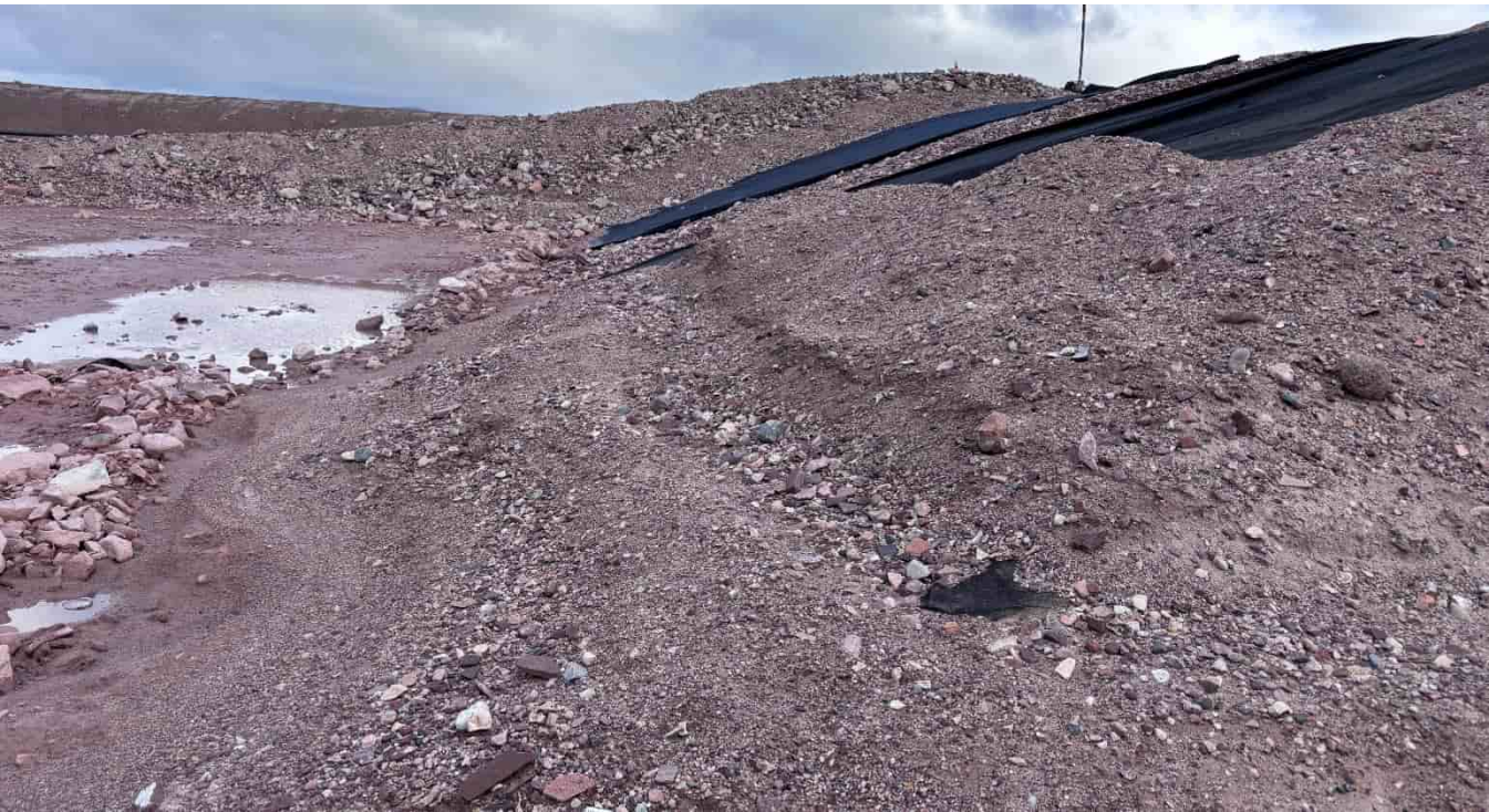
M-196: Ponding water and exposed liner on northeastern berm
