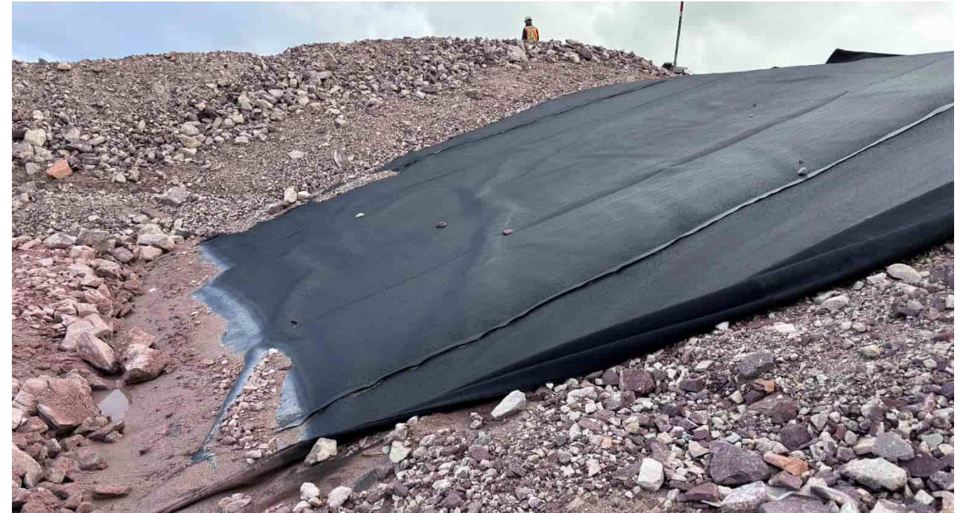
M-190: Exposed liner beside access to tank farm
