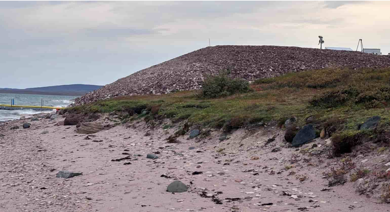
M-242: Middle anchor pad, looking S – Note shore erosion
