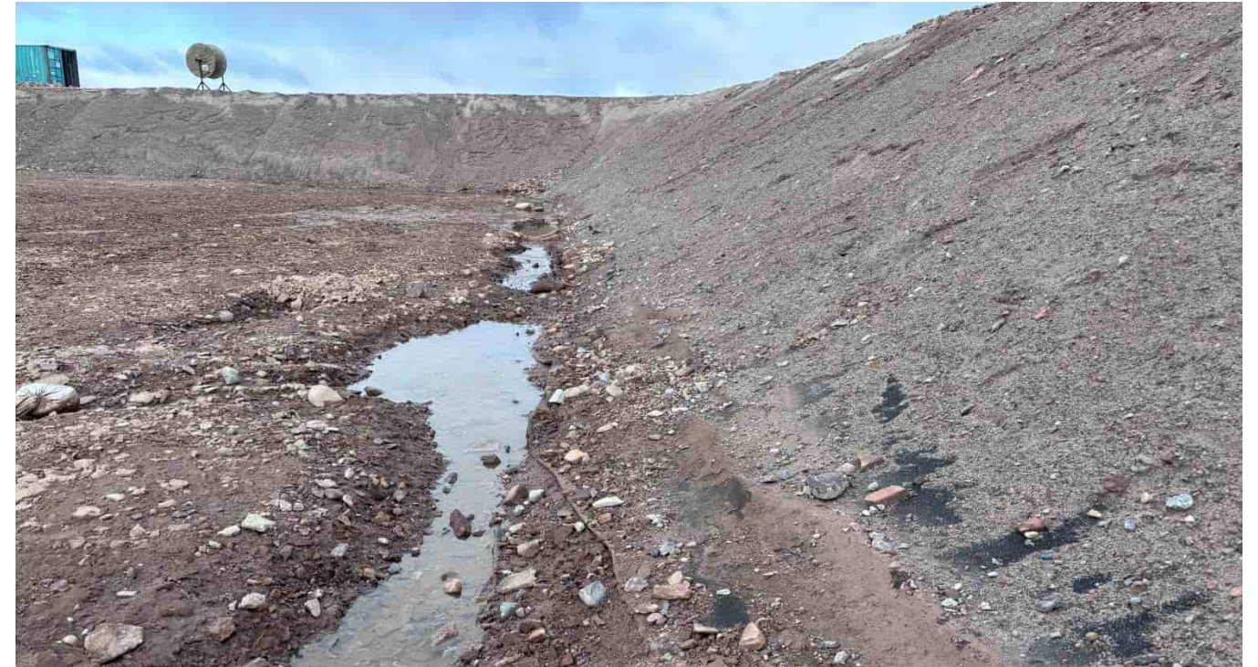
M-186: Ponding and exposed liner at NW corner of tank farm
