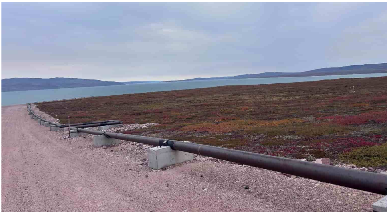
M-229: Typical pipeline configuration along edge of road embankment, looking S
