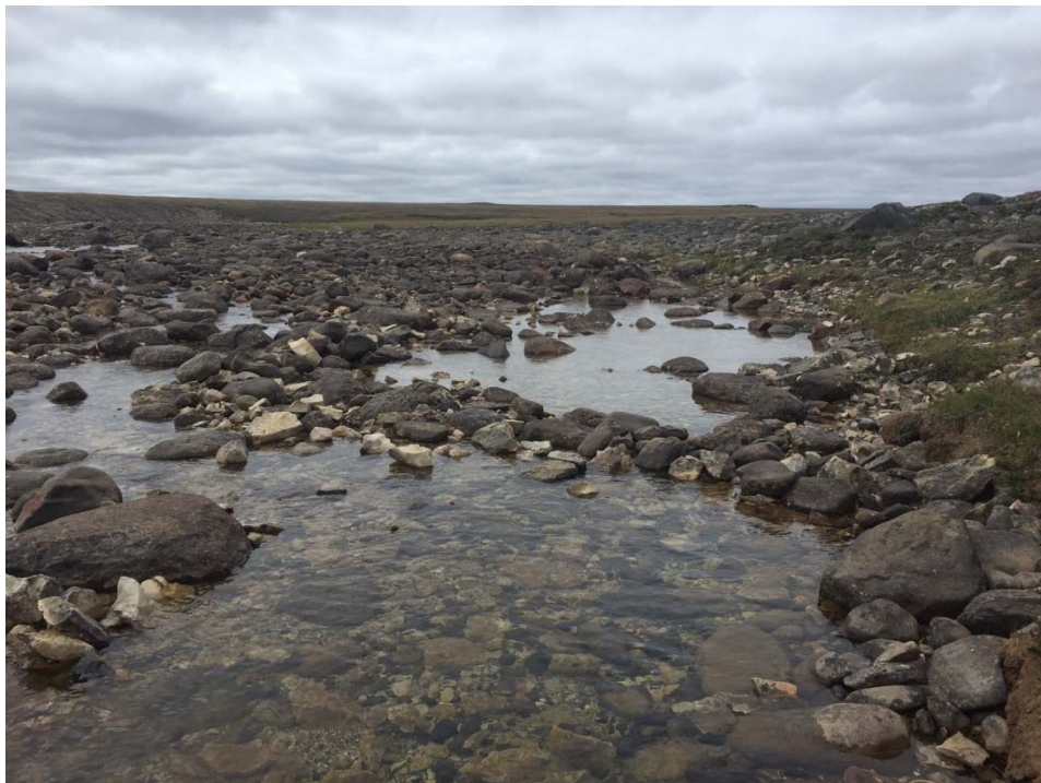
Photo 15: Upstream view of Directional Weir pre-repair at Site 5. 26 July 2017.
