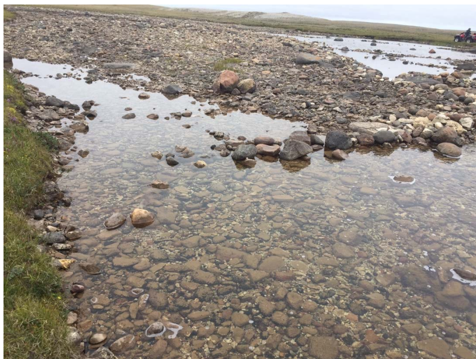
Photo 46: Blown out Directional Weir at 2012 Project 3 requiring remediation. 27 July 2017.
