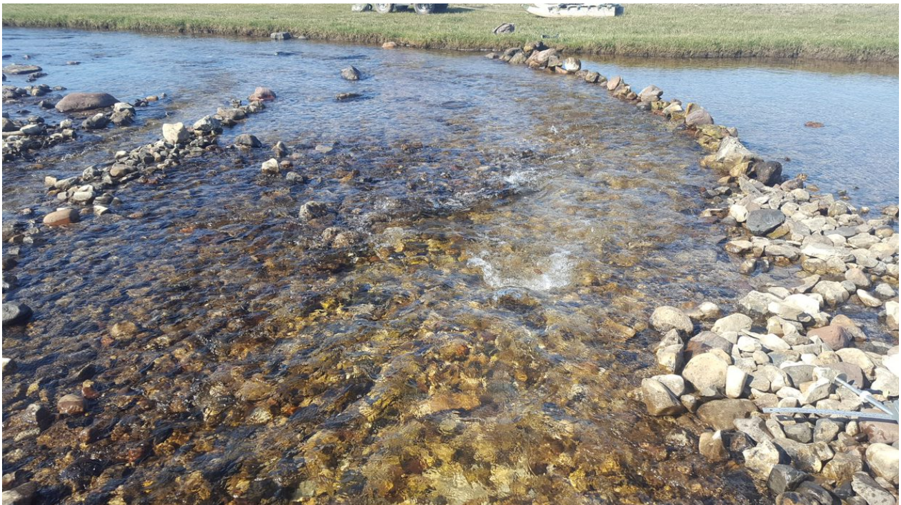
Photo A36: Downstream View of Low-flow Channel A, Pre-Repair, at 2012 Project 1, 25 July 2018
