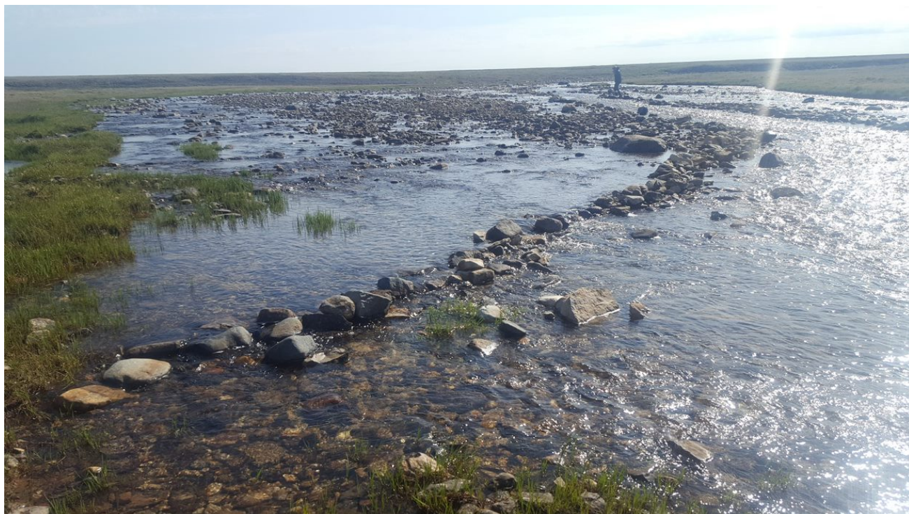
Photo A2: Upstream View of Directional Weir A Pre-Repair at Site 1 on 25 July 2018
