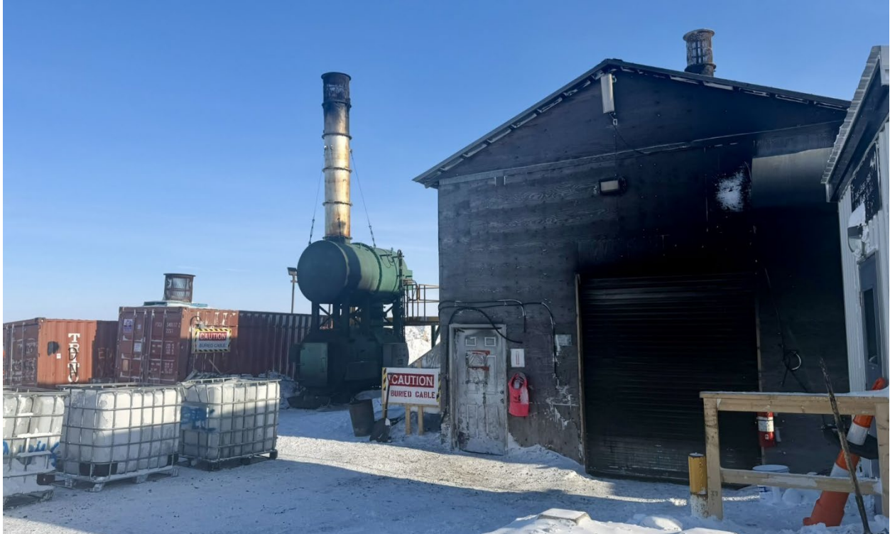
Photo 7: Incinerators - one housed inside the shed and one outside on the left when facing east
