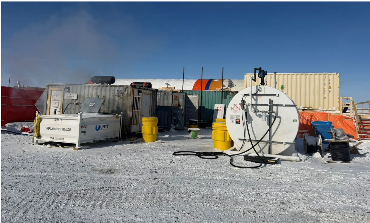
Photo 81: Fuel tanks and power generator
