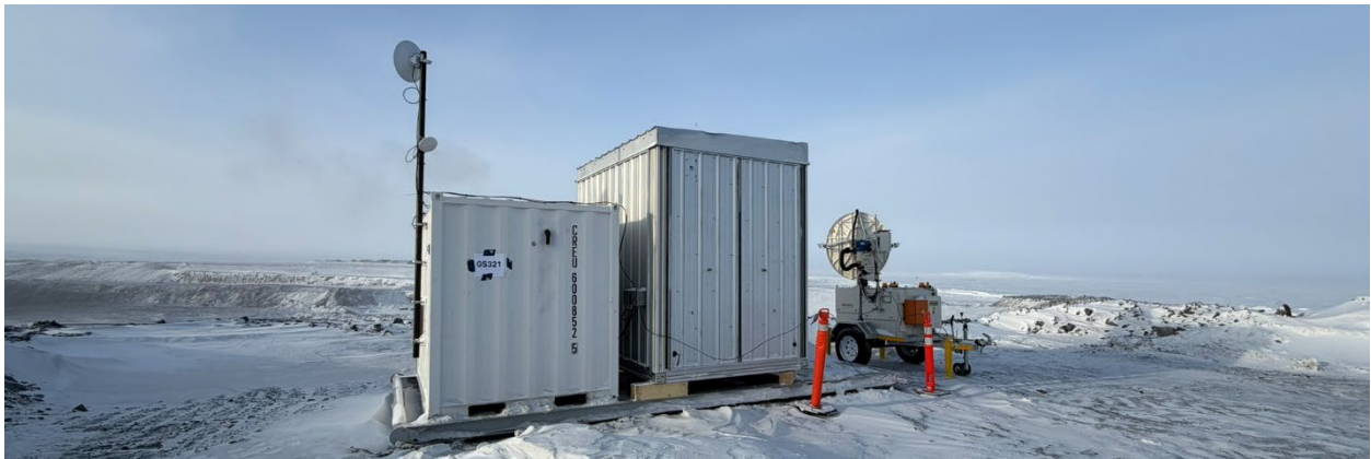
Photo 43: Geotechnical monitoring system for pit wall stability monitoring
