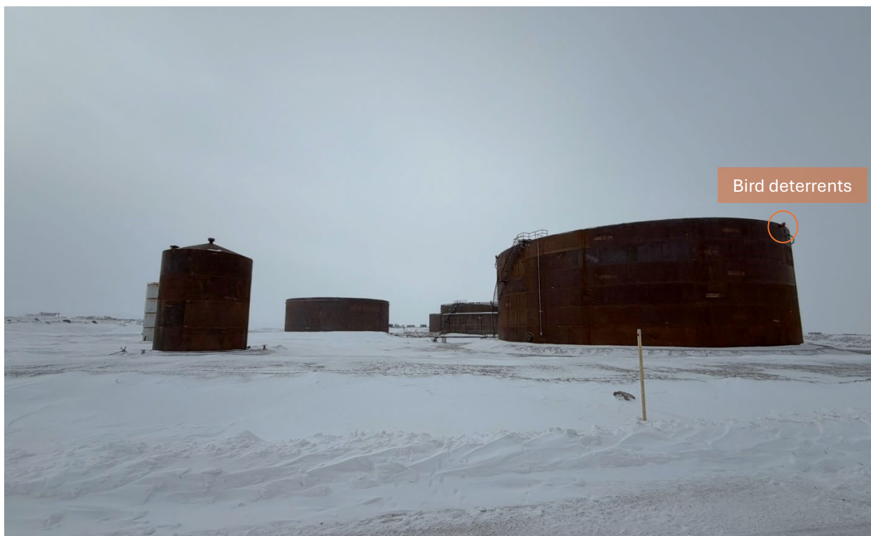
Photo 133: Fuel tanks within secondary containment, facing west
