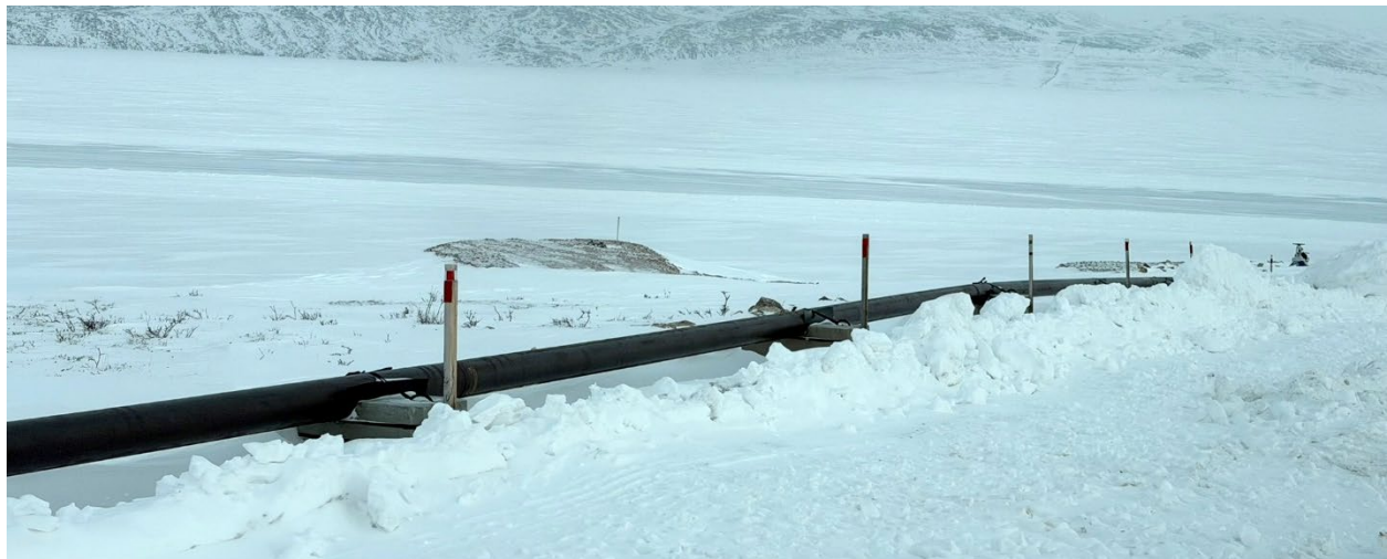
Photo 126: Marine fuel transfer line, facing east
