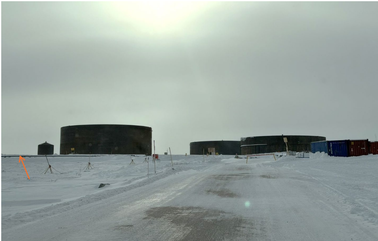
Photo 131: Fuel transfer line and Tank Farm, facing north
