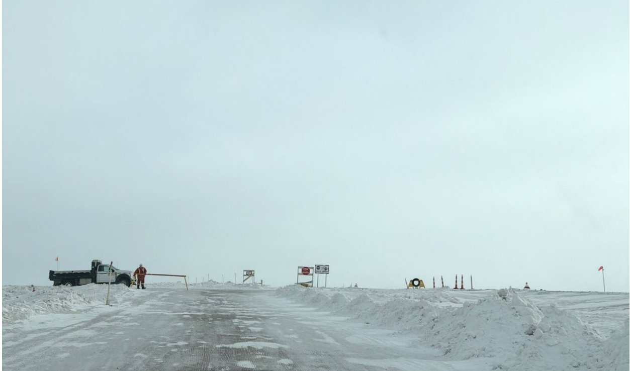
Photo 123: Bypass road closure in place to facilitate aircraft landing
