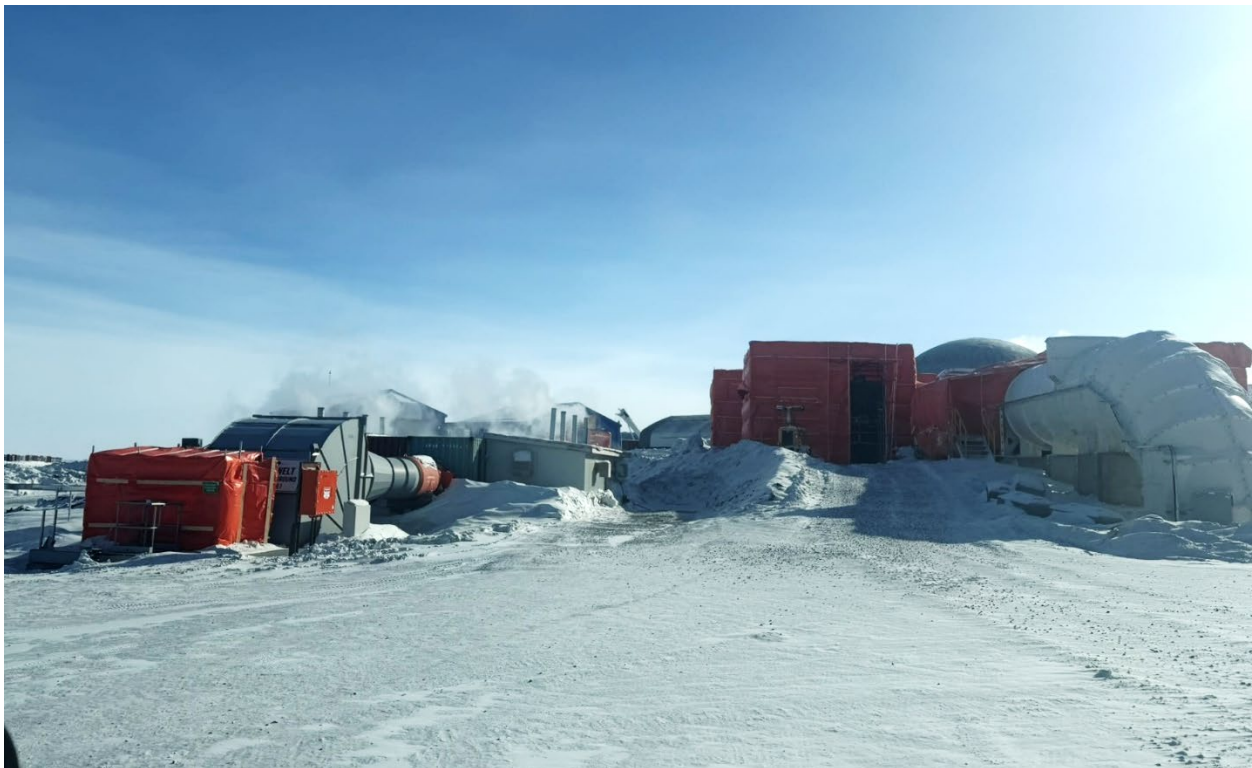
Photo 39: Fresh air intakes 1 (left) and 2 (right) for underground ventilation located north of the ore stockpile dome
