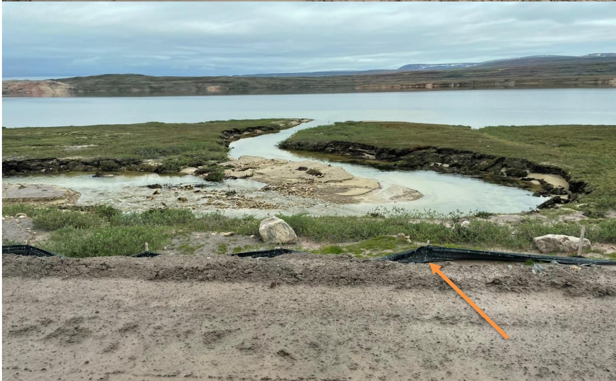
Photo 46: Erosion fence with silt build-up and deterioration at KM 89. Note extreme mudiness of the Tote Road.
