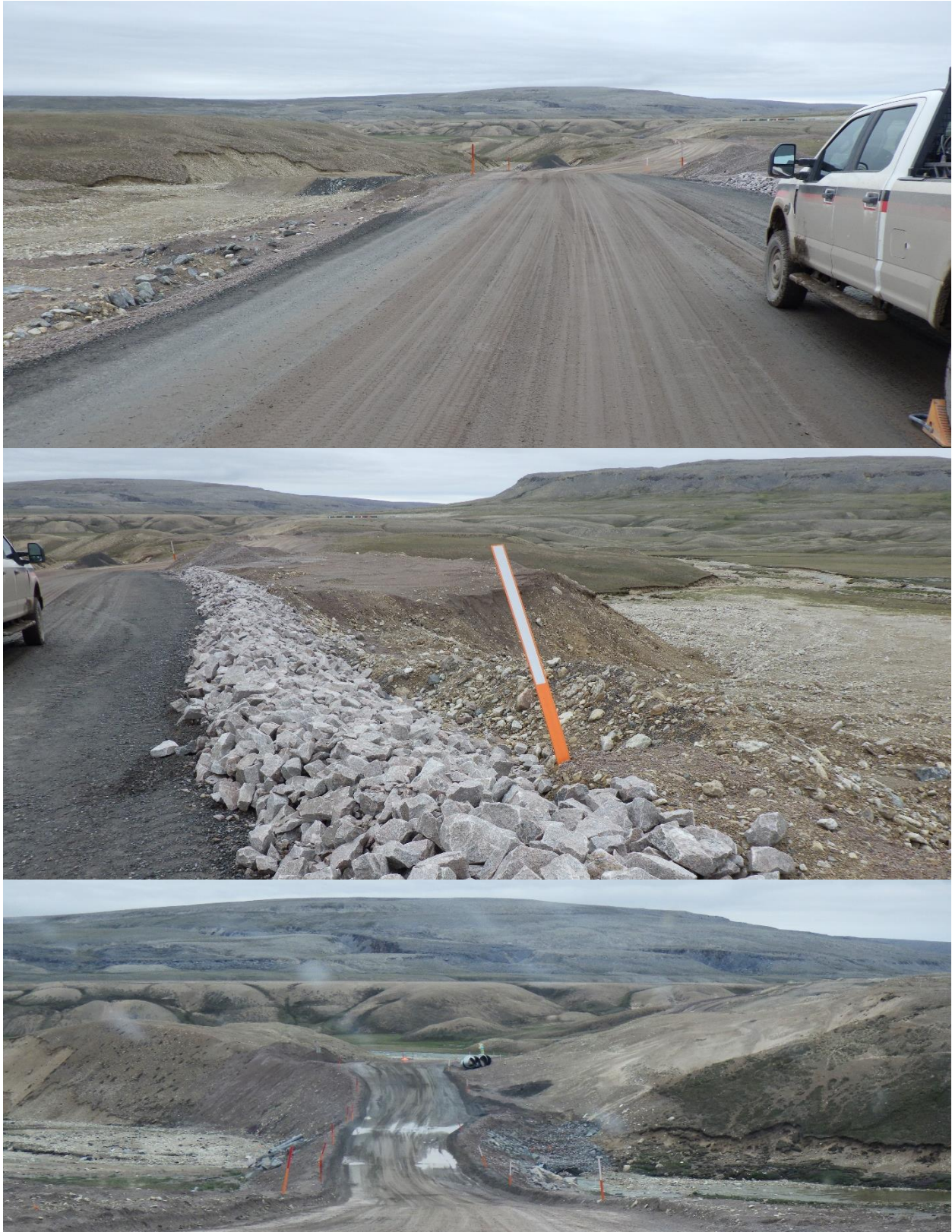
Photo 57: Area of September 2024 Washout After >1:1000-Year Rainfall Event; culverts replaced through Emergency Remediation
