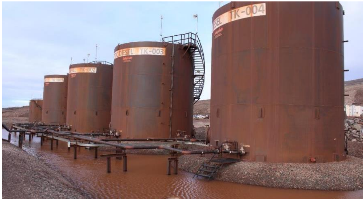
Photo 21: Mine Site Tankfarm (MS-03) (2024)
