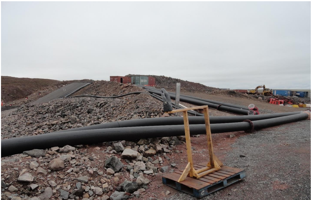
Photo 19: Waterlines for Dam at KM105
