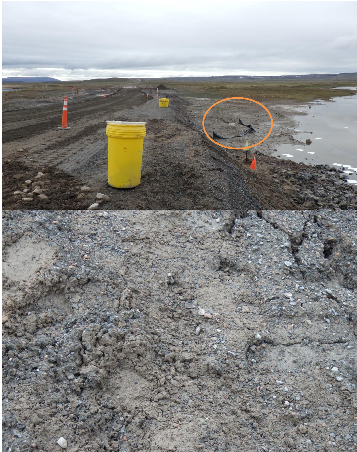
Photo 50: Road Surface at KM80 showing a soft, spongy surface
