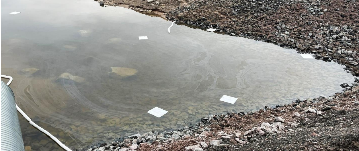
Photo 49: Culvert Outlet at KM80 (looking north) with hydraulic fluid spill
