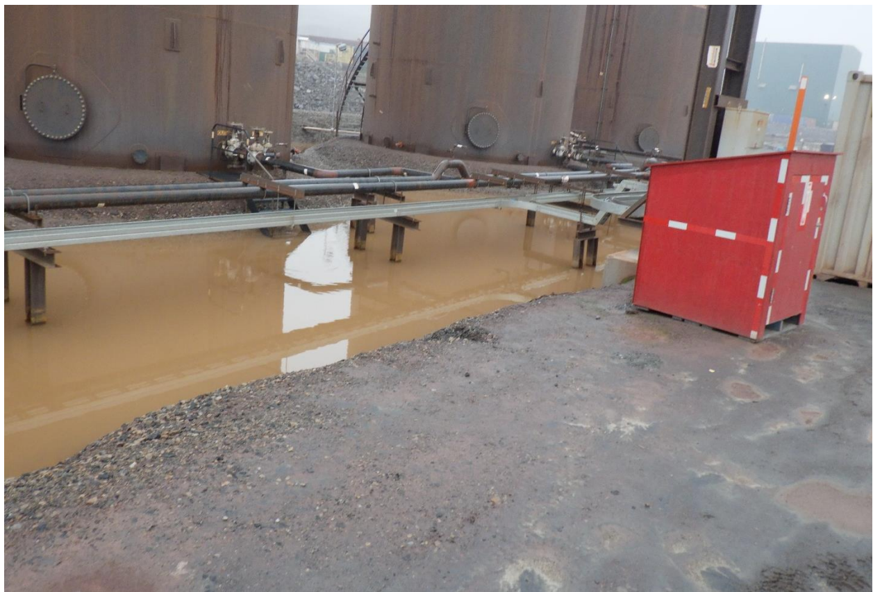
Photo 22: Mine Site Tankfarm (MS-03) (2025)
