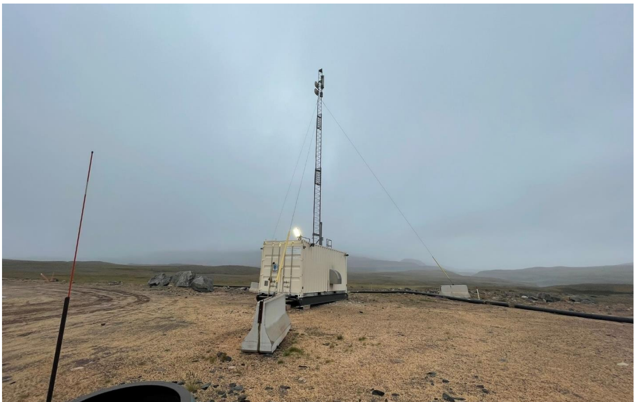
Photo 28: Communication and Monitoring Tower
