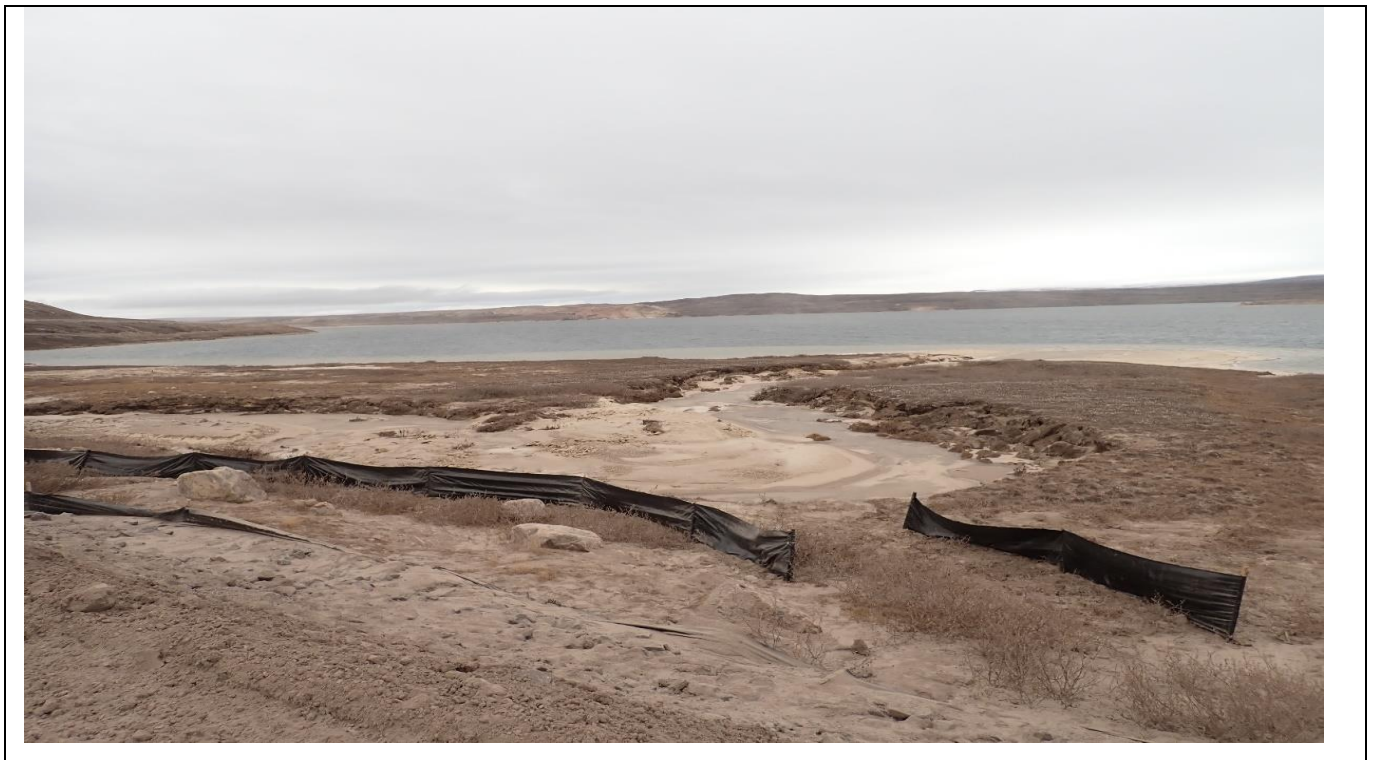
Photo 2. BG-24 (KM 87.5)- Follow up photo of new silt fences installed to mitigate erosion and sedimentation adjacent to the crossing.
