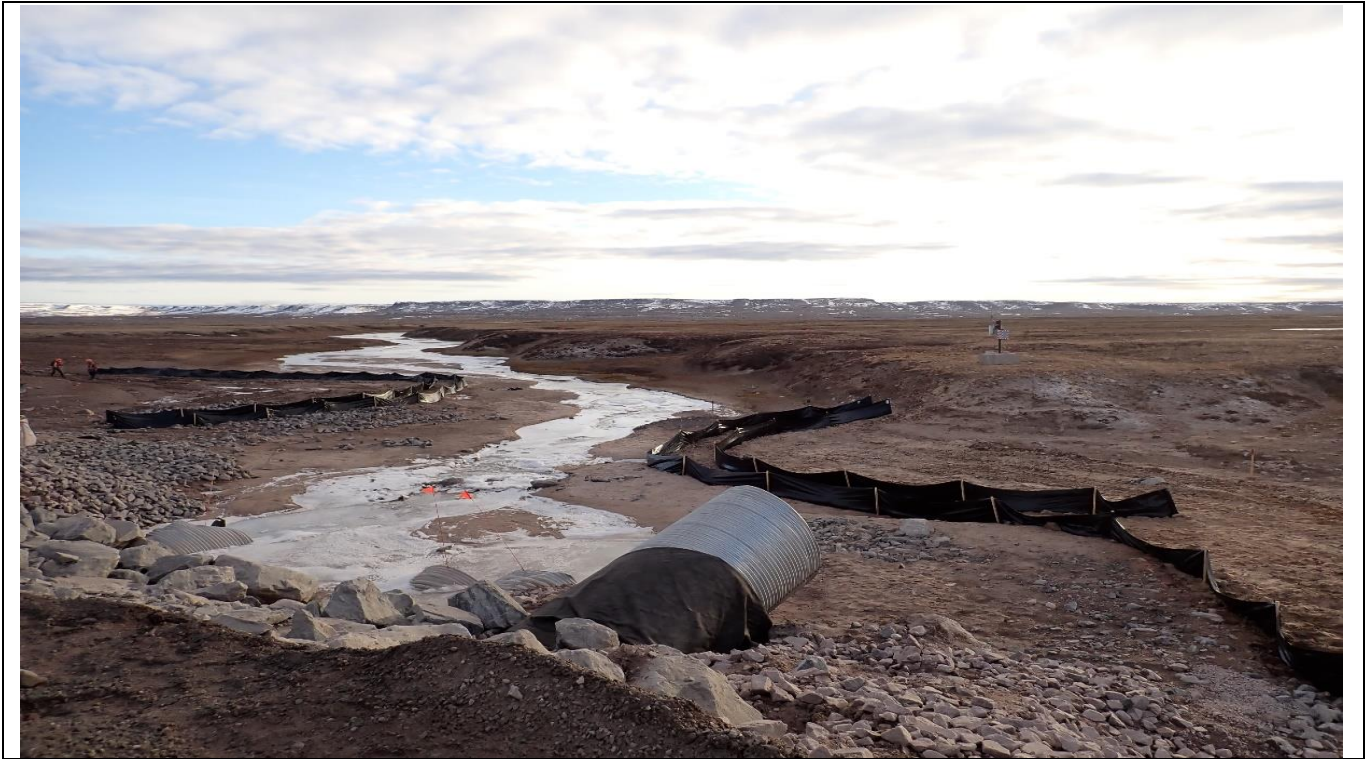
Photo 5. CV-216 (KM 82) – Follow up photos of new silt fences installed to mitigate erosion and sedimentation adjacent to the crossing.
