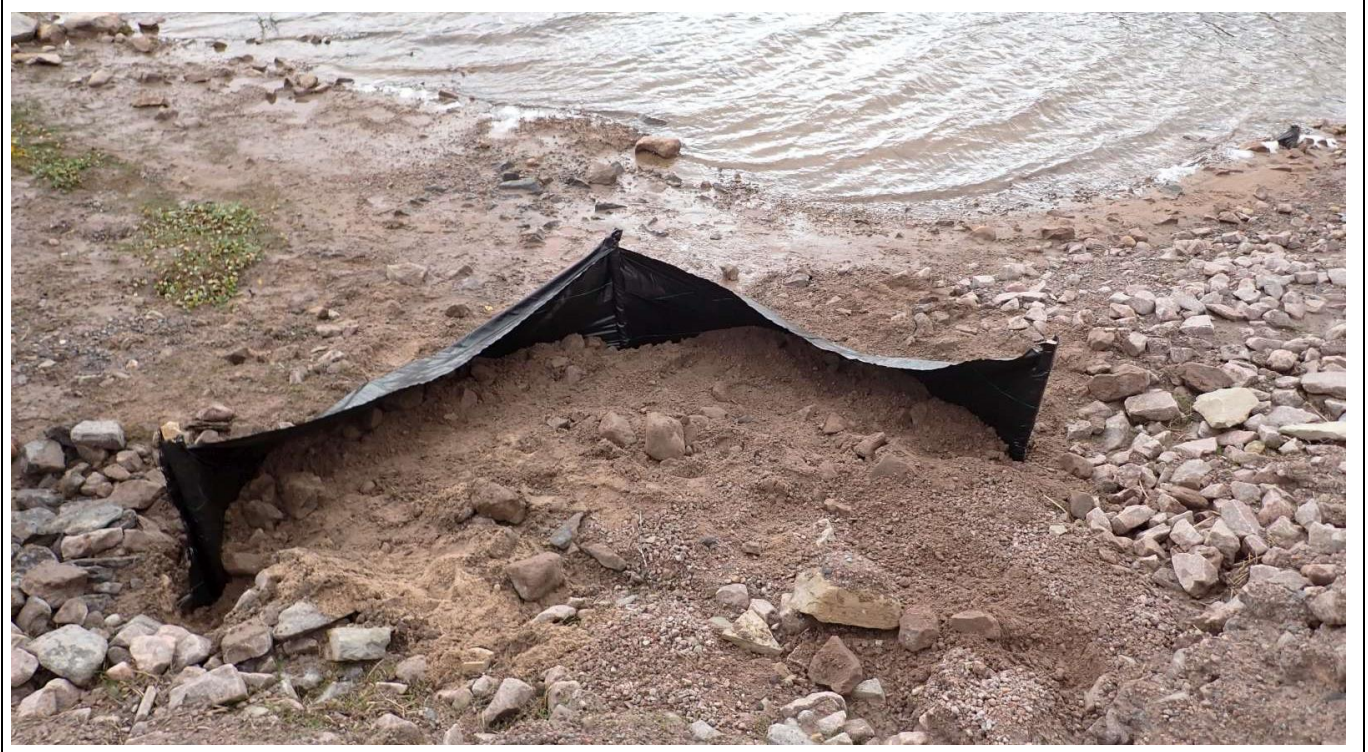
Photo 11. BG-29 (KM 85.5), Roadway bank erosion, silt fence installed upstream of crossing
