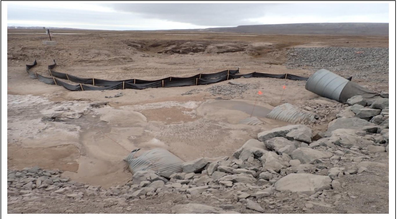
Photo 6. CV-216 (KM 82), Follow up photos of new silt fences installed to mitigate erosion and sedimentation adjacent to the crossing.
