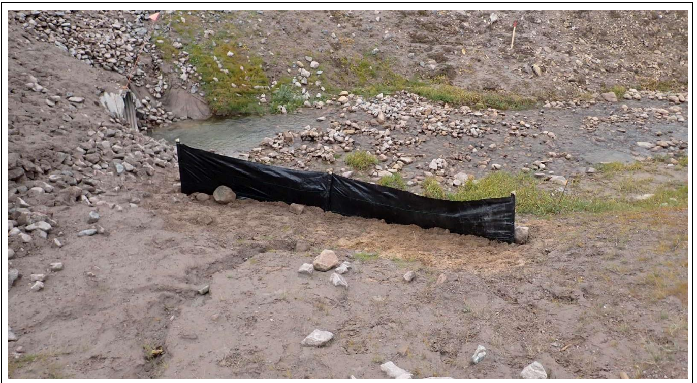
Photo 10. BG-30 (KM 85), Roadway bank erosion, silt fence installed downstream of crossing
