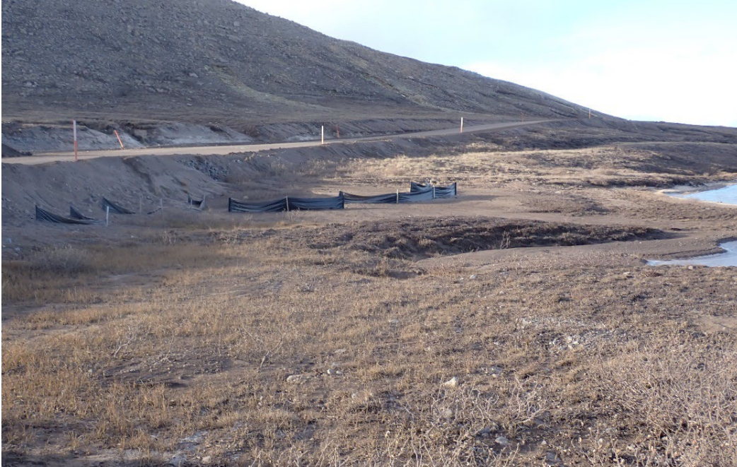
Photo 13. Erosion and Sediment Control Silt Fence at KM 87.5 Water Crossing – September 2025
