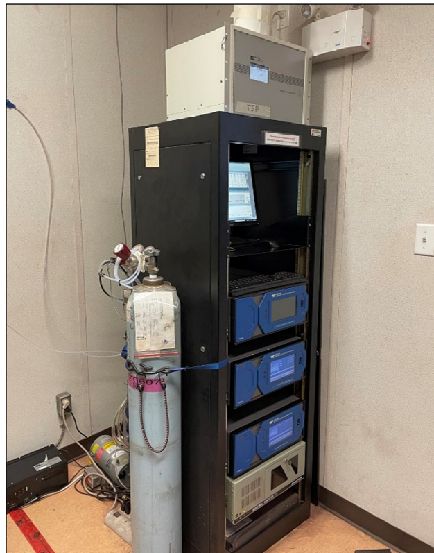
Photo 3.1-2 Rack-mounted Teledyne T100 (SO 2 ) and T200 (NO x -NO 2 ) continuous gas analyzers at the Port Site Complex ambient air quality station.
