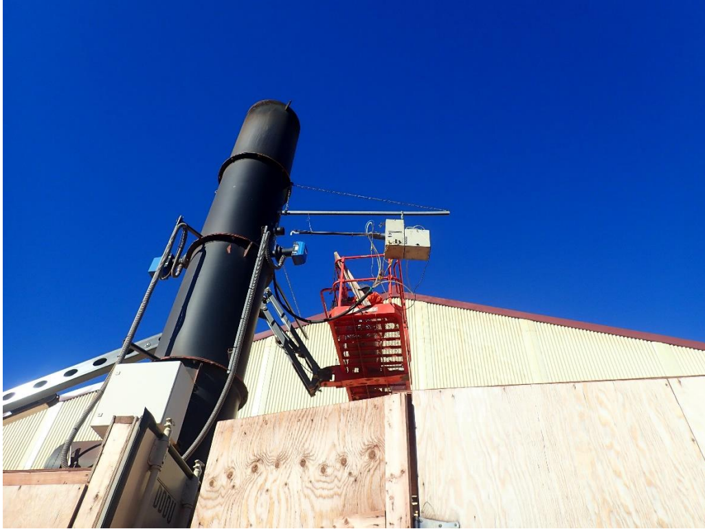
Figure 1: Eco Waste Incinerator Stack, Milne Port
