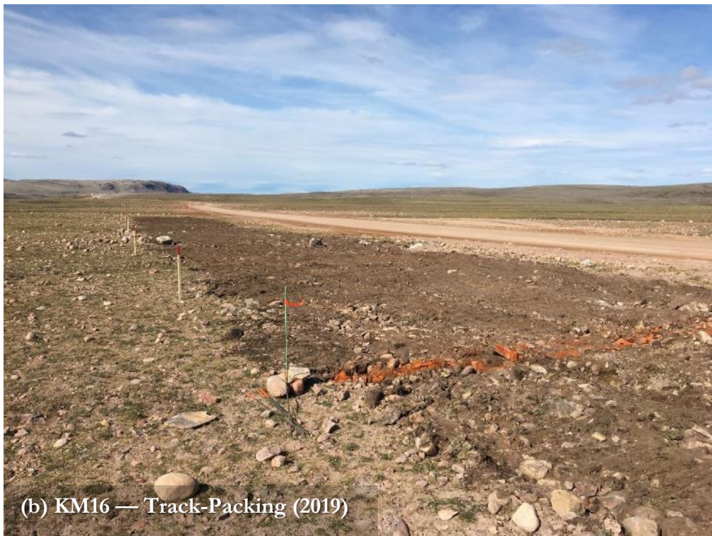
Photo 11. KM16 — Rough-and-loose (a) and Track-Packing (b).
