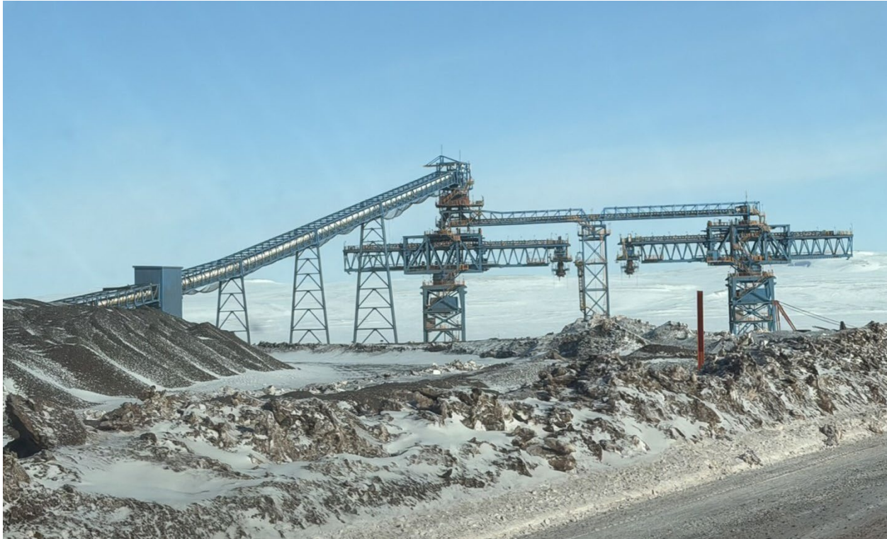
Photo 79: Milne Port ore dock showing two (2) ship loaders: one (1) currently operational, with a second unit under construction, facing north
