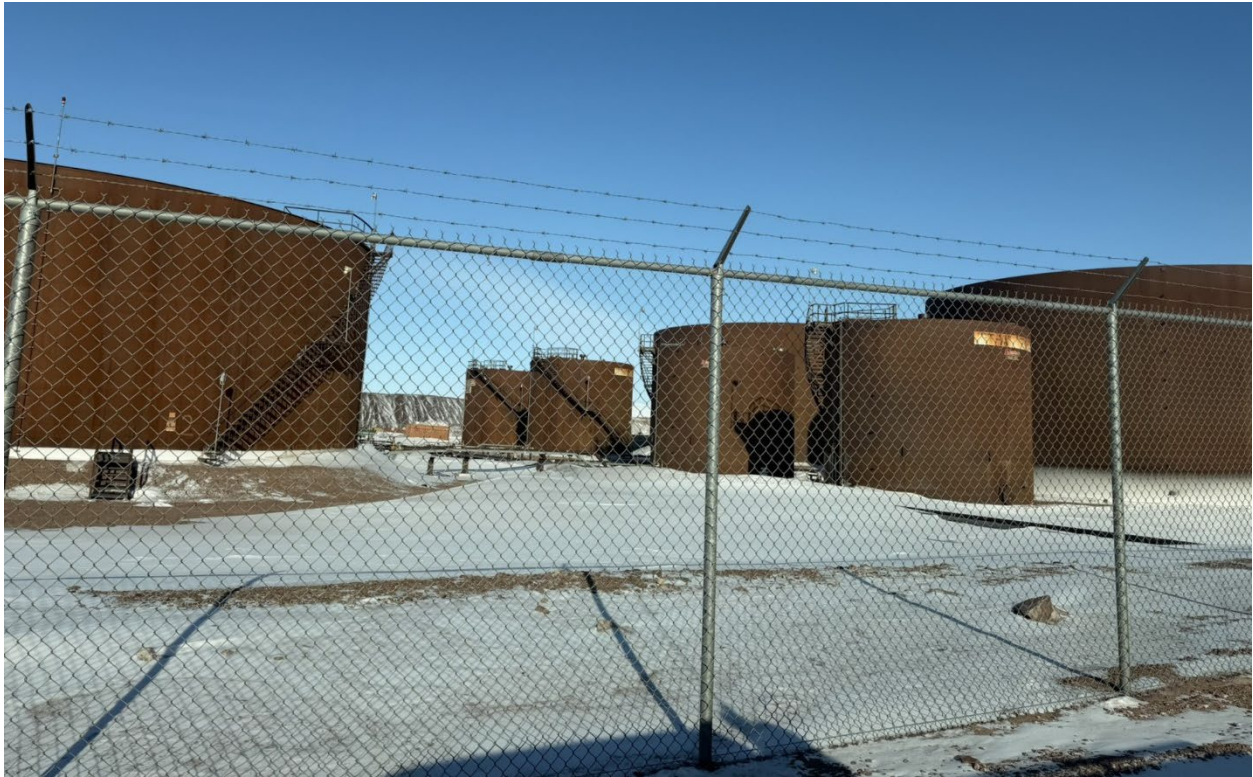
Photo 97: Fuel tanks at the fuel tank farm within secondary containment and perimeter fencing
