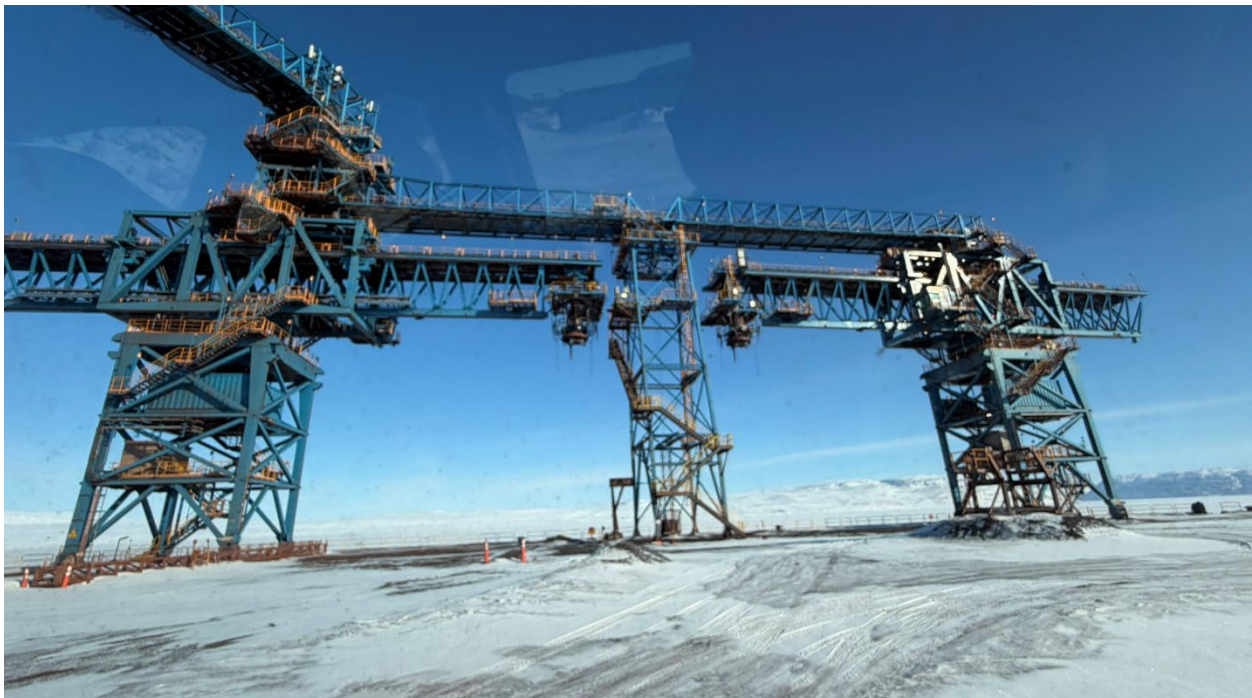
Photo 80: Closure view beneath the Milne Port ore dock ship loaders, capturing the scale of the operational unit alongside the structure under construction from ground level
