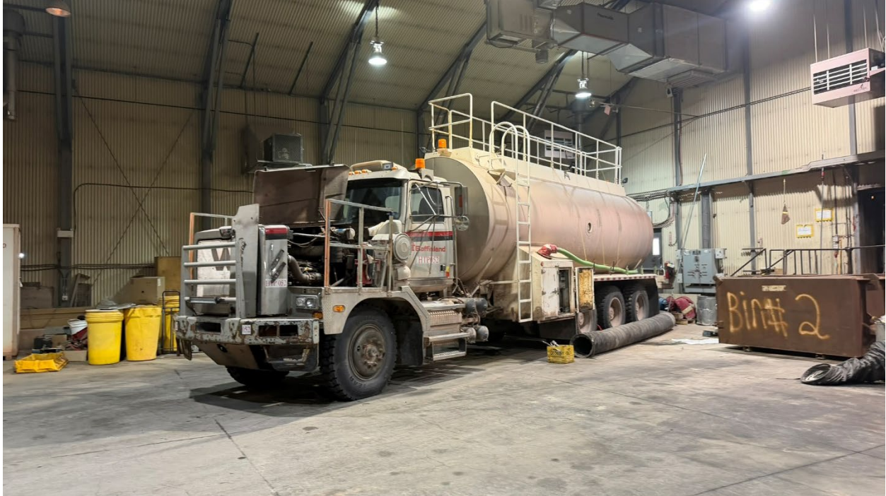
Photo 93: Interior of the incinerator building, well organized with ongoing cleaning activities and spill kits readily available
