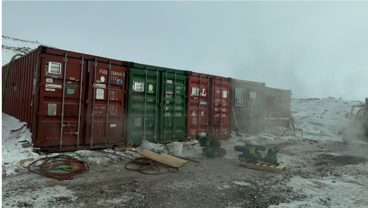
Photo 7: KM 105 Dam pumping station
