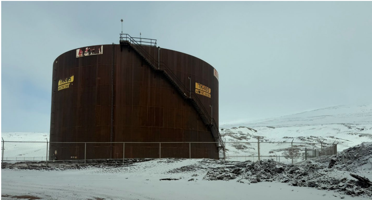
Photo 23: Chain link fence and secondary containment around Fuel tank farm (MS-03B)
