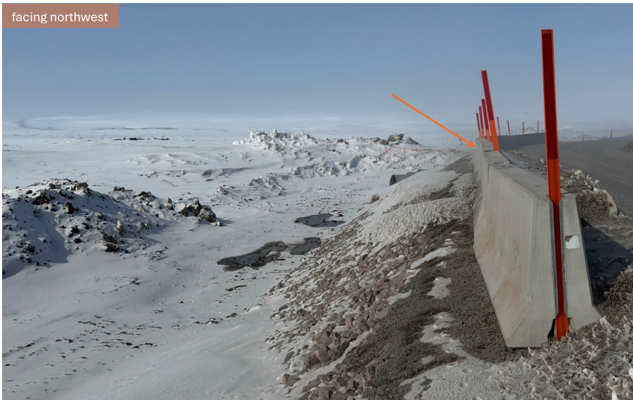
Photo 72: Concrete jersey barriers installed along both shoulders of the new by-pass road 8
