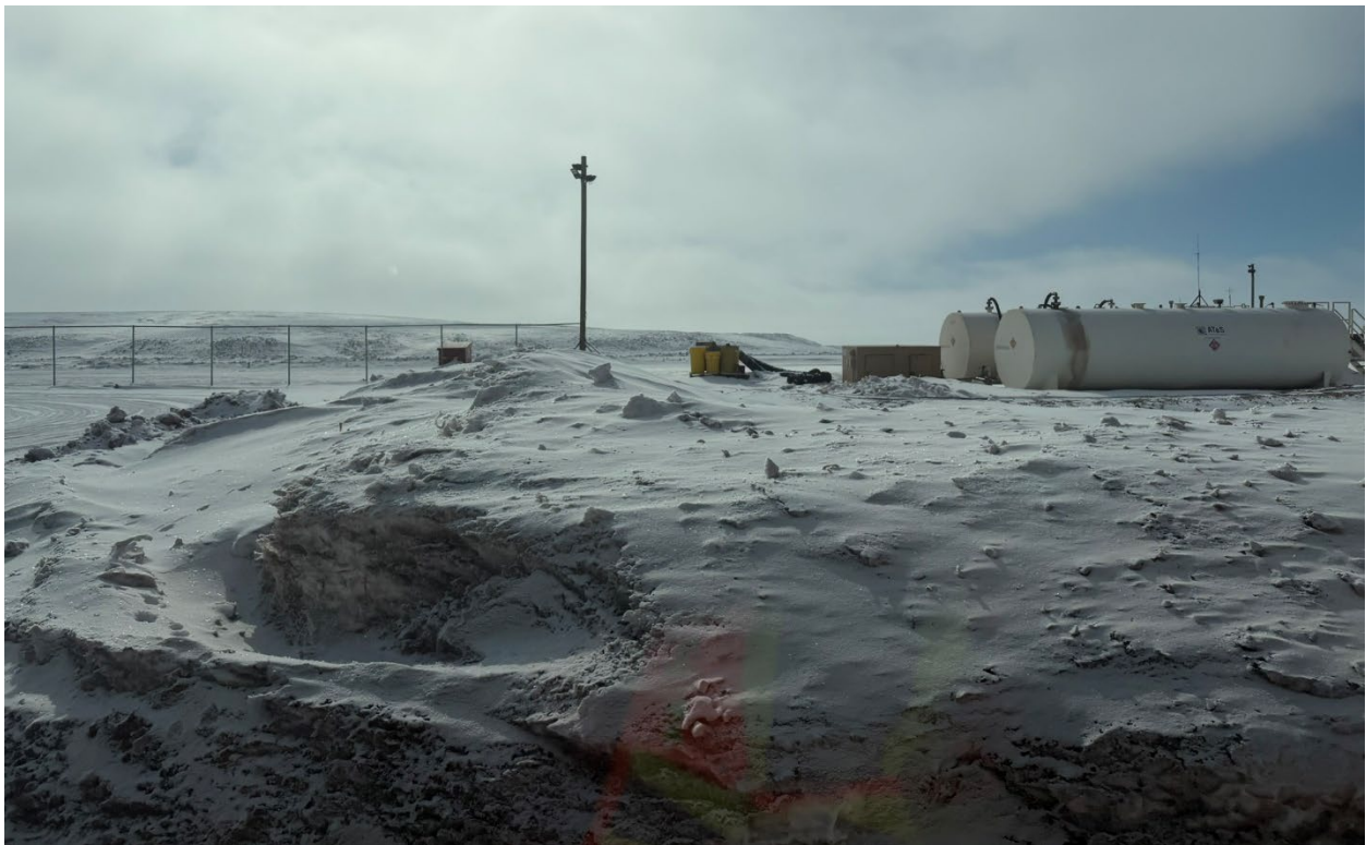
Photo 41: Fuel tanks within secondary containment at the helicopter pad (west of warehouse area); spill kits present
