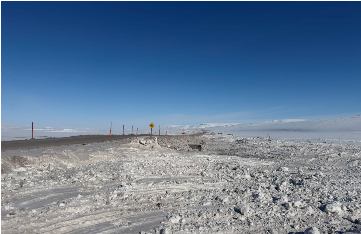
Photo 56: Fish passage culverts at KM 33, north-facing view
