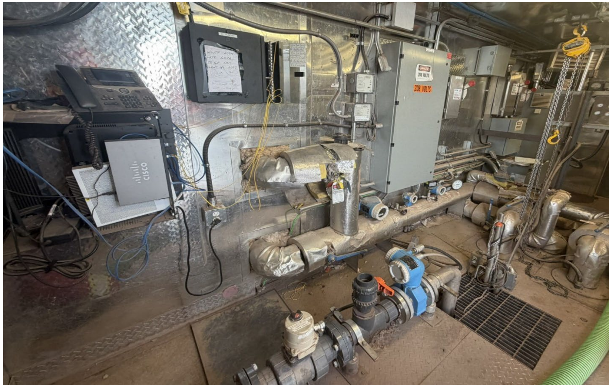
Photo 43: Pumphouse interior showing water intake system with results transmitted directly
