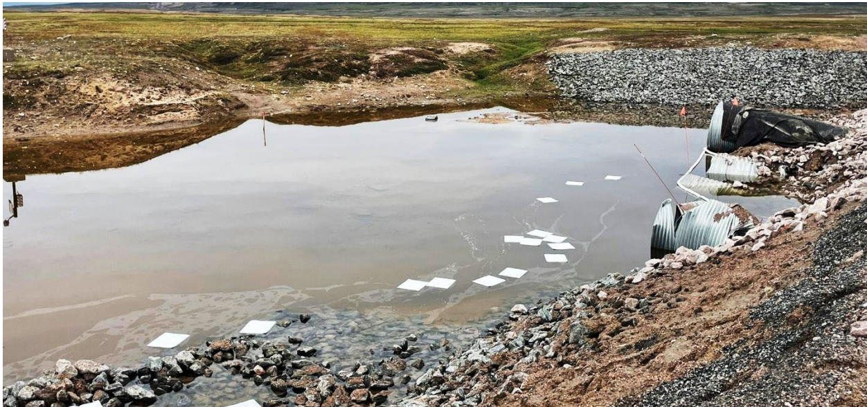
Photo 1: Culvert Inlet at KM80, hydraulic fluid spill observed (Source: 2025 NIRB Site Visit Report)
