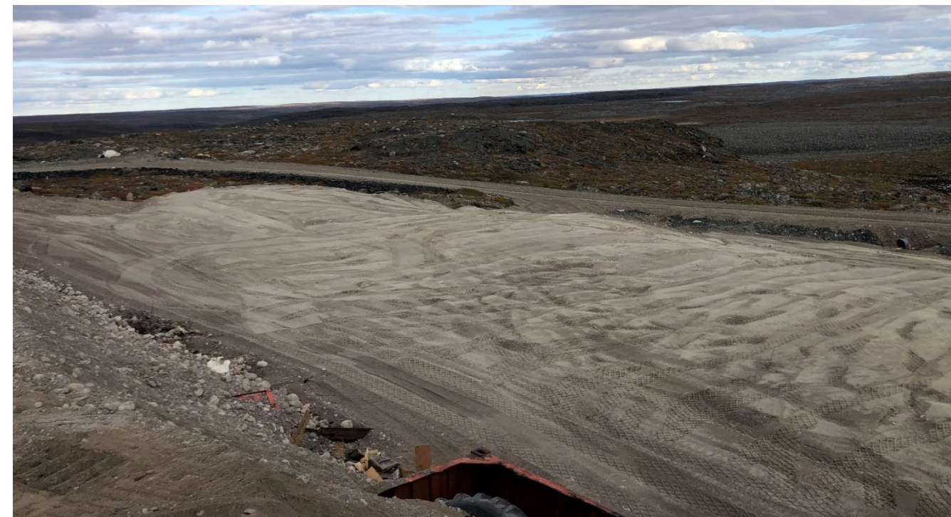
The north side of the site facing southeast with interim cover compaction on August 19, 2021
