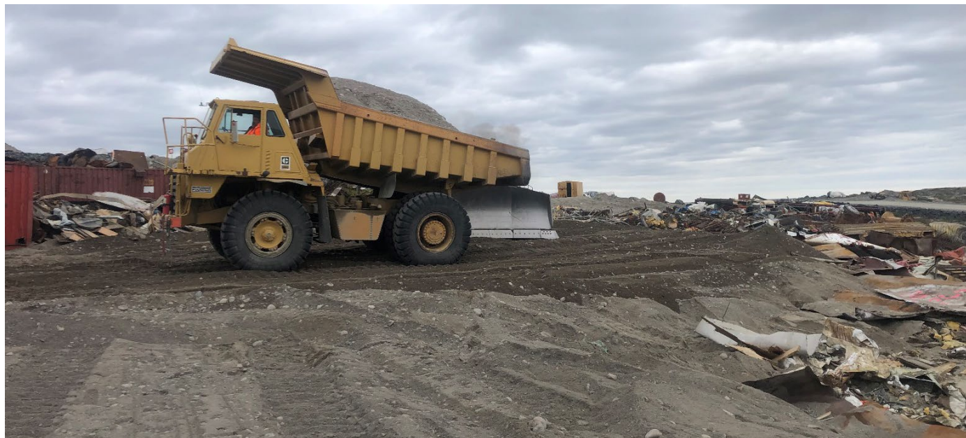
The north side of the site facing south with esker void fill and cover on August 9, 2021
