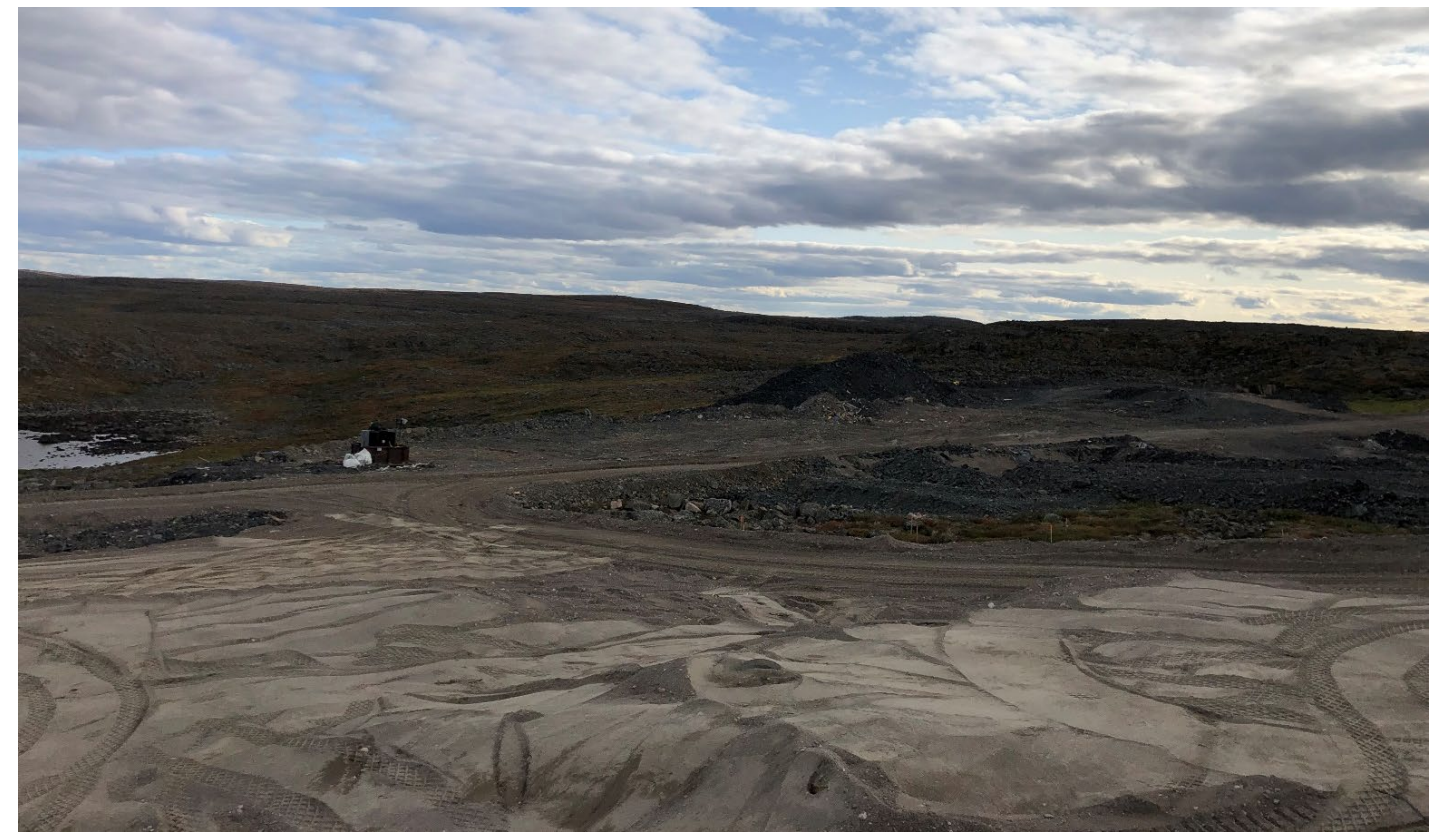
The north side of the site facing southwest with interim cover compaction on August 19, 2021
