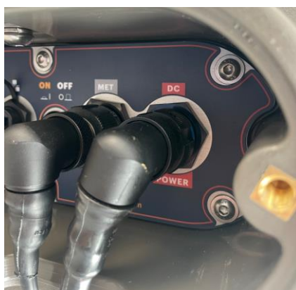
Figure 5 Lidar power connection
