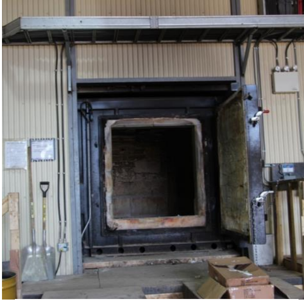
Picture 46: Incinerator at Mine Site
