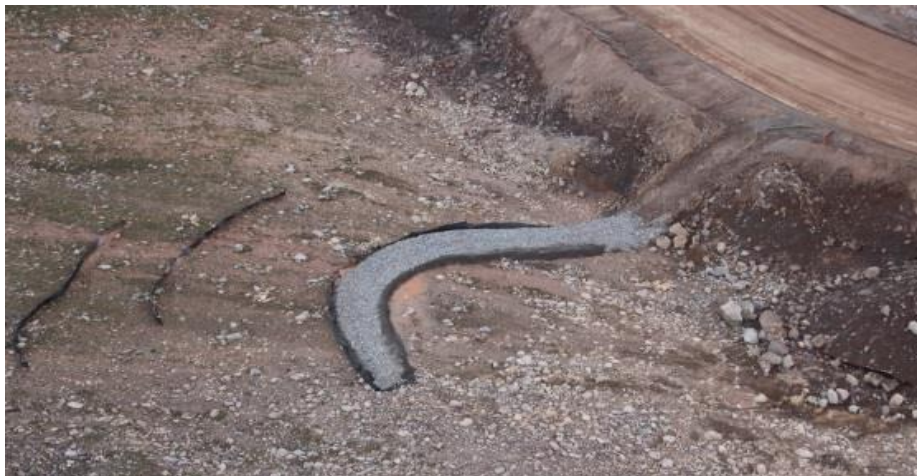
Picture 49: Check dam along the road to Deposit No. 1
