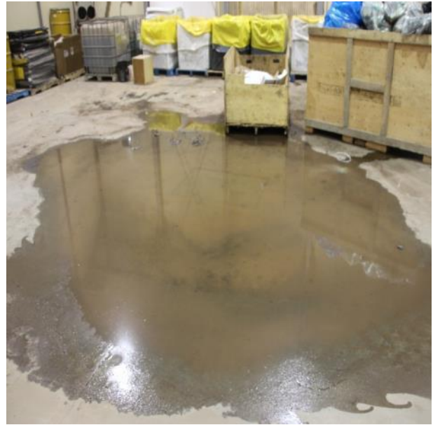
Picture 45: Water pooling at Incinerator
