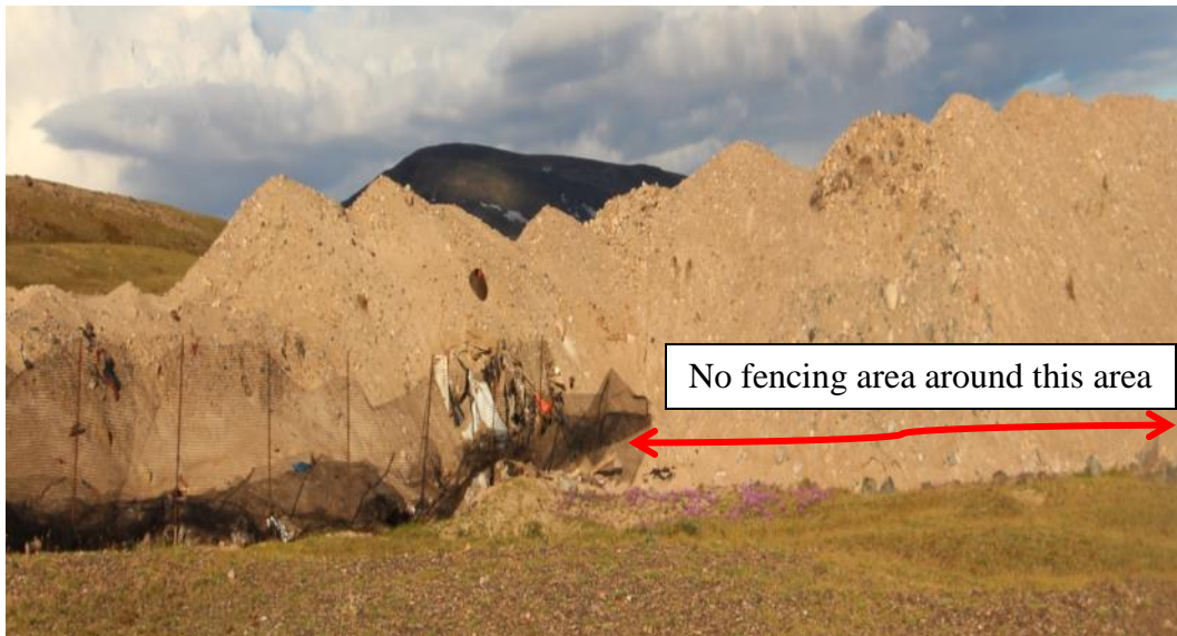
Picture 58: Deteriorated landfill fencing
