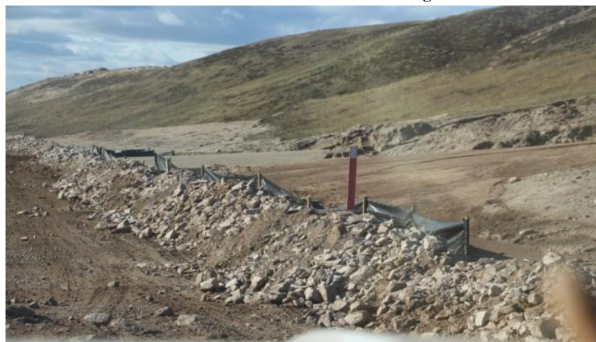
Picture 51: Use of silt fences at embankment failure areas
