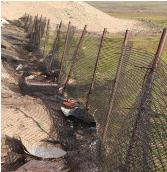
Picture 56: Deteriorated landfill fencing
