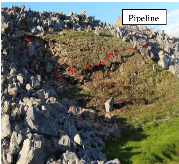
Picture 22: Slope deterioration
