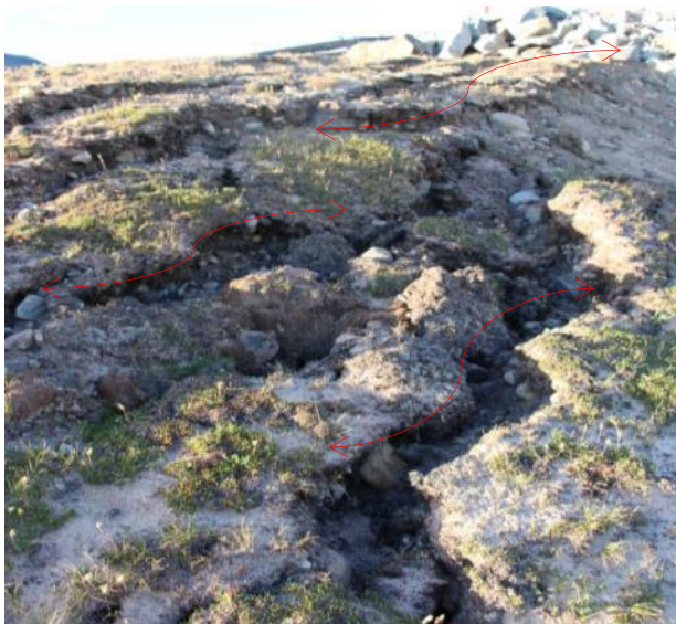
Picture 23: Terrain instability near outfall
