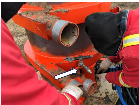
Figure 6: Waste fuel connection valve on incineration chamber
