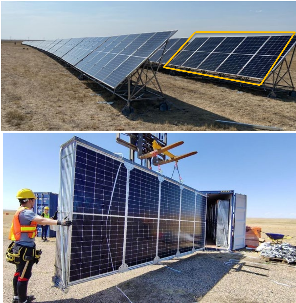
Photo 1: Examples of Solar Panel Array System
