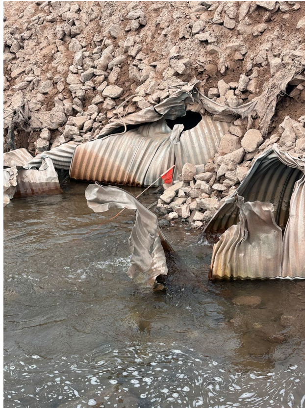
Photo 15 – Damaged culverts behind Sailiivik Camp (June 18 th , 2025).
