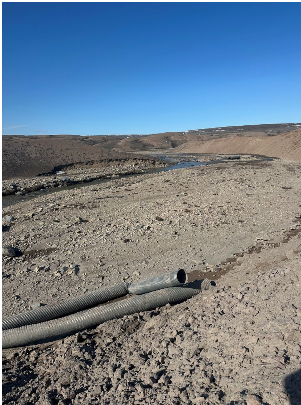
Photo 24 – Culverts still scattered at KM63.5 (June 19 th , 2025).
