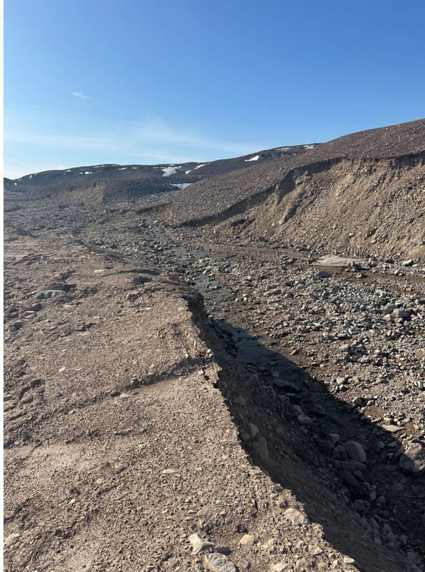
Photo 23 – KM63.5 washout (June 19 th , 2025).
