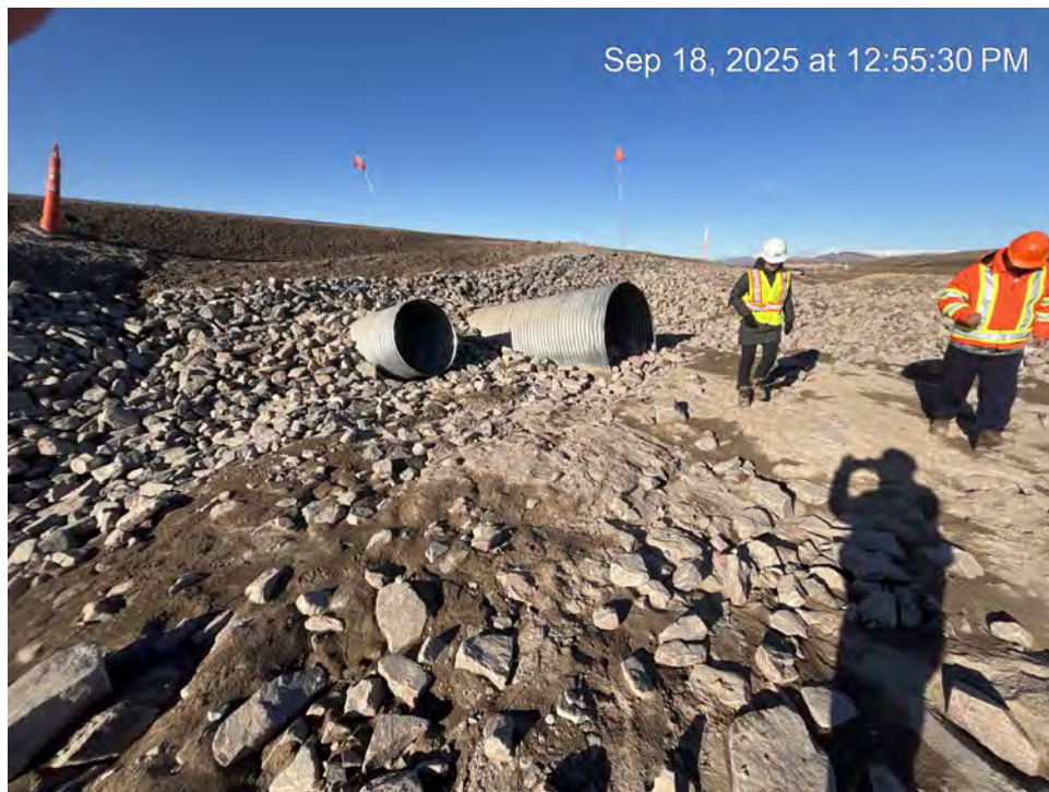
Photo 48 – Blocked culverts at KM33 (September 18, 2025).
