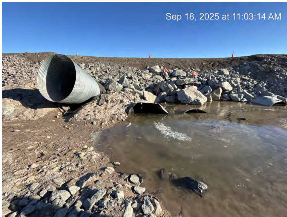
Photo 38 – Compressed culverts at KM216 (September 18, 2025).
