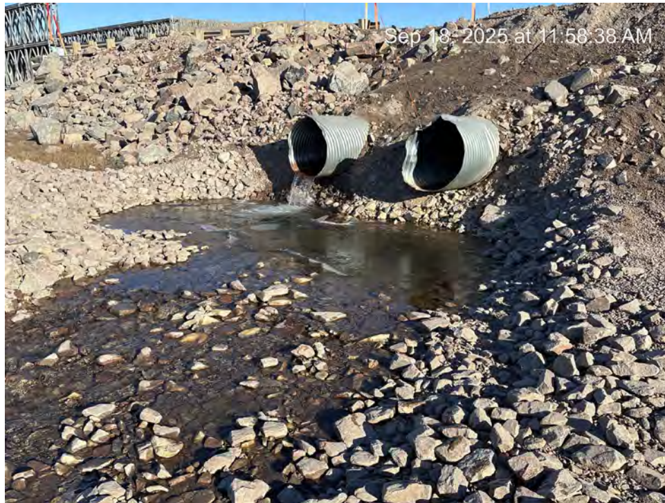
Photo 45 – Perched culverts at KM63 bridge (September 18, 2025).
