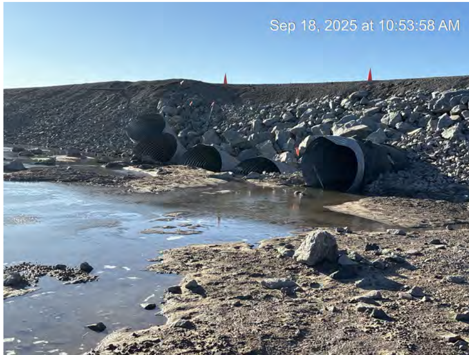
Photo 37 – Compressed culverts at KM216 (September 18, 2025).
