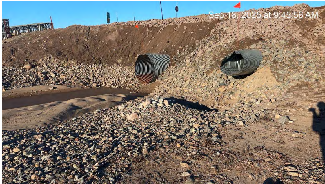
Photo 27 – Perched culverts at KM97 (September 18, 2025).
