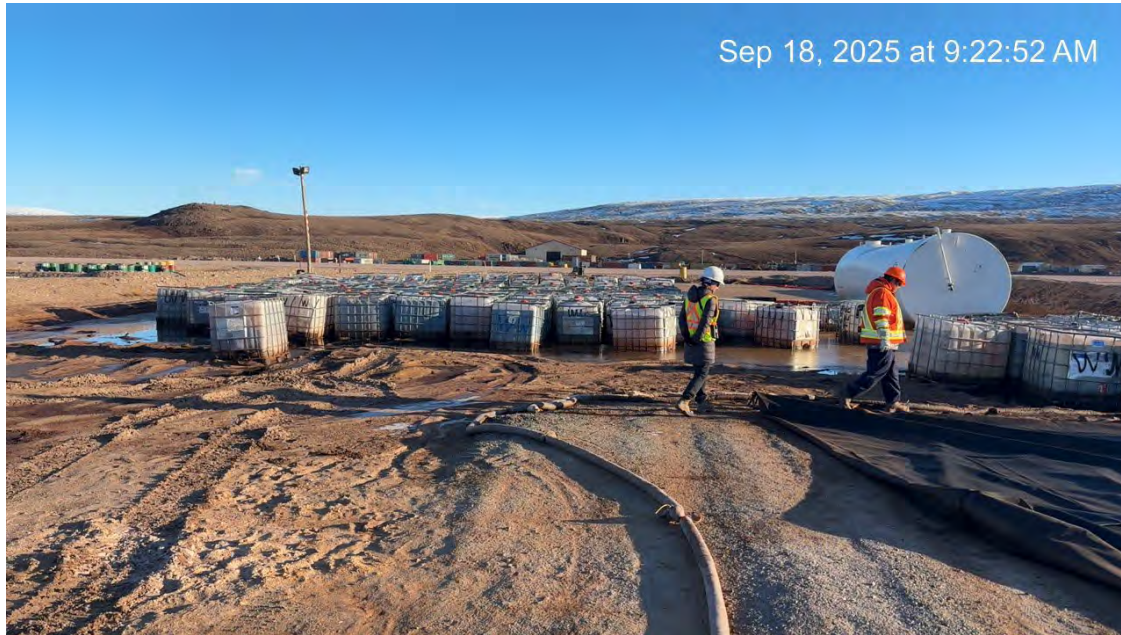
Photo 25 – Labelled totes at Oil Water Separator (September 18, 2025).
