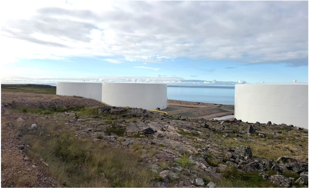
Photo 12: Vertical fuel tanks and surrounding containment berm
