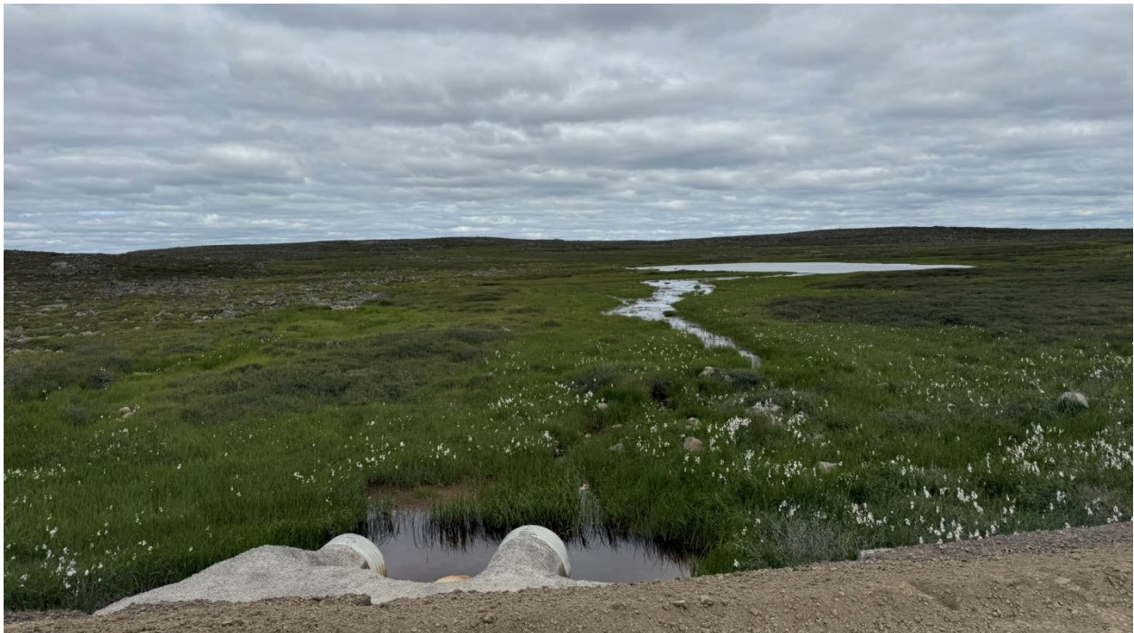
Photo 74: culvert outlets at KM 133, draining through a defined channel across the surrounding wetland toward the downstream waterbody
