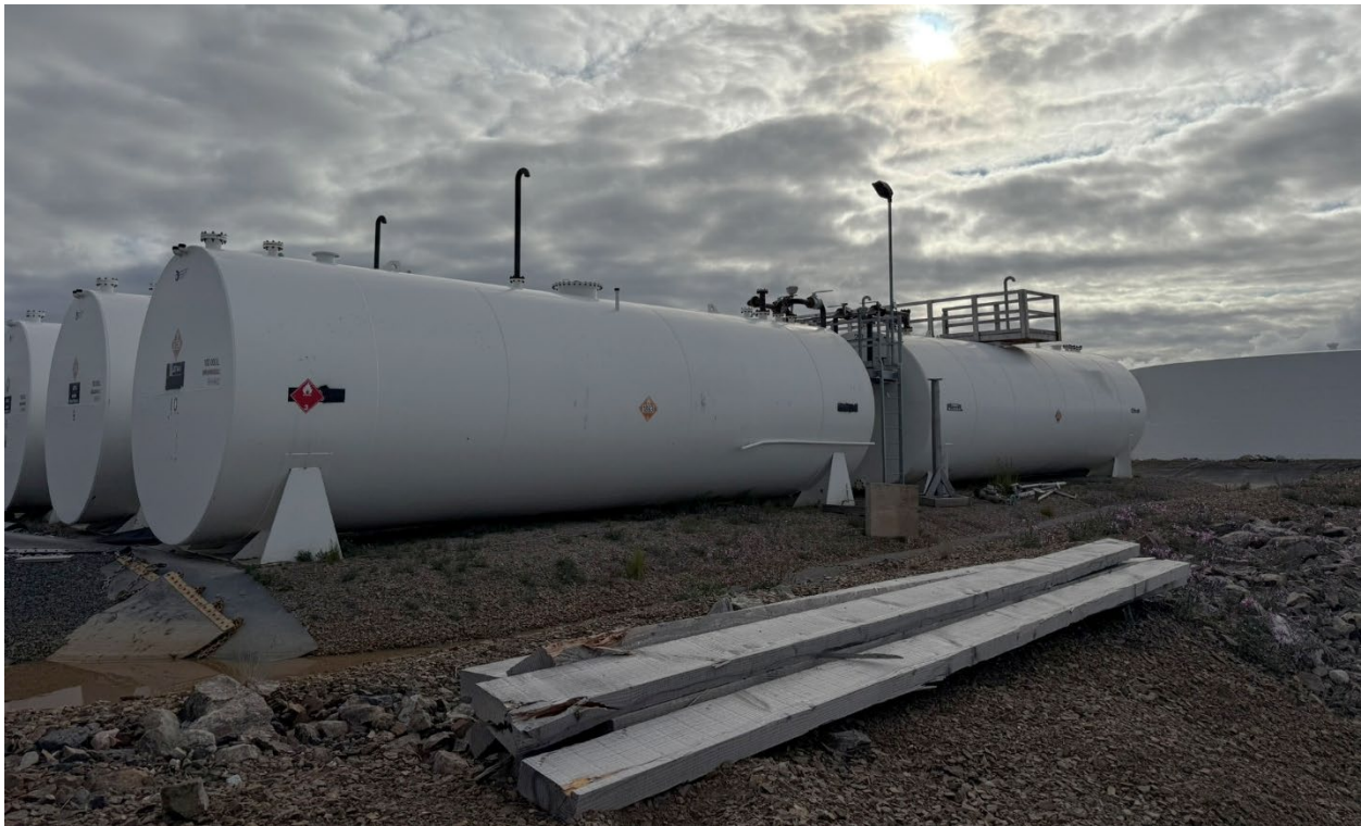
Photo 9: Horizontal fuel tanks in secondary containment
