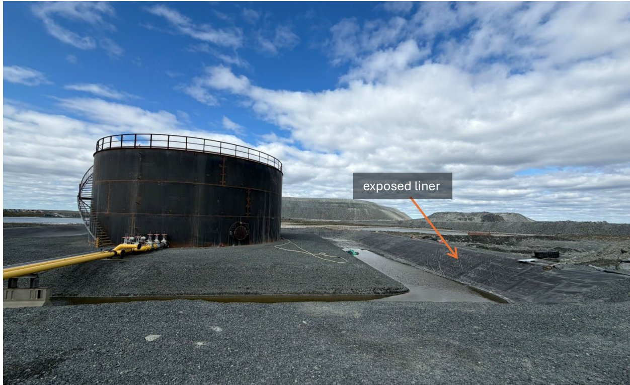
Photo 104: Single-Tank Fuel Farm within secondary containment, with the containment liner exposed
