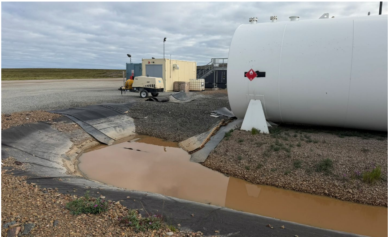
Photo 11: Exposed liner, vegetation growth, and standing water adjacent to horizontal fuel tanks
