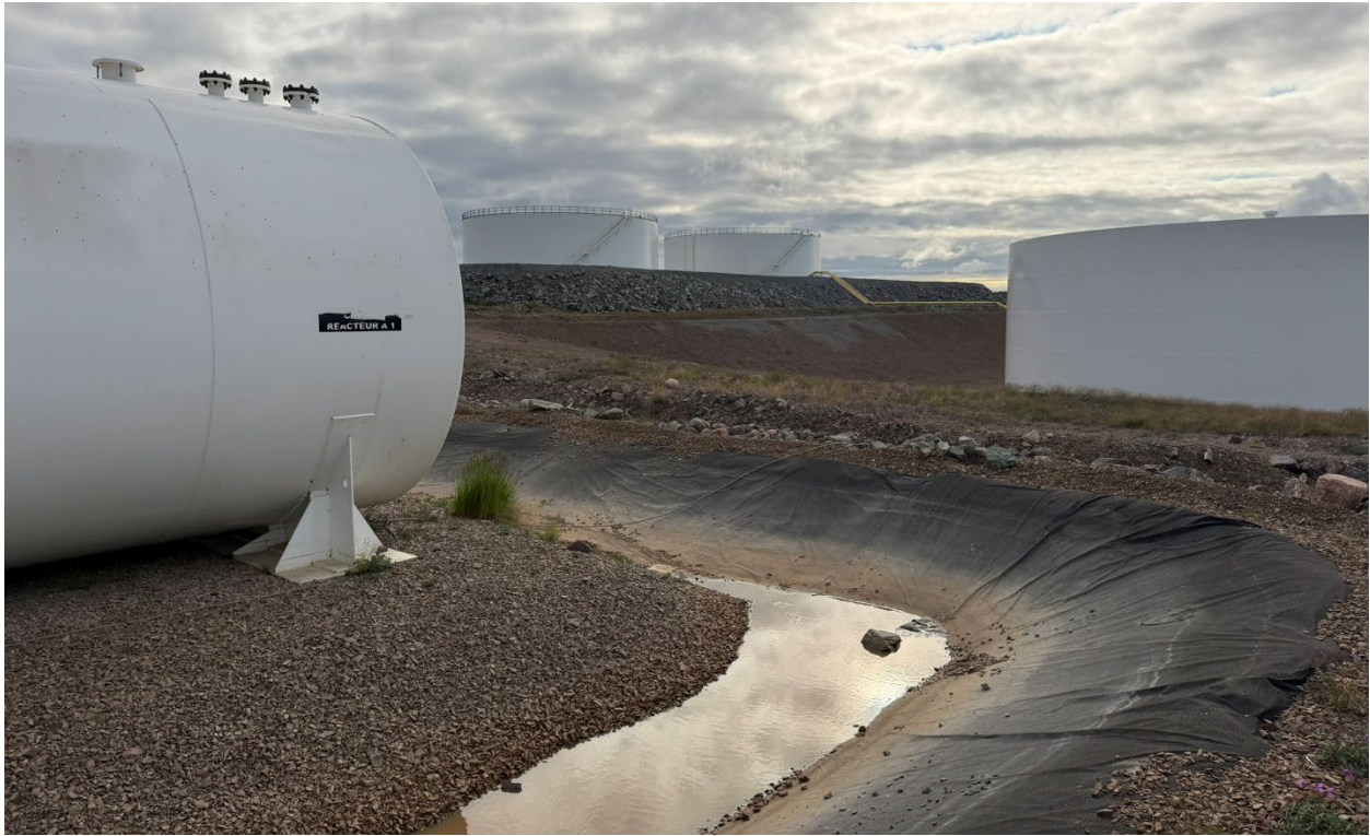
Photo 10: Exposed liner, vegetation growth, and standing water adjacent to horizontal fuel tanks
