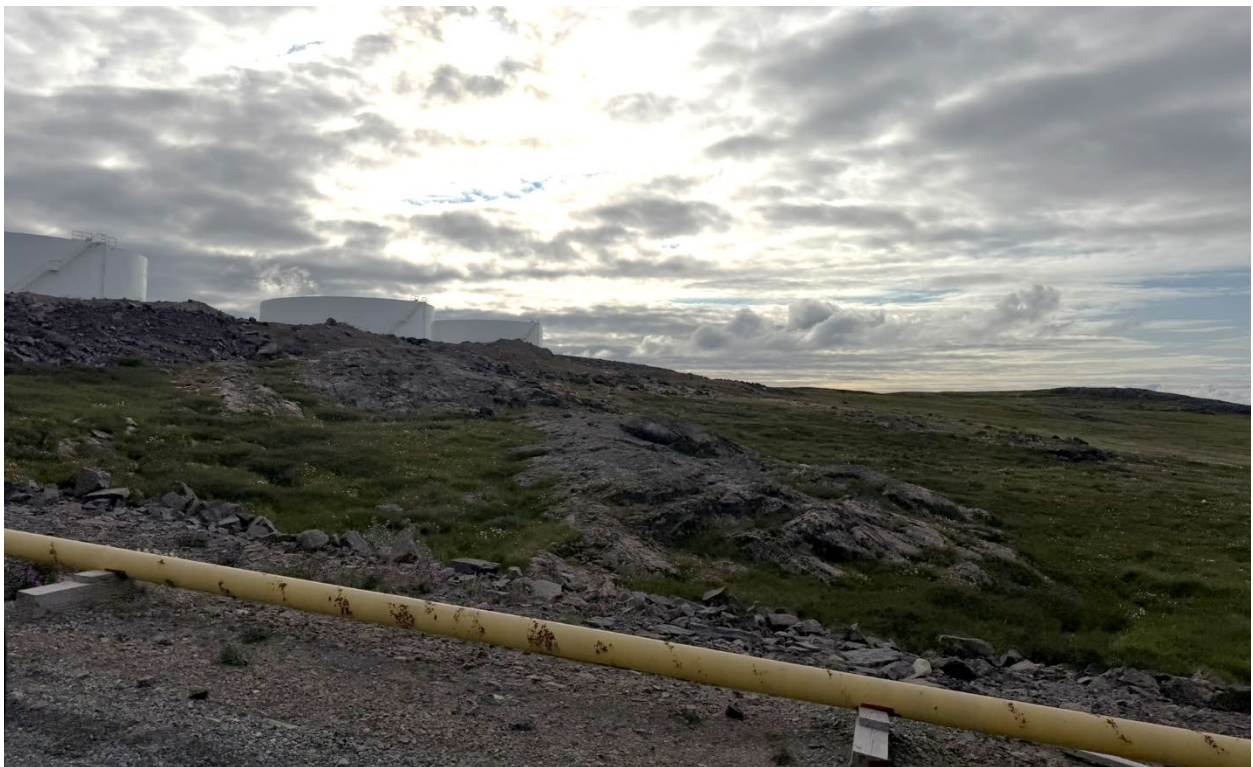
Photo 7: The rigid fuel transfer line running from shore to fuel storage tanks for sealift fuel transfer operations
