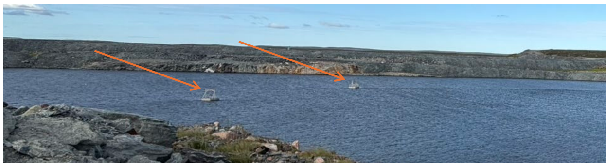
Photo 46: Goose Pit-aerators installed as part of the in-pit semi-passive water treatment system
