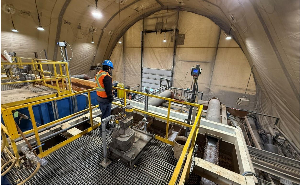
Photo 98: Interior of the Final Water Treatment Plant
