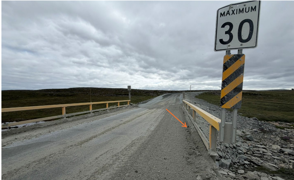
Photo 63: Bridge crossing at WTHR KM 102 with speed limit signage; note fine road material along the road edge and shoulder
