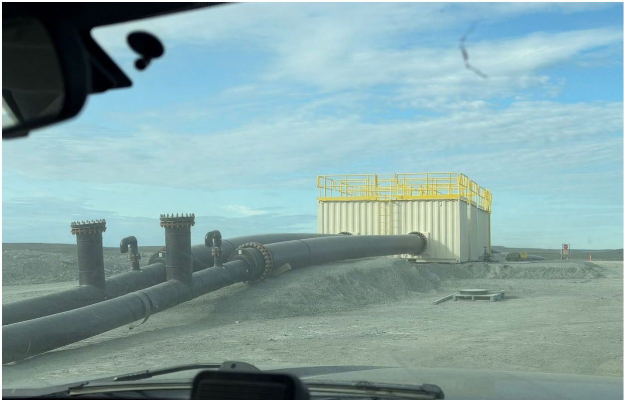
Photo 35: Vault waterline, with pressure relief housing at a high point on the line
