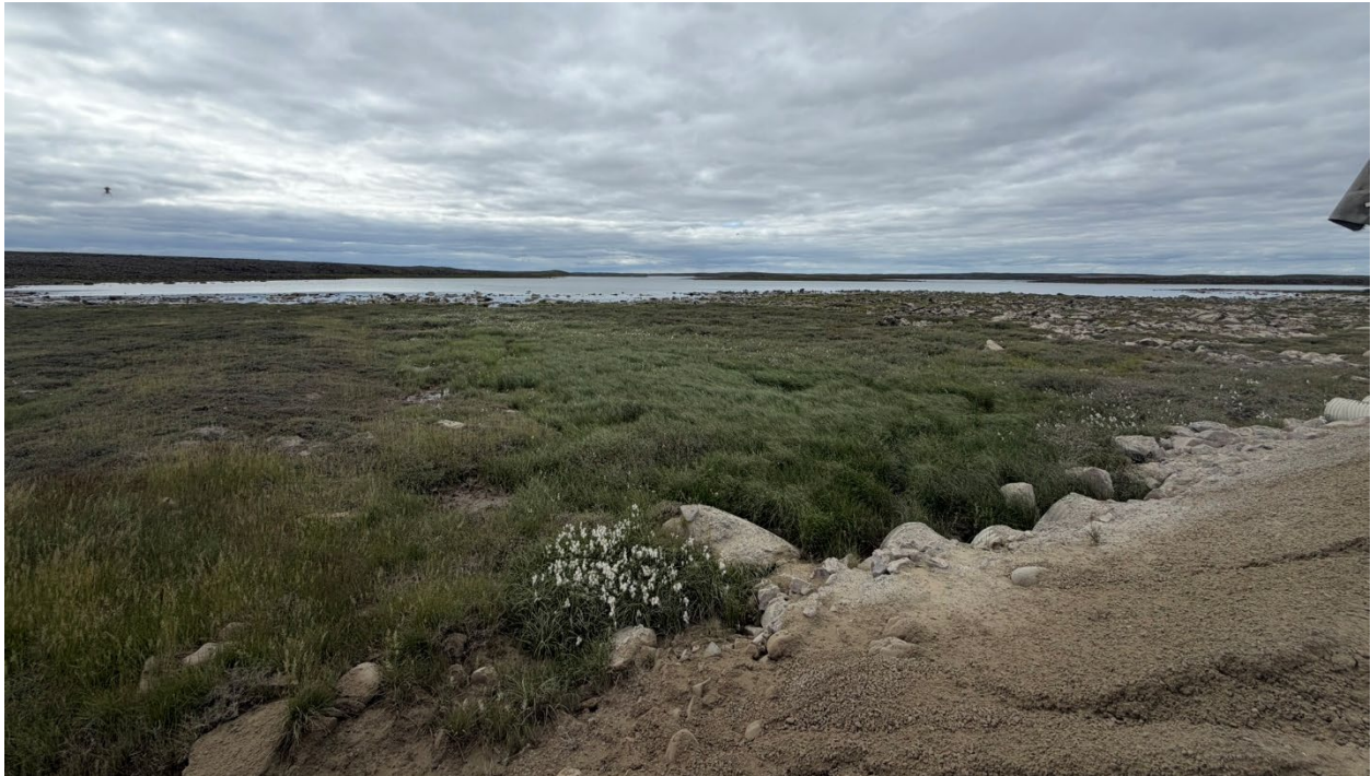
Photo 73: Culvert outlet at KM 133, showing erosion channels on the embankment slope above the outlet, with riprap placed at the toe 11
