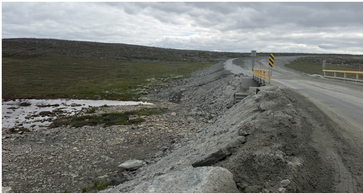
Photo 64: Bridge crossing at WTHR KM 102, showing accumulated road material and debris on the embankment slope above the watercourse 10
