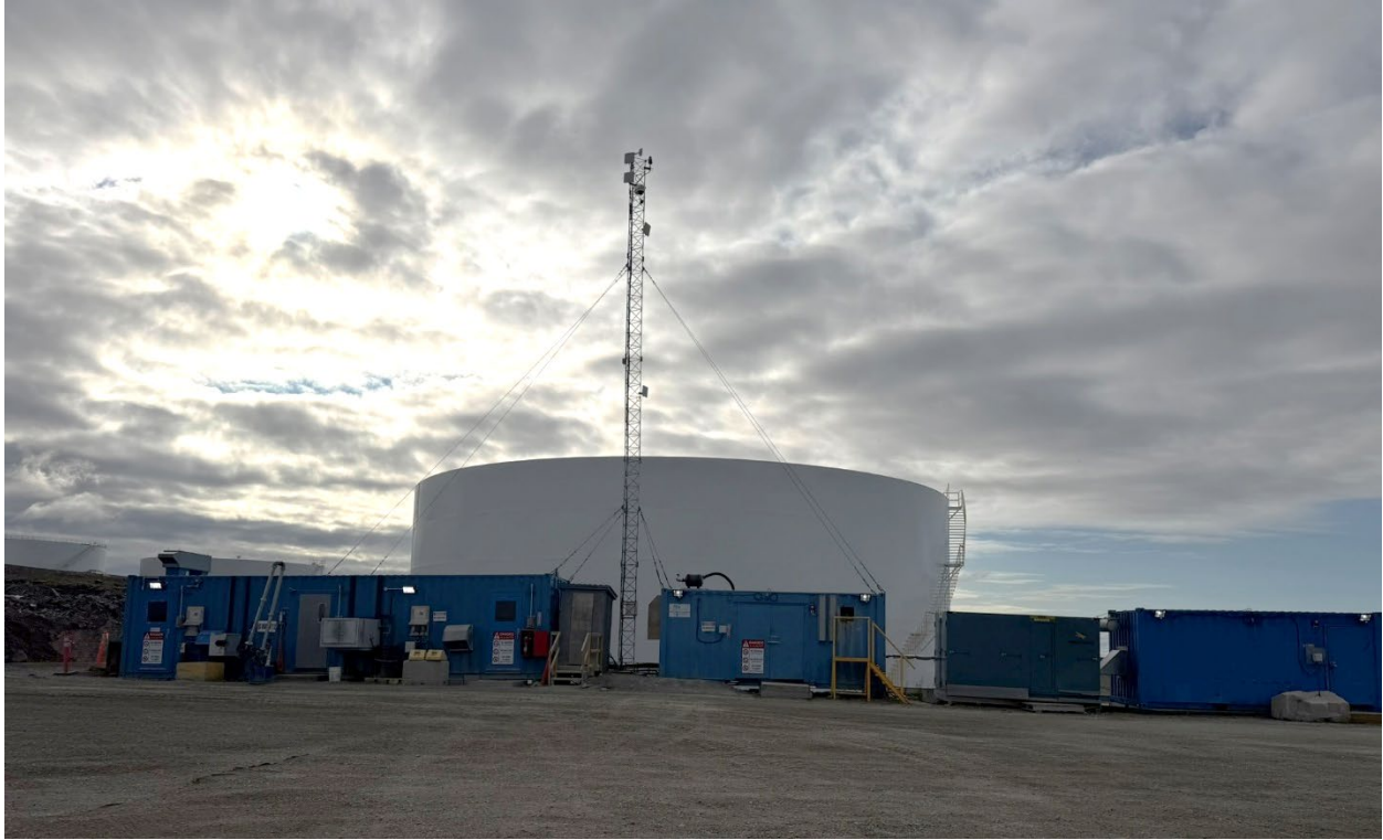
Photo 8: Security cameras and fuel dispensing modules
