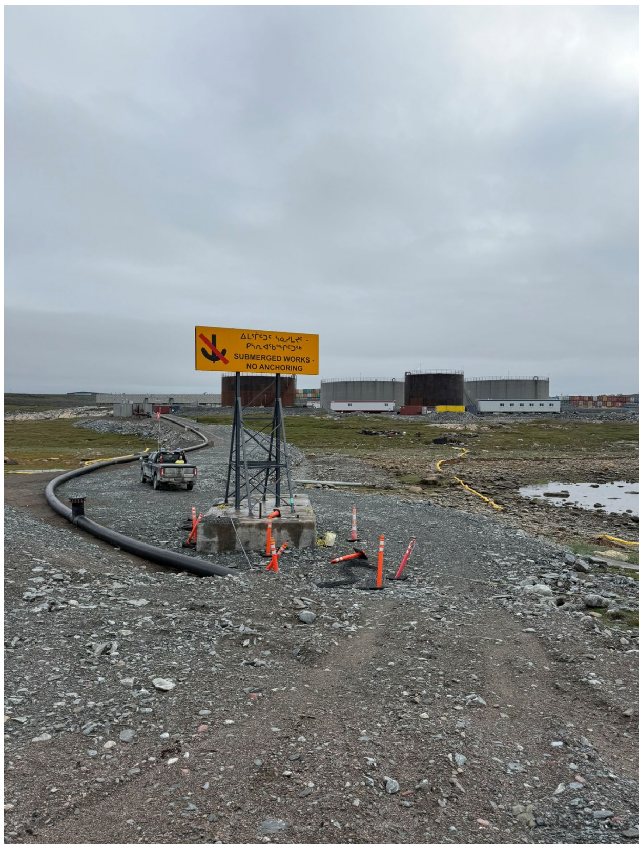
Photo 7: No Anchoring signage and the saline effluent waterline extending toward the offshore diffuser area
