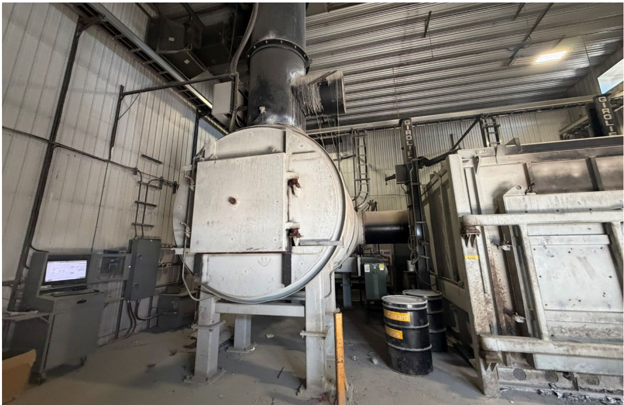
Photo 91: Incinerator housed within Incinerator Building
