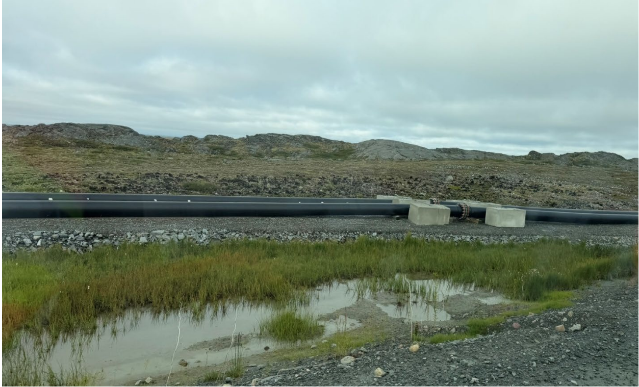
Photo 28: Exposed waterline and concrete anchor blocks at KM 16
