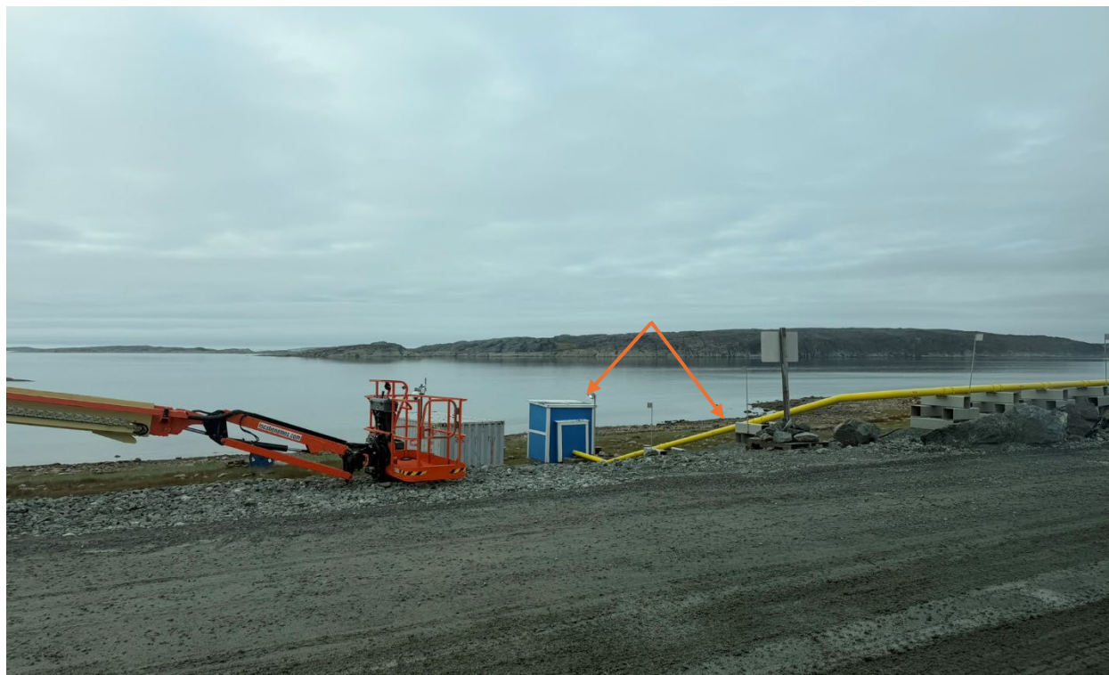
Photo 6: Rigid fuel transfer line and anchor point
