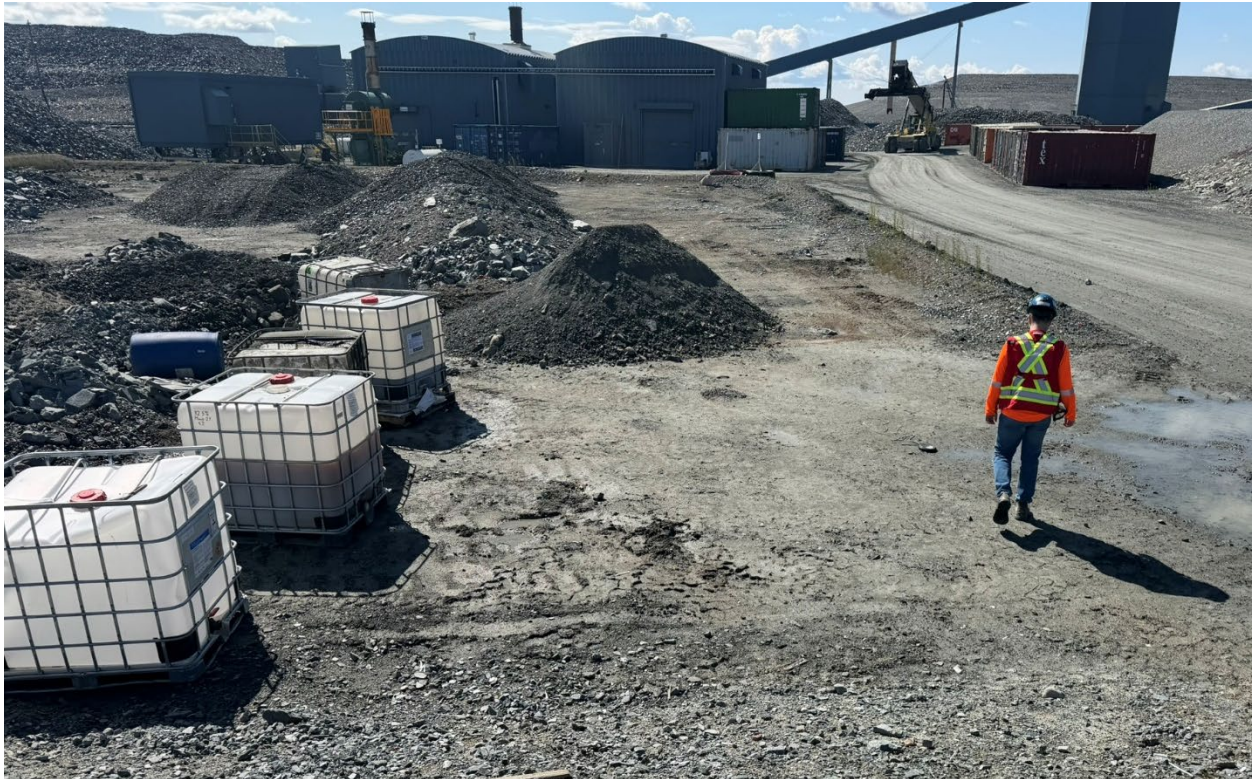
Photo 96: Totes containing hazardous materials staged at landfarm cells
