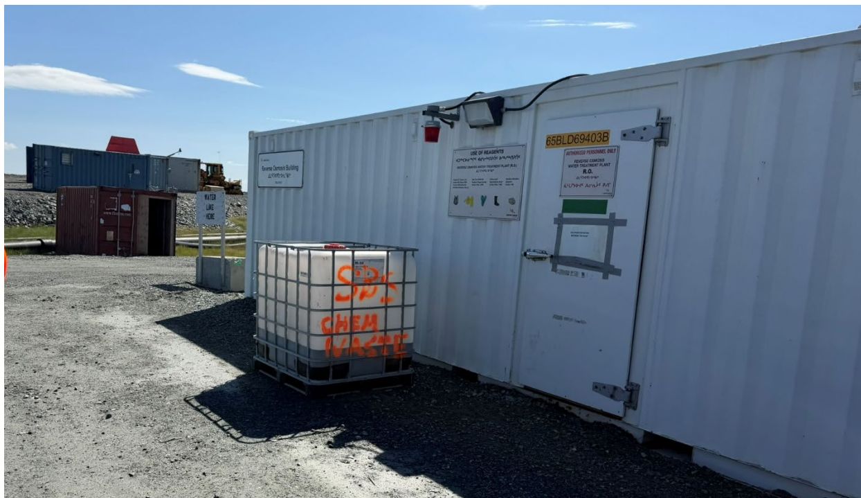
Photo 74: Reverse Osmosis (RO) Plant 9 , with chemical waste tote noted stored outside of secondary containment
