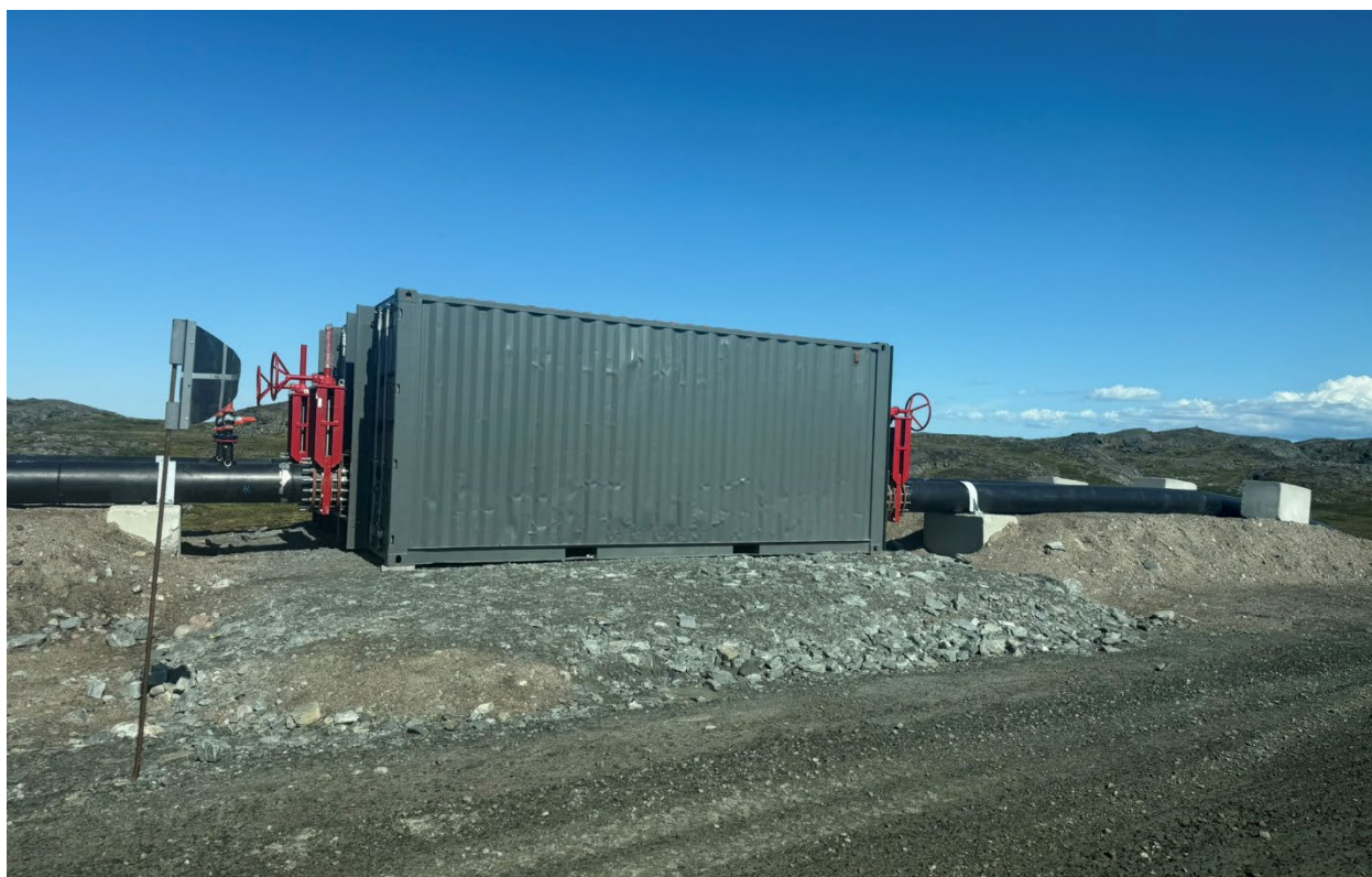
Photo 27: One of multiple seacans containing pressure relief valves and exposed waterlines along the corridor
