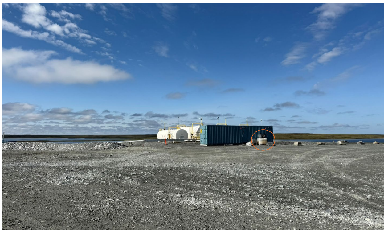
Photo 42: Manual fuel station near the West Vent Raise, with the DEF storage tank located outside secondary containment
