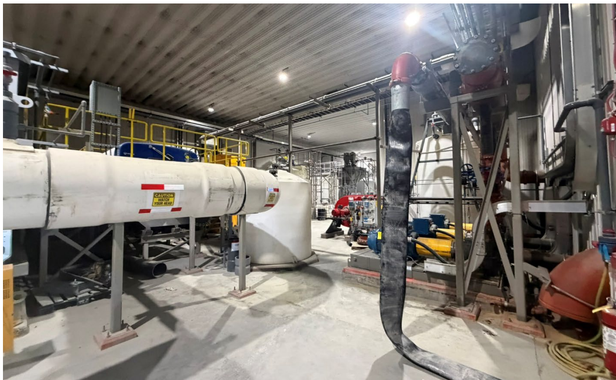
Photo 80: Water Treatment Complex - Saline Effluent Treatment Plant (WTC-SETP)
