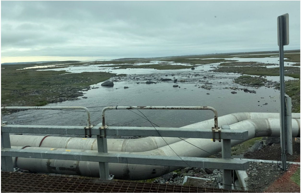
Photo 22: Waterlines attached to the Meliadine River bridge crossing
