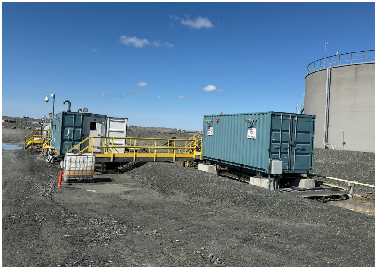
Photo 86: 3M Pumping Station, with the DEF storage tank located outside secondary containment
