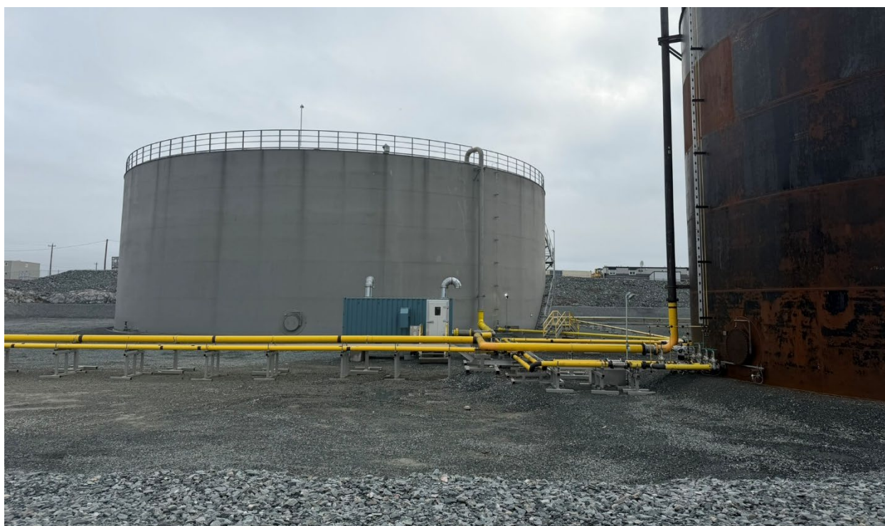
Photo 4: Fuel Tank Farm in secondary containment at Itivia 1
