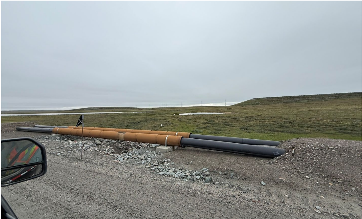
Photo 16: Exposed waterline section at KM 3 with no signage present
