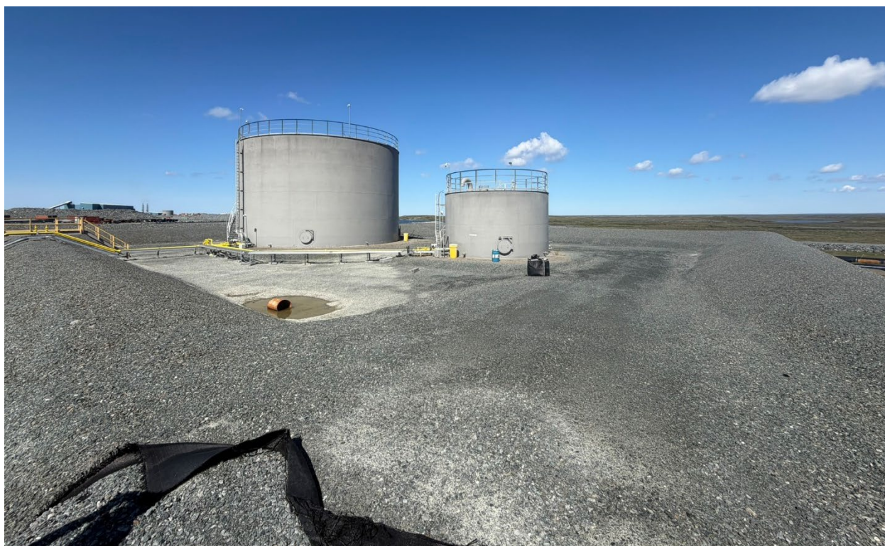
Photo 85: Fuel tanks at onsite 3M Fuel Tank Farm in secondary containment; noted exposed liner
