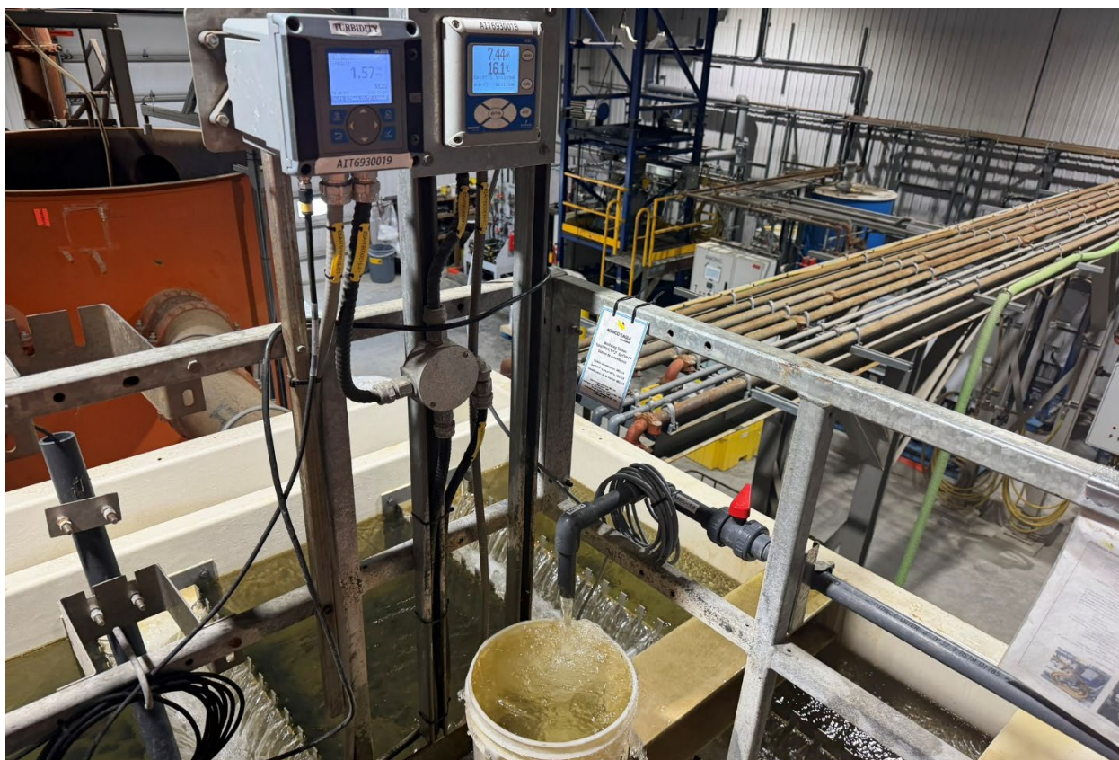
Photo 81: Water Treatment Complex - Effluent Water Treatment Plant (WTC-EWTP)
