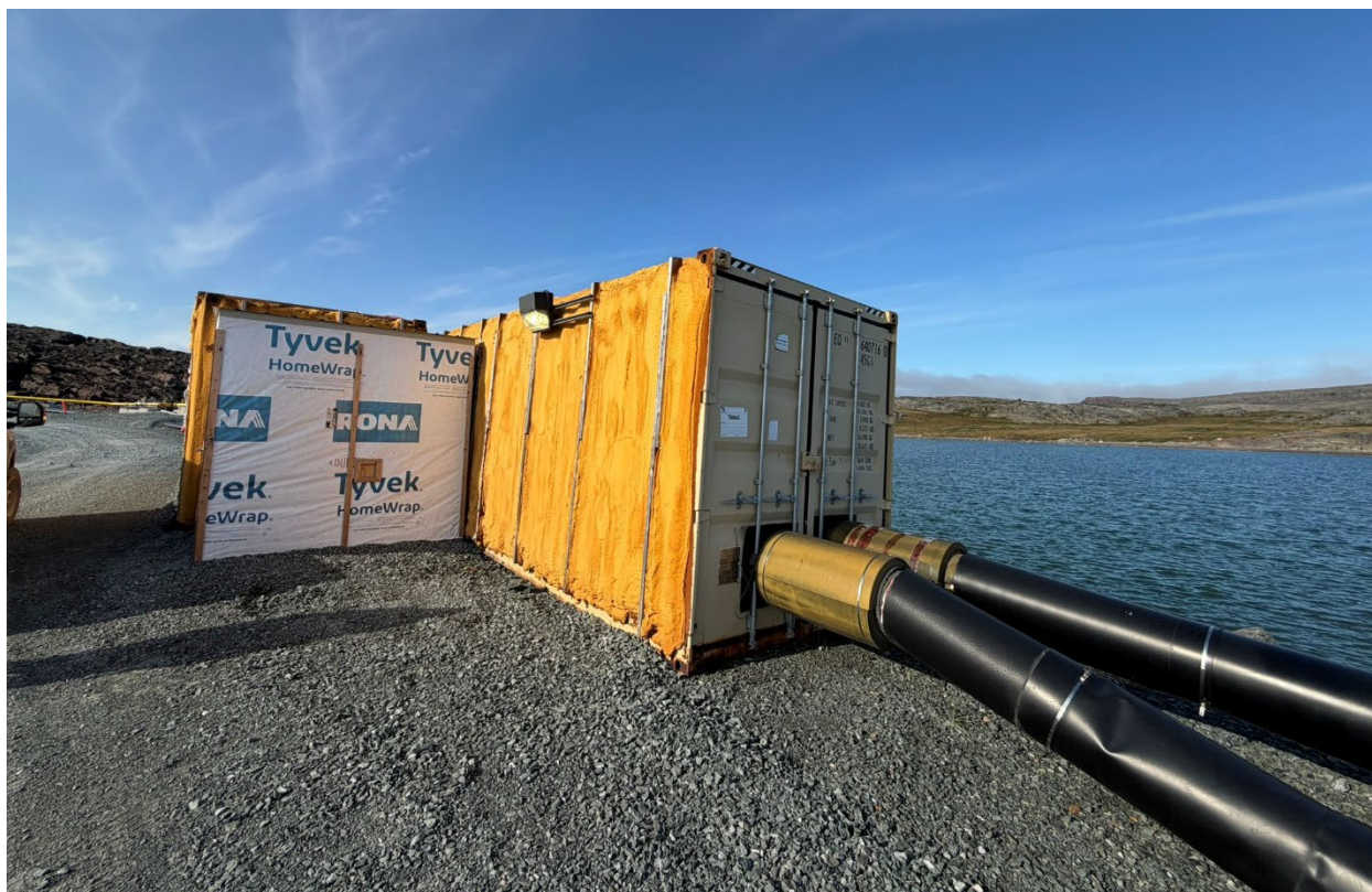
Photo 4: Treated effluent discharge pumphouse
