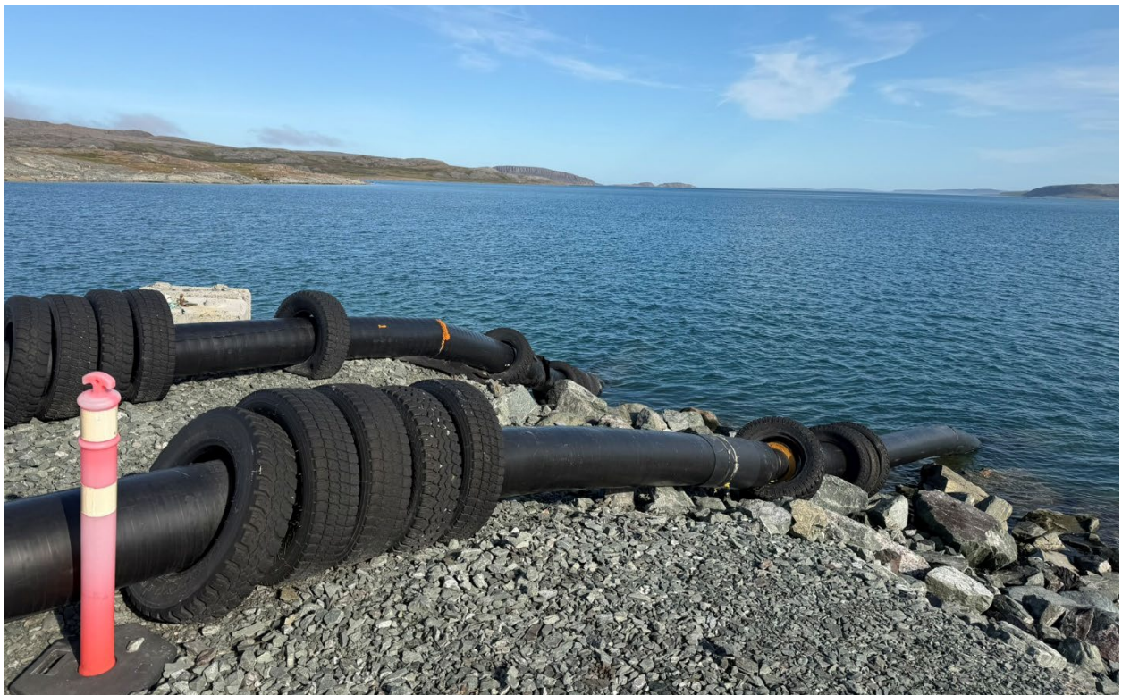
Photo 6: Entry point of the treated effluent discharge pipeline leading to the offshore diffuser
