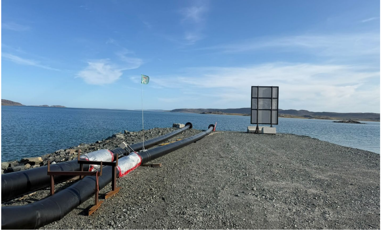
Photo 5: Treated effluent discharge pipeline
