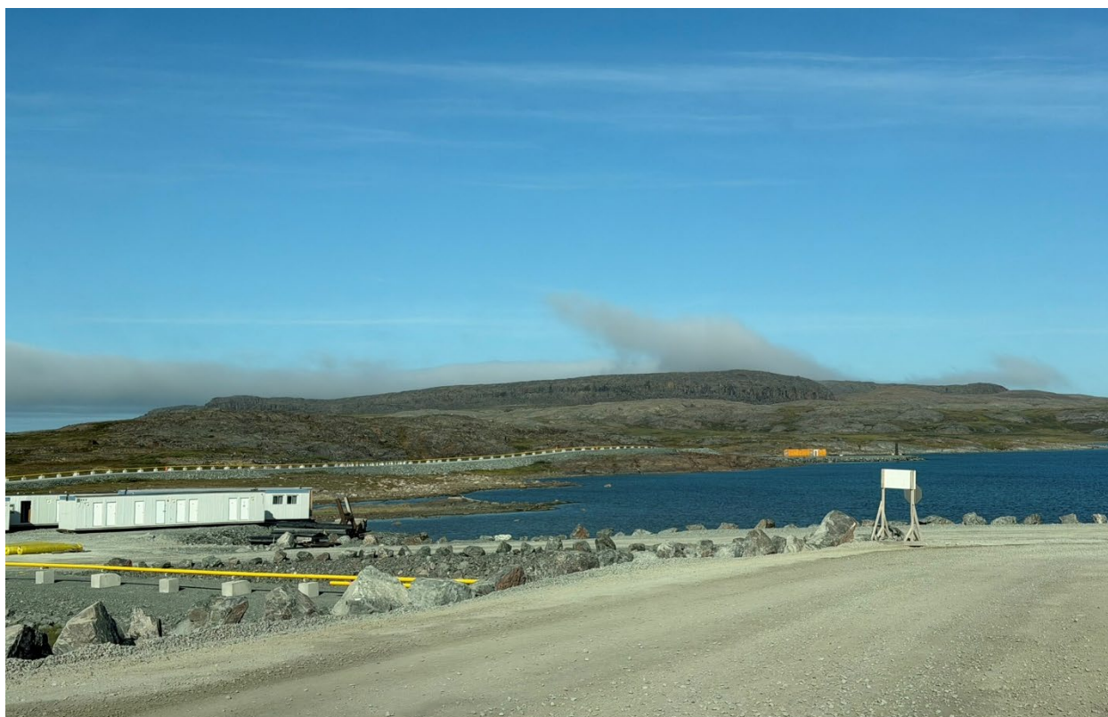
Photo 16: Rigid fuel line extending from the shoreline anchor point to the future tank farm area at Quarry AF
