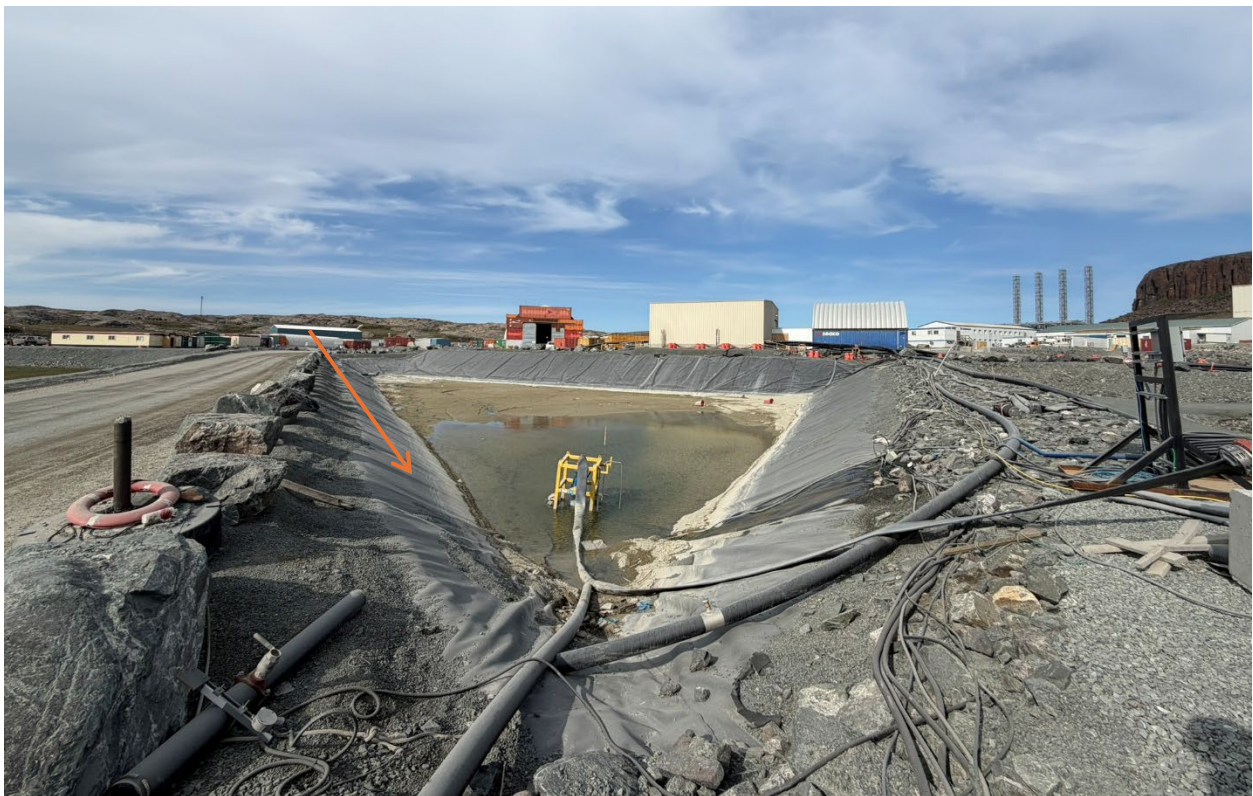
Photo 36: Sedimentation Pond, exposed liner noted
