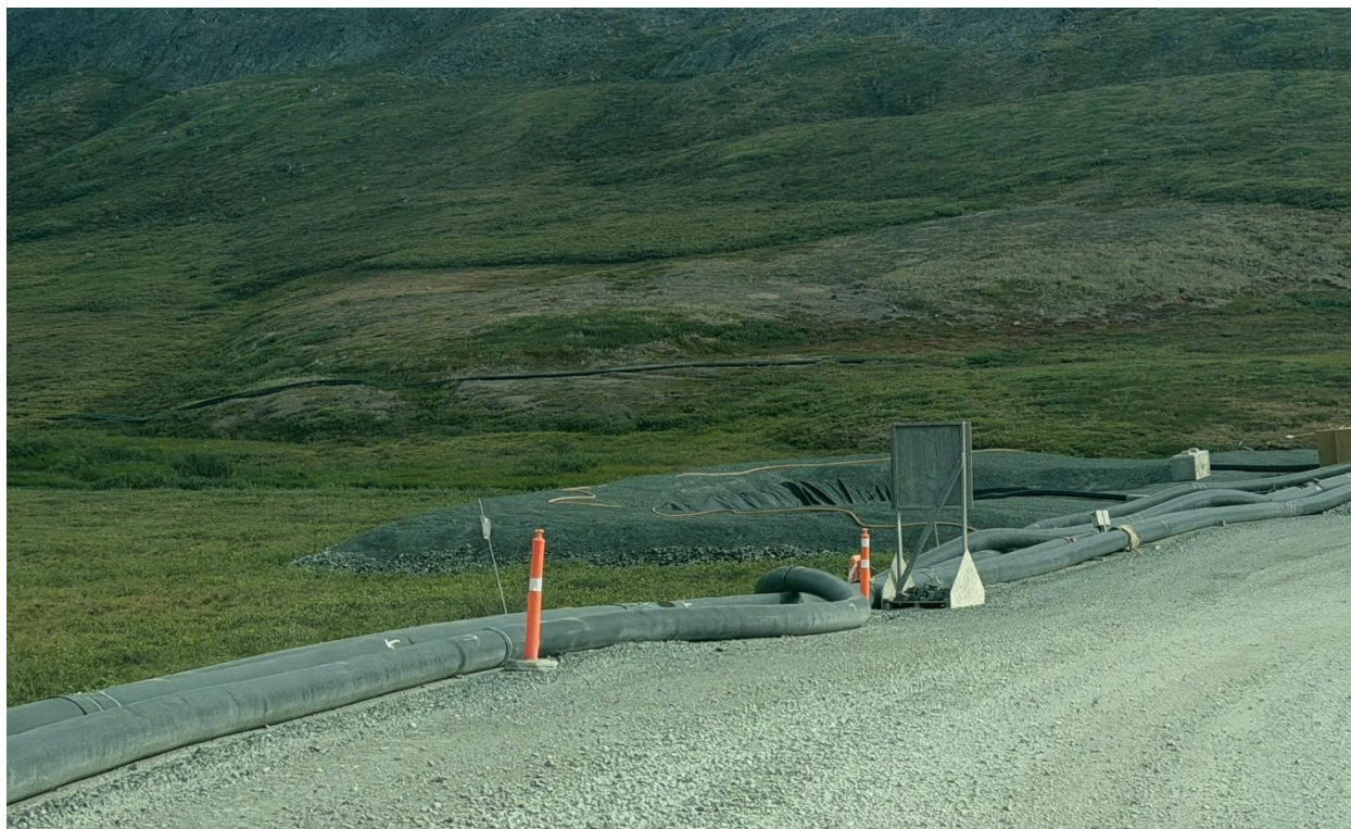
Photo 54: Catch Basin 1 - one of two catch basins located on opposite sides of Doris Creek Bridge for emergency discharge
