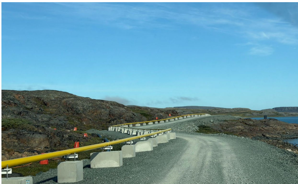
Photo 8: Rigid fuel pipeline connecting the shoreline fuel receiving anchor point to the fuel tank farms
