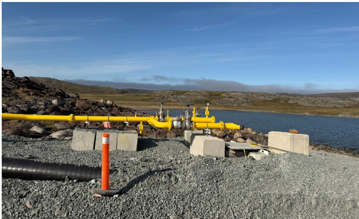
Photo 7: Shoreline rigid fuel line anchor point for receiving fuel deliveries via barges
