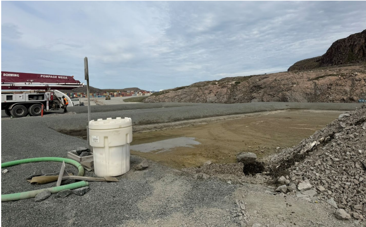
Photo 31: Landfarm cells adjacent to Quarry 2
